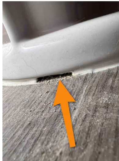
Sealant Gaps – Detail
