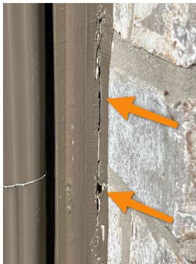
Sealant Gaps – Detail
