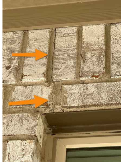
Minor Brick Crack – Detail
