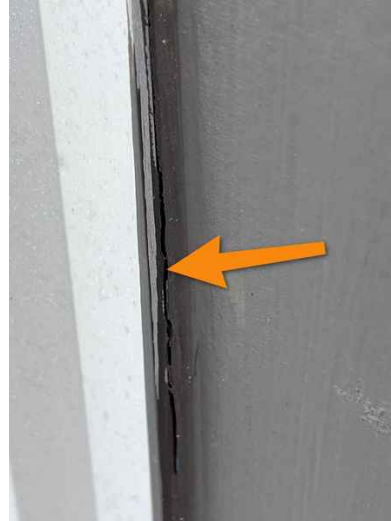
Sealant Gaps – Detail
