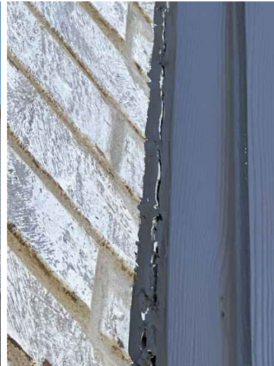
Sealant Gaps – Detail
