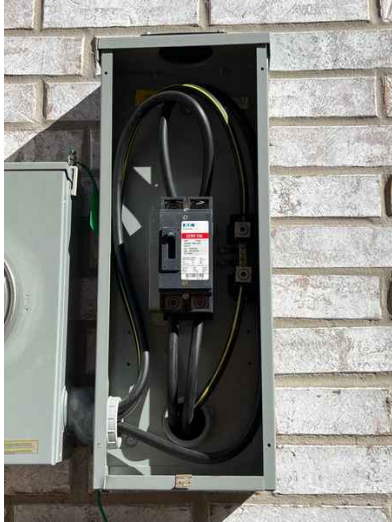
Main Panel Interior
