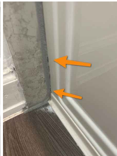
Sealant Gaps – Detail
