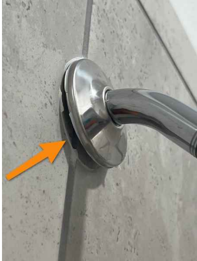
Sealant Gaps – Detail
