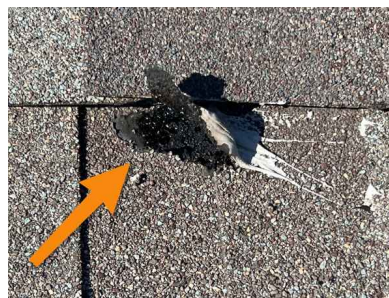
Sealant Peeling – Detail
