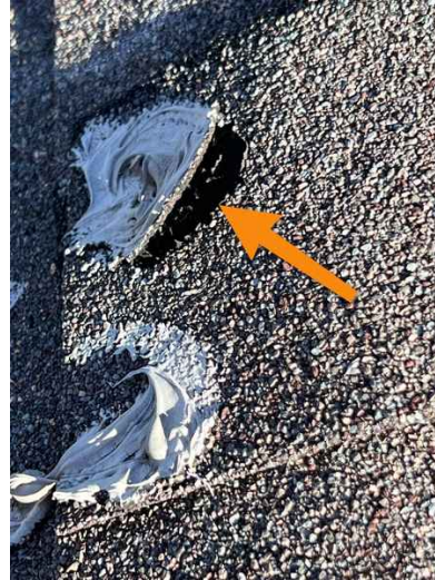
Sealant Peeling – Detail
