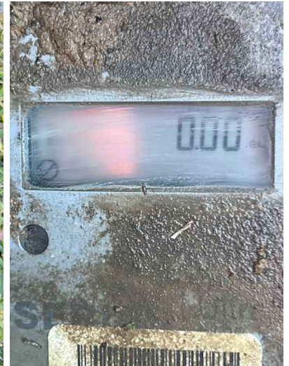
Water Meter Flow Rate
