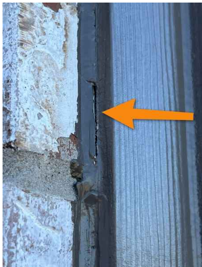
Sealant Gaps – Detail
