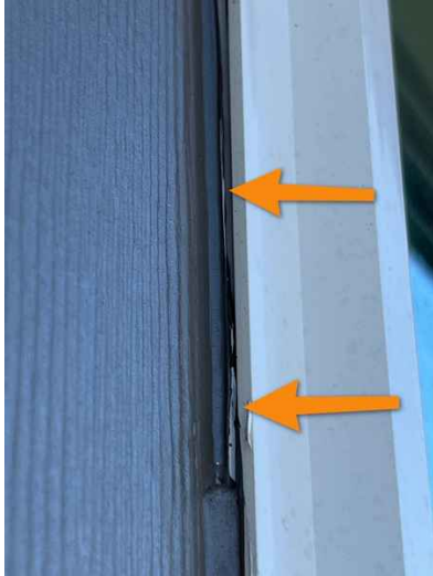
Sealant Gaps – Detail
