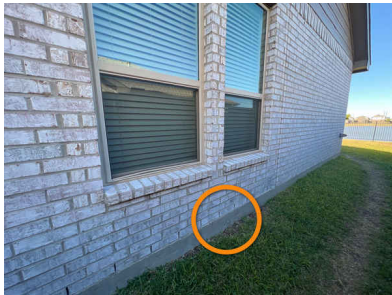
Exposed Cable End
