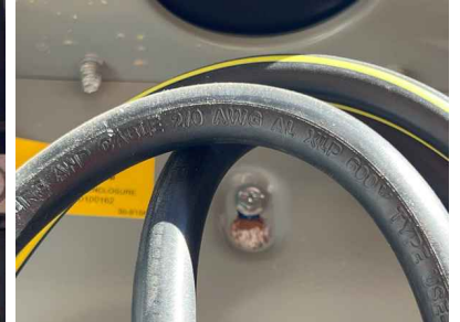
2/0 AWG Aluminum Service Entrance Conductors
