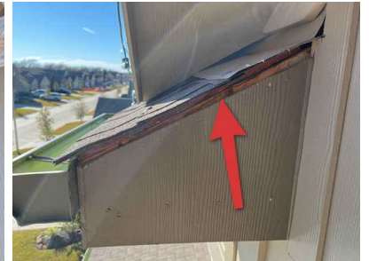
Gap in Siding – Detail
