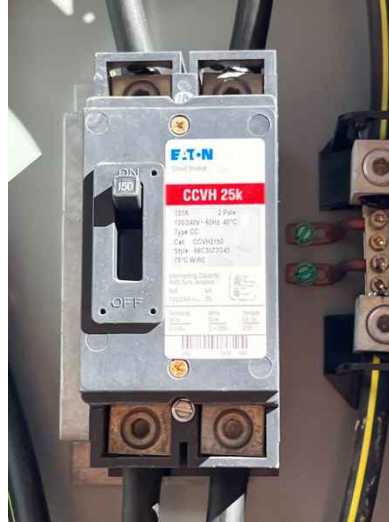
150 amp main breaker
