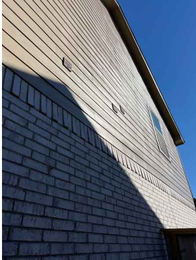
Sealant Gap Around Vent Penetration
