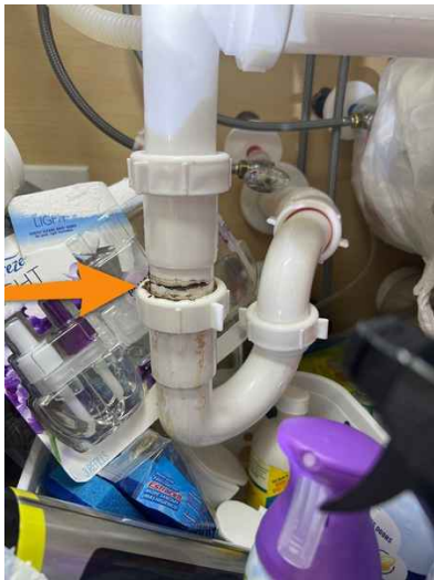
Loose Drain Connection
