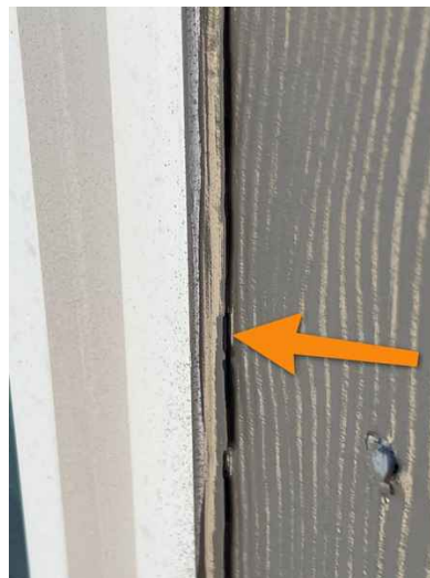
Sealant Gaps – Detail
