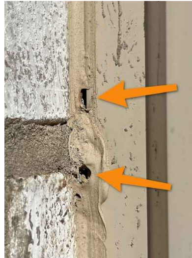
Sealant Gaps – Detail
