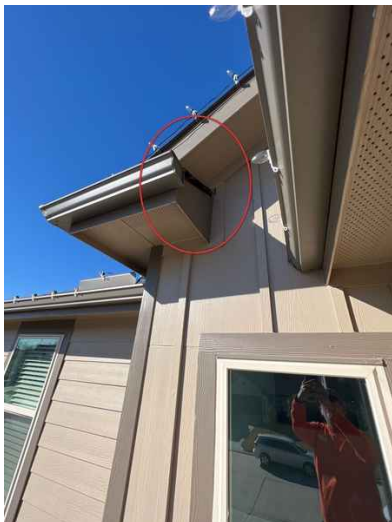
Missing Drip Edge Flashing Location
