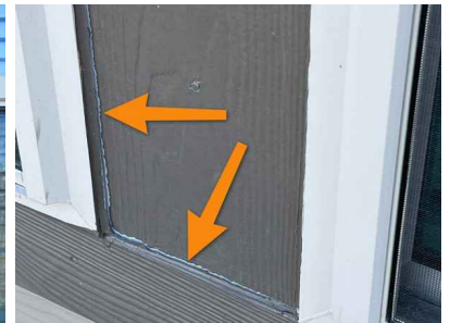
Loose Trim – Detail
