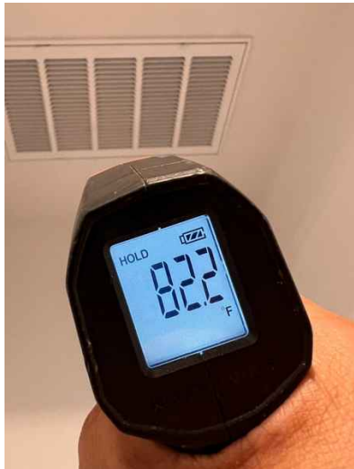
Temperature at Return Downstairs
