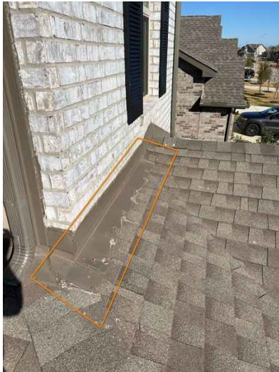
Flashing Lifting Location
