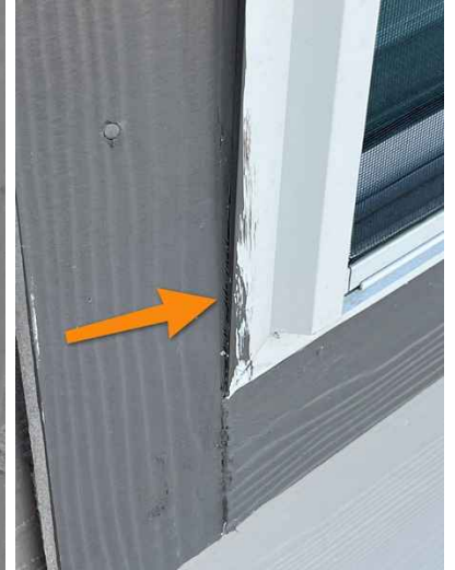
Sealant Gaps – Detail
