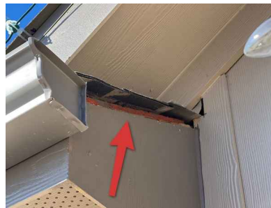
Missing Drip Edge Flashing – Detail
