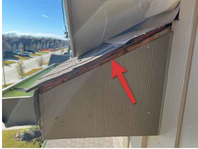
Missing Drip Edge Flashing (Alt Angle)
