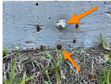
Exposed Cable End – Detail
