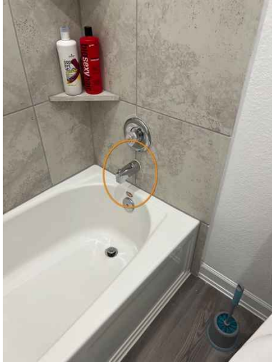
Spout Sealant Gap
