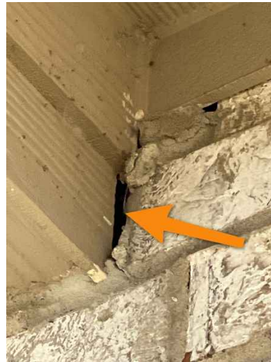
Sealant Gaps – Detail
