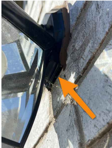
Sealant Gaps – Detail
