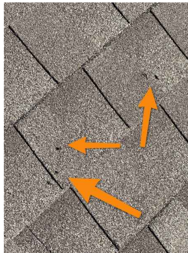
Nail Holes – Detail
