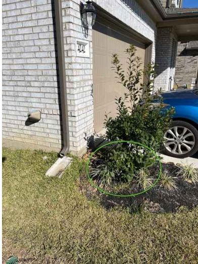
Main Cleanout Location
