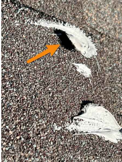
Sealant Peeling – Detail
