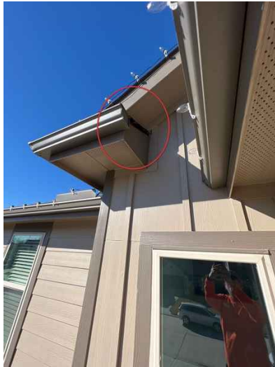
Gap in Siding
