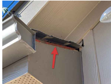
Gap in Siding – Detail
