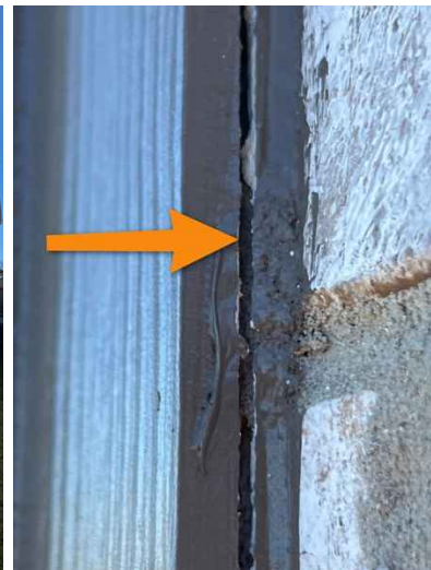
Sealant Gaps – Detail
