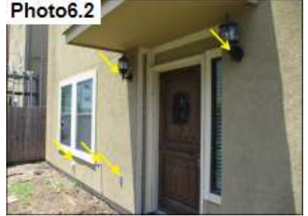
Penetration Sealants / Seal
