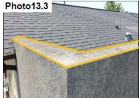
Missing Metal Cap / Install
