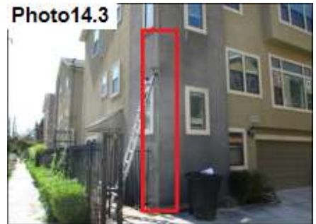
Substrate Damage / Assess & Repair
