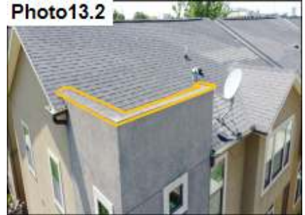
Missing Metal Cap / Install
