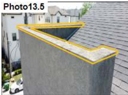
Missing Metal Cap / Install
