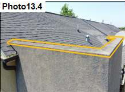
Missing Metal Cap / Install
