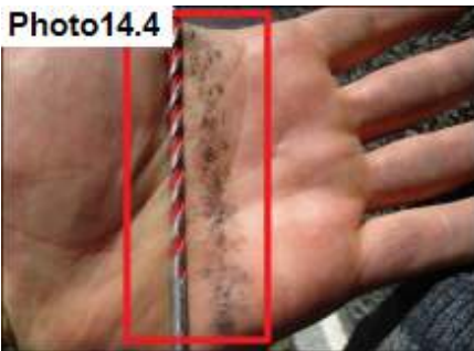
Substrate Damage / Assess & Repair
