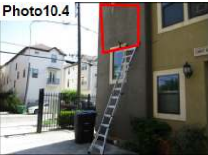
Substrate Damage / Assess & Repair
