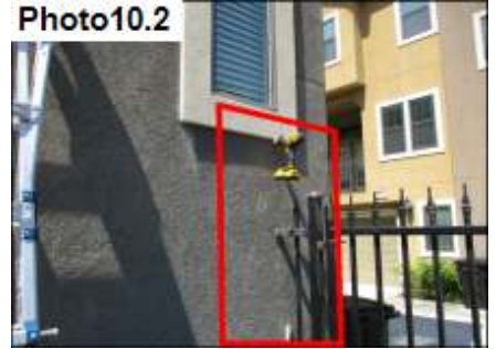
Substrate Damage / Assess & Repair
