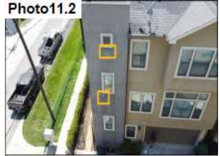
Efflorescence / Clean as Needed
