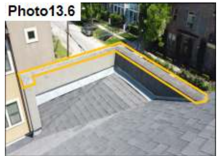
Missing Metal Cap / Install
