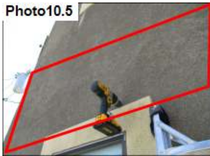
Substrate Damage / Assess & Repair
