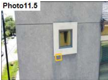
Efflorescence / Clean as Needed
