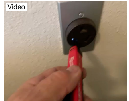
Laundry room: power confirmed at dryer outlet
