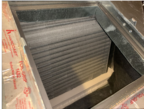
Unit 2 Evaporator coils
