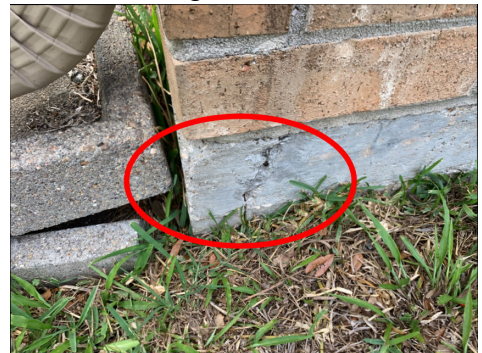
Rear Left: Corner crack
