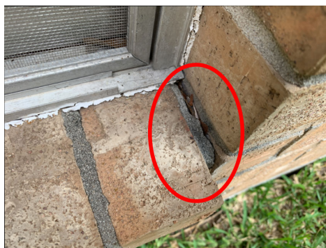
Left: Deteriorated mortar
