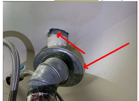
Loose fire stop
