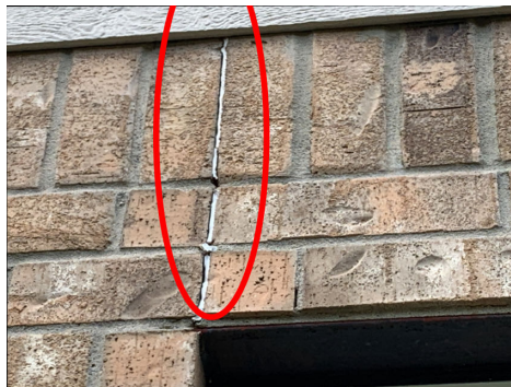
Left: Caulk deteriorated at expansion joint
