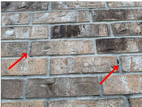
Left: Deteriorated mortar
