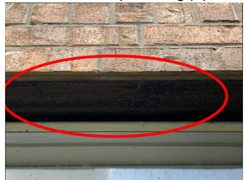
Rear: Rust on lintels
