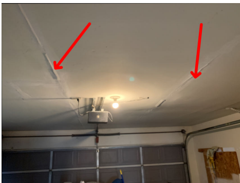
Garage: Hairline crack
