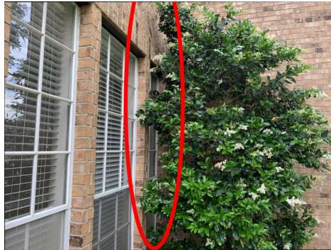
Front: Foliage close to structure
