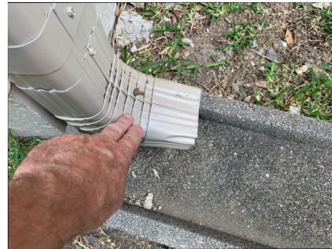
Downspout extension missing
