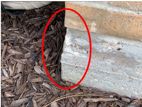
Front: Corner crack
