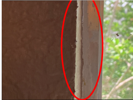
Bathroom 2: Deteriorated caulk
