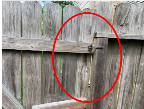
Unable to operate the gate
