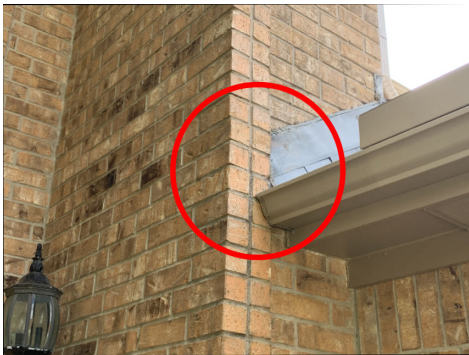
Front: Missing kickout flashing
