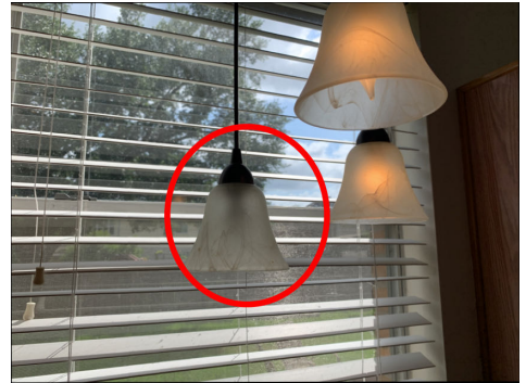
Kitchen: inoperative light fixture
