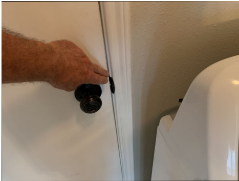
Garage Man Door: Would not latch
