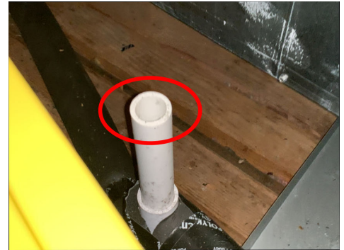
Unit 2 Cap missing on primary condensate drain line cleanout
