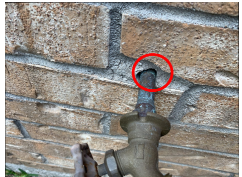
Left: Hole at plumbing pipe
