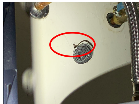
Garage: Hole in firewall separation
