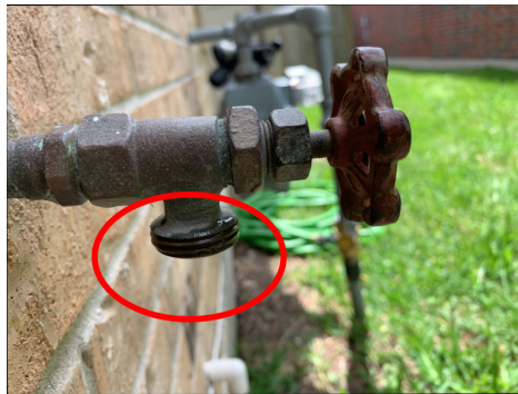
Around house: Back flow preventer recommended
