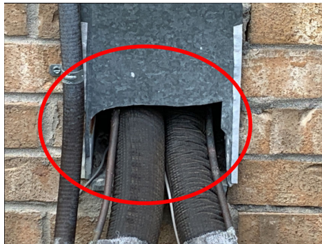
Left: Hole in wall at AC lines
