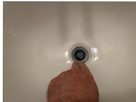
Half Bathroom: Inoperable stopper
