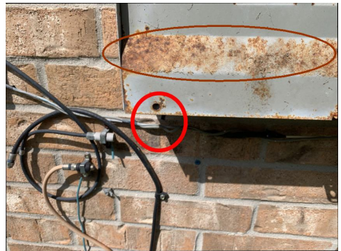
Screw missing and rust on dead front
