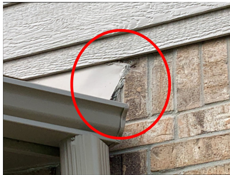
Rear: Missing kickout flashing
