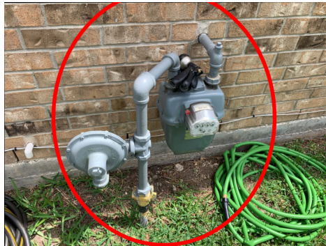
Right: Gas meter
