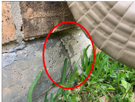
Front: Left: Corner crack
