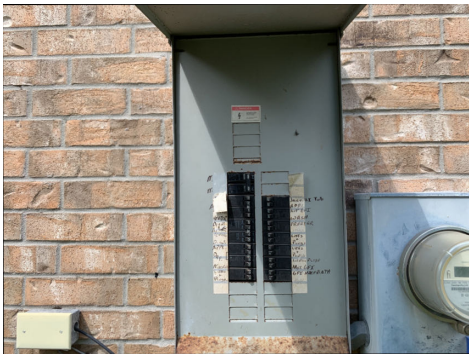
Rear: Service Panel
