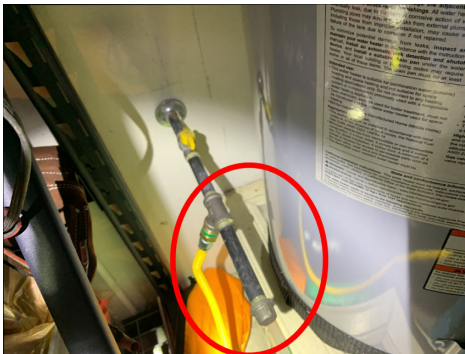
Improper drip leg installation
