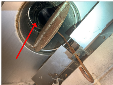
Damper locked open
