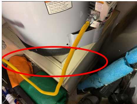
Missing drip pan
