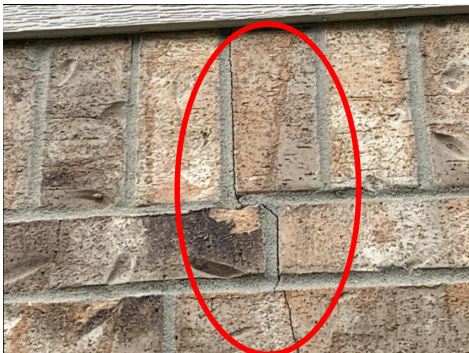
Rear: Step crack
