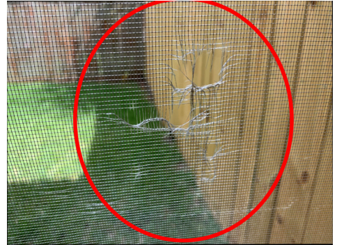
Dining Room: Damaged screen
