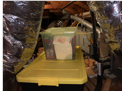
FYI: Owner's belongings obstructing path to HVAC equipment
