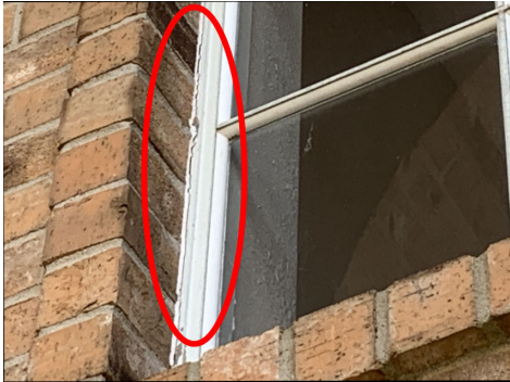
Front: Deteriorated caulk
