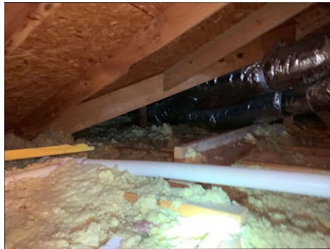
Insulation improvement needed
