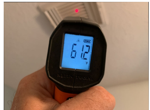
2nd floor: vent temperature
