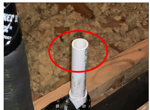
Unit 1 Cap missing on primary condensate drain line cleanout
