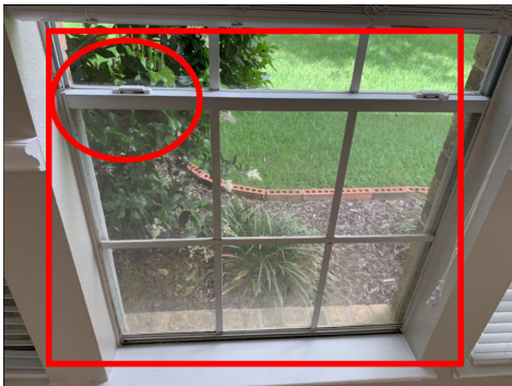
Front Room: Inoperative window / faulty latch
