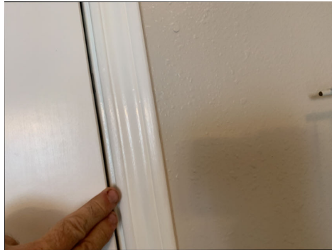
Garage man door: Rubbed on frame
