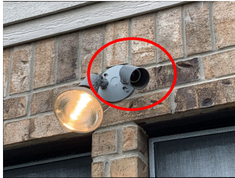
Rear: inoperative light fixture
