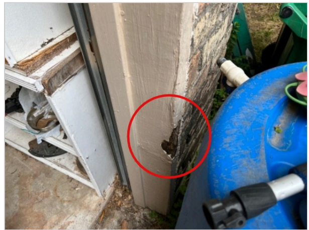
Wood damage - overhead garage trim
