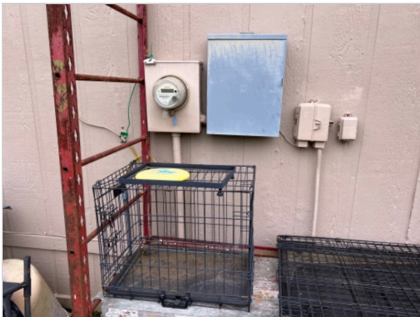
Electric meter and main panel box
