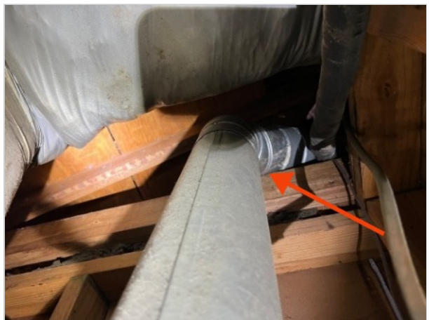
Flue in contact with combustibles
