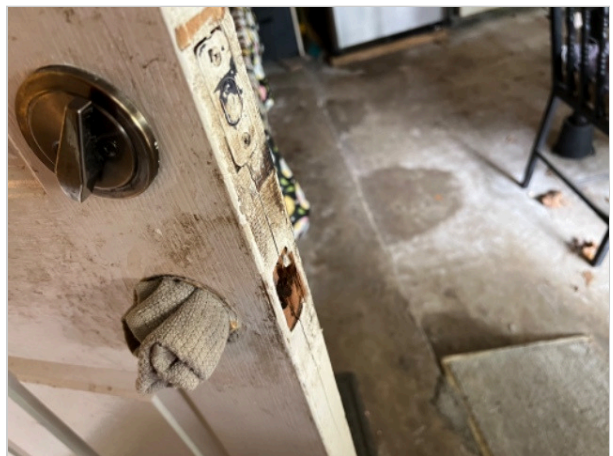
Damaged door from living area to garage
