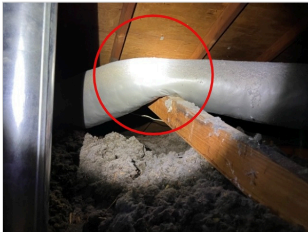
Duct in attic with restricted airway
