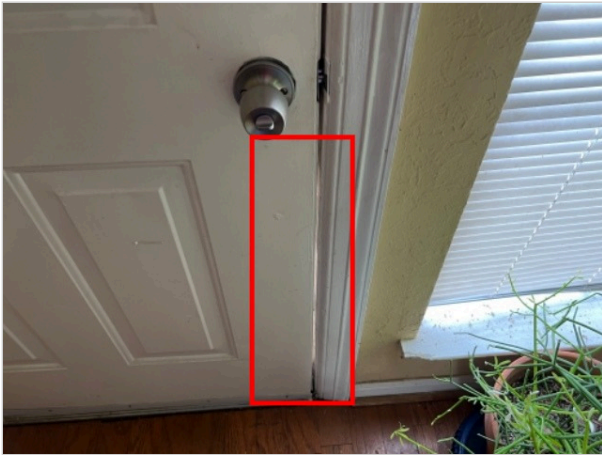
missing weather stripping at front door
