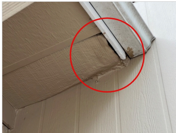
Damaged wood - above garage
