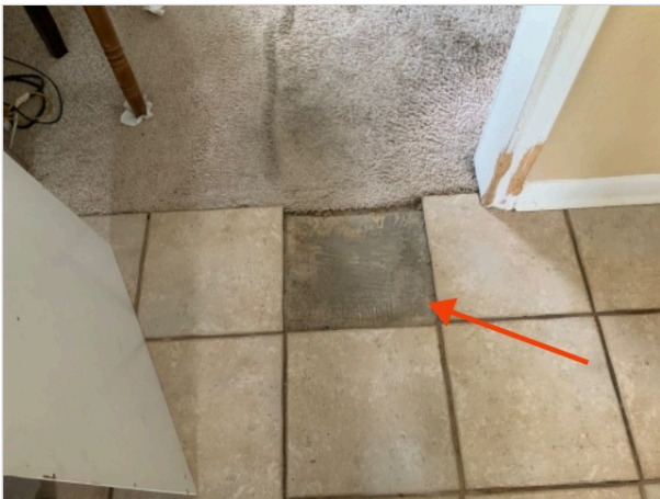
Tile piece missing from upstairs breakfast / dining room area
