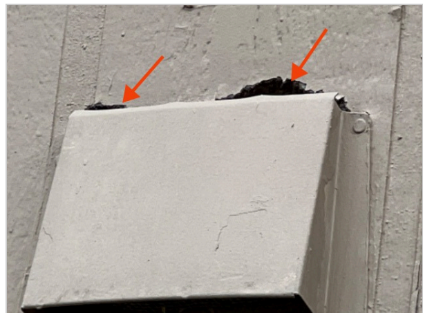
Void in rear wall
