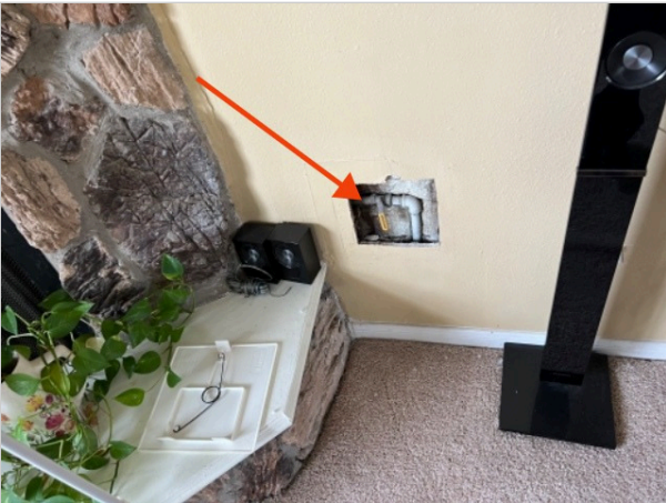
Gas valve for fireplace
