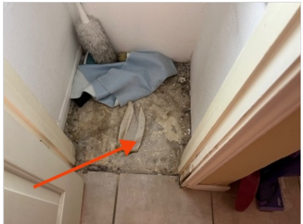
Tile missing from downstairs hallway closet floor
