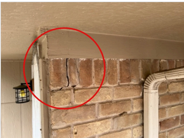
Loose brick - front porch
