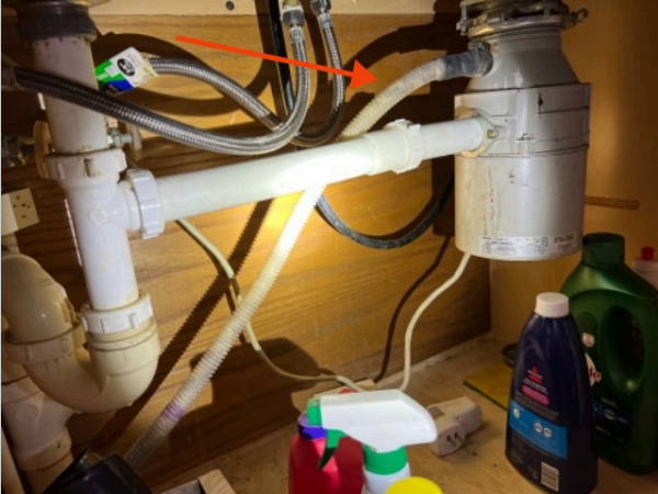
Improper dishwasher drain line loop
