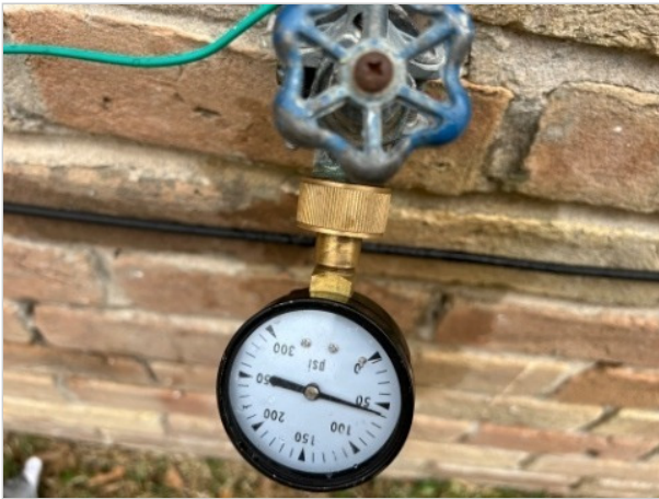
Water pressure reading (in the proper range)
