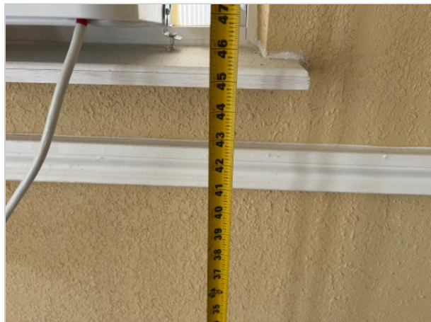
Upstairs bedroom window - Taller than 44" from the floor
