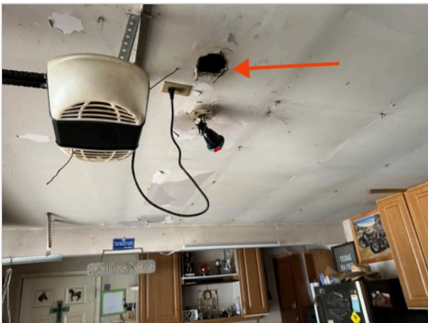
Garage ceiling - void / peeling
