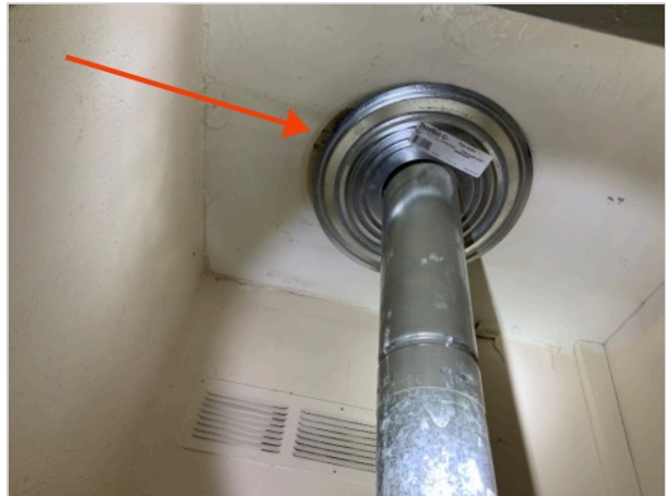
Flue pipe fire stop partially detached from ceiling
