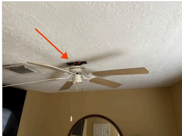
Partially detached fan & open splices not properly covered
