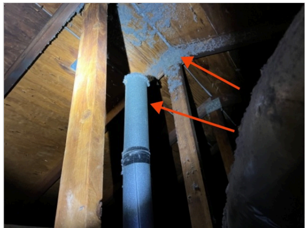
Dryer vent termination in attic / lint on combustible decking
