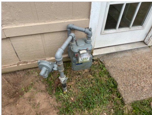
Gas meter / rear wall
