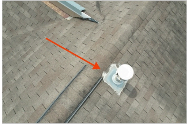
Improperly installed flashing
