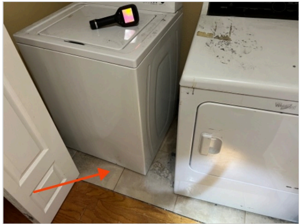
No pan under washing machine
