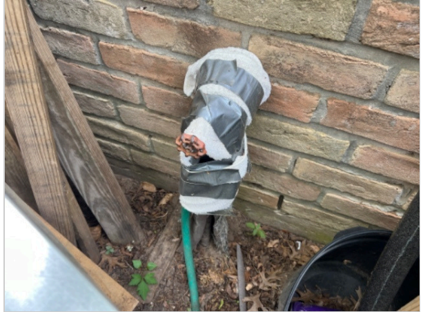
Main water valve - right side
