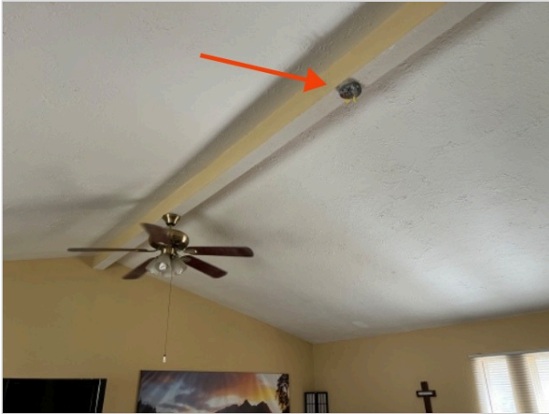
Electrical junction box without a fixture or cover
