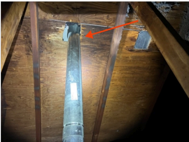
Flue pipe within 1" of combustibles
