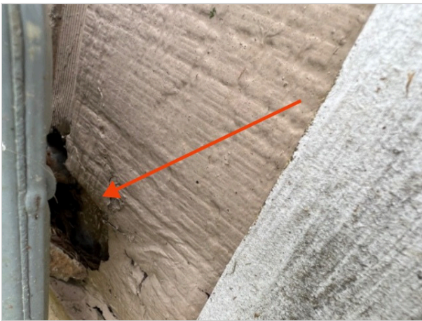
Void in rear wall
