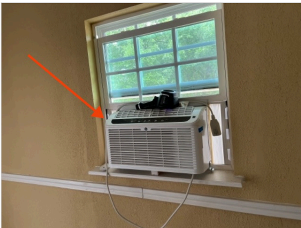
Only openable window in the upstairs bedroom - AC unit may block egress
