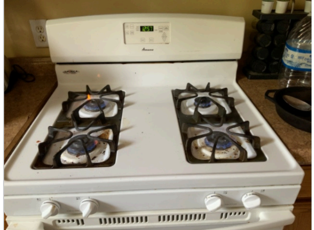
Cooktop burners functioning
