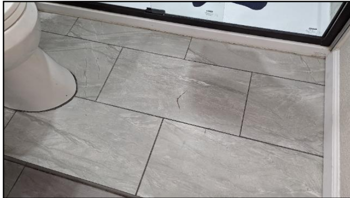
82. Odor around toilet
