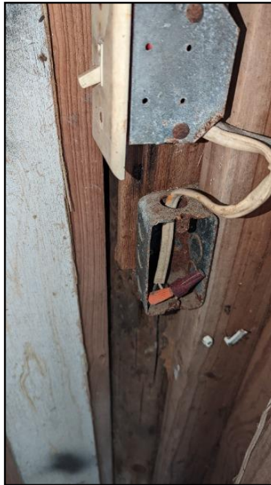
41. Cover loose or missing
