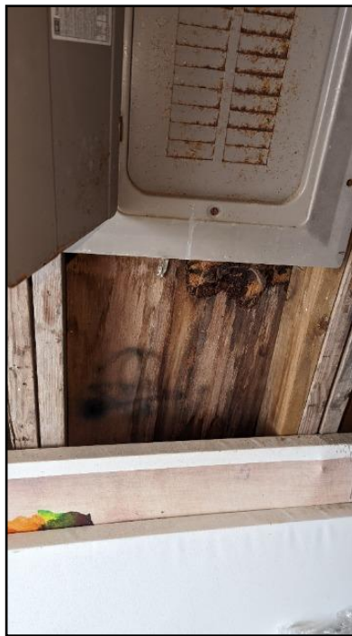
34. Inappropriate mounting surface
