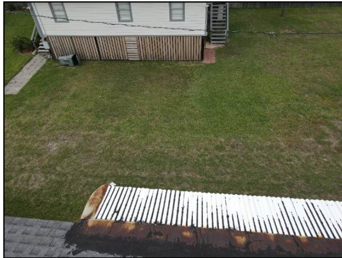
6. Damage, punctures, tears, bent metal
