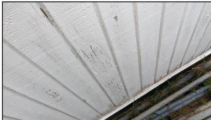
10. Paint or stain - needed
