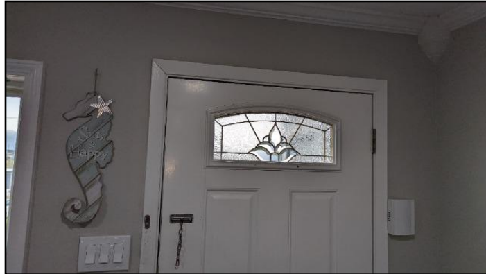
97. Loose or poor fit
