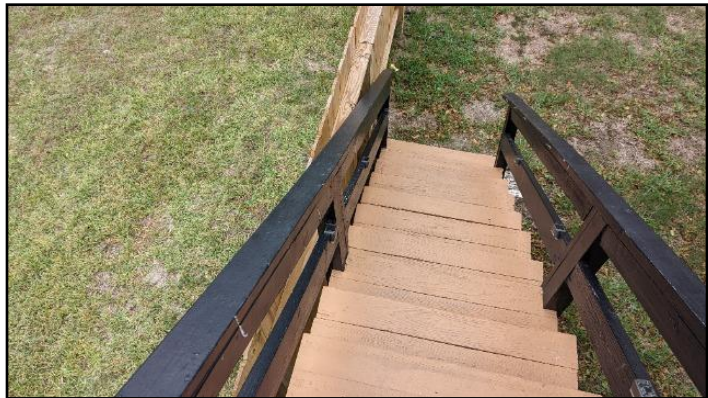
22. Openings between spindles (balusters) too...
