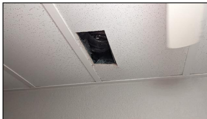
54. Disconnected or leaking
