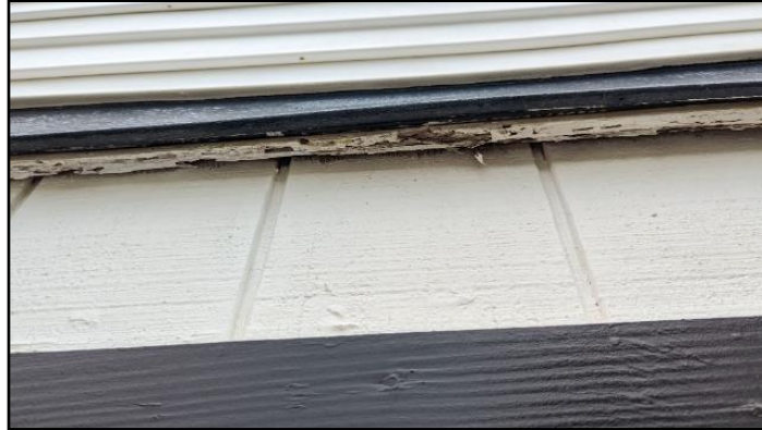
9. Flashings incomplete or ineffective
