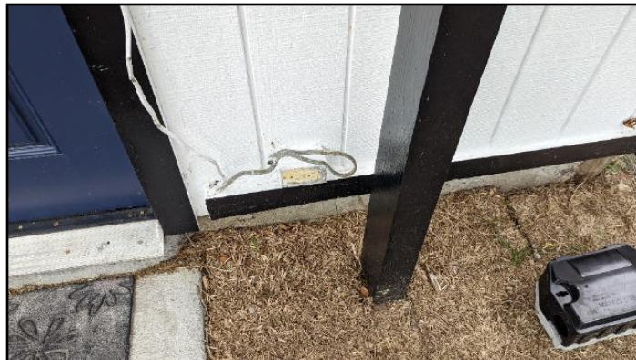
40. Wires too close to grade
