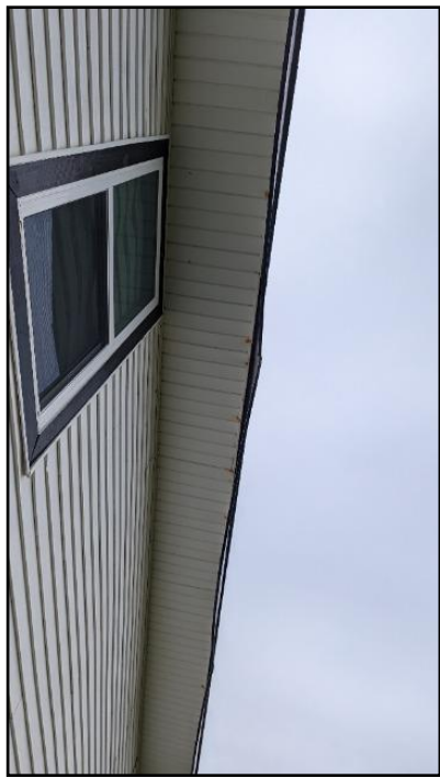
8. Vents - ineffective / missing
