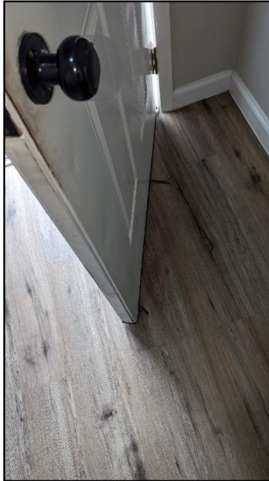
99. Weatherstripping missing or ineffective
