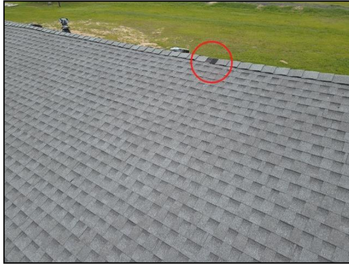
3. Missing, loose or torn
