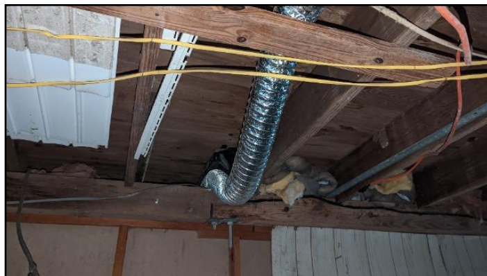
106. Dryer vent material not smooth wall
