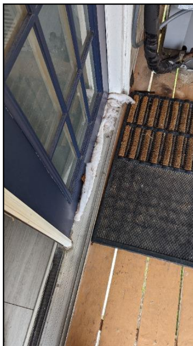
24. Door not tight-fitting and weatherstripped
