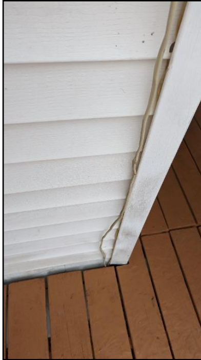
38. Indoor wire used outdoors
