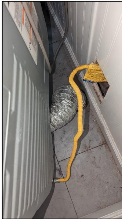
73. No drip leg (sediment trap, dirt pocket)
