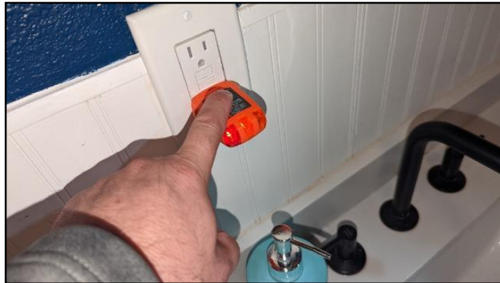
46. Test faulty on GFCI/GFI (Ground Fault...
