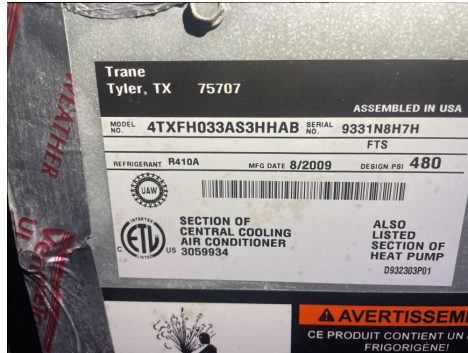
First floor rear Evaporator coil 2009 Trane R410a
