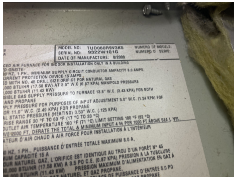
First floor rear heater 2009 Trane.
