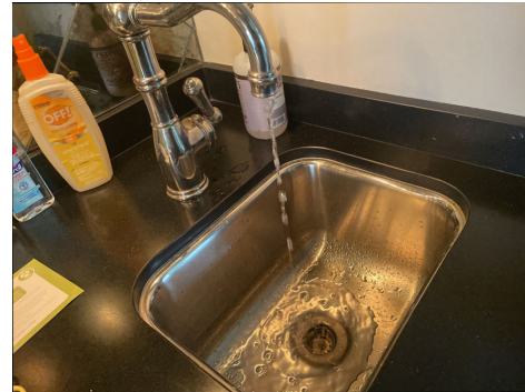
Low water pressure at Wet bar.
