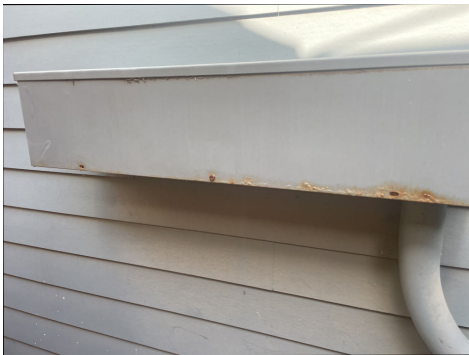
Could not open gutter box middle screw was too rusted/ stripped.
