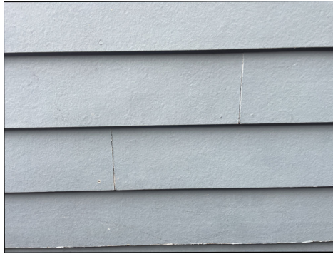
Caulk joints in siding.
