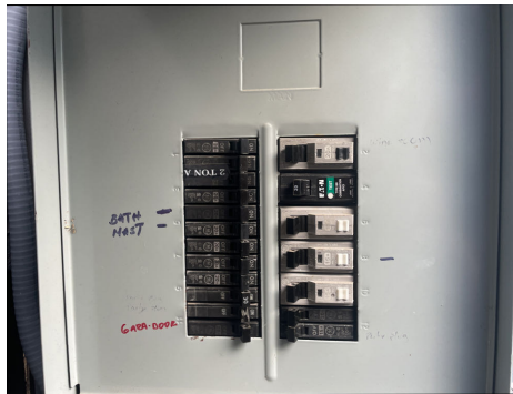
Sub panel is not labeled.
