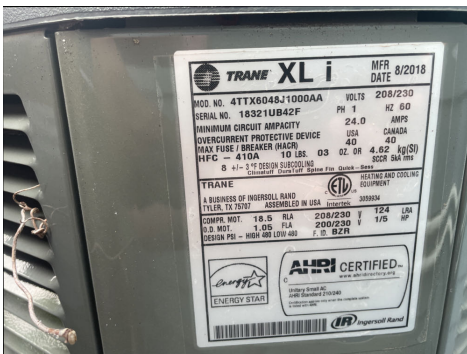
Second floor condenser 2018 Trane 4 Ton R410a
