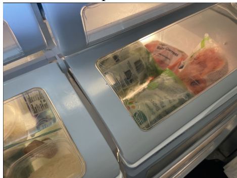
Damaged drawers observed in unit.
