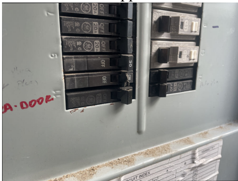
Breaker in sub panel is broken.
