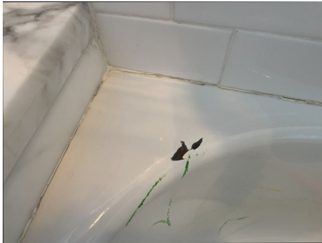
Porcelain damage to Jack and Jill tub.
