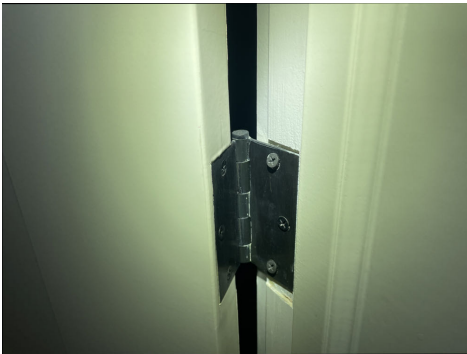
Hinge is loose.
