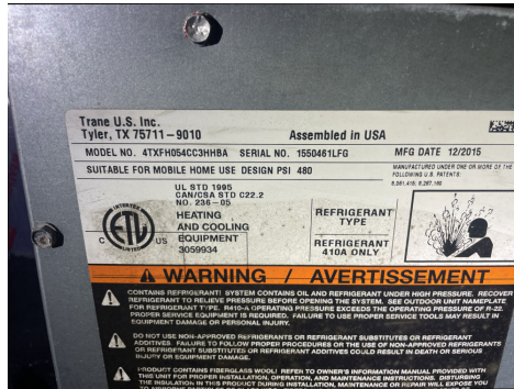
First Floor Front Evaporator coil 2015 Trane R410a
