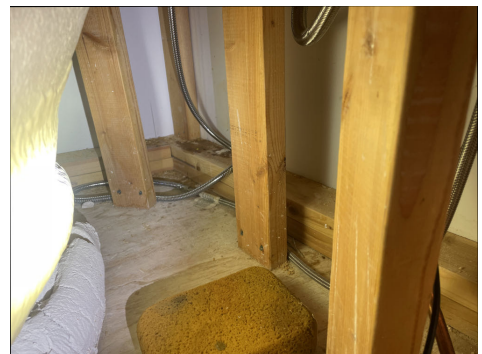
Stem washer leak drips below tub.
