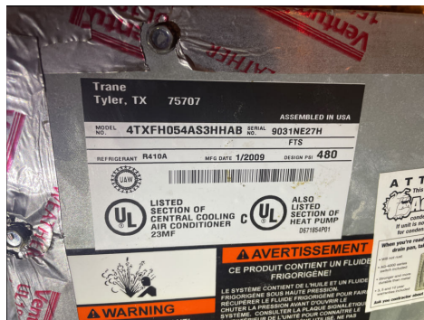
Second floor Evaporator Coil 2009 Trane R410a
