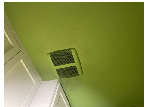
Microbial growth observed in Laundry area.
