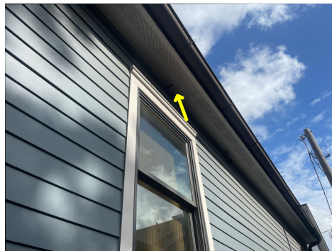
Drain line missing elbow.
