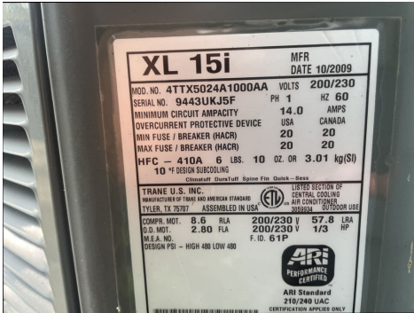
First floor rear condenser 2009 Trane 2 Ton R410a
