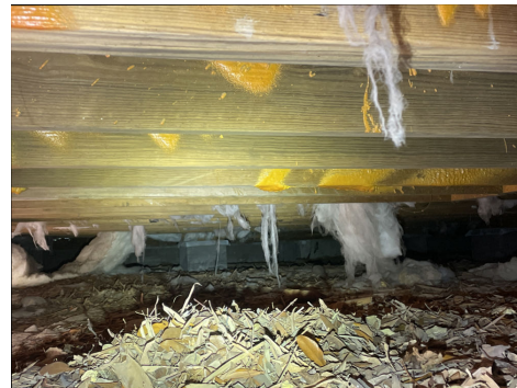
Insulation below house has fallen at one or more locations.
