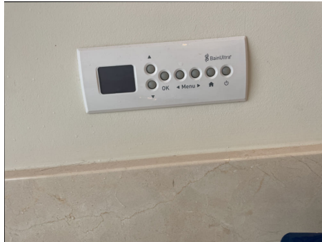
Control LCD screen was not operational.
