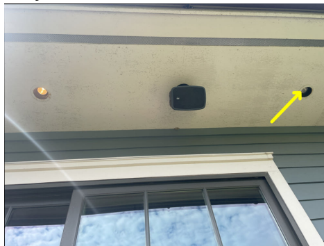
Light not operational.
