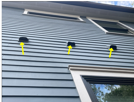
Exterior vent flapper door damaged.
