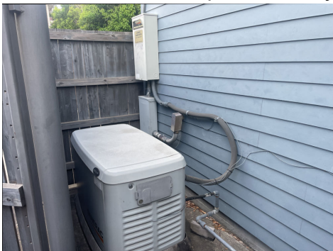
Generator not checked/ inspected.
