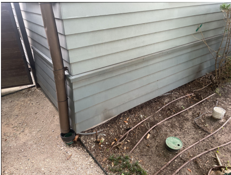
No foundation vents with in 3 feet of corner.
