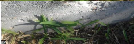
Spalling on the south side
