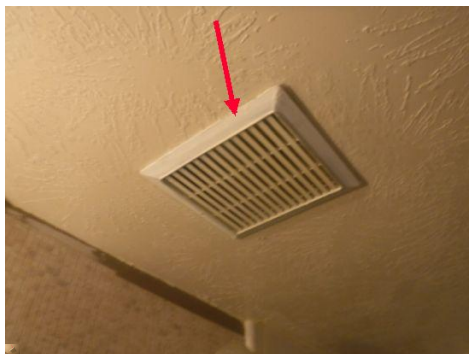
Fan is vibrating
