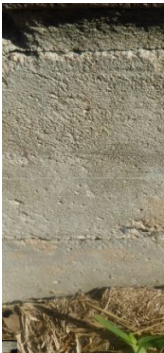
Vertical shrinkage crack
