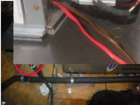
Missing sediment T trap
