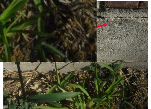
Vertical shrinkage crack
