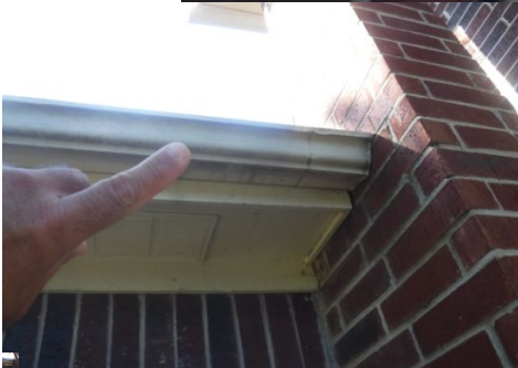
Congested rain gutters/needs cleaning/leaning gutters
