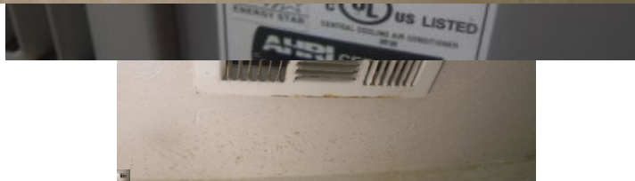
Rust on the AC vent in the master
