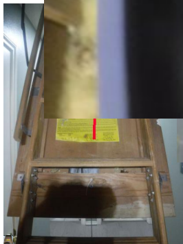
Attic access hatch needs insulation
