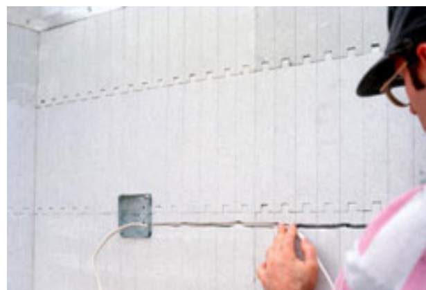
Utilities are typically recessed into cutouts in foam after concrete has been placed
