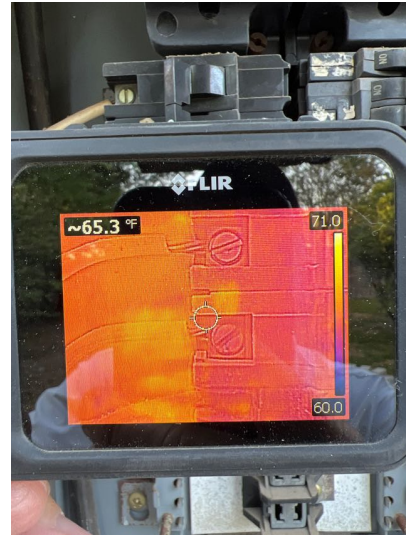
Thermal imaging camera used to detect over heating electrical components. No issues.
