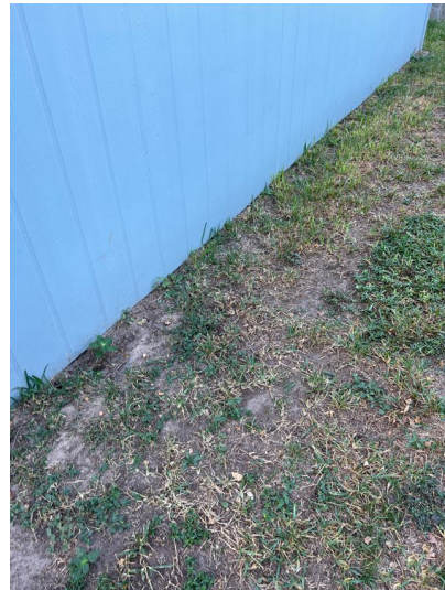
High soil, back side of garage
