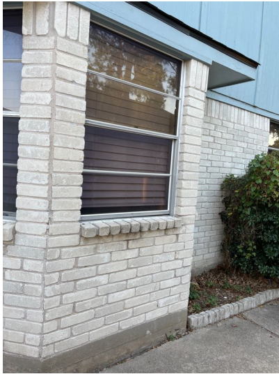
Windows missing screens.
