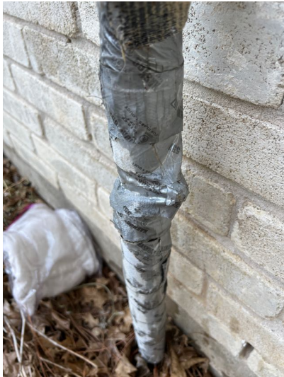
Water shut off valve
