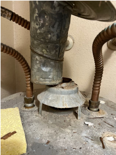
Improper flue pipe venting was noted and further evaluation is recommended
