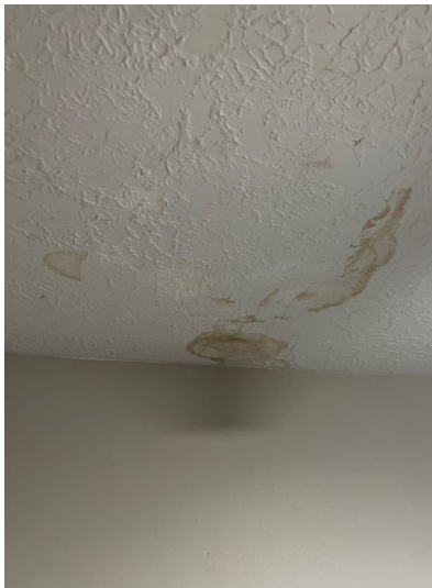
Moisture stain on ceiling.
