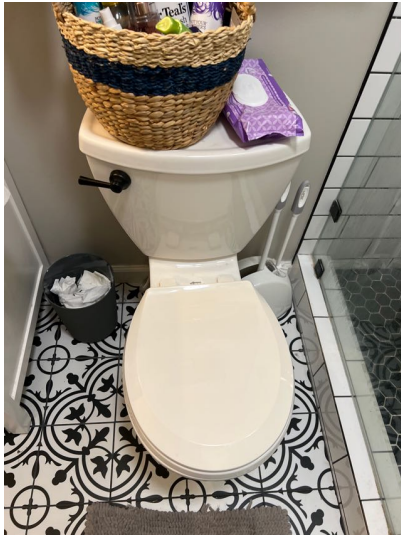
Master bathroom toilet loose where attached to floor
