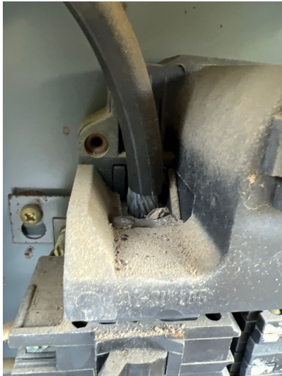
Aluminum service conductors missing anti-oxident grease.
