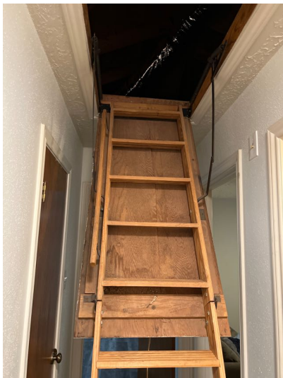
Attic access missing insulation.
