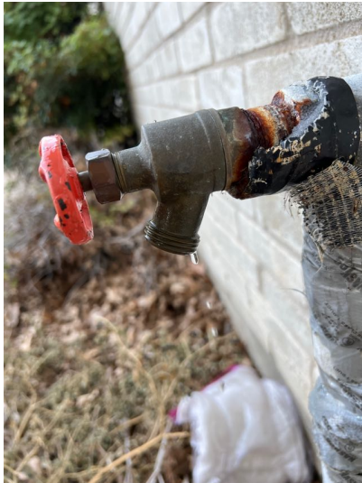
Hosebib missing anti-siphon device.
