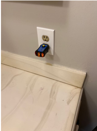
Bathroom electrical receptacle not GFCI protected.
