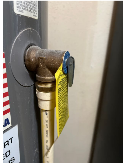
Water heater temperature and pressure relief valve is damaged.
