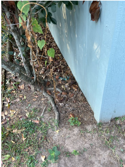
High soil right side of garage
