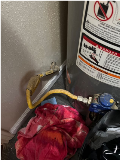
Water heater gas piping missing sediment trap.
