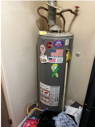
Picture of water heater
