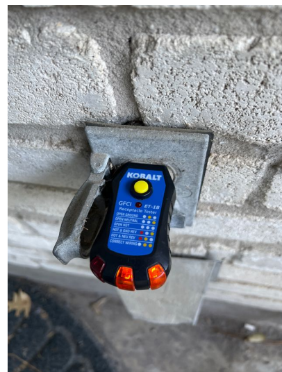
Exterior electrical receptacle not GFCI protected.
