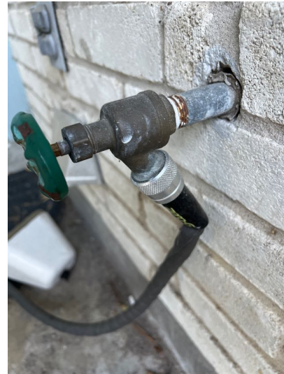
Hosebib missing anti-siphon device.
