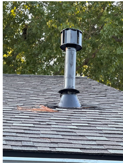
Water heater exhaust pipe
