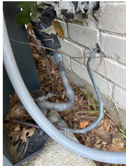
Damaged insulation on freon line at AC condensing unit.
