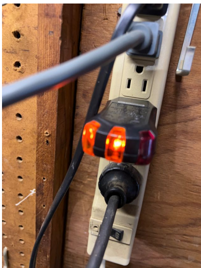
Garage electrical receptacle not GFCI protected.
