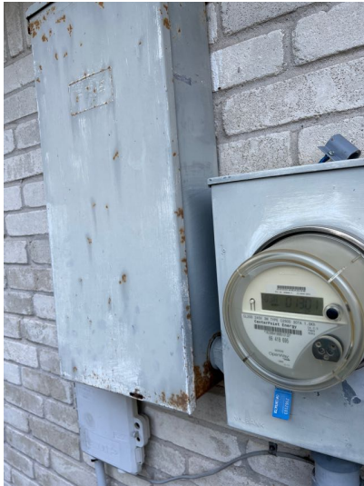
Picture of electrical service panel.
