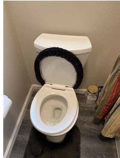
Hall bathroom toilet loose where attached to floor
