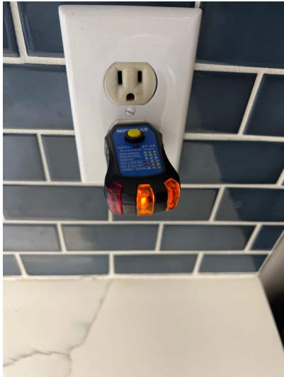
Kitchen electrical receptacle not GFCI protected.
