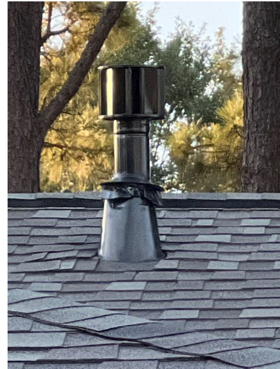
Furnace exhaust pipe
