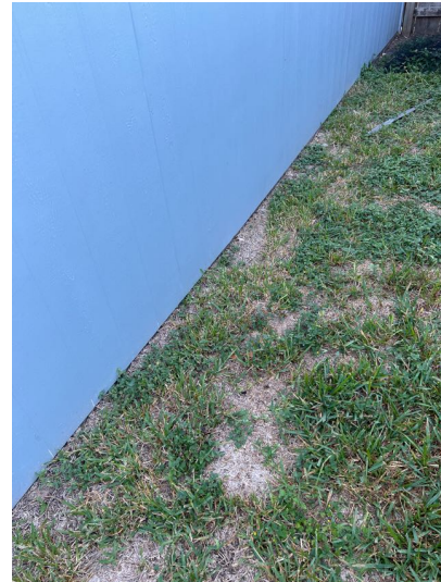
High soil left side of garage .
