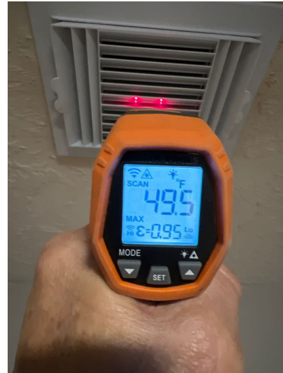
Air temperature measured at supply air vent.
