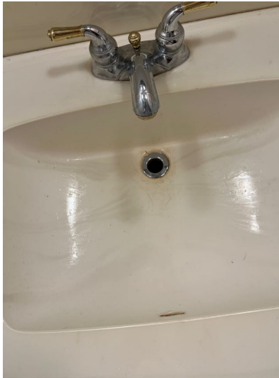
Hall bathroom vanity noted with missing drain stop
