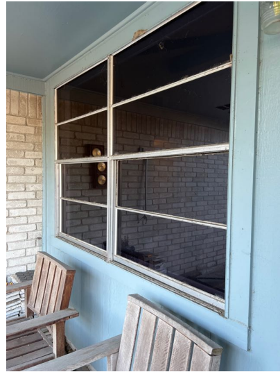
Windows missing screens.
