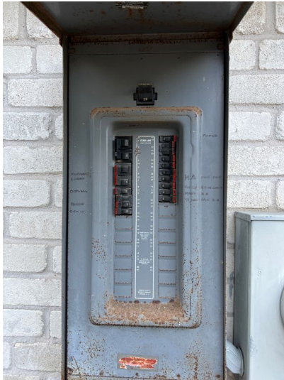
Picture of electrical service panel.
