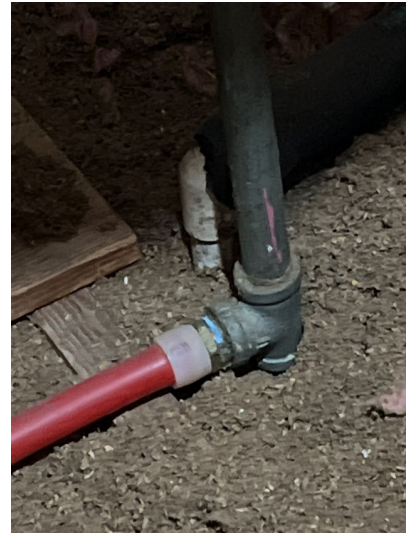
Galvanize steel water piping and PEX water piping
