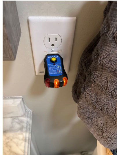
Bathroom electrical receptacle not GFCI protected.
