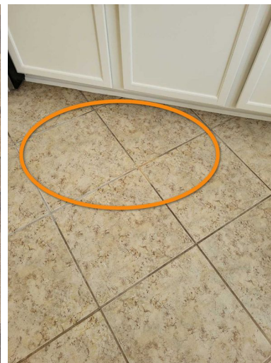
Floor sounds hollow in area near oven
