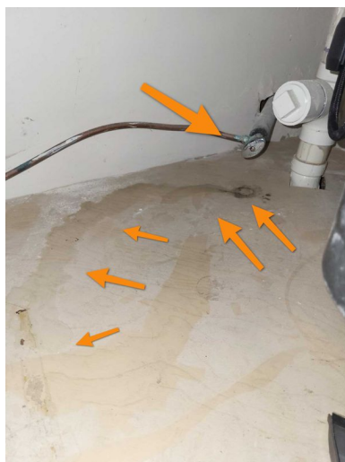
Leaking at water shut off
