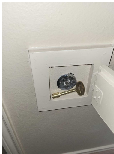
Emergency gas shut off
