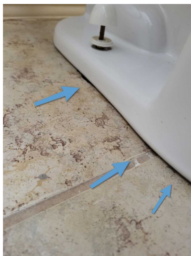
Toilet master bath
