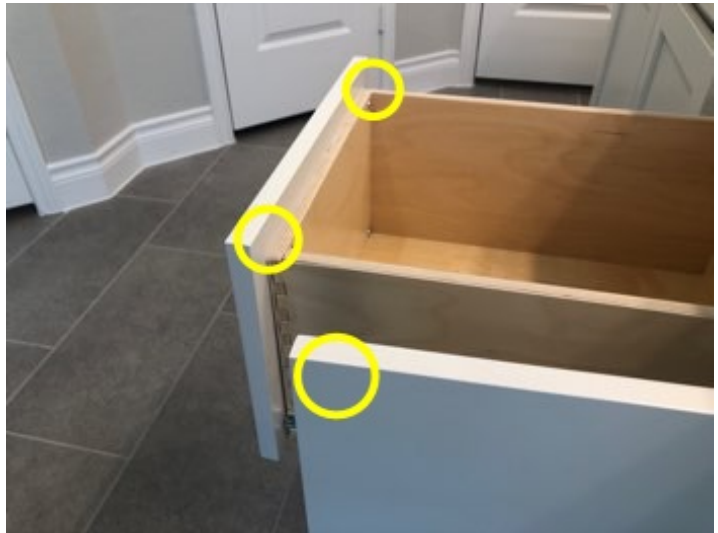
Install missing rubber bumpers to all cabinet doors and drawers at kitchen and bathroom areas.
