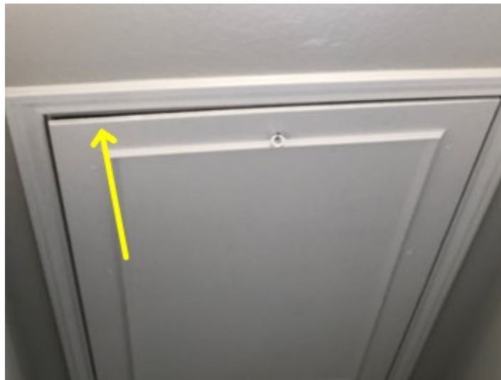
The drop-down attic access door above the second-floor hallway area does not appear to adequately/fully shut. Adjust/repair as needed in order to completely shut as intended.
