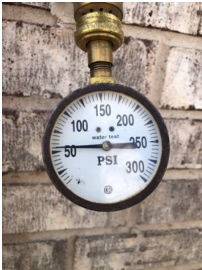
Static water pressure reading is 56 psi.
