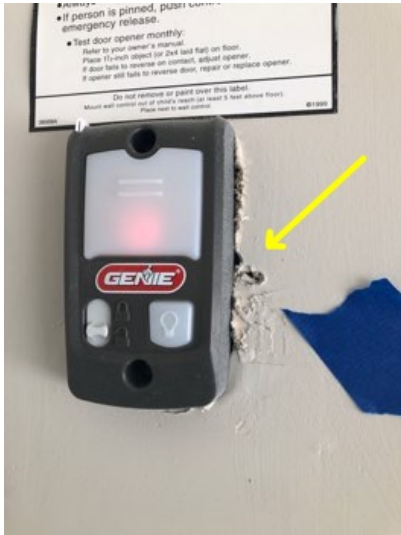
Repair the damage to the wall near the garage door opener pushbutton control North of the garage area.
