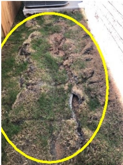
Missing/trampled sod observed near the AC condensing units SE of the house.
