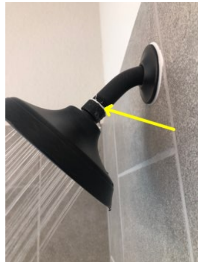
Repair the leak from the showerhead/pipe connection at master bathroom.
