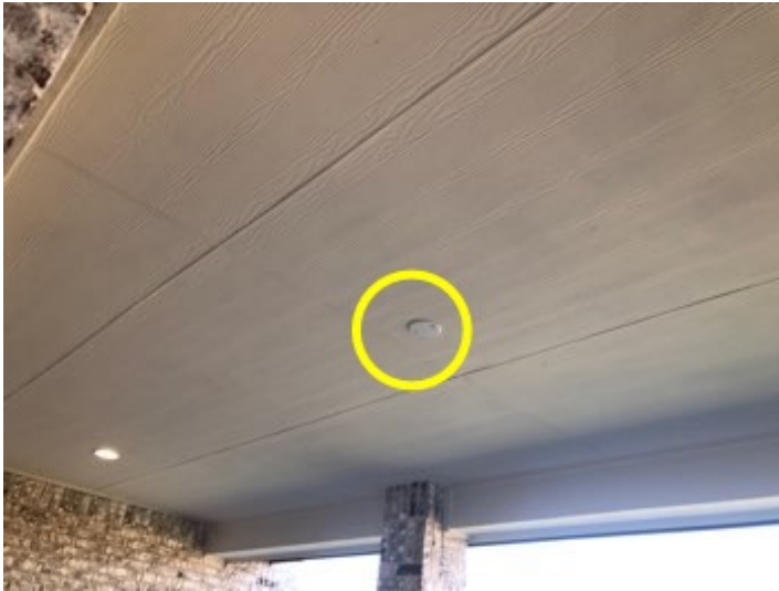
Install missing electrical fixture to the junction box at ceiling above the covered patio at bat of the house.
