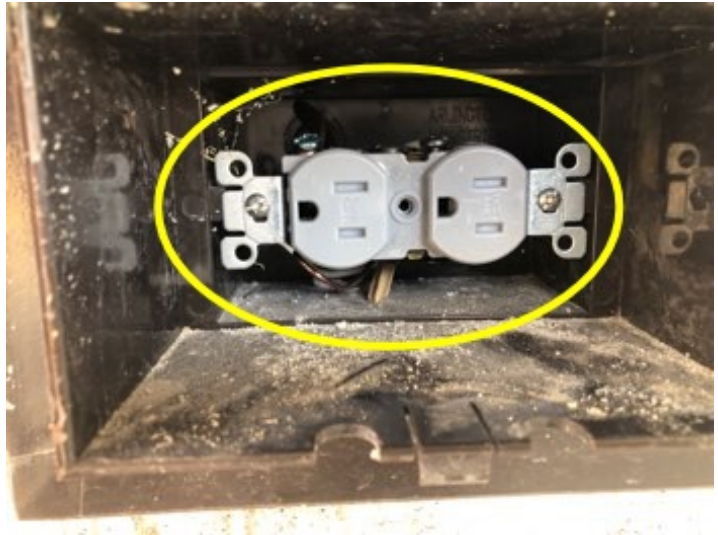
Install missing cover plate to the outdoor receptacle at covered patio at back of the house for proper safety.
