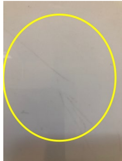
Retouch paint marked walls within the garage area marked with blue tape.
