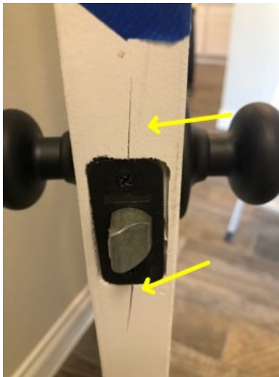
Slight crack observed to the utility room door near the latch.
