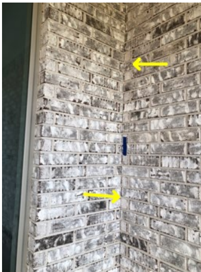
Caulk/seal the corner abutted brick joint that is void at SE corner of the covered patio at back of the house.
