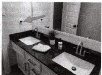
Upstairs bathroom electrical outlet receptacle is not GFCI protected.
