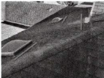
Sky light flashing and chimney flashing need to be painted.
