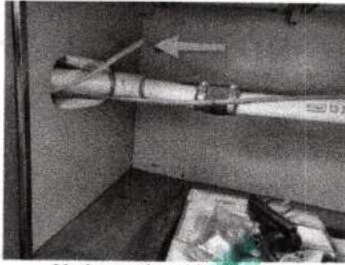
Under outdoor kitchen sink.
