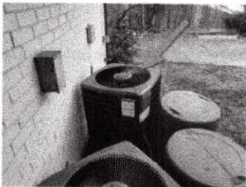
First air conditioning condenser unit not functioning at the time of the inspection.
