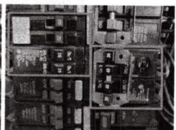
Circuit breakers not manufactured by Bryant.
