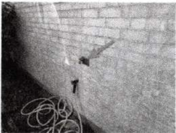
Exterior electrical outlet receptacles on the home.
