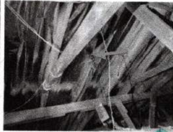
Branch wire splices need to be fully encased inside a junction box in the attic above the 2nd Floor of the home
