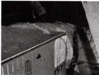
Right unit in the attic above the 2nd Floor
