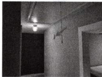
Carbon monoxide alarms missing outside the bedrooms of the home.
