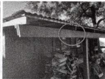
Rear covered patio header splice not supported from below.
