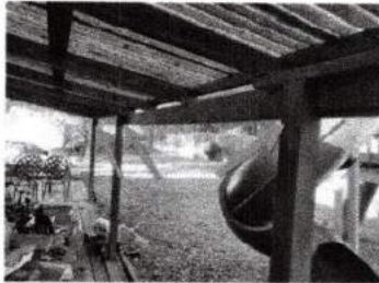
Rear covered patio header not supported from below.
