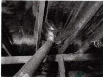
Left furnace above the 2nd Floor of the home
