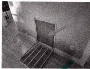
2nd Floor return air filter.
