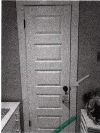
Upstairs rear left bedroom closet door.
