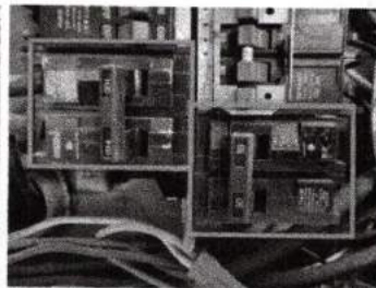
Circuit breakers not manufactured by Bryant.
