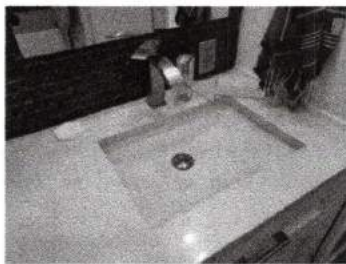
Right master vanity sink makes a hammering noise when in operation.
