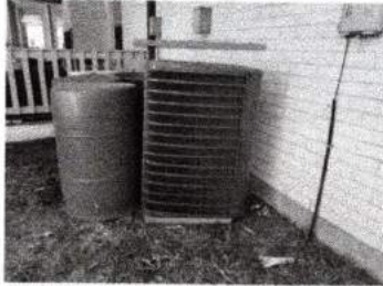
Left air conditioning condenser unit at the rear of the home.
