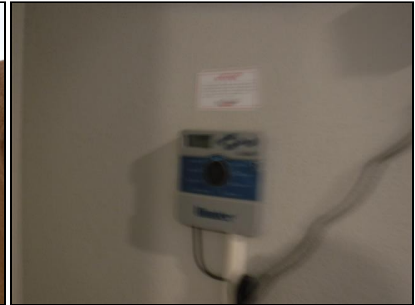
Irrigation control panel located within garage.
