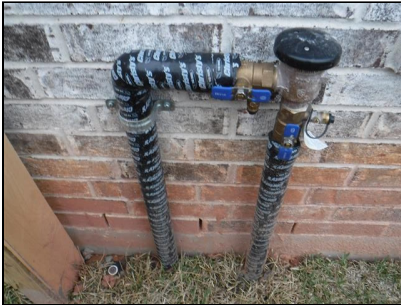
Irrigation back flow preventer located right side of residence.
