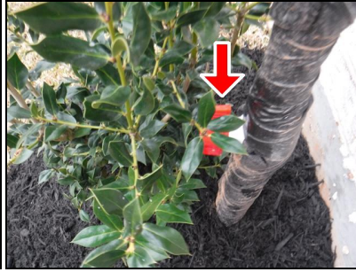
Main water shut off located right side of residence.
