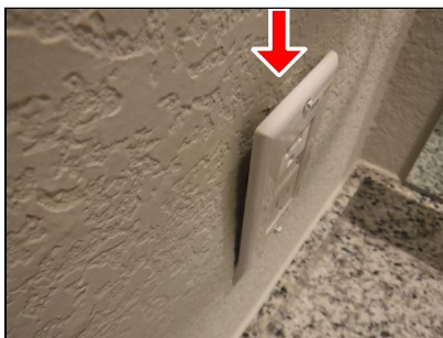
This cover plate within guest bathroom is not attached.
