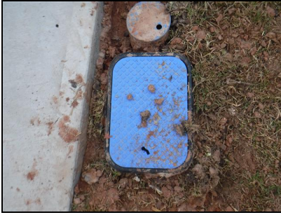
Water meter located front of residence.
