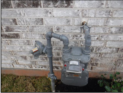
Gas meter located left side of residence.
