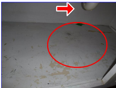
Full bathroom sink base
