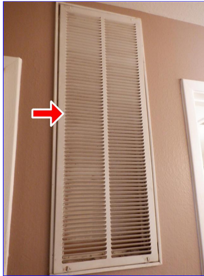
Missing air filter
