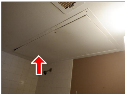
Attic evaporator unit panel door
