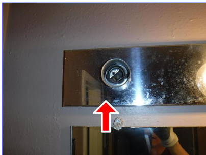
Full bathroom lighting
