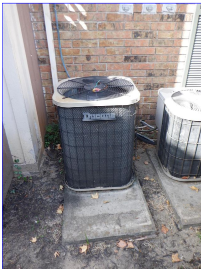
Outside AC unit
