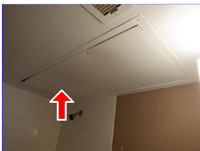
Attic evaporator unit panel door
