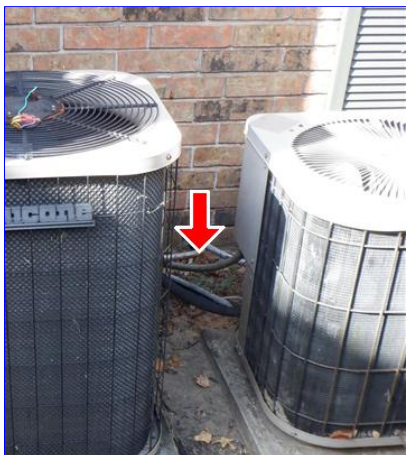
AC condenser line
