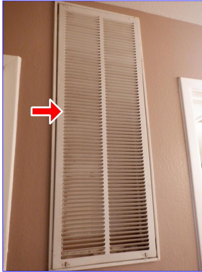
Missing air filter
