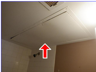
Unable to open evaporator unit panel
