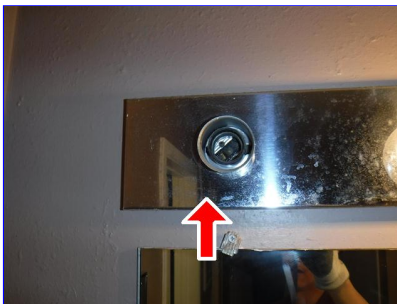
Full bathroom lighting
