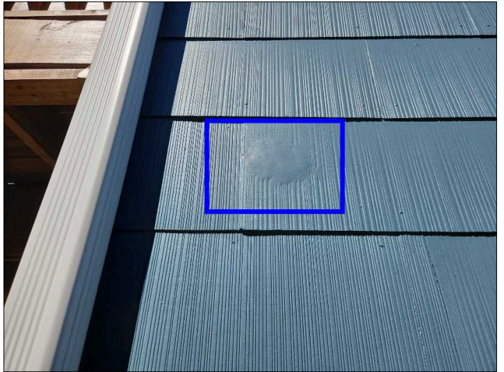
- There are signs of previous repairs in the siding. Unable to determine condition of underlying materials. Mainly at - left side
