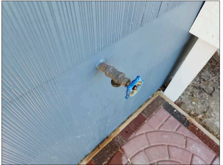
- Recommend adding or replacing insulation to exterior faucets to help prevent freezing.
