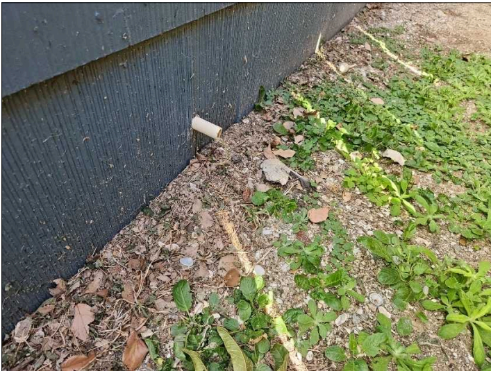
- The water heater pan drain or T&P (Pop-Off) valve drain line does not have a properly installed 90 elbow to safely direct the high-pressure discharge from the valve where it exits the exterior.
