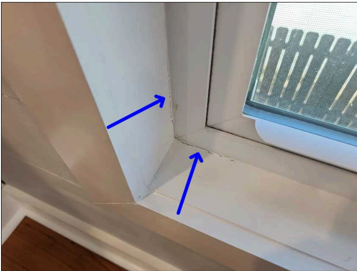
- Sealant is needed around various windows between the window framing and exterior brickwork or trim to help prevent water penetration, recommend checking all windows for proper sealant.
