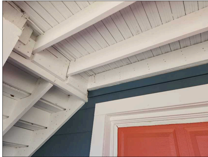
- Joist hangers are missing on the patio cover joist.
