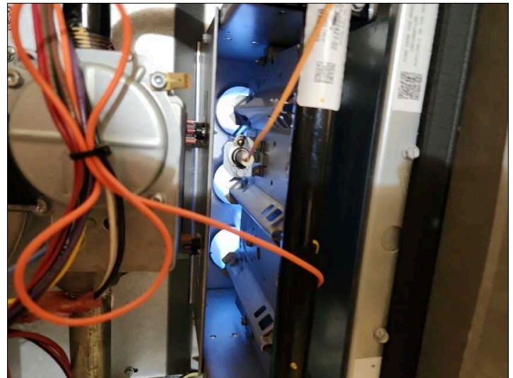
Overview of furnace burner compartment.
