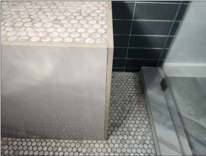
- Recommend sealing the shower surround to help prevent water penetration to underlying materials. Mainly at - hall bath
