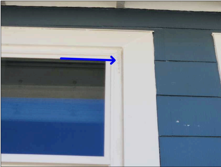
- Sealant is needed around various windows between the window framing and exterior brickwork or trim to help prevent water penetration, recommend checking all windows for proper sealant.
