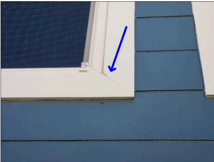
- Recommend sealing trim to help prevent water penetration. Mainly at - right side
