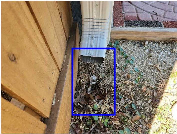
- Splash blocks or downspout extensions should be installed to direct water away from foundation.
