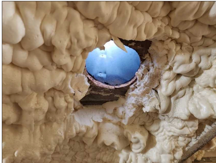
Unused vent. Recommend sealing to help retain proper insulation.
