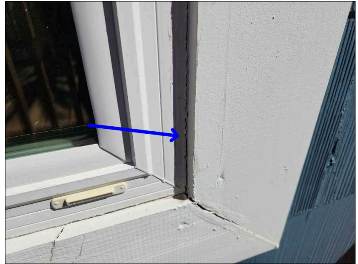
- Sealant is needed around various windows between the window framing and exterior brickwork or trim to help prevent water penetration, recommend checking all windows for proper sealant.
