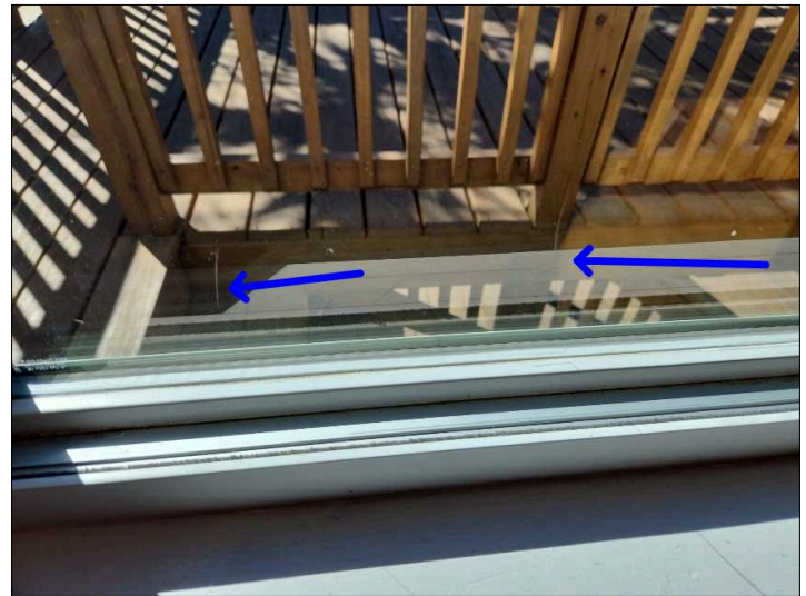
A scratch was noted in a window pane. Mainly at - rear bedroom
