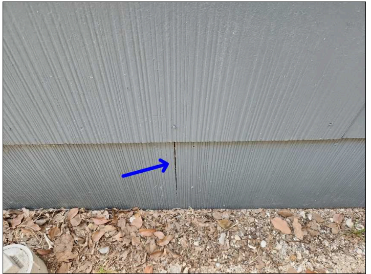
- There are gaps at the joints in the siding in various locations due to shrinking and expansion of siding materials, recommend sealing all open joints in the siding to help prevent water penetration.
