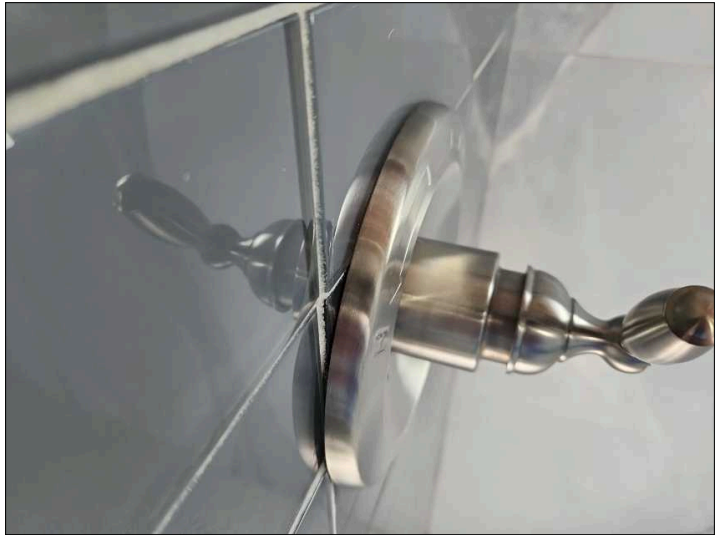
- All tub shower faucets and spouts should be sealed to help prevent water penetration behind the fixture.
