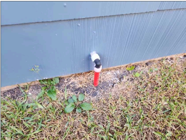
- PEX pipe material should not be used outdoors unless buried or otherwise protected. PEX piping will deteriorate in the prolonged presence of ultraviolet rays, so it should not be used outdoors if there is a chance that it will be exposed to sunlight for any duration.
