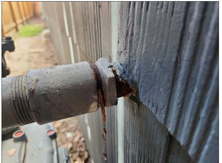
- Paint pipe at gas meter to help prevent premature deterioration.
