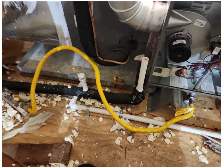
- Gas flex line exceeds proper length. Mainly at - furnace
