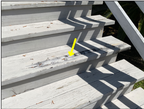
Rot/deterioration front stair treads.
