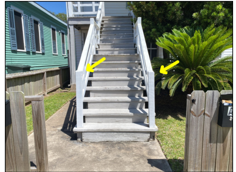
Loose railings front exterior stairs.
