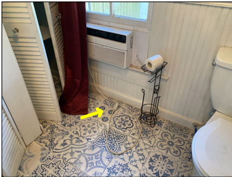
No outlet for unit first floor bathroom.
