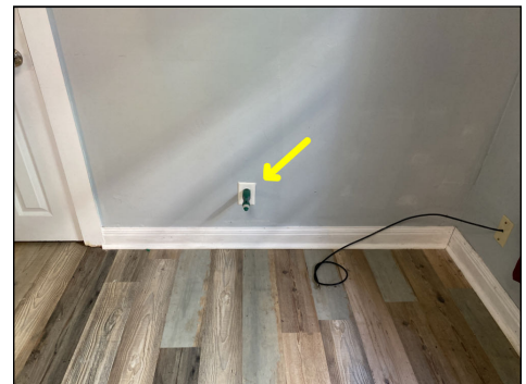
No power to outlet rear first floor bedroom.
