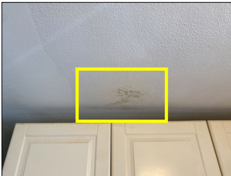
Organic like growth first floor kitchen.
