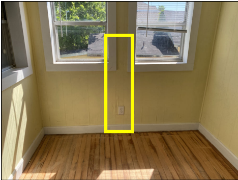
Prior leakage evidence laundry room.
