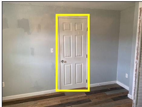
Door sticks front first floor bedroom.
