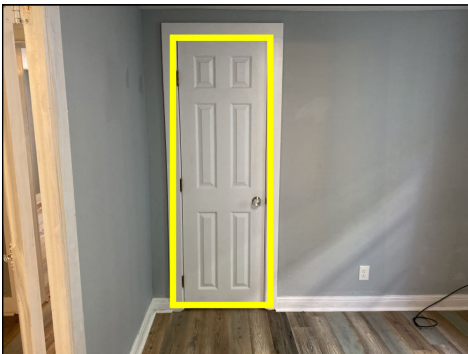
Door will not latch rear first floor bedroom closet.
