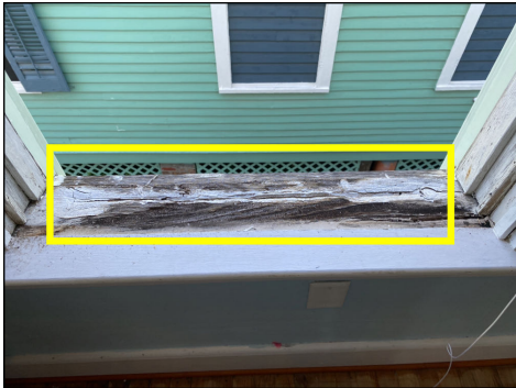
Rot/deterioration window trim second floor.
