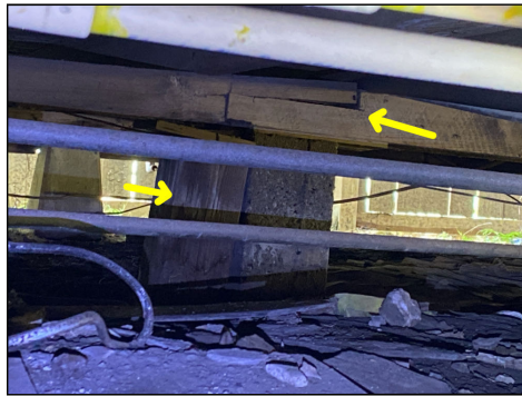
Leaning piers/damaged beams.
