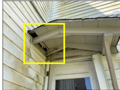
Rot/deterioration first floor kitchen exterior door patio cover.
