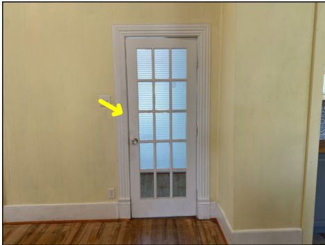
Door sticks second floor bathroom.
