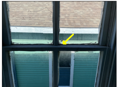
Missing window latches second floor bathroom.
