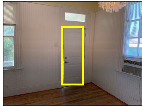
Door sticks second floor front.
