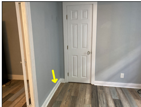
Missing doorstop example.
