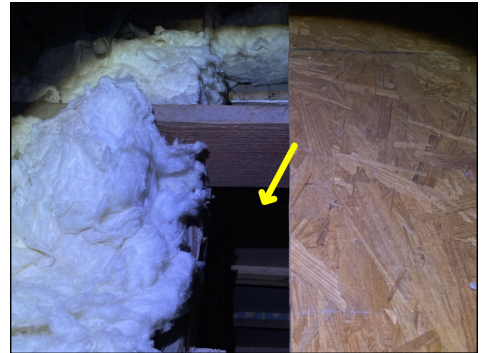
Missing fire blocking.
