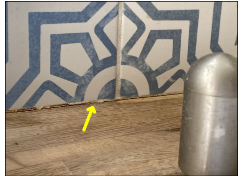
Unsealed countertop edge second floor kitchen.
