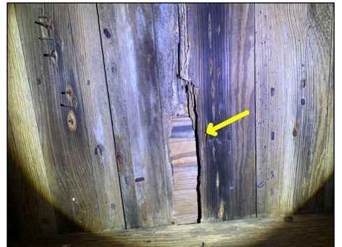
Rot/deterioration of subfloor first floor.
