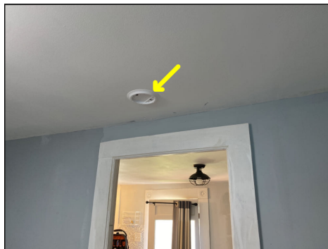
Missing bedroom smoke detectors example.
