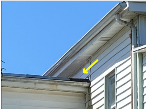
Gutter not draining.
