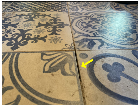
Crumbled grout first floor bathroom.
