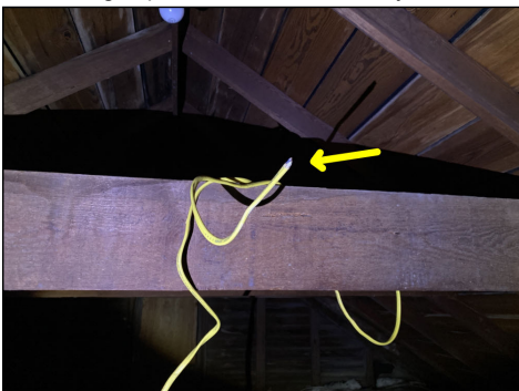
Energized exposed wiring attic.
