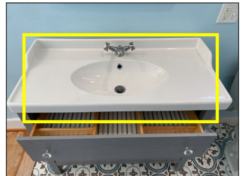
Sink/vanity not secured second floor bathroom.
