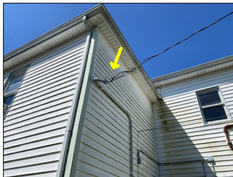
Improper drip loop/weather head.
