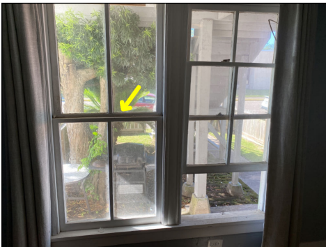
Missing window latch first floor bedroom.
