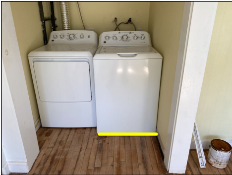
No laundry drain pan.
