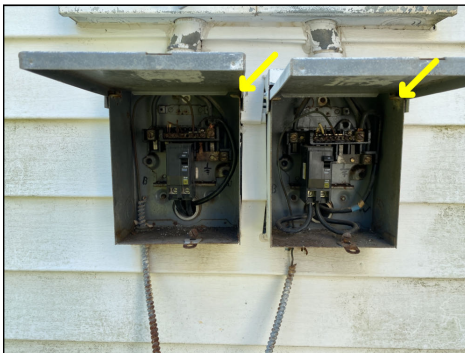
Missing dead fronts exterior disconnects.
