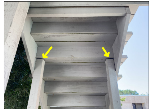
Front stairs not bearing on posts.
