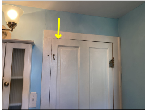
Door sticks first floor bathroom/bedroom.
