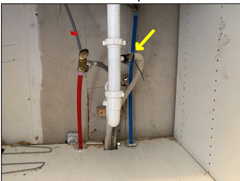
Missing drain air gap/high loop first floor kitchen.
