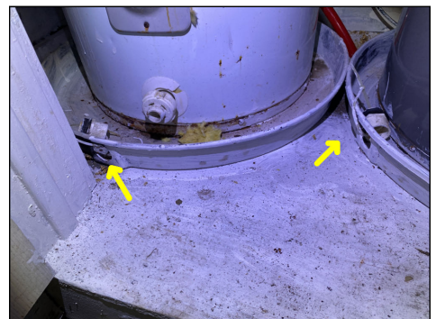
No drain pan drain lines.
