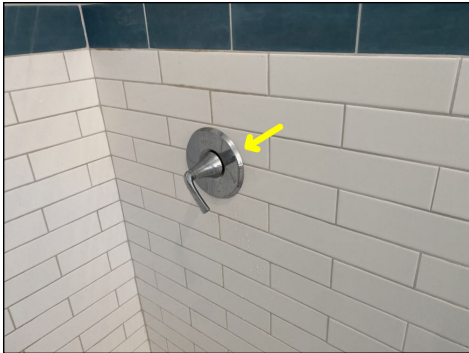
Hot/cold reversed second floor bathroom shower stall.
