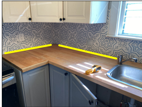
Unsealed countertop edge first floor kitchen.
