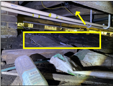
No vapor barrier/floor insulation.
