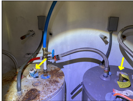
No TPR drain lines.
