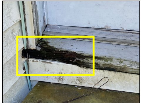
Rot/deterioration first floor kitchen exterior door.
