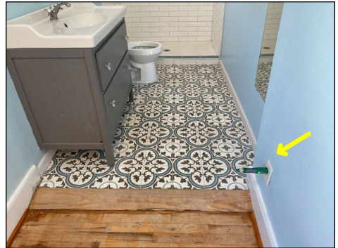
Missing gfci protection second floor bathroom.
