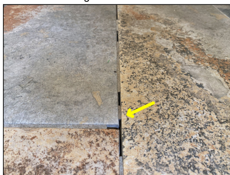
Crumbled grout second floor kitchen.
