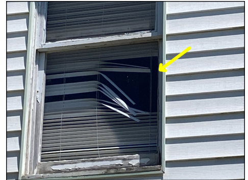
Damaged blinds example.
