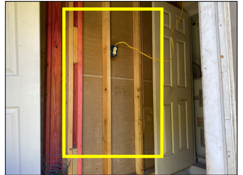
Missing wall insulation exterior closet.
