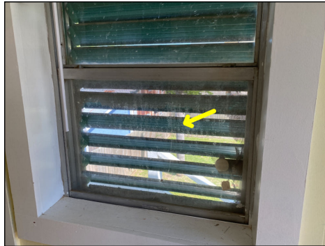
Damaged window laundry room.
