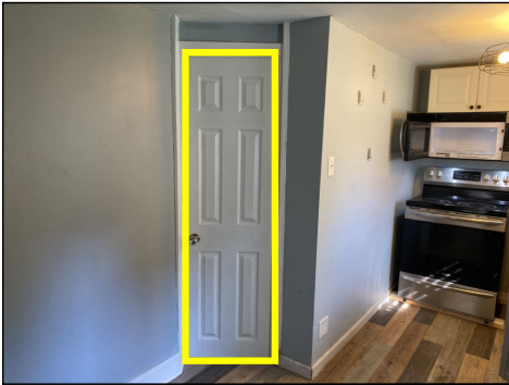
Door sticks first floor bathroom/kitchen.
