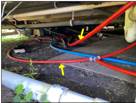
PEX piping not secured as required.
