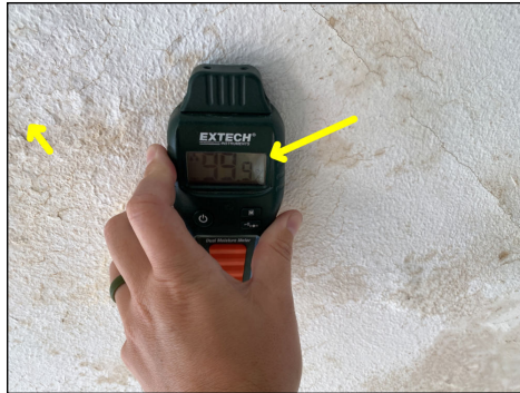
Active leakage laundry room.
