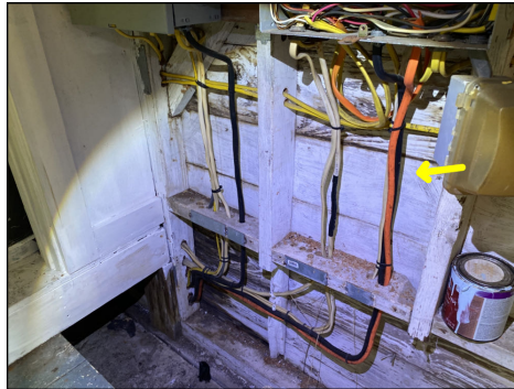
Wiring exposed on interior exterior closet.
