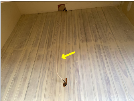
Wiring exposed on interior second floor living room closet.
