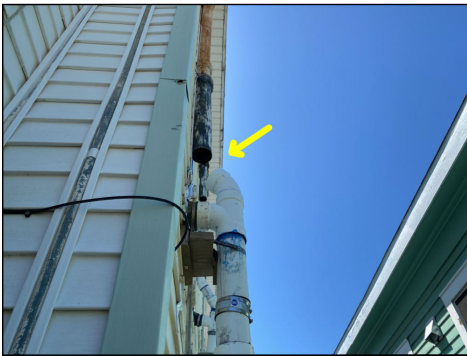
Drain piping voids rear of home.
