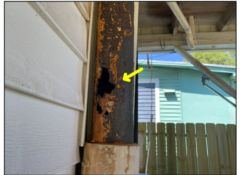
Corrosion/deterioration of drain piping rear of home.
