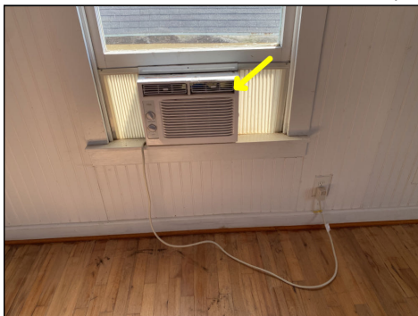
Inoperative unit second floor bedroom.
