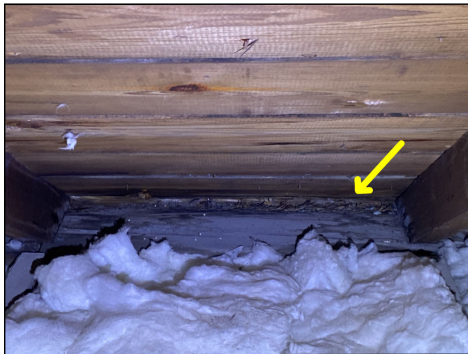
Rot/deterioration of attic framing.
