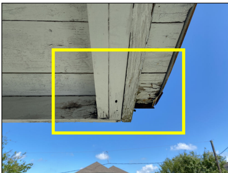
Rot/deterioration laundry room exterior patio overhang.
