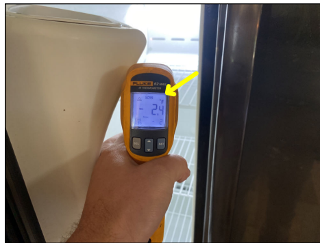
First floor kitchen freezer temp.
