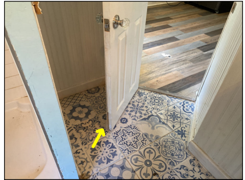
Damaged door first floor bathroom/kitchen.
