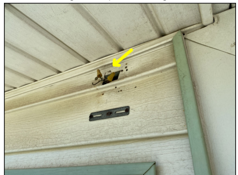
Abandoned wiring rear of home.
