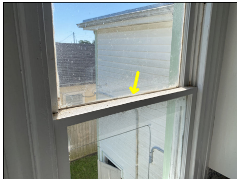
Missing window latch second floor kitchen.
