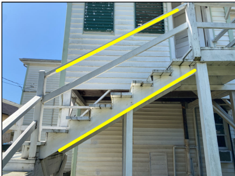
Stair baluster spacing.
