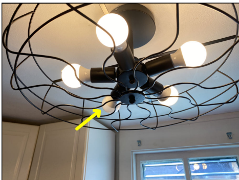
Inoperative light first floor kitchen.
