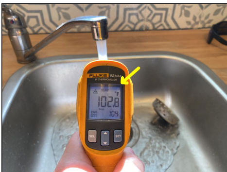
Heated water temp first floor kitchen sink.
