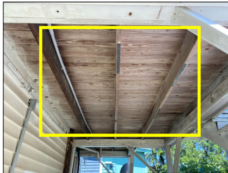
No floor insulation below laundry room.
