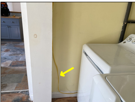
Wiring exposed on interior laundry room.
