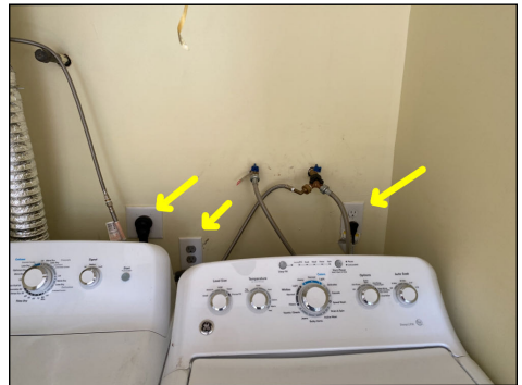
No gfci protection laundry room.
