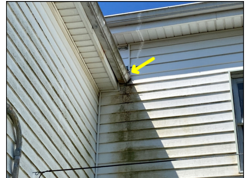
Loose gutter/spill out evidence rear of home.
