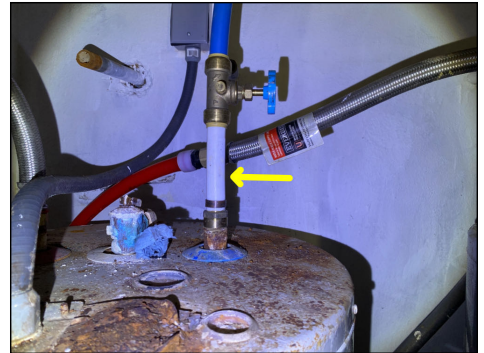
PEX connected direct to unit GE.
