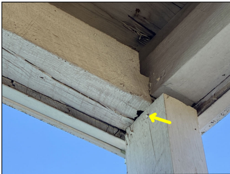
Rot/deterioration laundry room floor structure.
