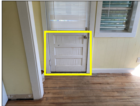
Deterioration, weatherstripping, door sticks laundry room exterior door.
