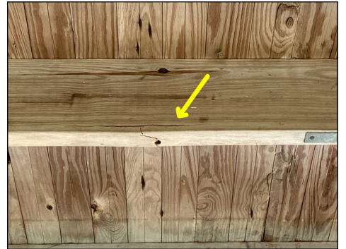
Damaged joist below laundry room.
