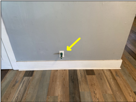
No power to outlet first floor living room.
