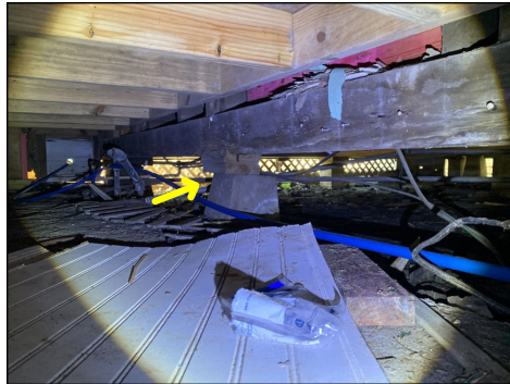
Beams not centered on piers.
