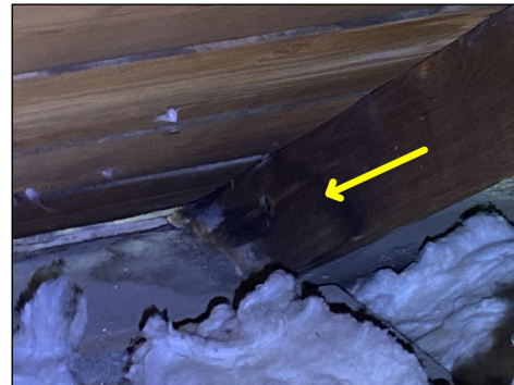
Prior leakage/organic like growth.
