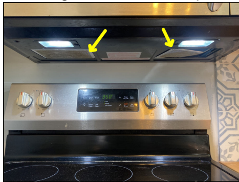
Dirty filters first floor kitchen unit.
