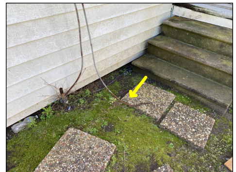
Ground wire not connected at rod.
