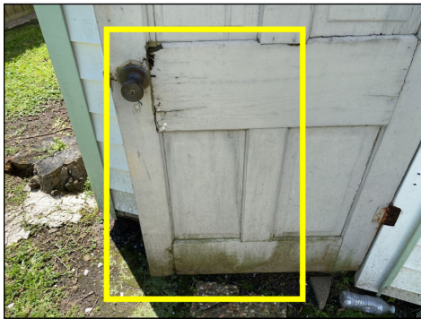
Rot/deterioration exterior closet door.
