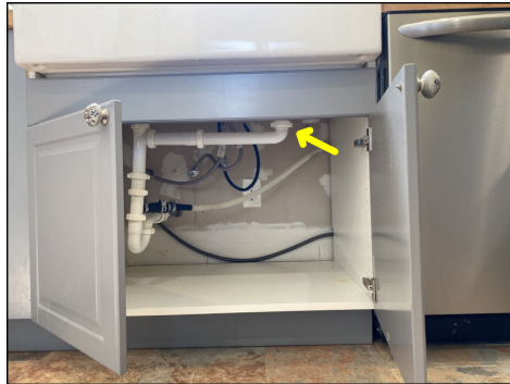
Drain leaks second floor kitchen sink.
