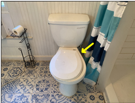
Loose commode seat first floor bathroom.
