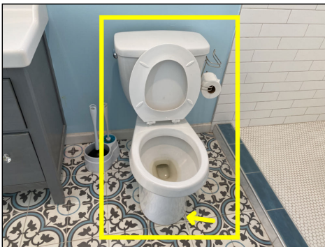
Loose commode/not sealed to floor second floor bathroom.
