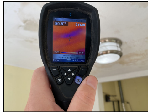
Thermal anomalies laundry room.
