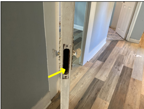
Missing hardware rear first floor bedroom door.
