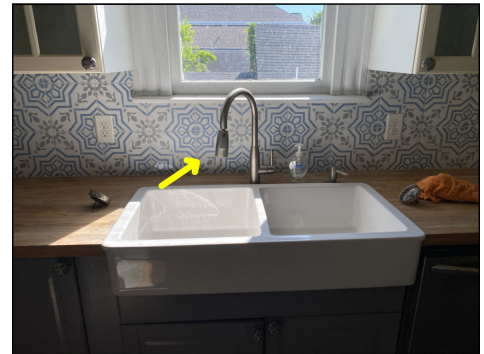
Faucet leak (slow drip) second floor kitchen sink.
