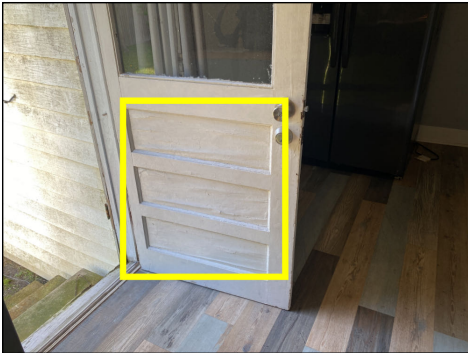
Deterioration first floor kitchen exterior door.
