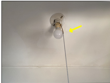
Missing protective light globe second floor bedroom closet.
