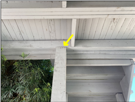
No structural strapping front deck.
