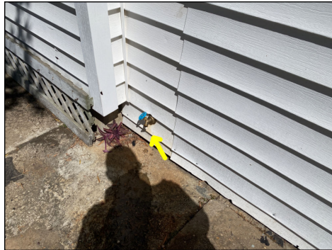
Missing anti backflow devices exterior hose bibs.
