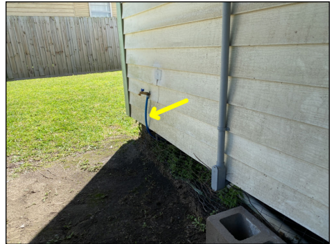
Exterior PEX piping not protected from freeze/UV deterioration.
