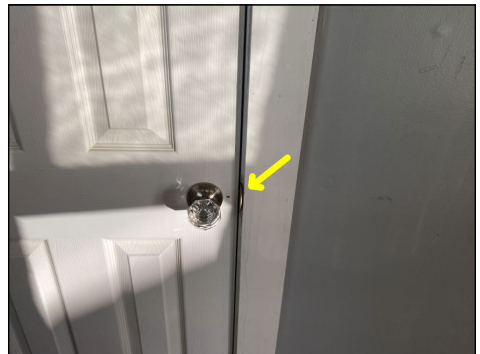
Damaged hardware first floor living room (latch will not turn).
