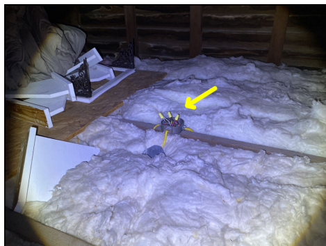
Open junction boxes attic (multiple).
