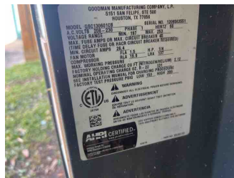
5 ton unit built in 2013, uses R22 coolant, min/max amps: 26.4-45
