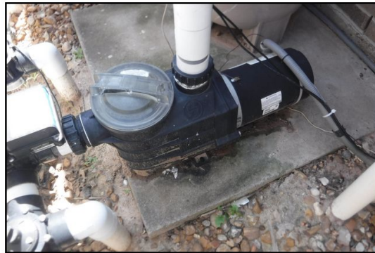
Pool filter pump
