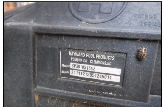
Filter pump data plate
