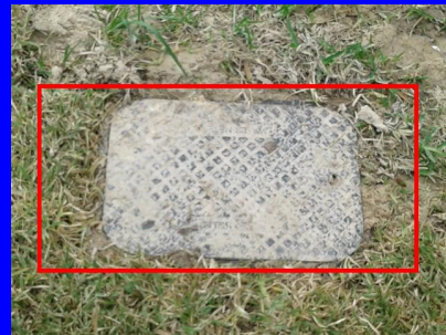
water meter front right of home
