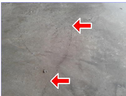
F. Item 1(Picture) multiple areas garage
