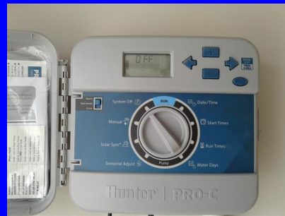
sprinkler system control panel inside garage
