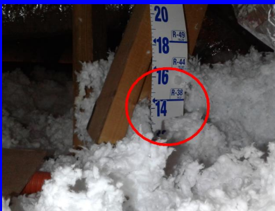
14 inches fiberglass blown insulation
