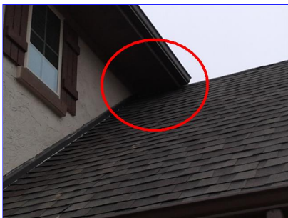
E. Item 4(Picture) multiple areas roof line
