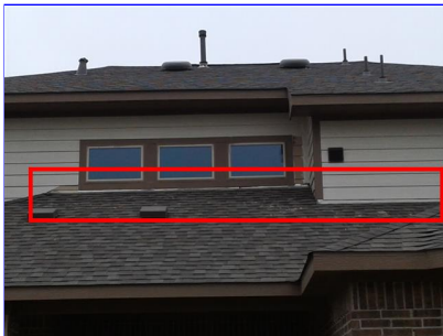
C. Item 3(Picture) multiple areas roof line
