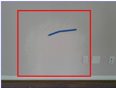
E. Item 1(Picture) multiple areas throughout home
