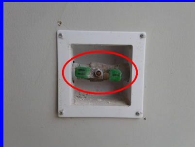
water shutoff inside garage
