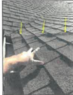
Rear, wave in roof decking
