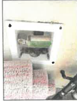
Garage, main water valve
