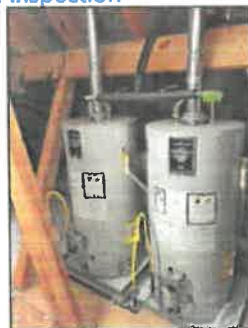
Attic, two Bradford White 40 gallon water heaters
