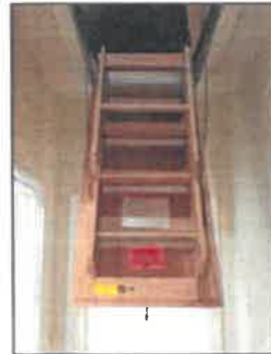
Attic ladder missing insulation
