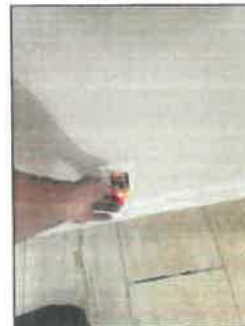
Living room, loose receptacle should be corrected
