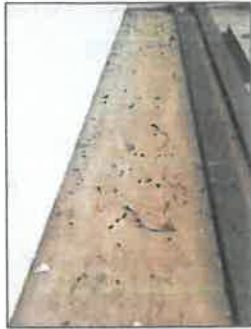
Garage, rodent droppings observed on floor
