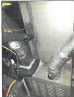
Attic, rear unit Carrier Evaporator: primary drain, p-trap, secondary drain
