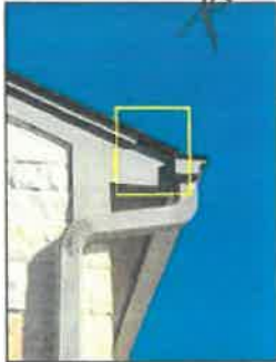
Left side, fascia board trim is damaged and should be repaired
