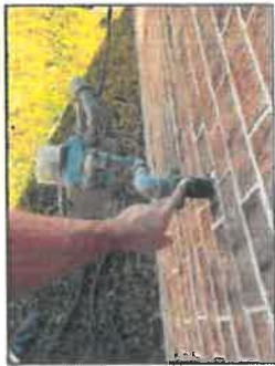
Gas supply line is bonded/grounded
