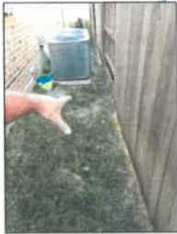
Right side, evidence of poor drainage via swale
