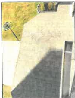
Front lower, overview / mechanical damage
