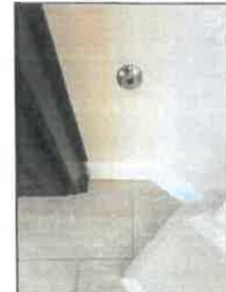
Left side, gas valve in wall
