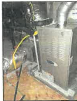
Attic rear unit, Carrier Furnace: gas valve, sediment trap, exhaust vent
