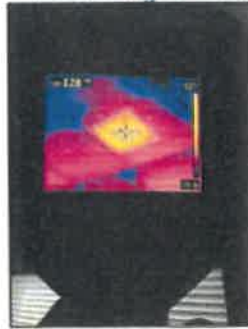
2nd floor heat is functional, 128°
