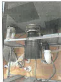
Badger disposal, functional, noisy/vibrating
