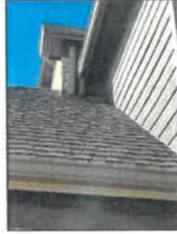
Some gutter downspouts terminate onto roof covering, may cause granule loss
