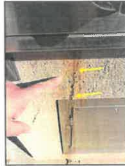
Outdoor grill structure, crack in stucco
