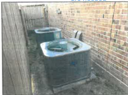
Right side, two Carrier condensers
