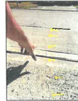
Driveway, crack recommend fill and monitor
