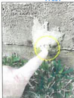
Right side, one or more exposed cable ends
