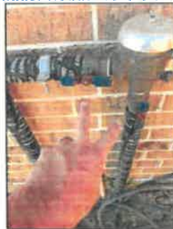
Handles on valves are rusting, recommend wire brush and paint
