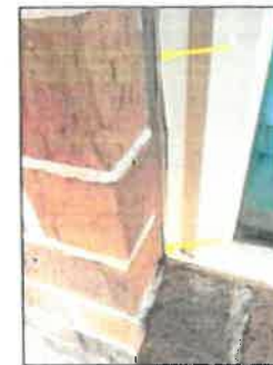
Rear patio, windows need caulking improvements
