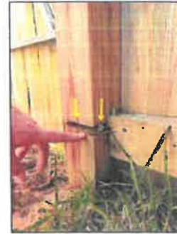
Gate post is damaged and should be corrected
