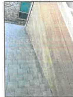
Rear upper, funagl growth observed on exterior of structure should be pressure washed
