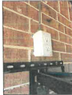
Under current standards; exterior GFCI protected receptacles require a weatherproof bubble type cover
