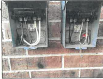
White conductors not marked as hot in condenser disconnect boxes
