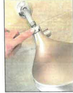
Primary bathroom, cosmetic damage to shower head
