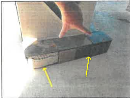
Outdoor grill structure, loose / missing tiles
