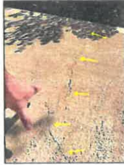
Front porch, hairline cracks recommend monitor
