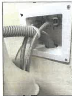
Washer supply and drain lines
