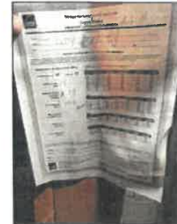
R38, minimum settled thickness of Blown-in insulation should be 13.25"
