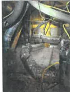
Ducts appear to be properly hung and seperated
