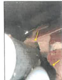
Right side, refrigerant line entry should be properly sealed (mortar or foam)
