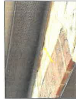
Front, void between cornice trim and stone
