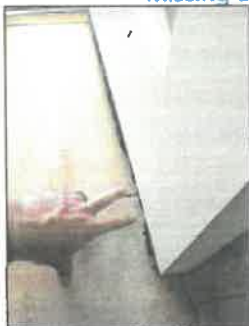
Door to garage, damaged bottom sweep and no self closing device
