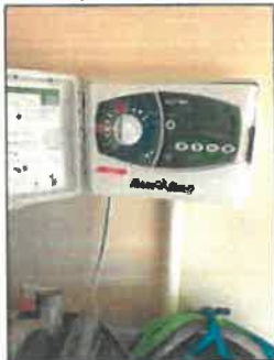
Garage, Rain-Bird ESP-Me controller
