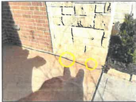
Front porch, stone missing weep holes
