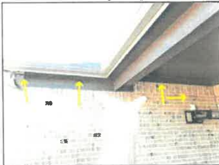
Exposed romex type wiring was noted and should be encased in steel pipe or PVC conduit raceway
