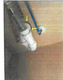
Holes in the back of cabinets for plumbing lines should be fully sealed
