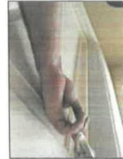
Half bath, door bowed or not aligned with frame / need to apply pressure to latch
