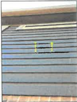
Right side, one or more cement boards observed to be loose or lifted and should be repaired
