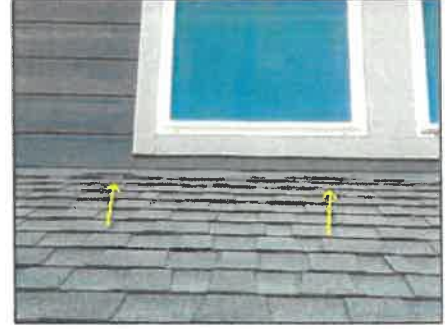
Rear, headwall flashing slightly lifted recommend having re-seated and sealed
