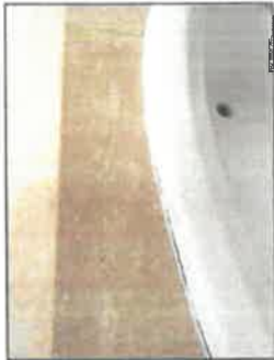
Primary bathroom, tub deck need caulking improvements
