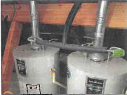
Cold water valves, supply lines, vent hoods, exhaust vents
