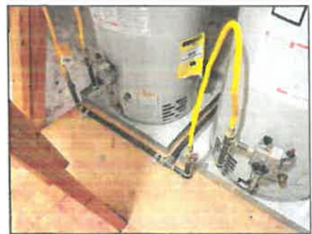
Gas valves, sediment traps, heat controls
