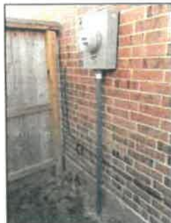
Right side, meter / no intersystem bonding bridge
