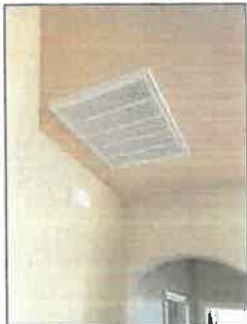
2nd floor, humming noise noted when HVAC was functioning
