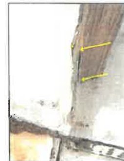
Garage trim, recommend caulking improvements
