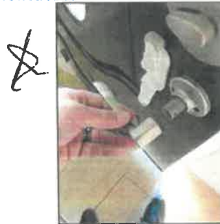
Front door, handle is damaged / missing set screw
