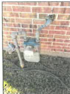
Right side, gas meter
