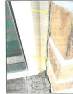
Rear, window needs caulking improvements
