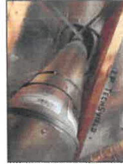
Exhaust vent through roof penetration
