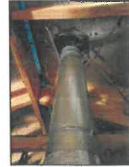
Exhaust vent through roof penetration
