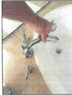
Primary bathroom, tub spout is loose and should be tightened
