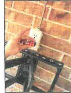
Rear patio, not GFCI protected
