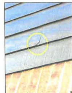
Right side, mechanical damage to cement board
