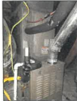
Attic, front unit Carrier Evaporator: primary drain, p-trap, secondary drain
