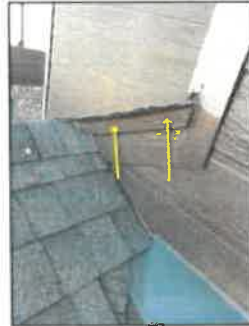
Rear rake, no drip edge flashing
