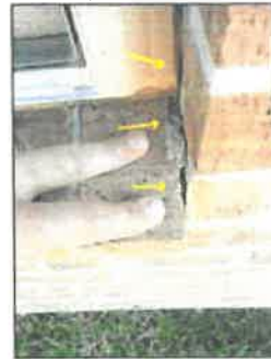
Rear, corners of brick window sill needs mortar pointing
