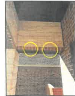
Front porch, missing weep holes
