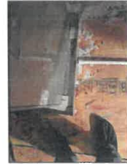
Pan and drain line, no float switch
