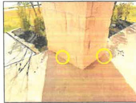
Front column, missing weep holes
