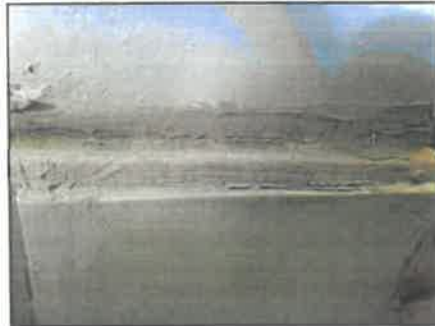
Cracks in mastic, improvements are needed
