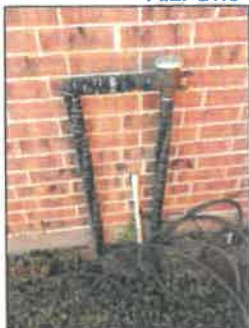
Right side, high loop / backflow preventer
