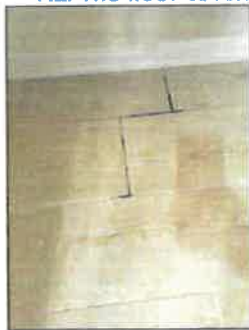
Primary bathroom closet, stains observed in grout
