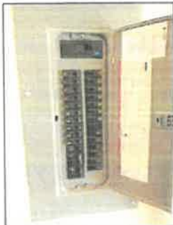
Garage, Square D panel: 125A, labeled, ARC fault breakers observed
