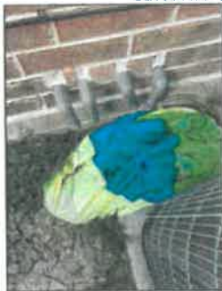
Right side, termination point of drain lines
