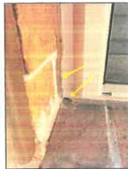
Front, window needs caulking improvements
