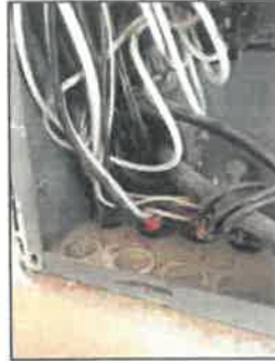
Bonding bushing observed on knockout for main service line entry
