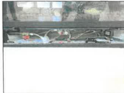
Under unit, gas valve and battery backup box for igniter
