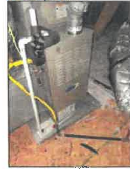
Attic front unit, Carrier Furnace: gas valve, sediment trap, exhaust vent
