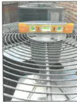
Both condensers are not level
