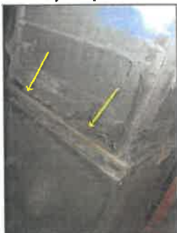
Cracks in mastic, improvements and needed
