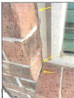
Front, window needs caulk and corner of sill needs mortar pointing
