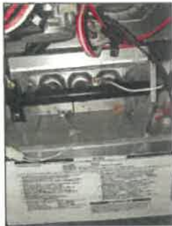
Burner / heat exchanger
