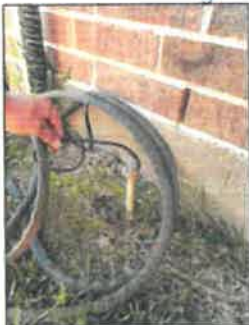
Right side, ground conductor, ground rod, clamp
