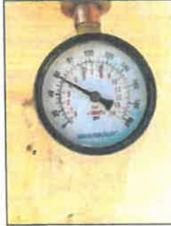
Static water pressure 60PSI
