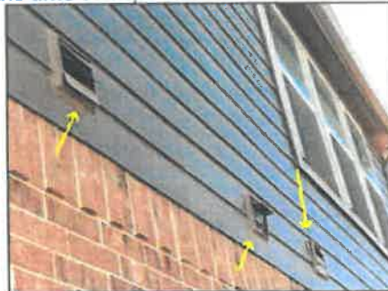
Right side, vent covers need to be repaired and/or re-secured
