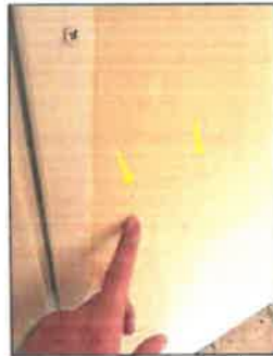
Garage, minor stress crack observed
