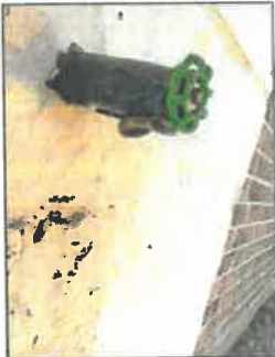
Right side, missing backflow preventer
