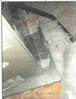
Pan and drain line, no float switch
