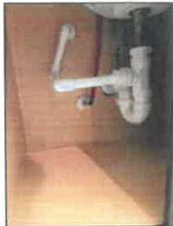
Primary drain line to sink(s) drains appears to be glued pipe
