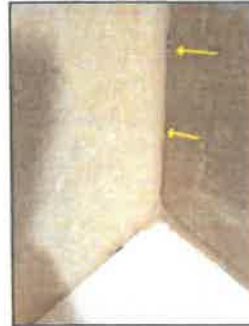
2nd floor left side bathroom, needs grout and/or caulking improvements
