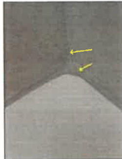
J&J bath, needs grout and/or caulking improvements
