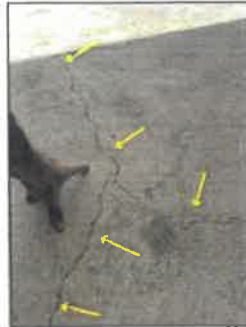
Garage, hairline cracking observed recommend monitor
