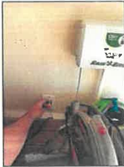
Garage, note that more than one receptacle not GFCI protected
