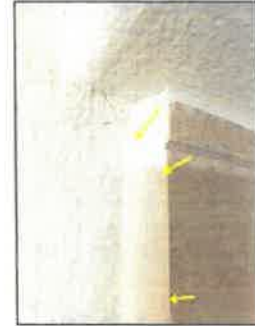
2nd floor left side bathroom, some minor cracks around outside of tile wall
