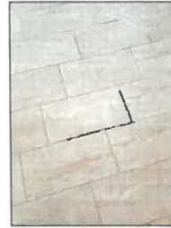
Living room, stains in grout
