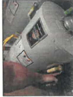
TPR valves and drain lines
