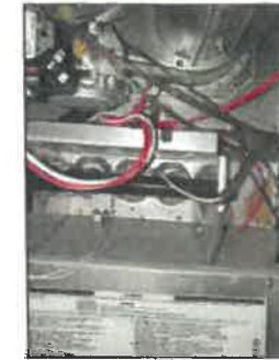
Burner / heat exchanger
