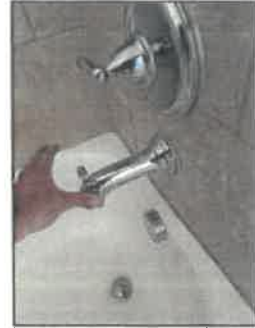
2nd floor bathrooms, tub spout are loose and should be corrected
