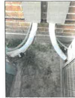
Refrigerant line insulation
