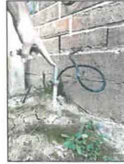
Ground rod(s) sticking out excessively
