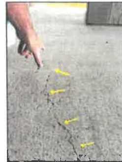
Rear covered patio, hairline crack recommend monitor
