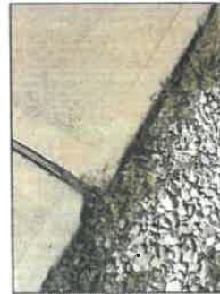
Driveway, minor damage to edge recommend repair
