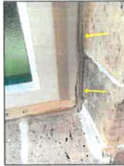
Right side, window needs caulking improvements
