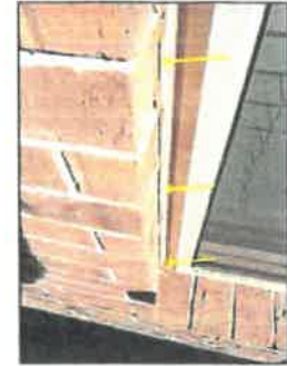
Left side, window needs caulking improvements
