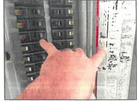
Garbage disposal and dishwasher are on the same circuit breaker (20A)
