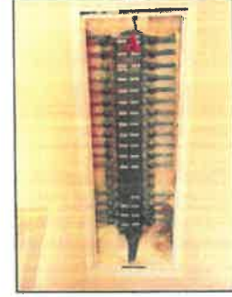
Garage, Pex manifold system
