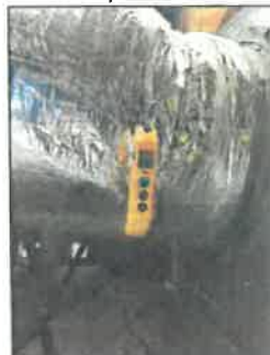
Measuring tool pierced through duct was left in place. Recommend removing and sealing hole duct
