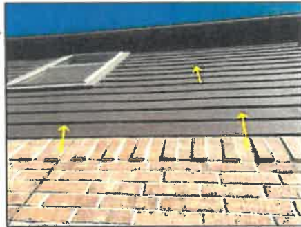
Left side, one or more cement boards observed to be loose or lifted and should be repaired
