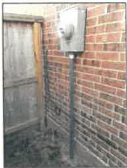
Right side, meter / no intersystem bonding bridge
