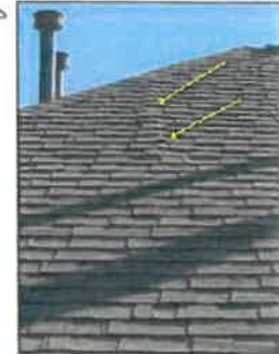
Rear, wave in roof decking
