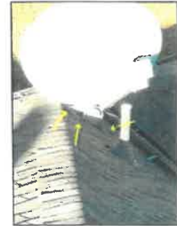
Right side, satellite mounting bolts are prone to leak and should be monitored/maintained with sealant
