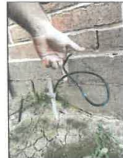
Right side, grounding conductor #2, ground rod, clamp
