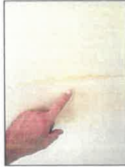
Garage, water stains observed / dry at the time of inspection
