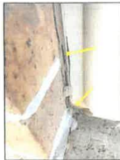
Rear, window needs caulking improvements
