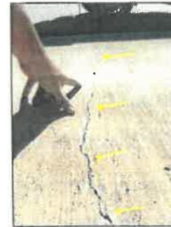
Sidewalk, crack recommend fill and monitor
