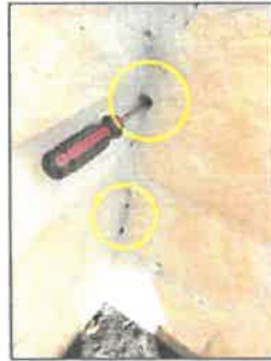
Front column, needs mortar pointing
