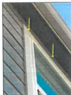
Right side, no Z-flashing observed above windows
