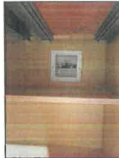
Lower cabinet, gas valve in wall
