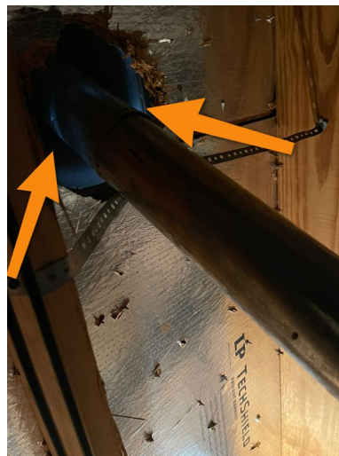
Water heater vent pipe
