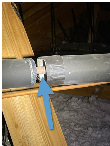
At the unit in the attic
