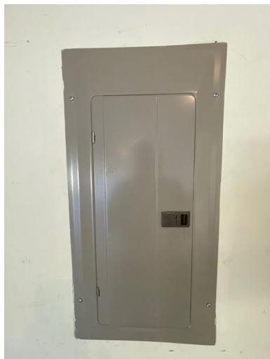
Amperage rating for main service disconnect: 125 Amps
