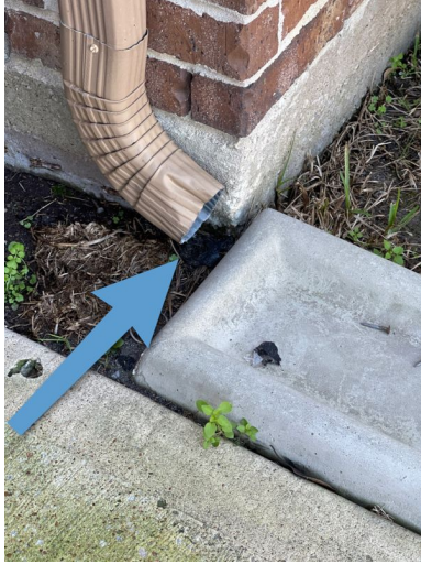
Splash block is not properly installed at the front entrance of the home to divert water away from home
