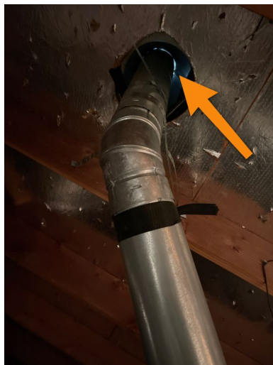
Furnace vent pipe
