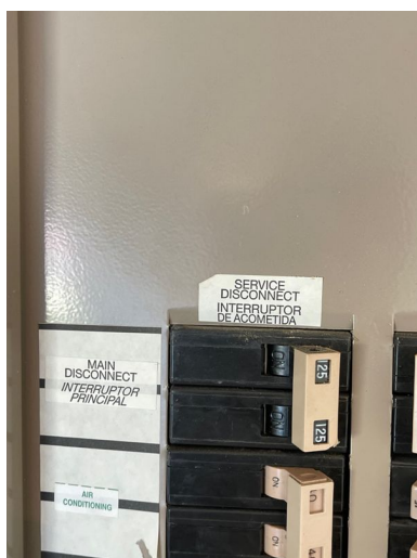
Type of Feeder Wires found in main and sub panels: Aluminum
