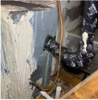
Evaporator Coil (1/6) 11/22/2022 12:46 PM
