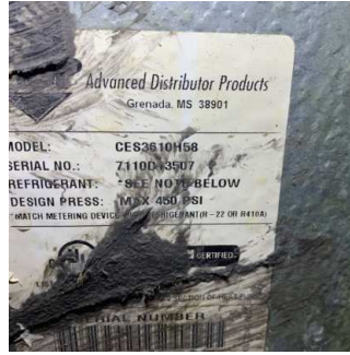
Evaporator Coil (3/6) 11/22/2022 12:46 PM
