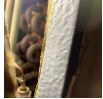
Evaporator Coil (4/6) 11/22/2022 12:49 PM
