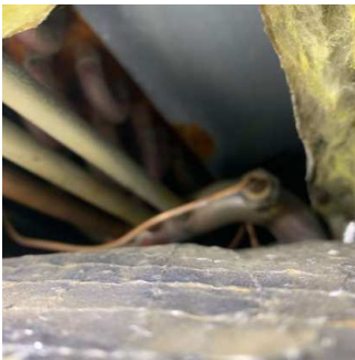
Evaporator Coil (5/6) 11/22/2022 12:49 PM
