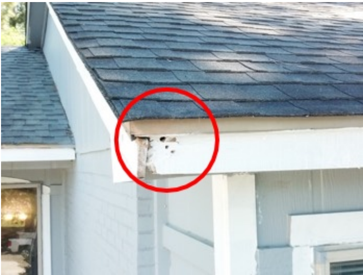
Damaged fascia board
