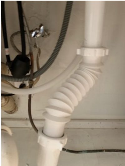
Flexible drain pipe present, drain tail piece pipes are required to have smooth interiors to prevent blockage.
