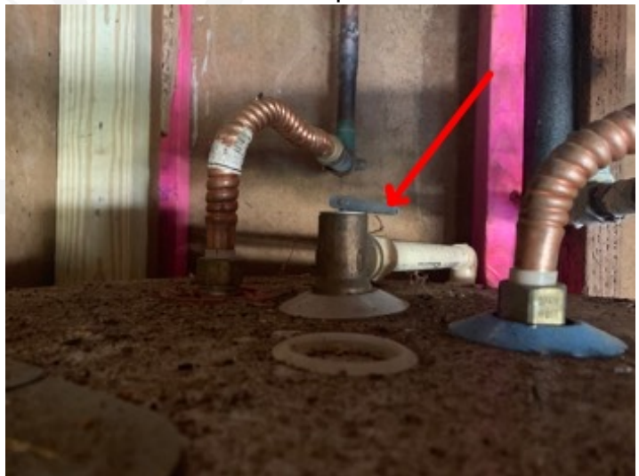
Temperature pressure relief valve
