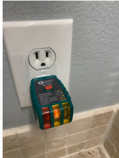
Electrical outlet wired with an open ground
