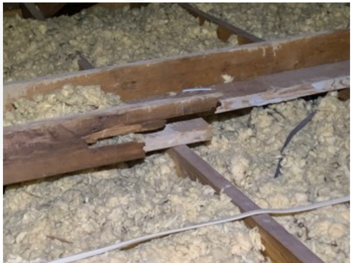
Split/Broken framing boards observed.
