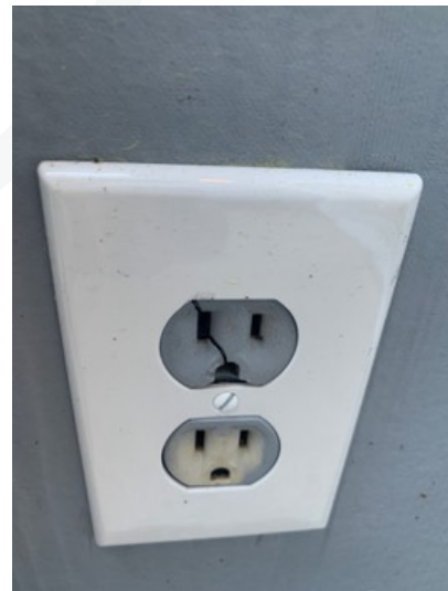
External electrical outlets are missing its waterproof covering
