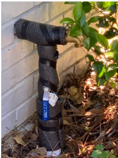
Main water shut off valve
