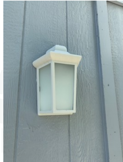
Light fixture not working properly, may have a short or may be in need of light bulb replacement.
