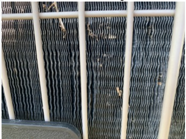
Air-conditioning unit condenser coil fins are damaged, recommend an HVAC technician to repair by combing the fins.
