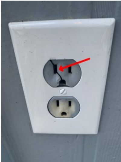
Exterior electrical outlet top receptacle is damaged.
