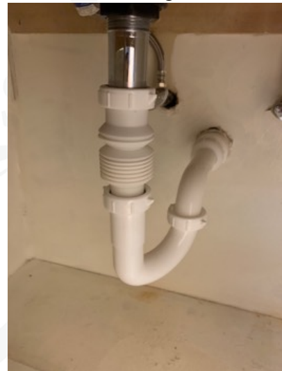
Flexible drain pipe present, drain tail piece pipes are required to have smooth interiors to prevent blockage.
