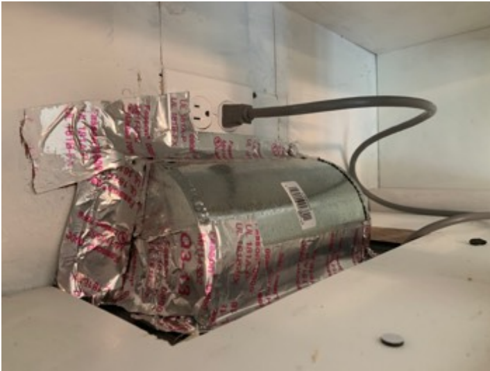
Self filtering with vent to the exterior
