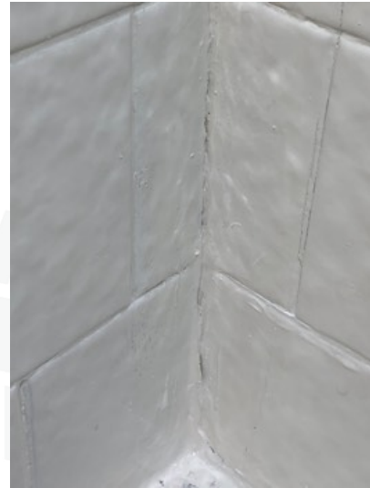
Missing or deteriorated grout lines around the guest bathroom tub area , this can allow water to penetrate behind the tiles and damage walls and or floor areas.
