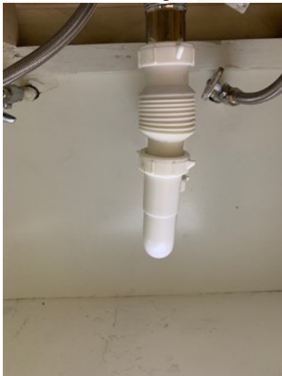
Flexible drain pipe present, drain tail piece pipes are required to have smooth interiors to prevent blockage.
