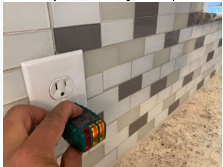
Electrical outlets within 6 feet of the kitchen sink are not GFCI protected
