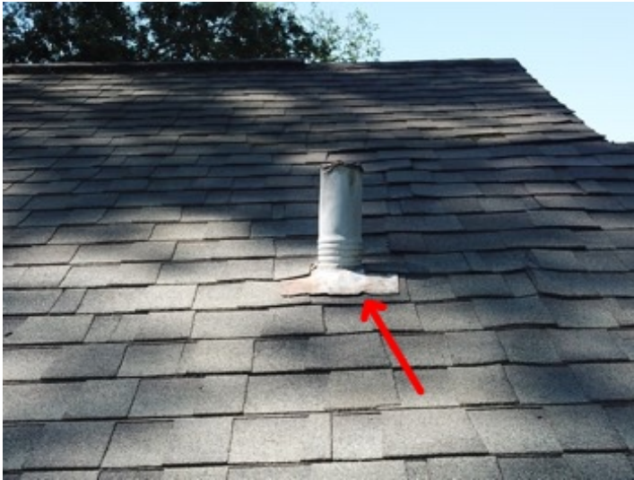
Roof jack flashing is lifting
