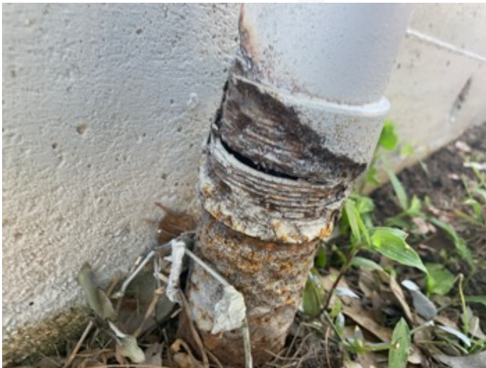
Rusted union at the base of the service entry conduit.
