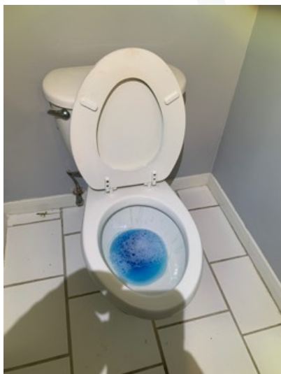
The toilet in the downstairs guest bathroom is loose, may need a wax seal replacement and it does need to be properly secured to the floor
