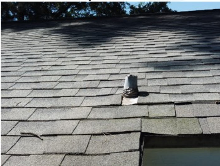
Plumbing vent penetration does not meet it's required 6 inch height
