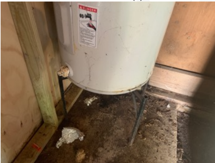
water heater is missing drain pan at the bottom of the water heater.
