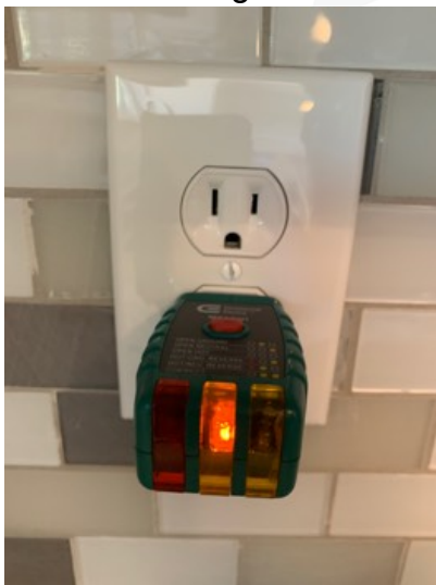
Electrical outlet wired with an open ground
