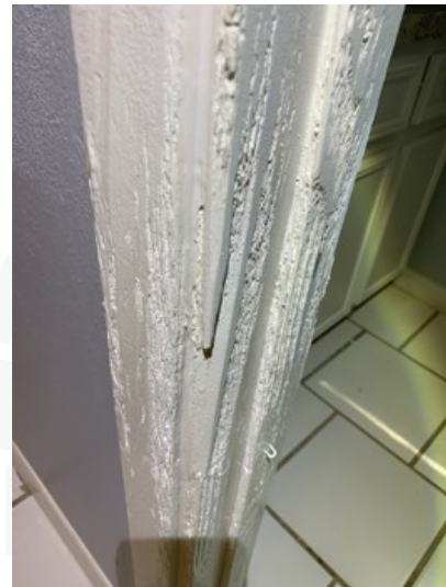
Bathroom door jamb has been repaired with a less the workmen like quality
