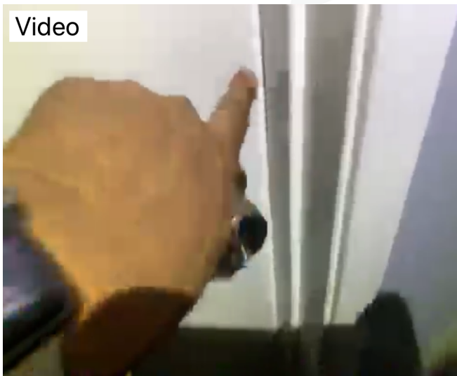
Master bedroom closet door did not latch properly, may be in need of striker plate adjustment.
