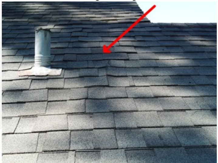
Shingles lifting, shingles are lacking the proper amount of adhesive to keep the roof integrity intact causing shingles to lift, because of this, the shingles could be damaged by high winds at some point.
