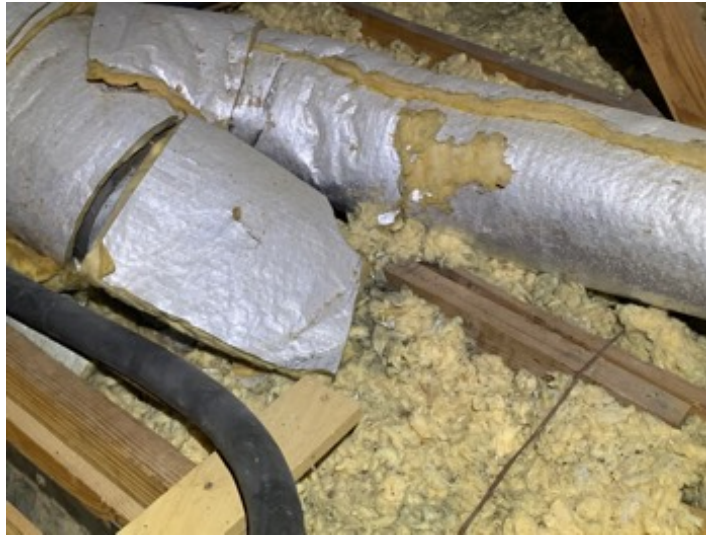
Ductwork is making contact with attic insulation. Condensation from the ductwork could damage insulation and ceiling drywall.
