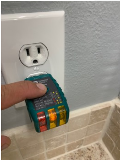
Electrical outlets within 6 feet of the master bathroom sink(s) are not GFCI protected.
