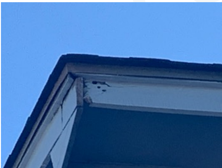
Damaged fascia board
