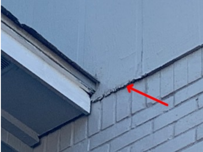
Exterior siding is deteriorated
