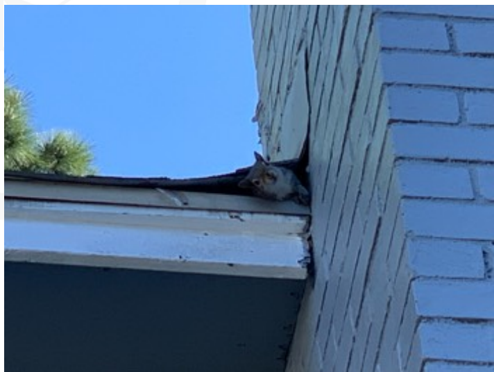
Flashing is lifting
