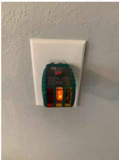
Electrical outlet wired with an open ground
