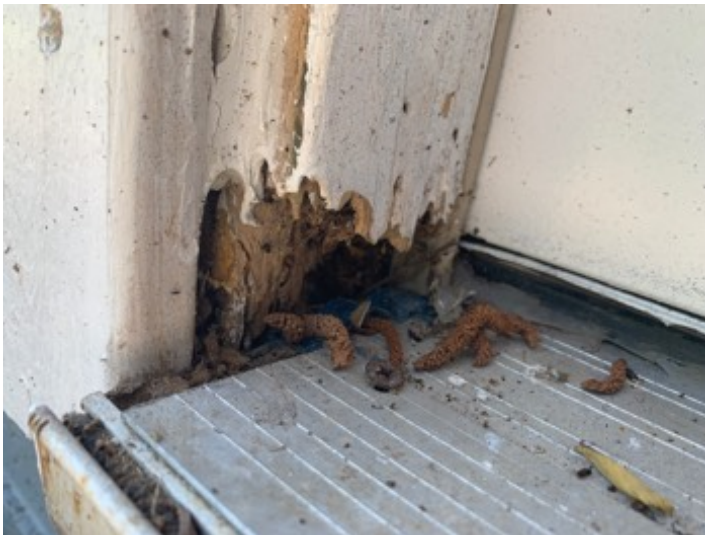
Damaged door frame at the rear exterior of the house
