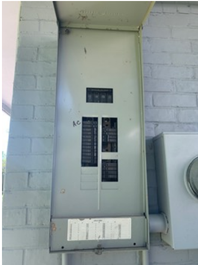
Electrical Service Panel
