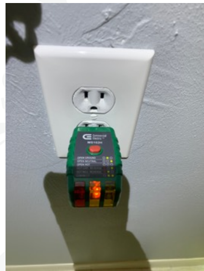
Electrical outlet wired with an open ground
