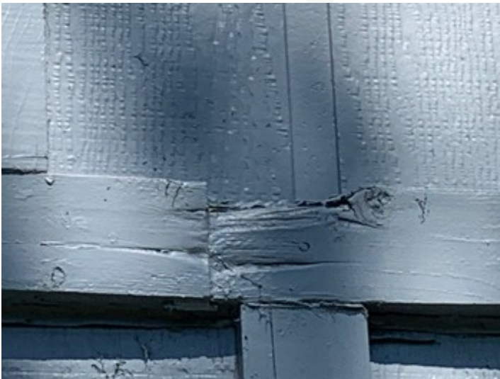
Exterior siding is deteriorated
