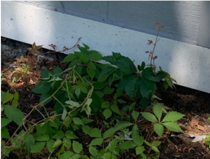
Earth to wood contact on the exterior siding
