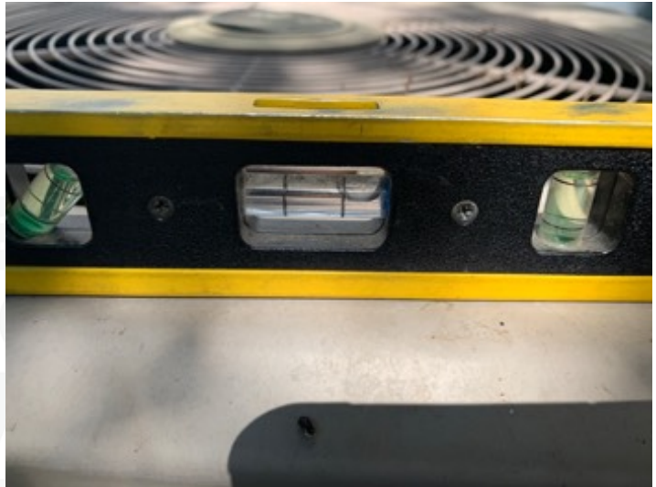
AC does sit not level, this can affect the movement of coolant through the lines.
