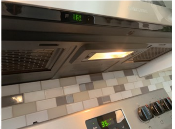
Missing grease trap
