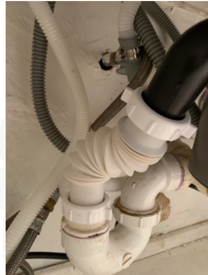
Flexible drain pipe present, drain tail piece pipes are required to have smooth interiors to prevent blockage.
