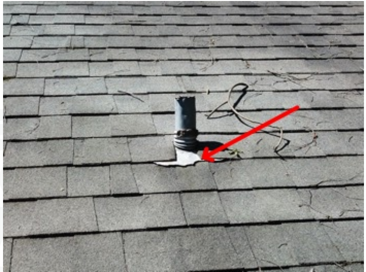
Damaged roof jack flashing
