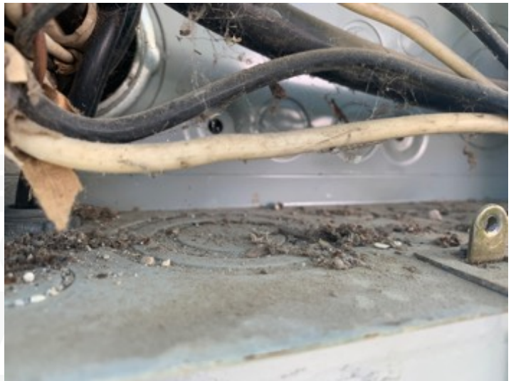
Debris/dust from drywall in the bottom of the electrical service panel. Can be considered a fire hazard at some point.
