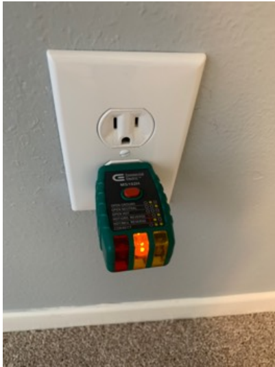
Electrical outlet wired with an open ground
