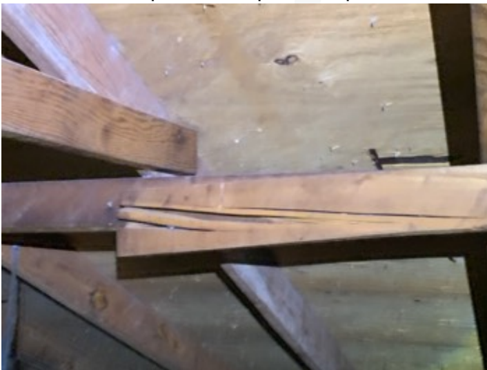
Split/Broken framing boards observed.
