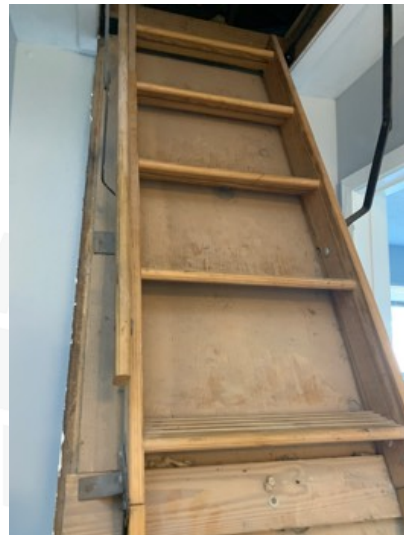
Missing insulation on the attic access door.
