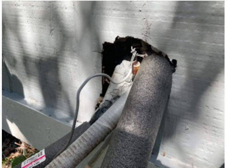
Wall penetrations for the A/C unit entering into the wall is not properly flashed.
