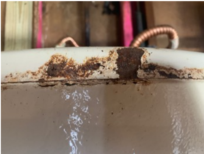
Rust is visible on the casing
