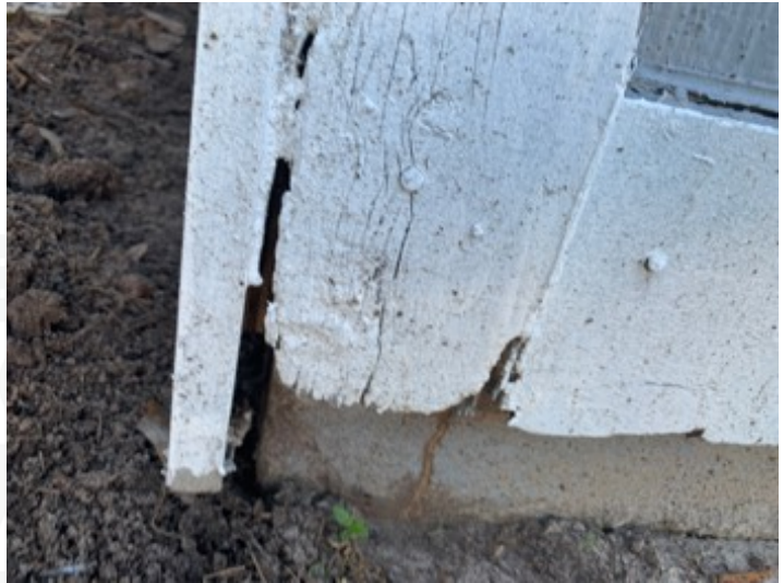
Exterior siding is deteriorated
