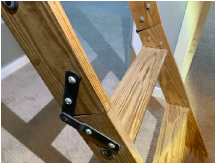
Attic Ladder appears damaged may not be able to handle the weight of both a person and appliance moving up and down the ladder. Recommend an evaluation possible repair or replacement
