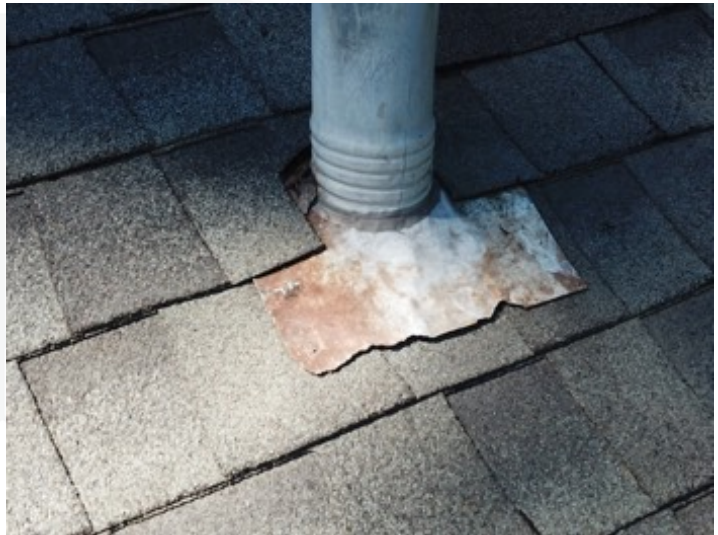
Damaged roof jack flashing
