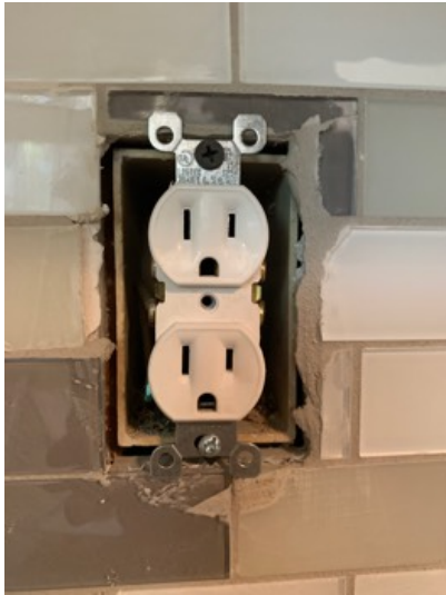
Missing box extender for electrical outlet in the kitchen area.
