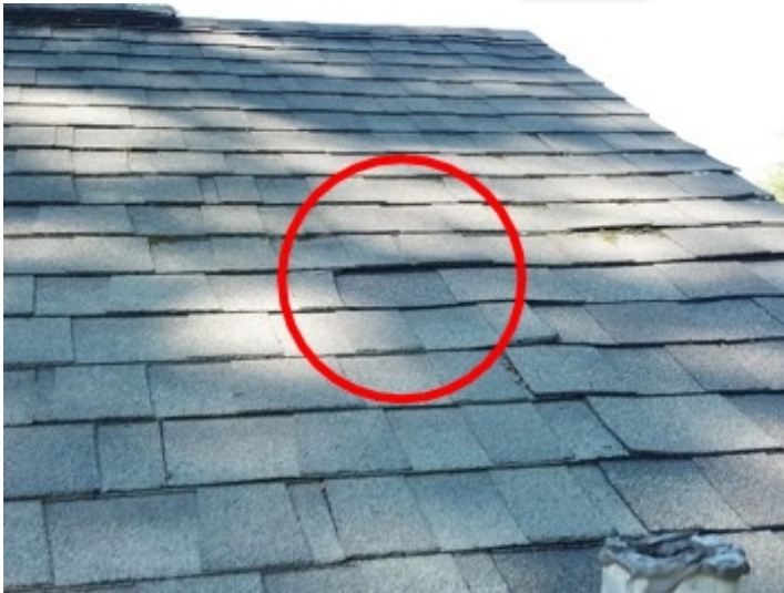
Shingles lifting, shingles are lacking the proper amount of adhesive to keep the roof integrity intact causing shingles to lift, because of this, the shingles could be damaged by high winds at some point.
