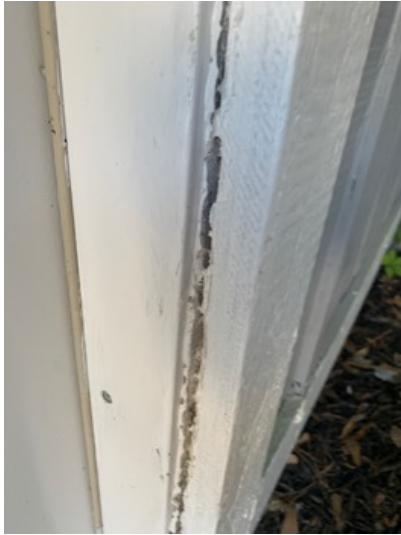
Missing or deteriorated caulking in between joints in the siding(exterior)
