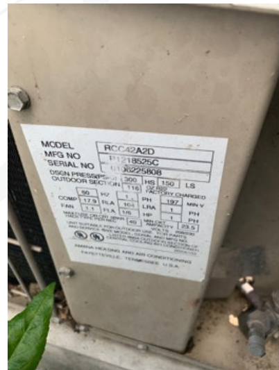
AC Unit Specifications
