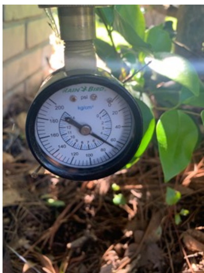
Static Water Pressure Reading: 65 PSI
