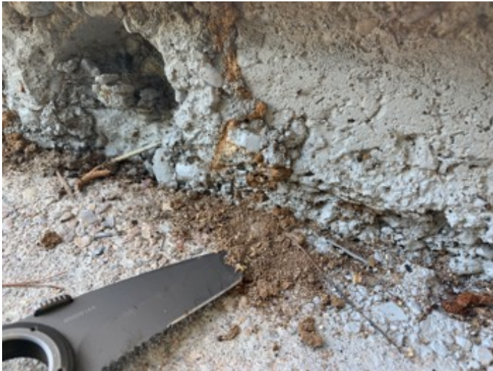
Wood destroying insects found present at the exterior of the structure by professionals from Scientific Exterminators Of Texas.
