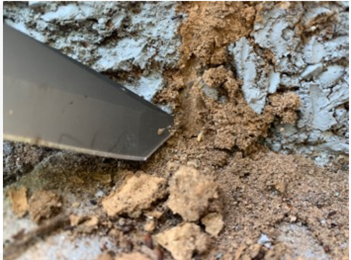
Wood destroying insects found present at the exterior of the structure by professionals from Scientific Exterminators Of Texas.
