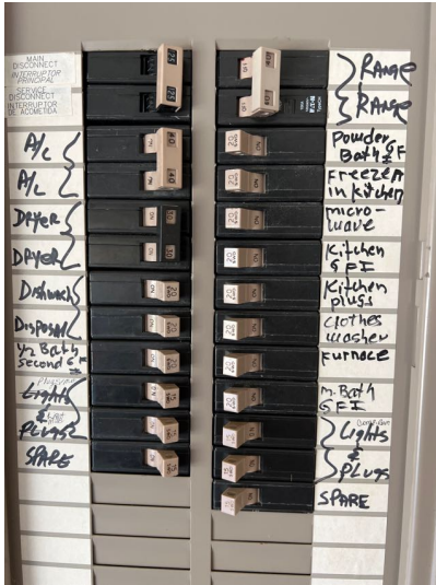
Picture of breakers
