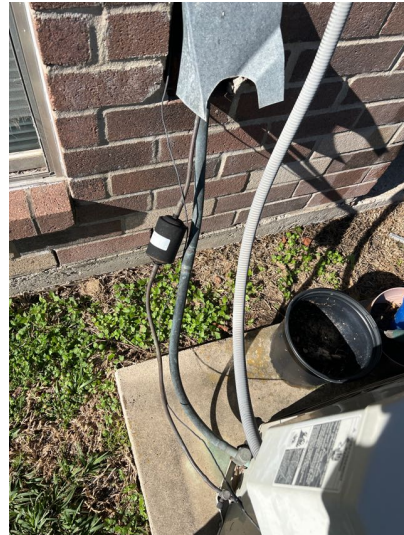
Damaged / missing insulation on freon line at AC condensing unit.
