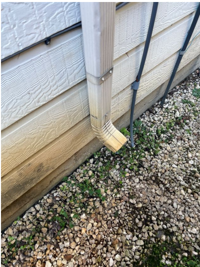
Gutter downspout discharging too close to the foundation.
