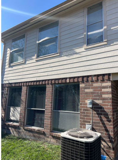
Damaged window screens
