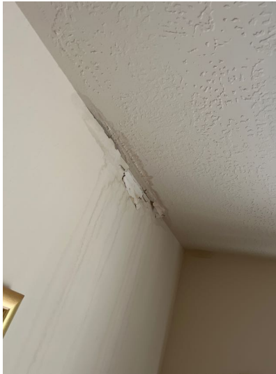
Moisture stain on ceiling.
