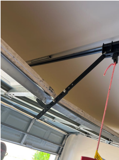
One or more of the garage door panels were observed to be damaged, weathered, warped and/or dented at the time of the inspection.
