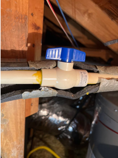
CPCV water piping
