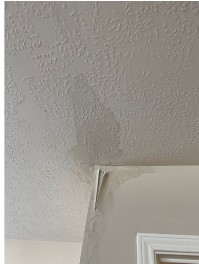
Moisture stain on ceiling.
