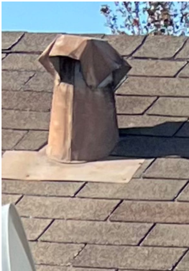
Unapproved roofjack used for dryer vent pipe.
