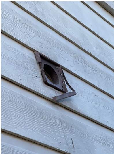
Bathroom exhaust fan noted with damaged termination cover
