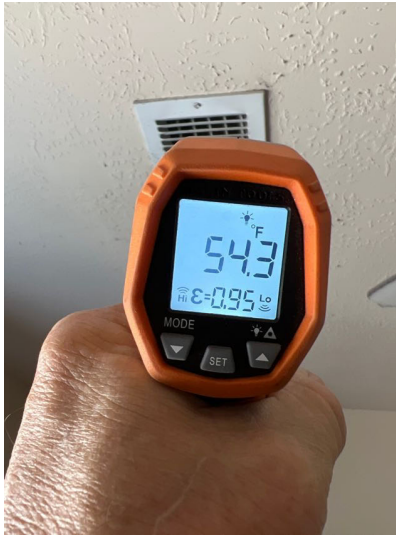
Air temperature measured at supply air vent.
