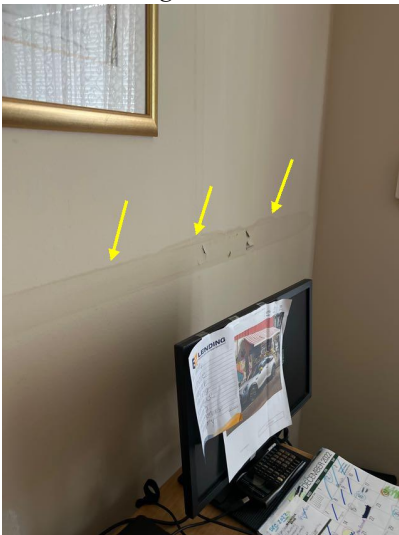
Moisture stains noted on wall in upstairs back left bedroom.
