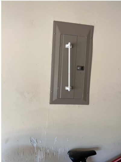
Picture of electrical service panel.
