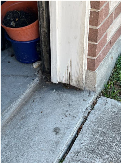
Damaged door trim.
