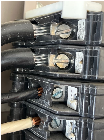
Aluminum service conductors missing anti-oxident grease.
