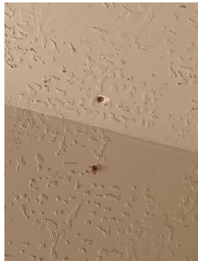
Nail pops or nails that have backed out were observed in one or more areas of the ceiling.
