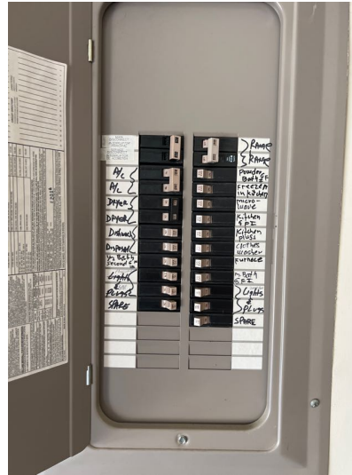
Picture of electrical service panel.
