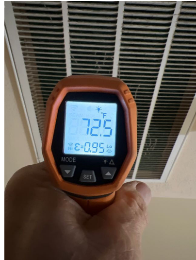
Air temperature measured at return air vent.
