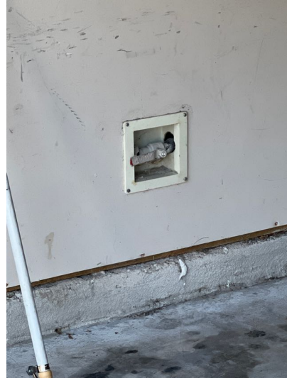
Water shut off valve
