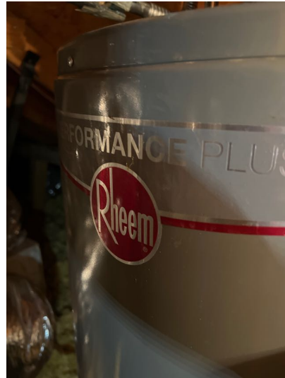
Water heater brand name
