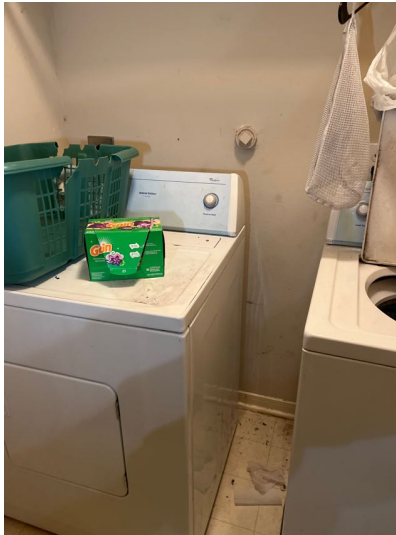
Electric and gas dryer connections present.
