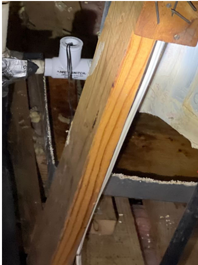
The AC Unit evaporator coil was noted defective due to water in secondary condensate containment pan.
