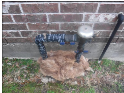
Irrigation back flow preventer located left side of residence.
