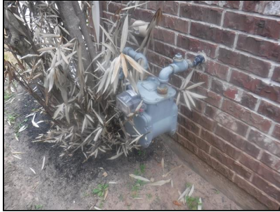
Gas meter located right side of residence.
