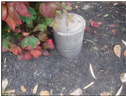
Cleanout located front of residence.
