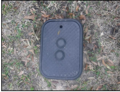
Water meter located left front of residence.
