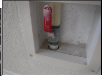
Main water bshut off located within the garage.
