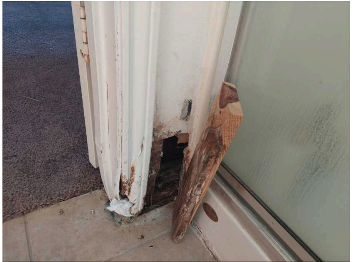
Interior wall damage, master bathroom
