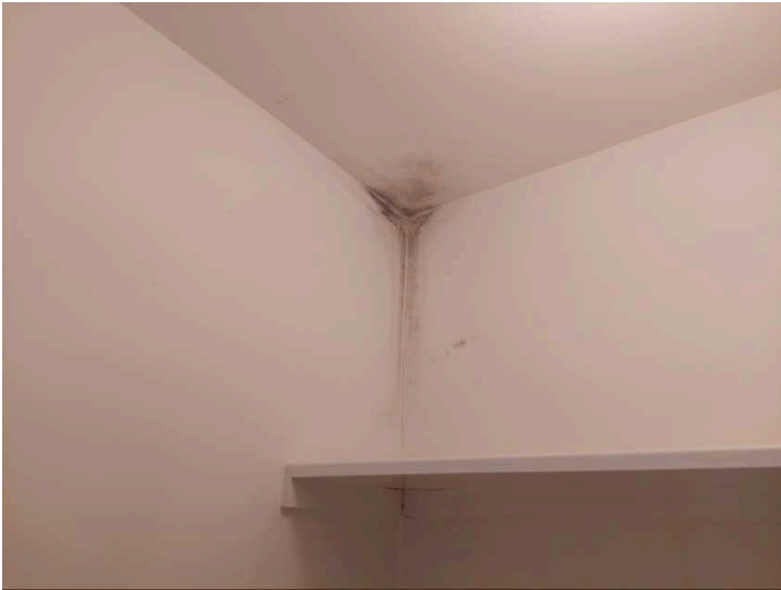
Evidence of moisture entering structure from interior water stains, upstairs closet
