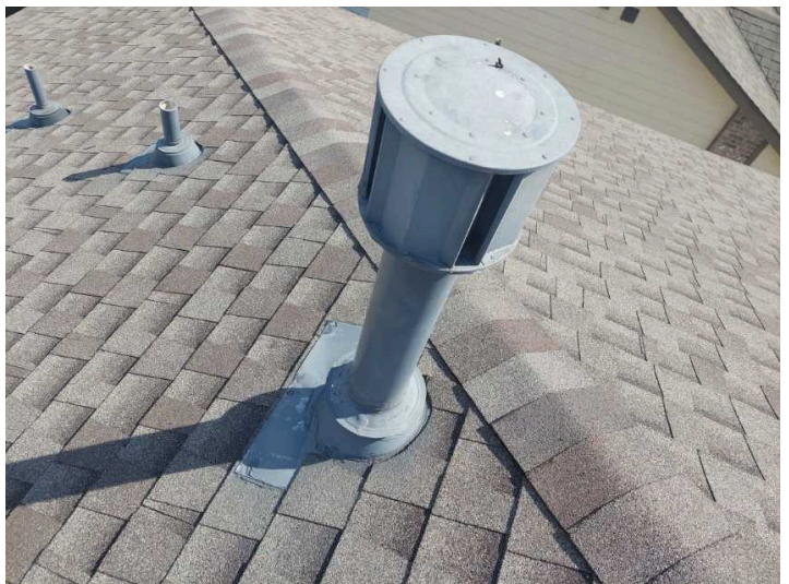
Gas furnace exhaust vent
