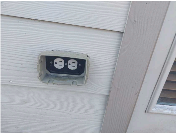
Exterior GFCI protected receptacles require a weatherproof bubble type cover
