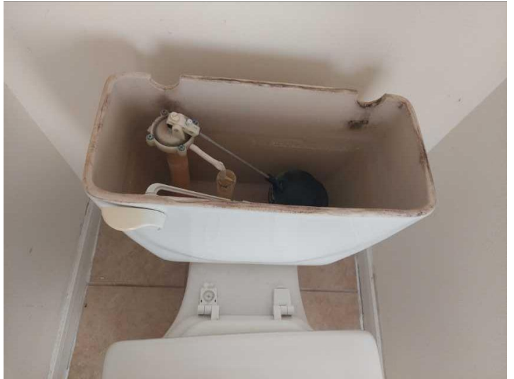
Master bathroom toilet does not flush
