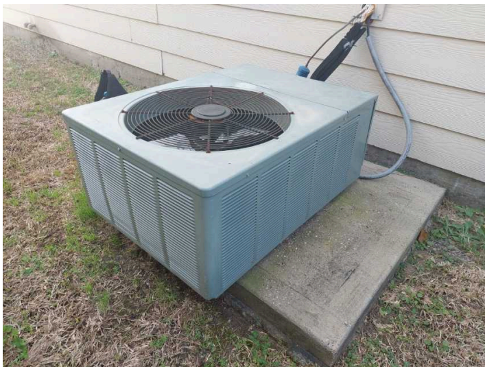
AC condensing unit
