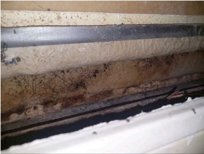
Possible master bathroom shower pan leakage has caused damage to walls
