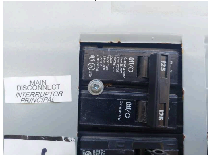
Main breaker (125A)
