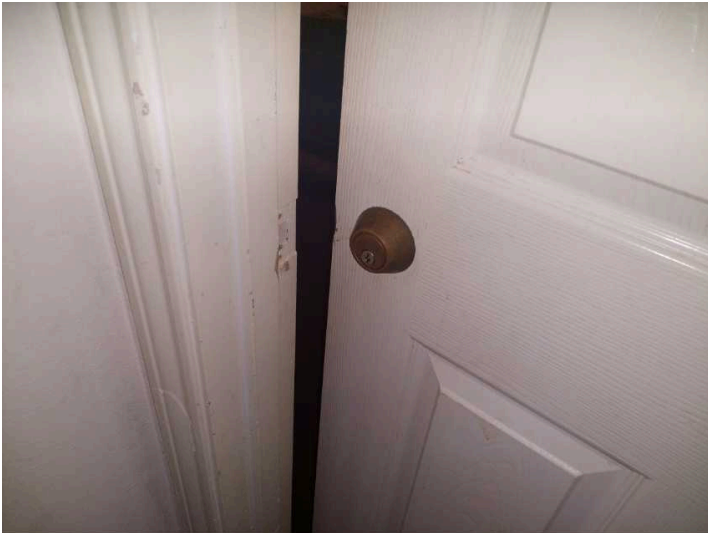
Missing doorknob for downstairs bedroom
