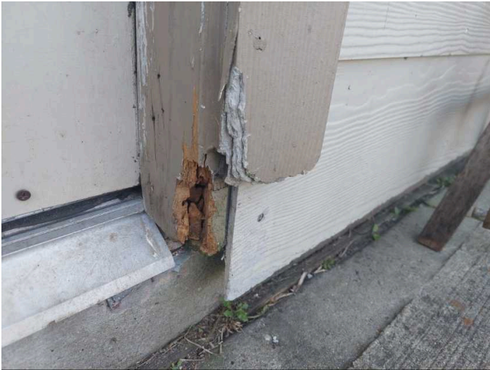
Damaged siding/door frame back side of house
