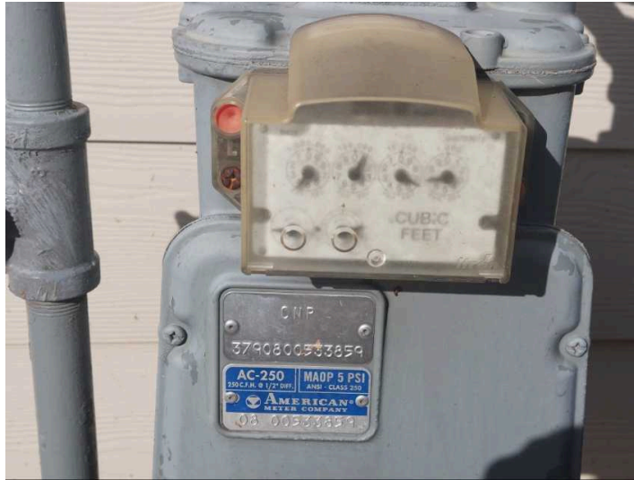
Picture of Gas Meter
