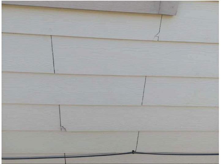
Damaged siding left side of house.
