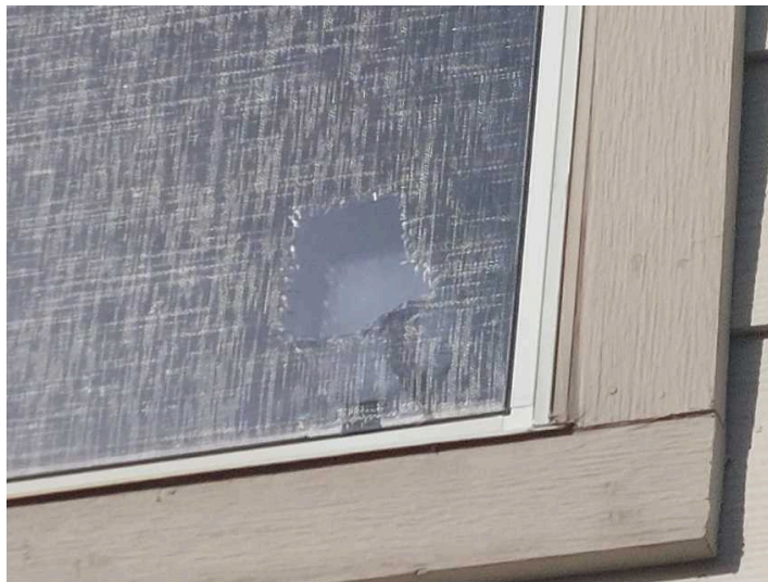
Damaged window screen
