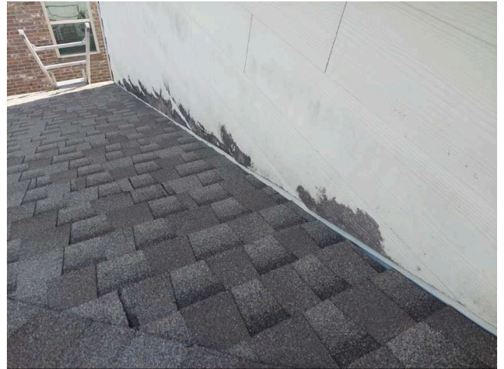
Damaged siding back side of house.
