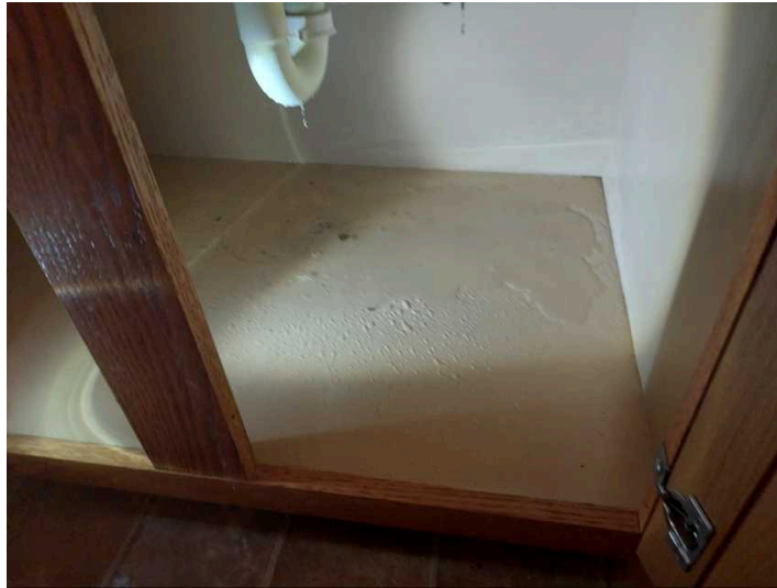
Hall bathroom vanity drain piping noted with water leak.
