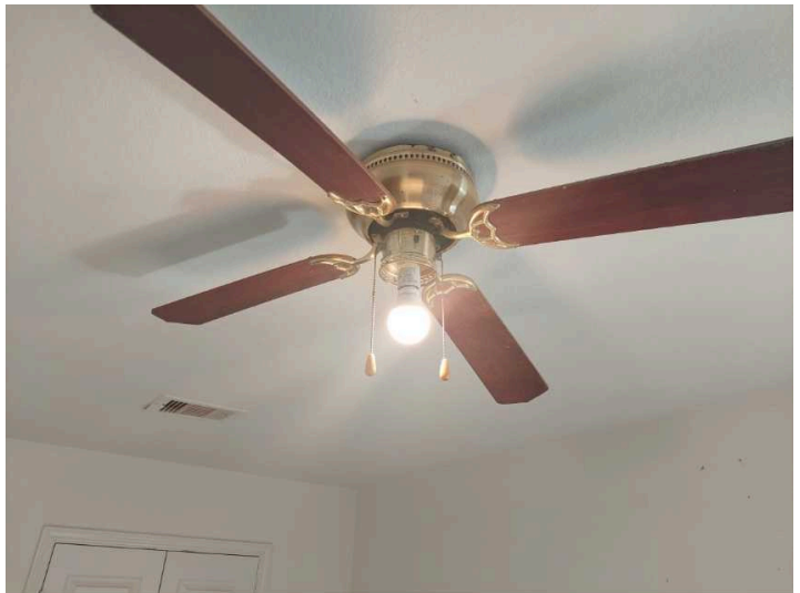
Ceiling light missing protective globe
