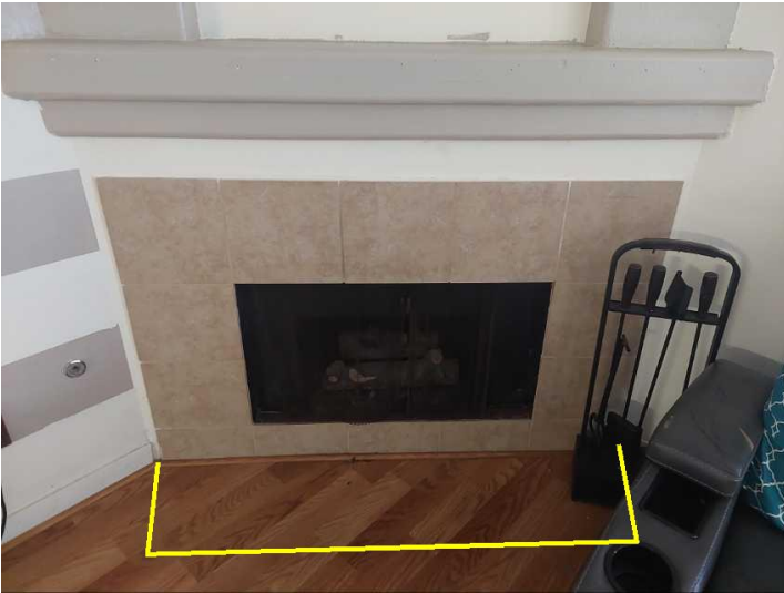
Fireplace missing a defined, noncombustible hearth extension.
