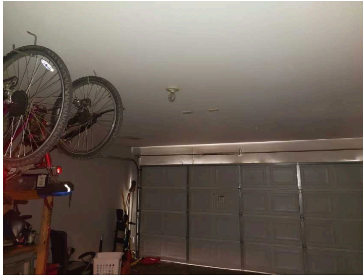
Garage door operator not installed
