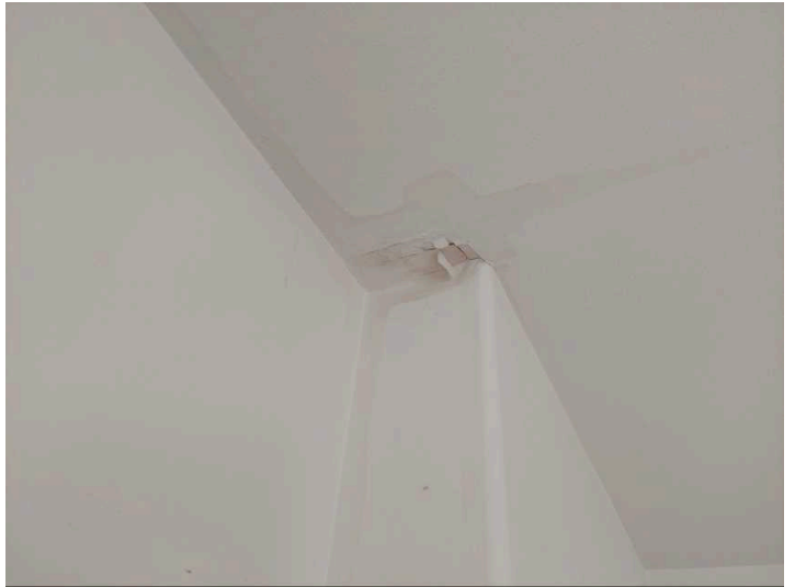
Moisture stain on ceiling, upstairs bedroom
