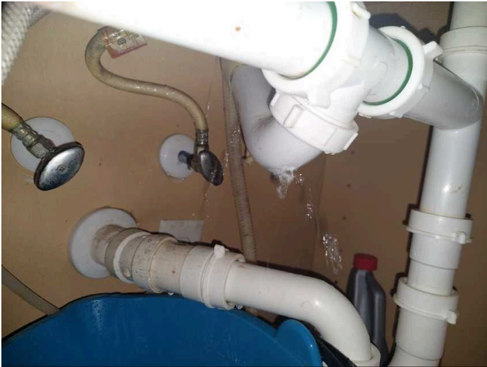
Kitchen sink drain piping noted with water leak.
