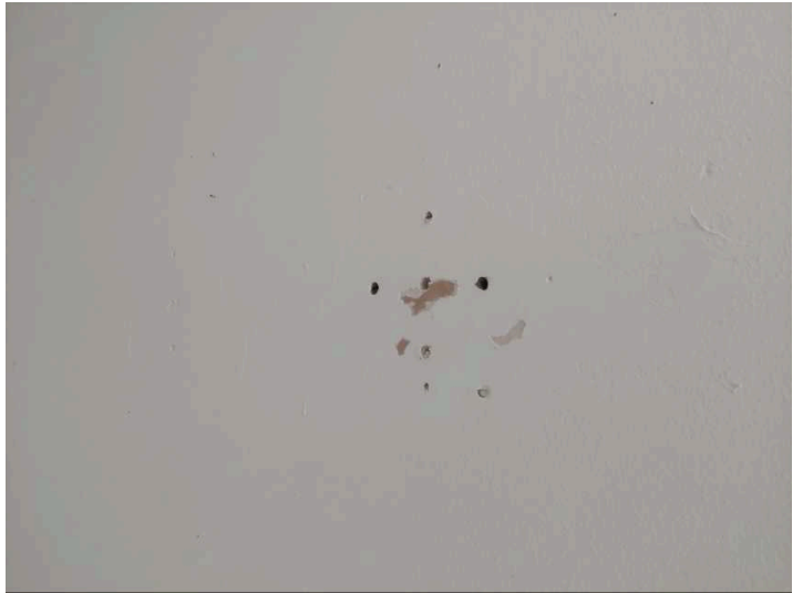
Interior wall damage in bedroom
