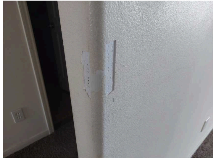
Interior wall damage
