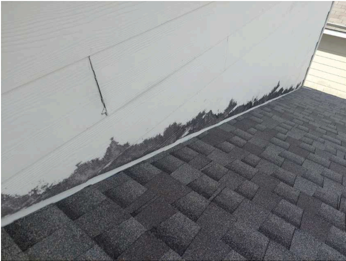
Damaged siding back side of house.
