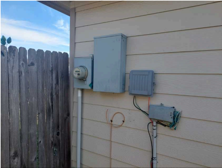
Picture of electrical service panel
