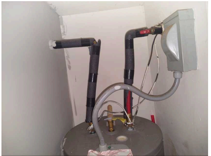
WH connections, with proper electrical disconnect
