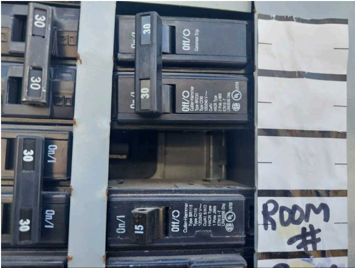
Open breaker slot on dead front cover panel
