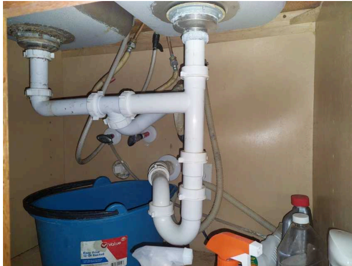
Food Waste Disposer not installed
