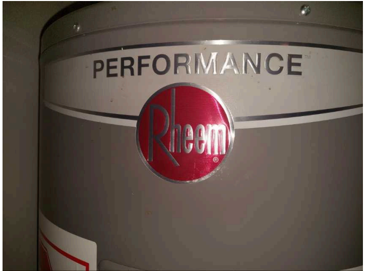
Water heater brand name
