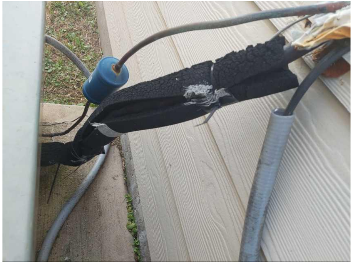
Damaged insulation on Freon line at AC condensing unit
