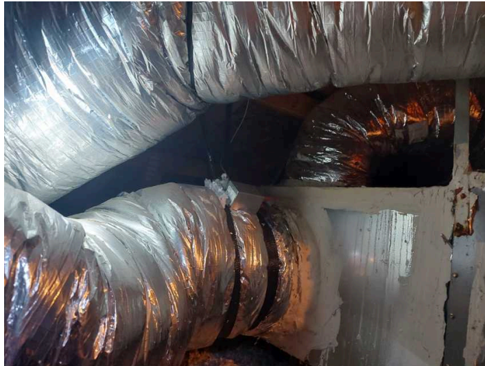
Picture of ducts in attic
