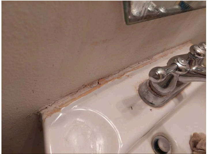
Caulking at downstairs hall bathroom is in need of repair
