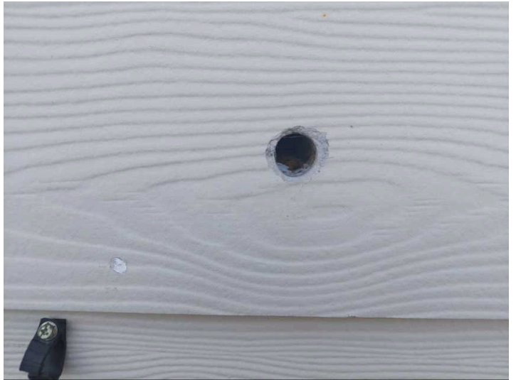
Exposed hole in back wall should be sealed
