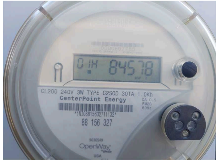
Picture of electric meter
