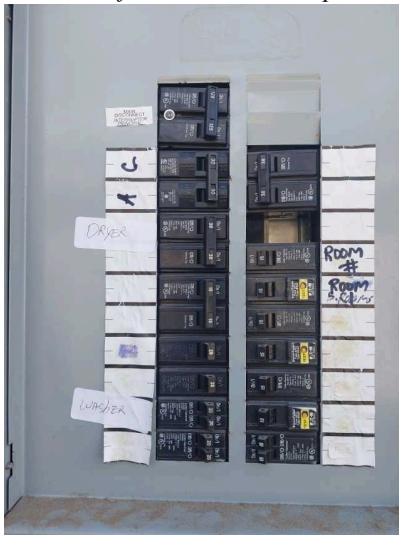
Picture of breakers
