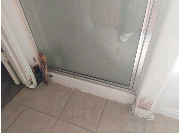
Interior wall damage, master bathroom
