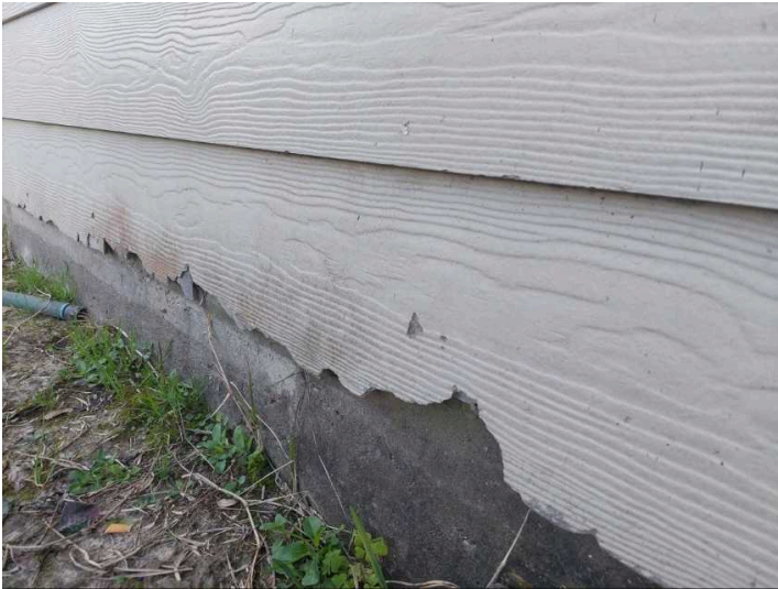
Damaged siding back side of house.
