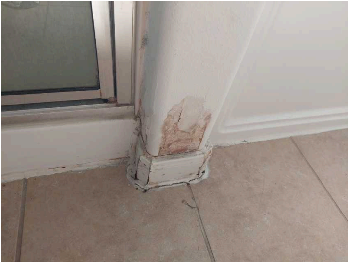
Interior wall damage, master bathroom
