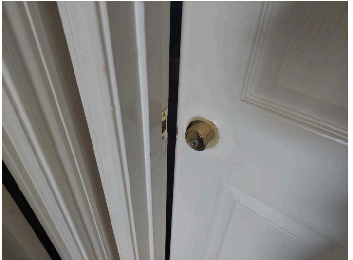
Bedroom door does not have proper door knob
