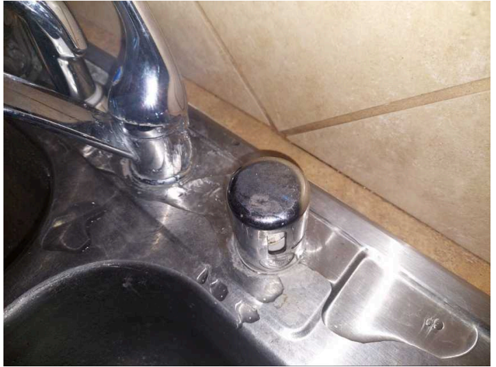
Leakage noted at kitchen faucet when turned on
