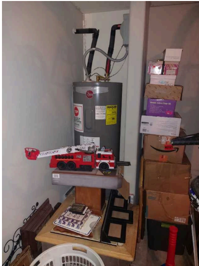
Picture of water heater
