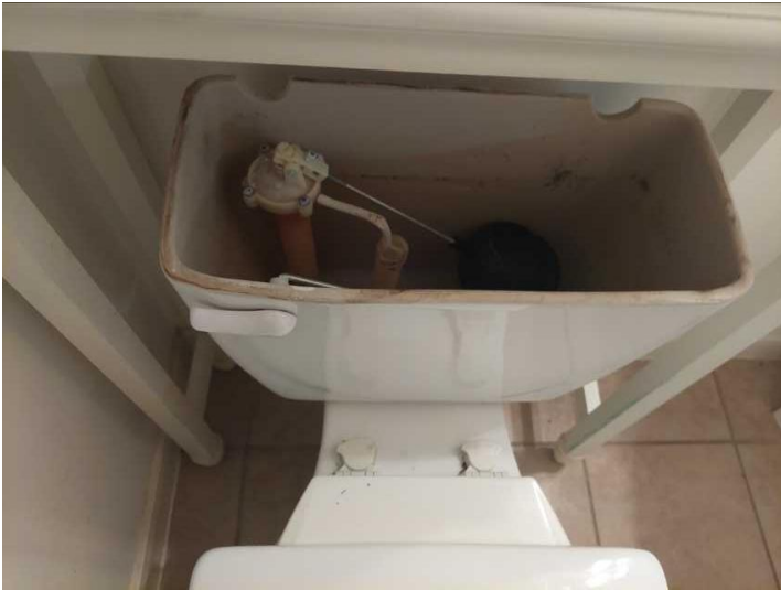
Downstairs hall bathroom toilet does not flush
