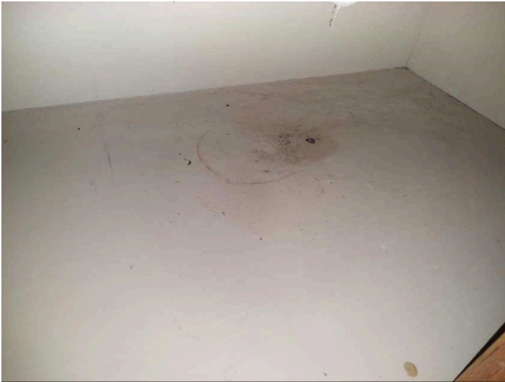
Water damaged cabinet floor in upstairs hall bathroom
