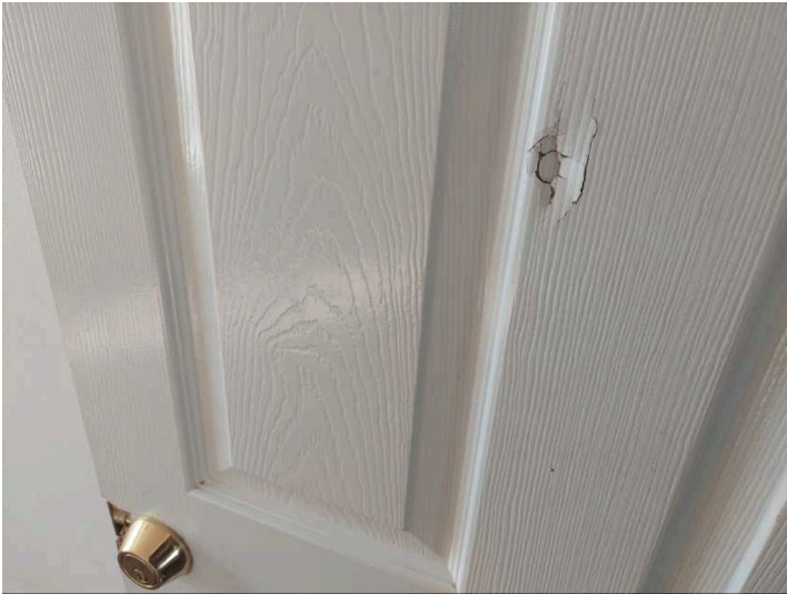
Bedroom door is damaged.
