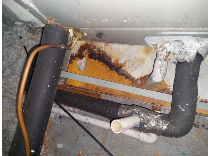
Corrosion present in evaporator overflow pan
