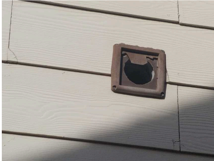
Dryer vent cover is missing backdraft damper
