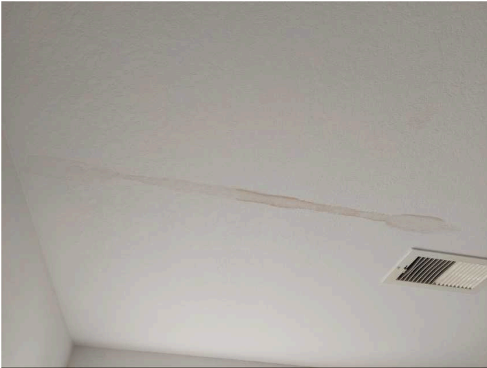
Moisture stain on ceiling, upstairs front bedroom
