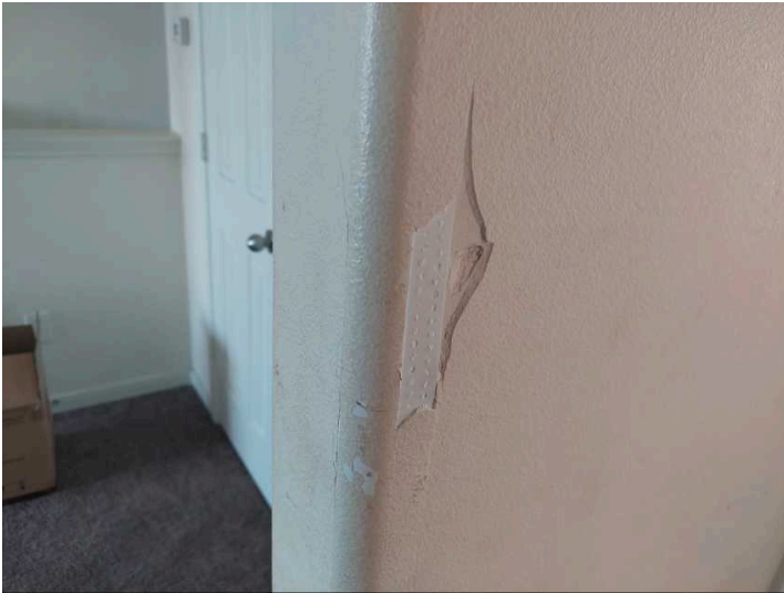
Interior wall damage
