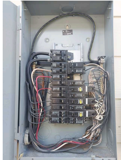
Picture with deadfront panel removed
