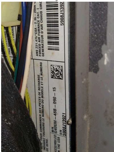
Furnace Data Tag (2008)
