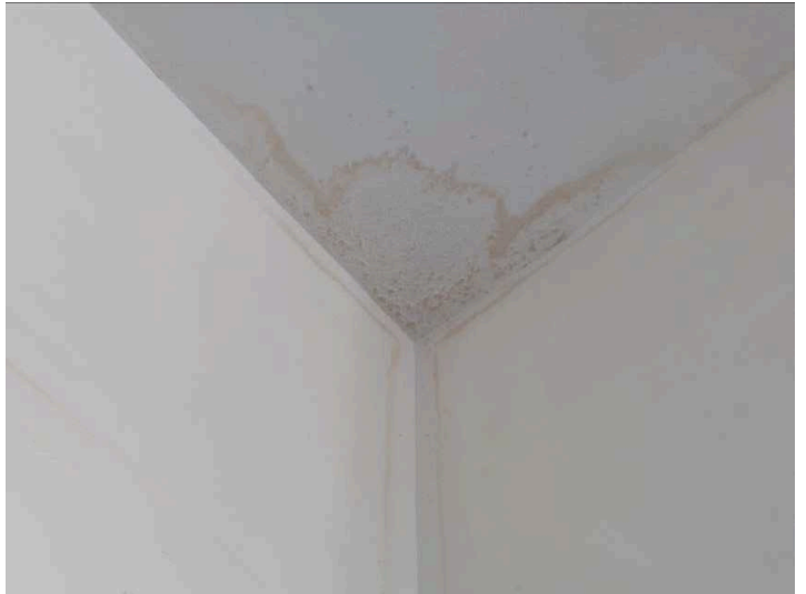
Moisture stain on ceiling, stairway
