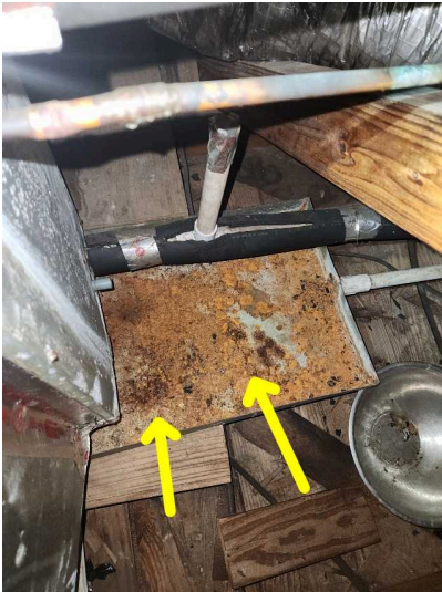
Rust in pan
