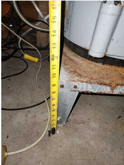
Water heater too low
