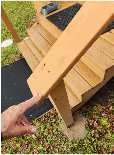
Not a grippable handrail
