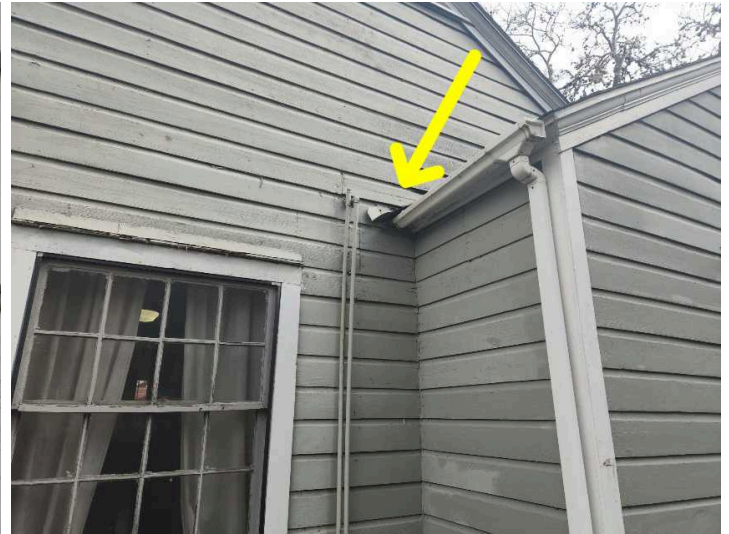
No kickout flashing
