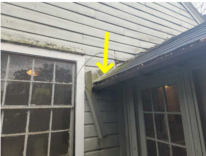
No kickout flashing
