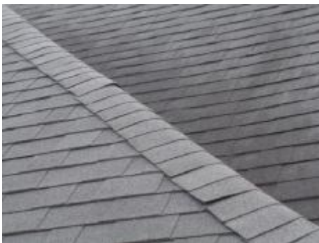
Roof raised shingle
