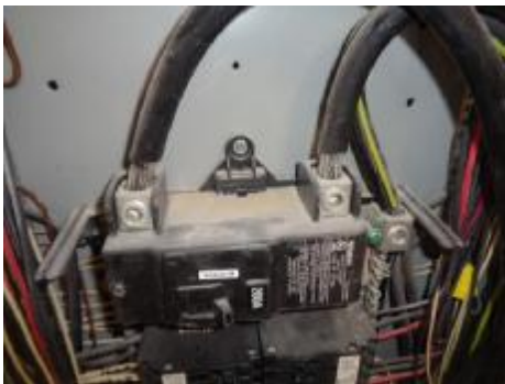
Missing anti-oxidant paste
