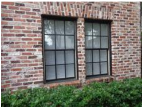
Window screens missing
