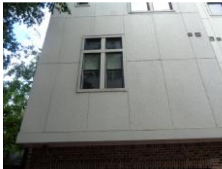
Window screens missing
