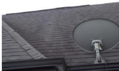
Roof raised shingle/fiberglass
