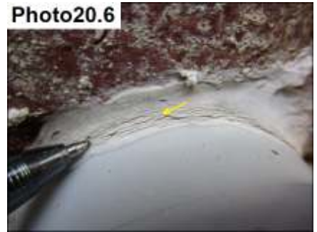
Penetration Sealants / Seal
