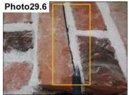
Crack Noted / Re Point As Needed
