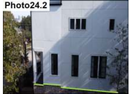
Brick/Stucco Termination / Maintain
