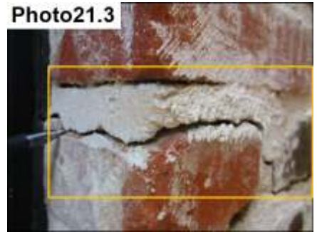
Crack Noted / Re Point As Needed
