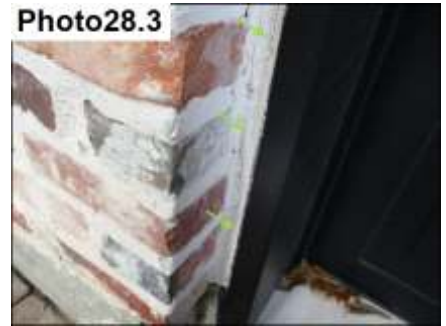
Door Sealant Separation / Seal
