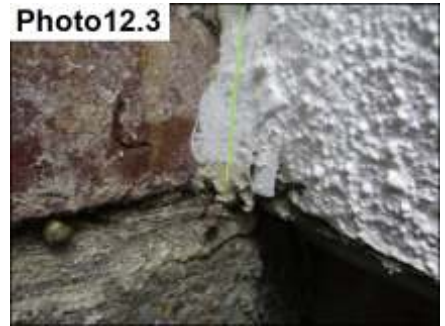
Brick/Stucco Termination / Maintain
