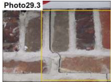
Crack Noted / Re Point As Needed
