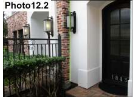
Brick/Stucco Termination / Maintain
