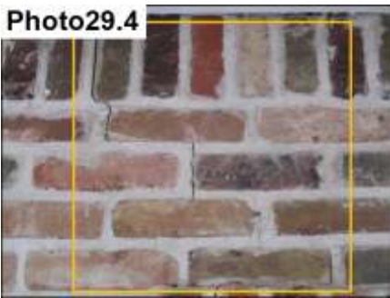
Crack Noted / Re Point As Needed
