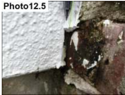
Brick/Stucco Termination / Maintain
