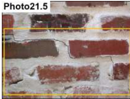
Crack Noted / Re Point As Needed
