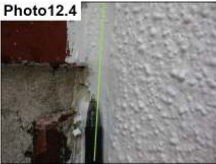
Brick/Stucco Termination / Maintain
