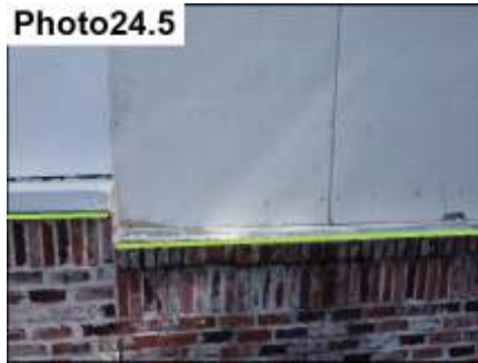
Brick/Stucco Termination / Maintain
