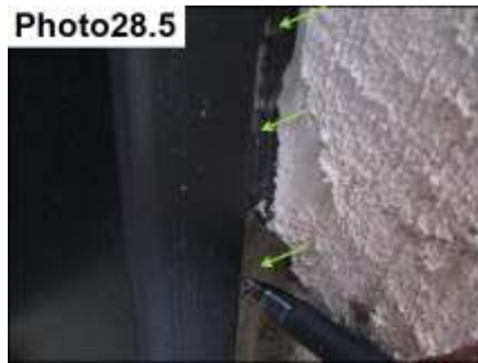
Door Sealant Separation / Seal
