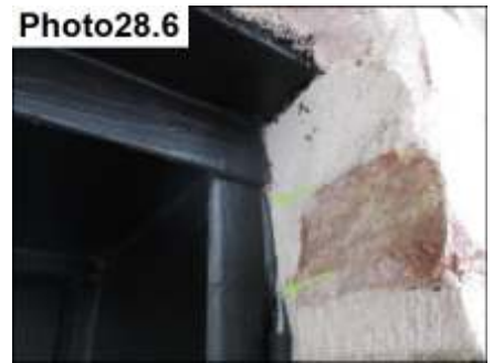
Door Sealant Separation / Seal
