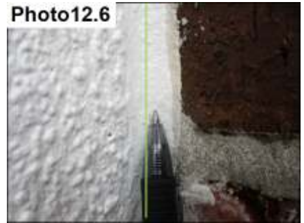
Brick/Stucco Termination / Maintain
