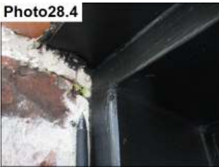
Door Sealant Separation / Seal
