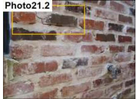
Crack Noted / Re Point As Needed
