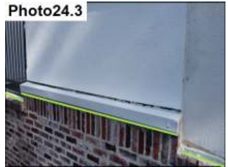
Brick/Stucco Termination / Maintain
