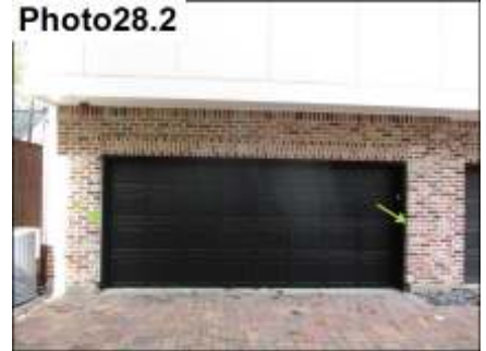
Door Sealant Separation / Seal
