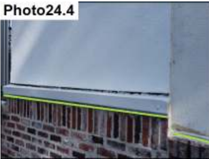
Brick/Stucco Termination / Maintain
