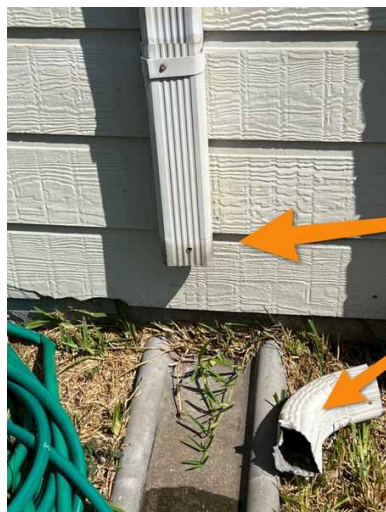
Elbow is disconnectd
