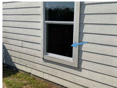
Missing screen, left side of the house.
