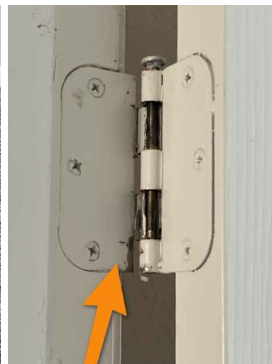
Second floor. Broken hardware at first door on the right side bedroom.
