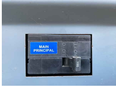
100 amps main breaker.
