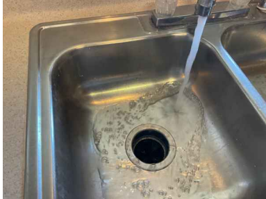
Kitchen faucet sink.
