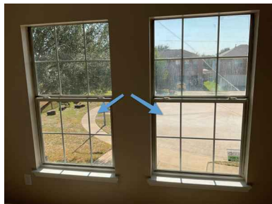
Missing screens. Second level front of the house.
