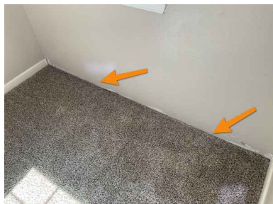
Middle room second floor. Missing trim in the closet.
