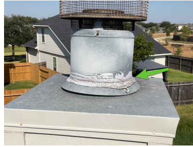
Old silicone needs to be replaced to prevent water intrusion.
