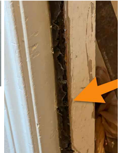
Garage door. Weatherstripping is damaged.
