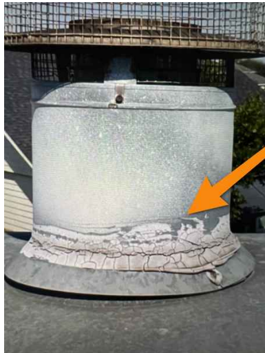
Need of sealing to prevent water from getting into the fire box
