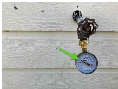
55 psi, Good water pressure for residential use.
