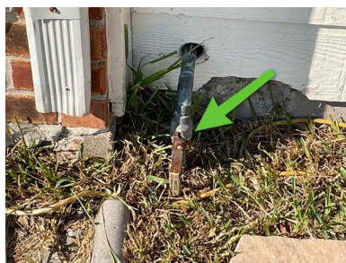
Location of the main water supply pipe and shut off water valve. Need to install insulation to protect from cold weather
