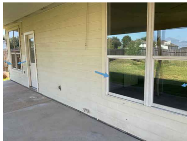
Missing screen on all 4 windows.
