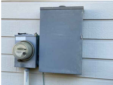
Location of the main panel
