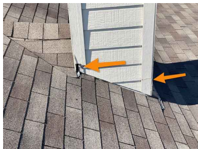
Damaged siding on the left side of the chimney.
