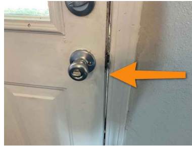
Back door. Damaged weatherstripping.
