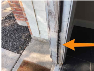
Front door. Damaged weatherstripping.
