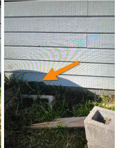
Back of the house next of condenser unit.
