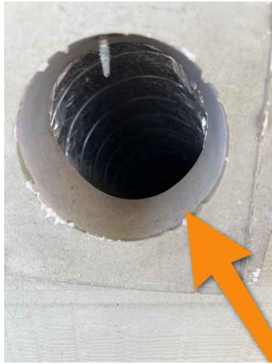
Missing dryer vent cover. And remove the trash from inside the duct.
