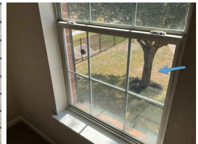
Missing screen. Second level.
