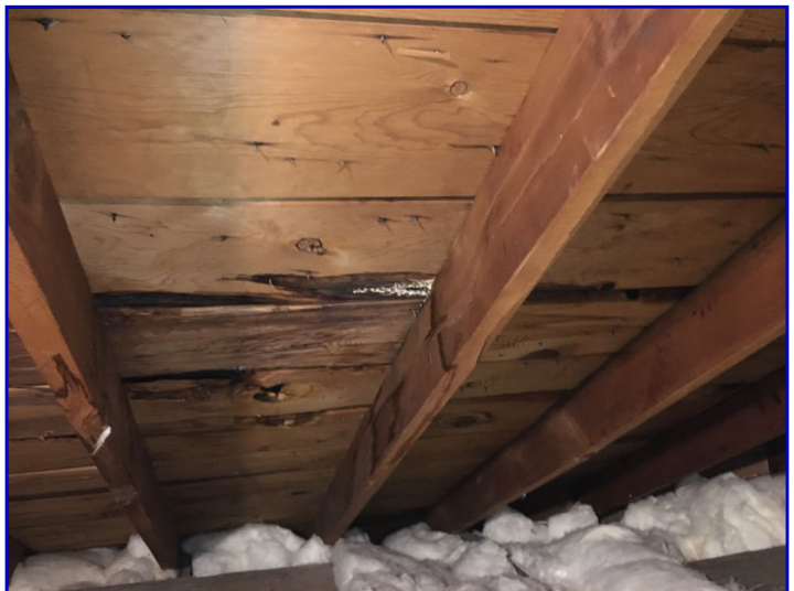
Dry roof sheathing stain observed on the front side of the attic
