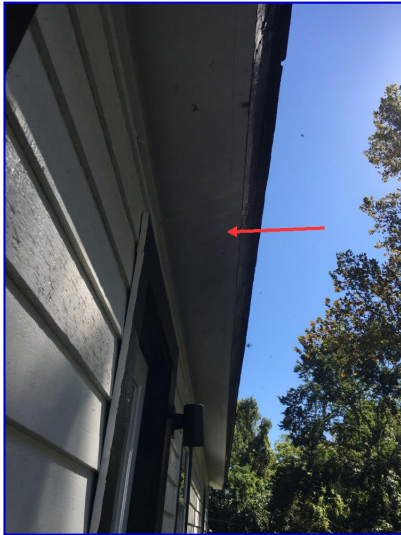
There were no soffit vents installed for the lower ventilation in the attic
