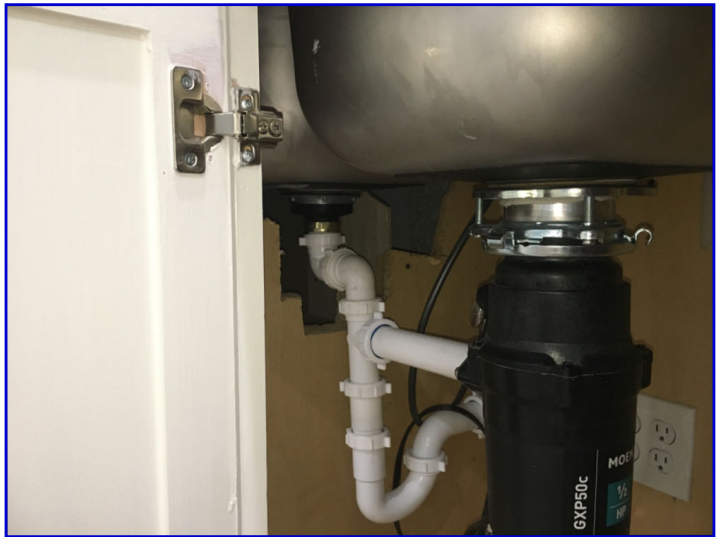
A section of the kitchen cabinet partition was removed to accommodate the kitchen sink drain line (which had a 90-degree fitting attached)
