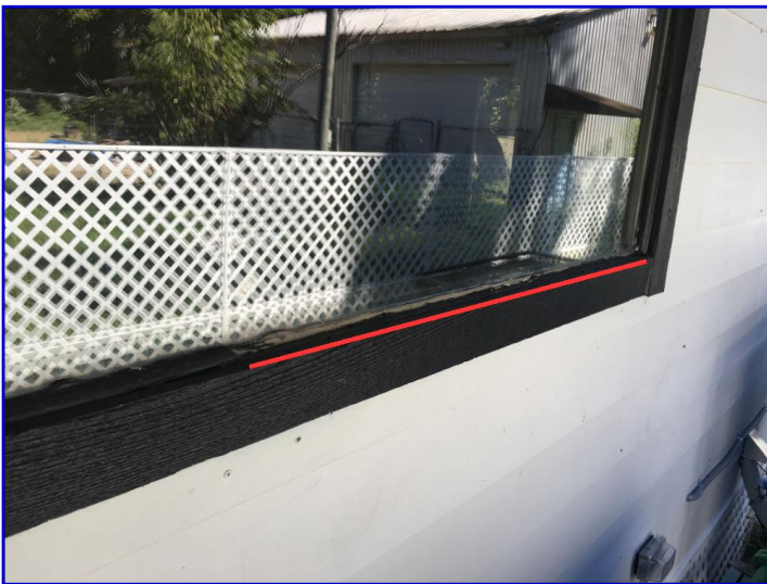
Damaged/missing wood glazing bead observed on the window on the right side of the home
