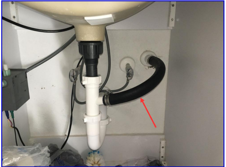
The attic AC unit primary condensate drain line was connected to the bathroom lavatory drain line
