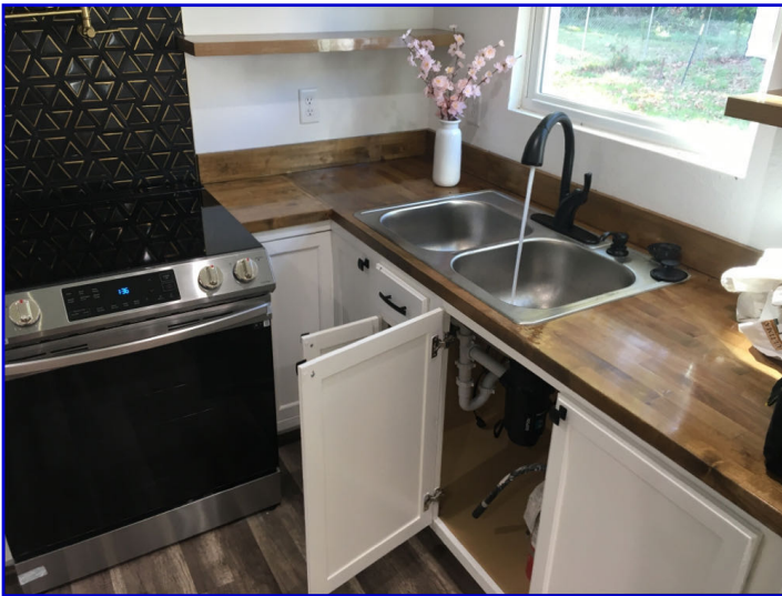
The sink was installed too close to the range (with limited space for access)
