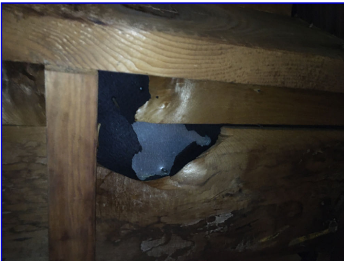
There were damaged sections of roof sheathing boards at various sections around the attic
