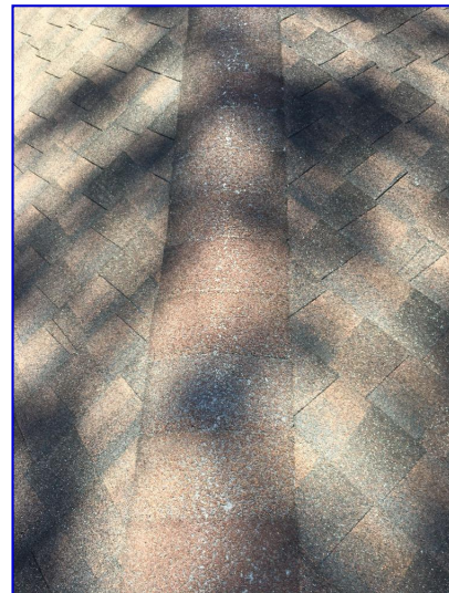
Granular loss and exposed felt observed to the hip shingles on the back side of the roof
