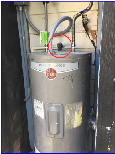
Water heater TPR safety valve
