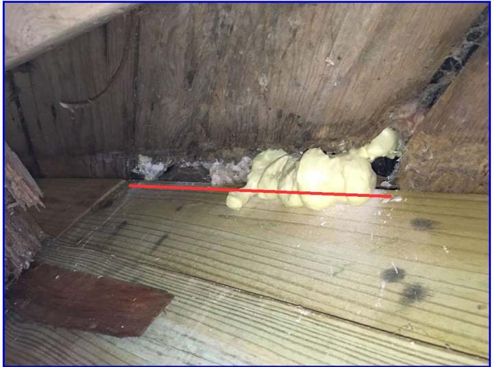
Deteriorated end of a sub-flooring board observed at the rim joist connection at the back left corner of the crawlspace
