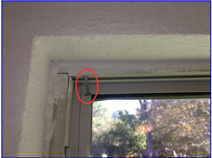
Observed incompletely installed window attachment screws in the front bedroom and middle bedroom
