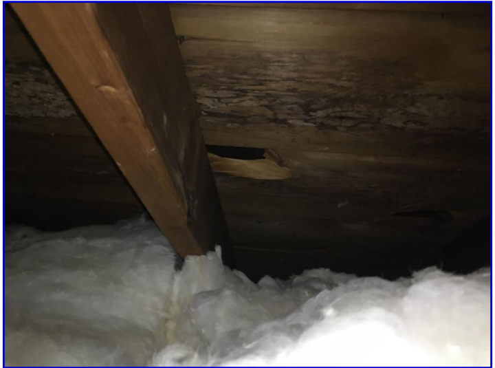
There were damaged sections of roof sheathing boards at various sections around the attic
