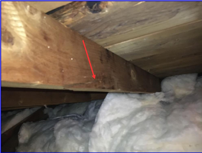
There was a cracked rafter on the front right corner of the attic
