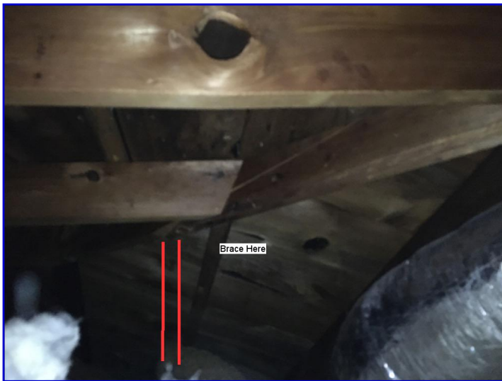
There was no support brace installed at the hip rafter joint at the back left corner of the attic
