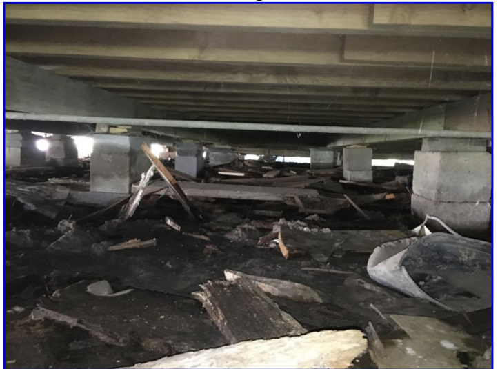
Only the left side and back side of the crawlspace were entered and inspected due to the build-up of debris
