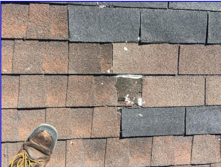
Damage to roof shingle observed on the right side of the roof
