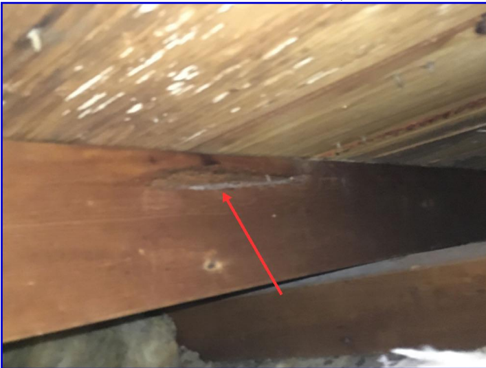
There was wood destroying insect damage to a rafter on the front left side of the attic
