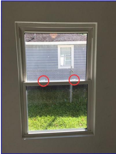
The middle bedroom window didn't close completely and lock
