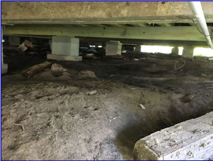
The grade under the home is currently lower than the level of grade on all sides, causing any water to remain under the home
