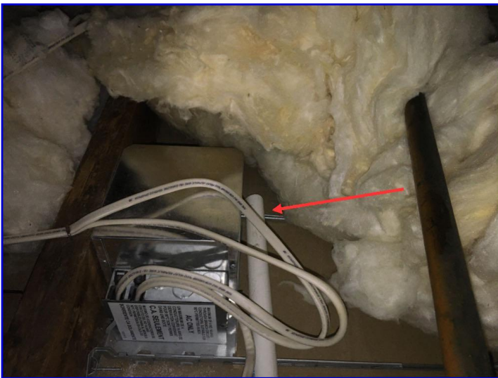
The AC unit secondary condensate drain line incorrectly terminated in the attic
