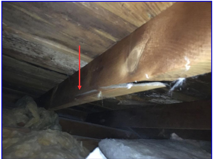
There was a cracked rafter on the front left side of the attic
