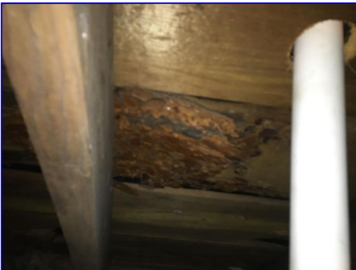
Moisture deteriorated roof sheathing board on the back side of the attic behind the range vent
