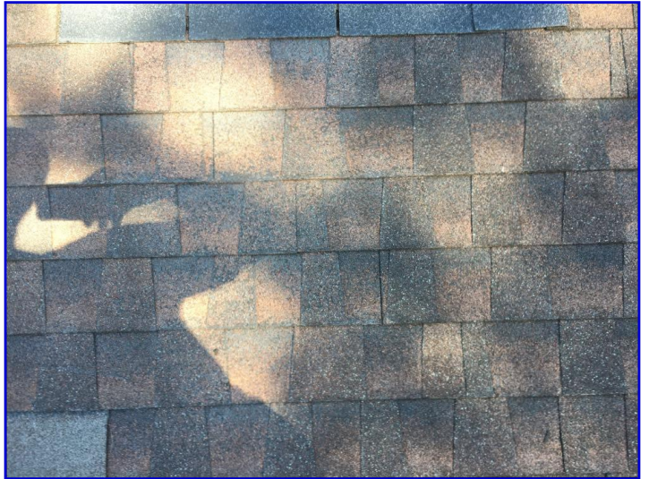
Granular loss observed to field shingles on the back side of the roof
