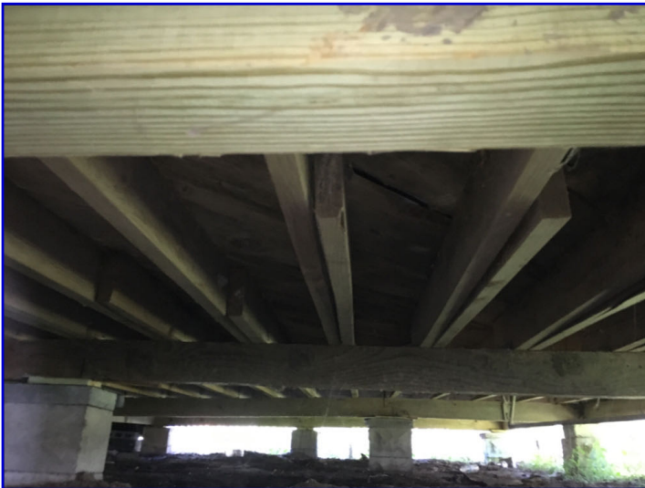
There was no underfloor insulation provided in the crawlspace
