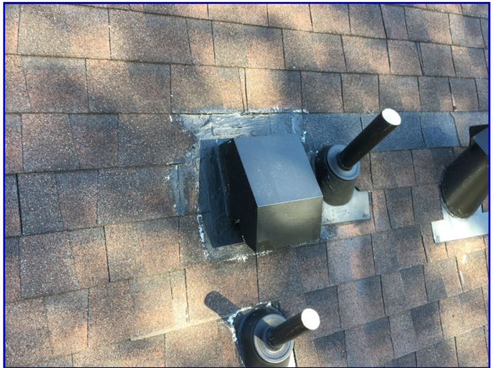
The range vent flashing on the back side of the roof was covered with mastic
