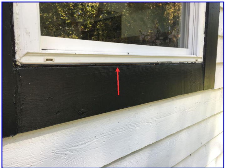
Observed gaps around window frames which should be sealed to prevent moisture entry
