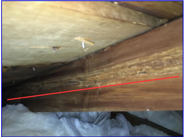
There was wood destroying insect damage to a rafter on the right side of the attic
