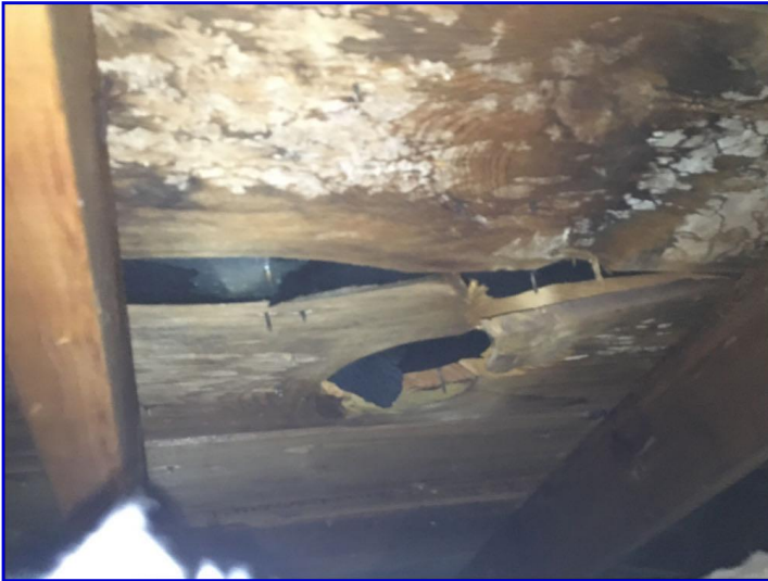
There were damaged sections of roof sheathing boards at various sections around the attic
