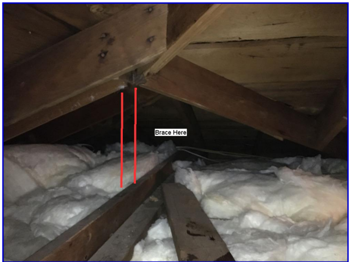
There was no support brace installed at the junction of the hip rafter and ridge rafter at the front right corner of the attic
