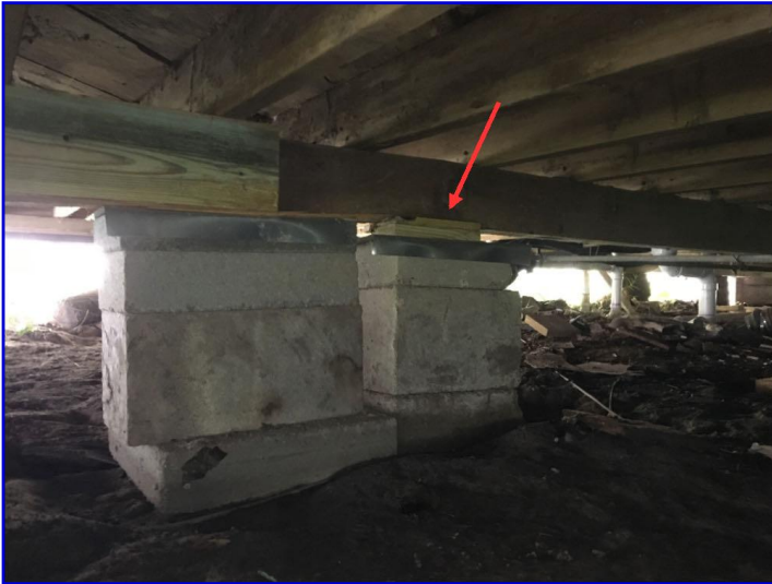
Wood shims were added to the tops of piers indicating previous settlement of the pier and beam foundation
