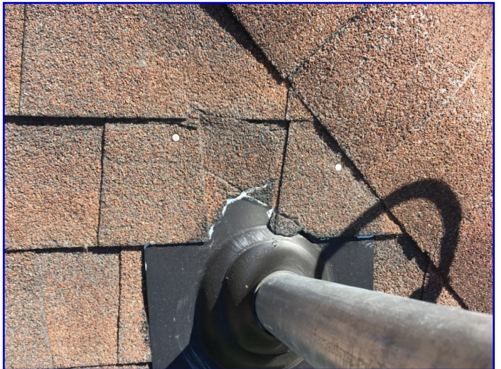
Damage to roof shingle observed on the right side of the roof
