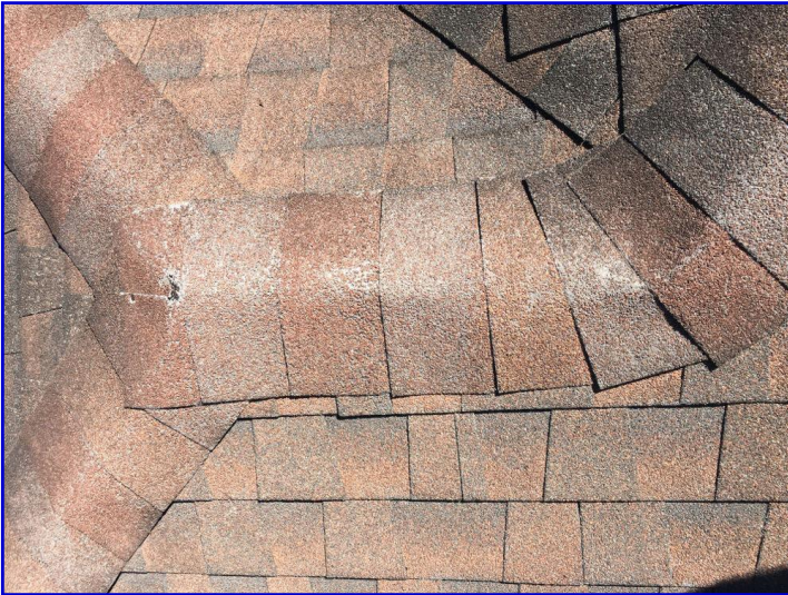
Granular loss and exposed felt observed to a short section of ridge shingles on the front right side of the roof
