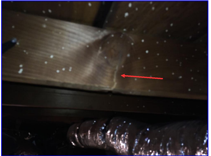
There was a cracked rafter on the back right corner of the attic
