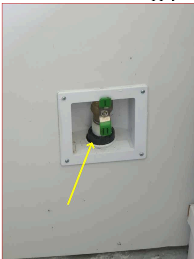
Main water supply side of home
