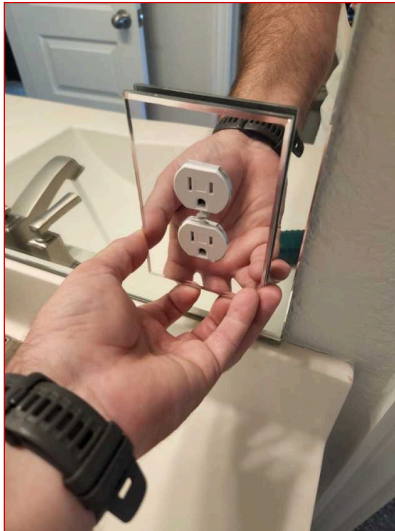
Outlet was loose in Jack and Jill bathroom.
