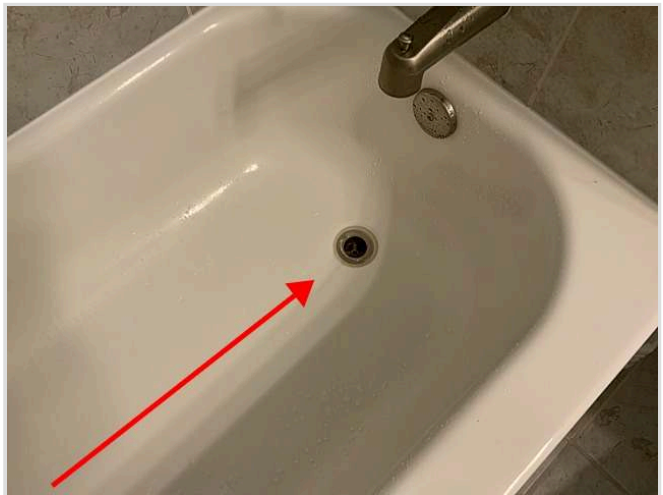
Second floor left side bathroom tub missing drain stop
