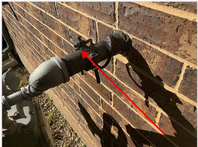
Grounding wire at the gas meter
