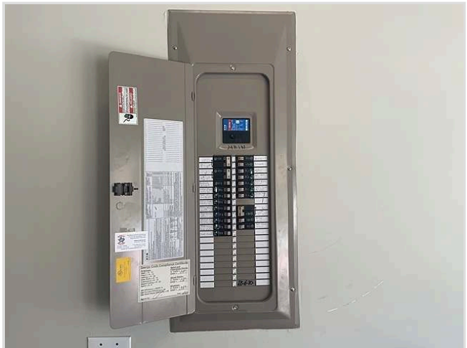
150 amp Cutler hammer electrical distribution panel board in the garage
