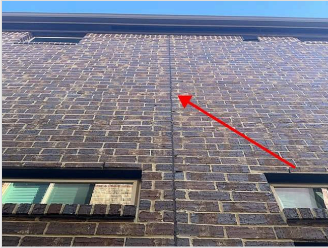
Separation at the expansion joint on the left side
