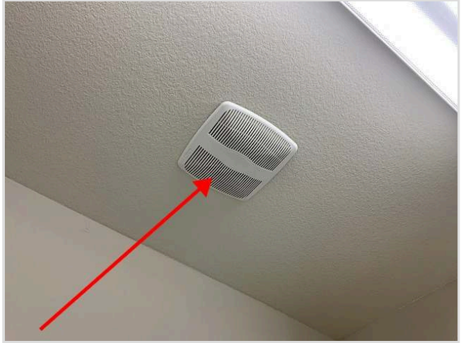
Laundry room mechanical exhaust fan
