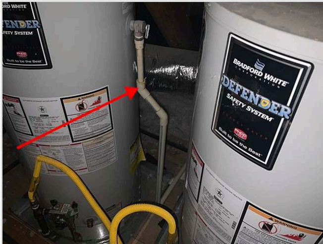
Discharge piping at the temperature and pressure relief valve
