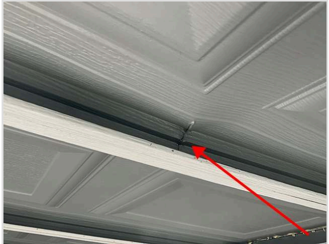
Damage to the overhead garage door
