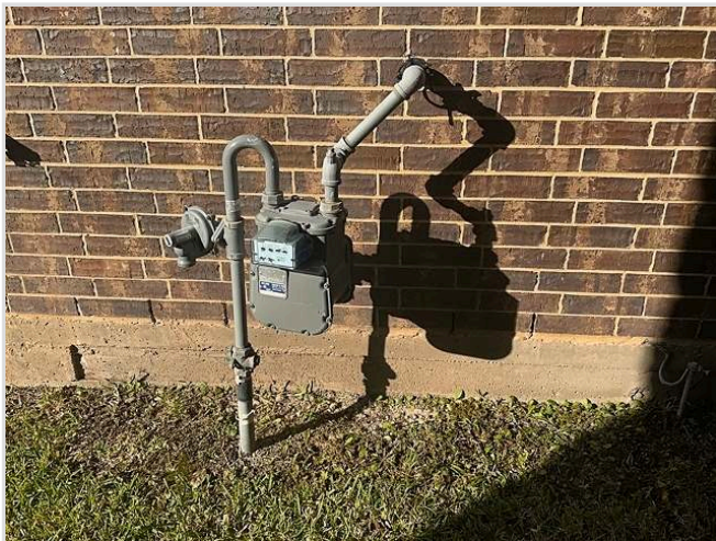
Gas meter at the right side exterior
