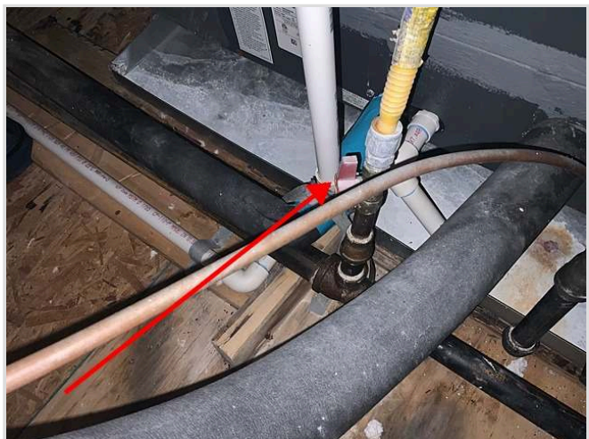
Gas supply line block valve at the heating unit in the attic
