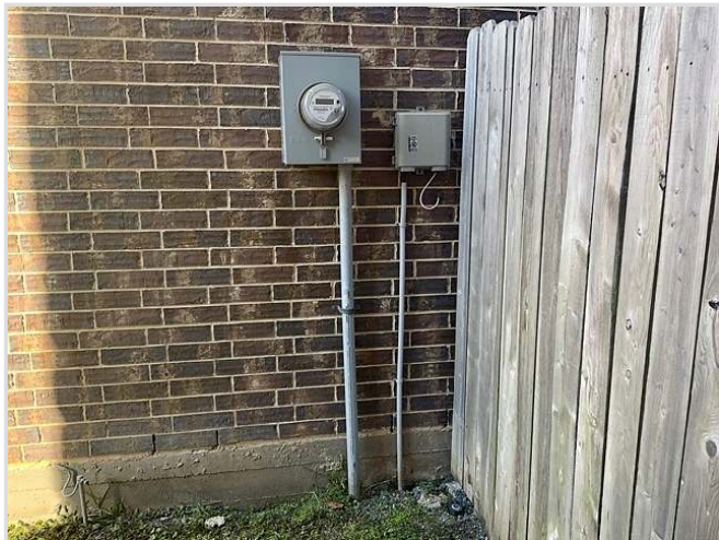
Underground electrical service at the right side exterior
