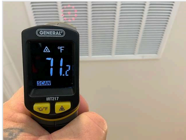
Return air temperature 71.2°
