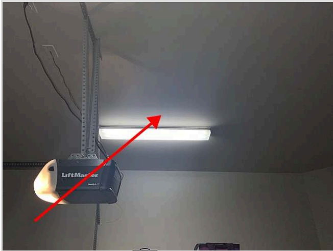
Cracks in the garage ceiling
