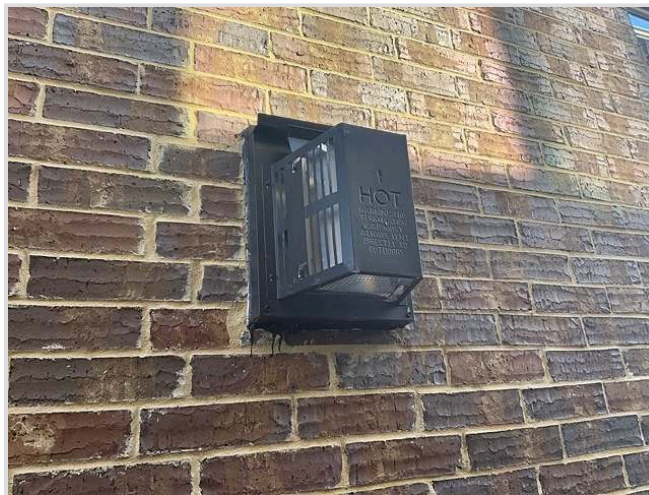
Exhaust vent for the gas powered fireplace insert/heating unit in the living room
