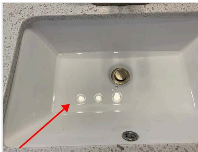
Second floor master bathroom sink not draining properly
