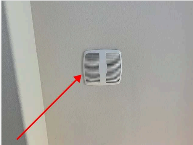
Second floor master bathroom mechanical exhaust fan
