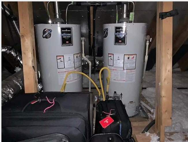
Water heating units in the attic space
