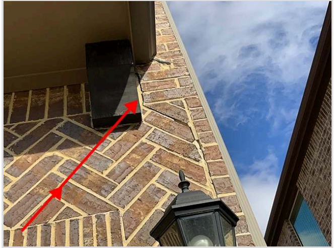
Cracks in the brick and mortar front side exterior
