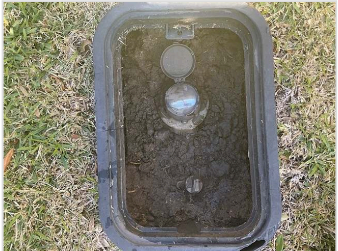
Water meter in the front yard near the street
