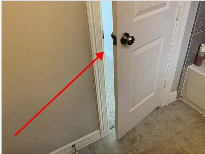
Second floor right side front bathroom door not latching in the closed position
