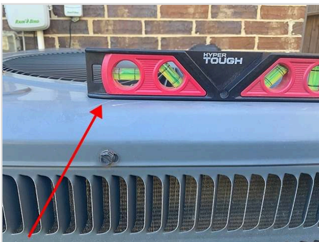
Condensing unit out of level
