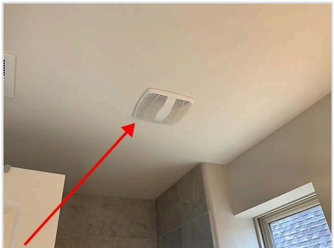
Second floor right side front bathroom mechanical exhaust vent
