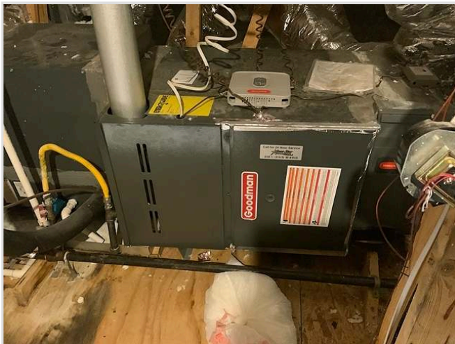
Heating unit in the attic space
