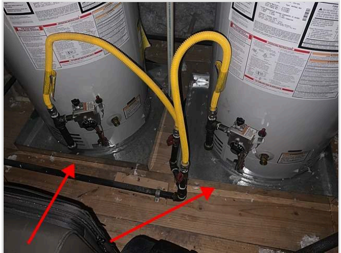
Pans beneath the units
