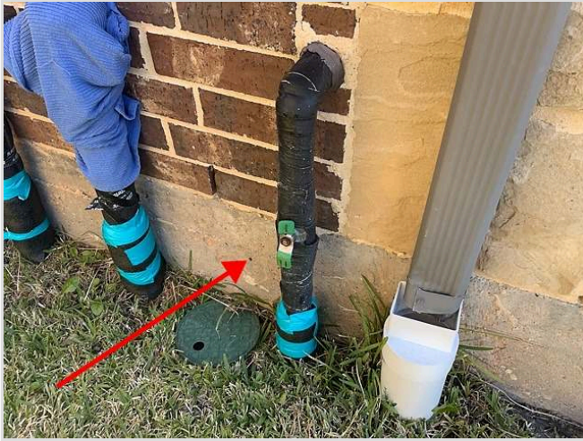
Water-main at the left side exterior of the house
