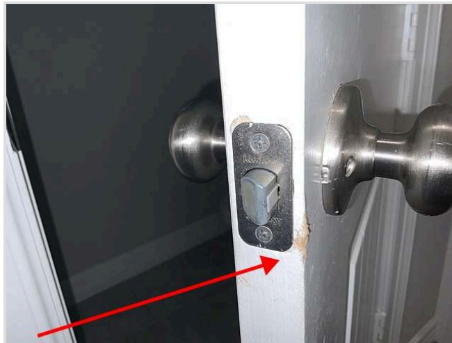
Damage to the half bathroom door
