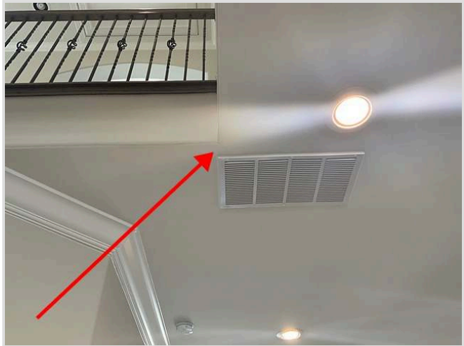
Cracks in the living room ceiling
