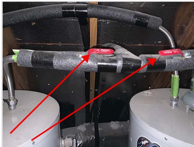
Cold water block valves at the water heating unit in the attic
