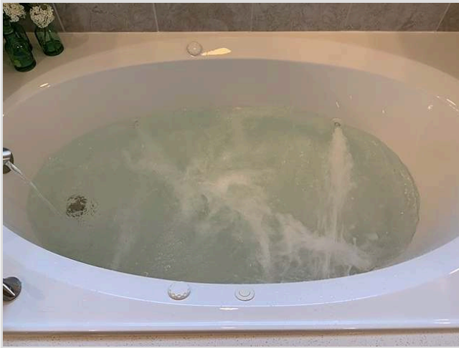
Second floor Hydro massage therapy tub performing as intended
