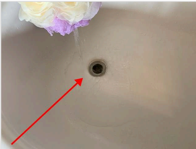
Second floor right side bathroom tub missing drain stop
