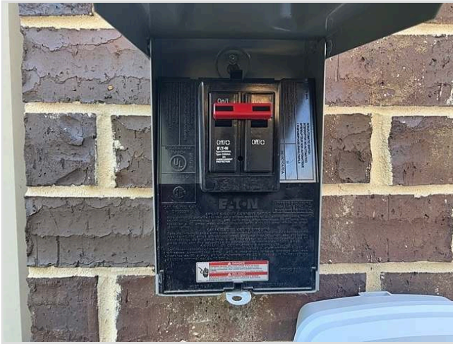
Condensing unit electrical disconnect
