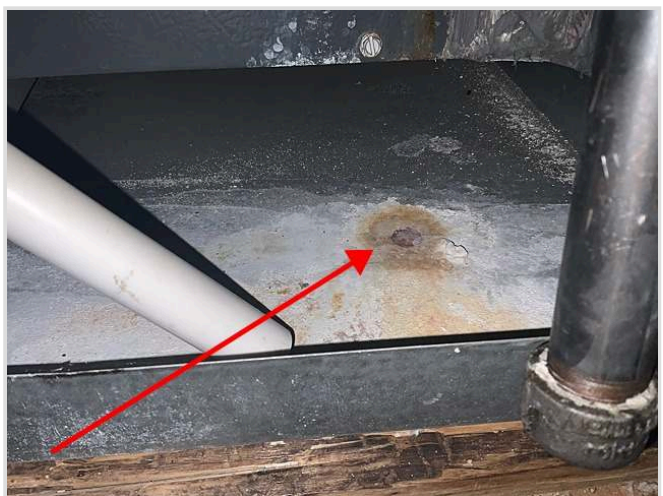
Corrosion in the pan beneath the evaporator coil housing
