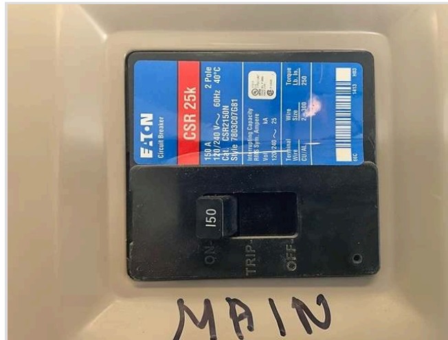
150 amp main disconnect
