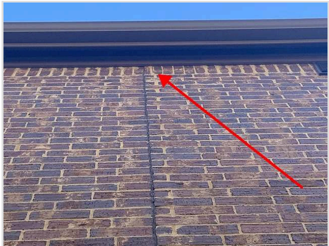
Cracks in the brick and mortar at the left side
