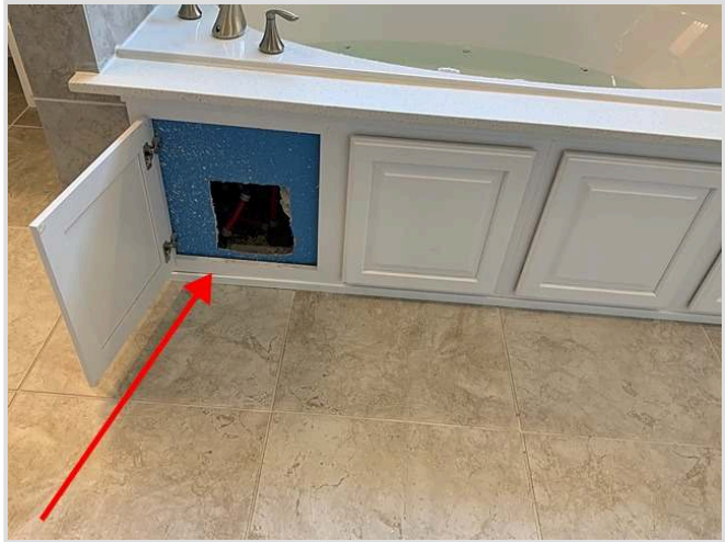
Hydro massage therapy tub pump access
