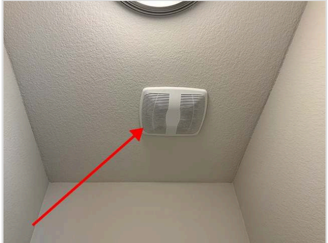
Second floor master bathroom water closet mechanical exhaust fan
