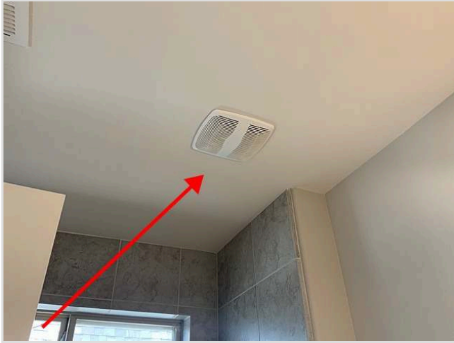
Second floor left side front bathroom mechanical exhaust vent
