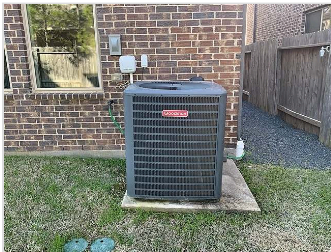
Condensing unit at the rear exterior
