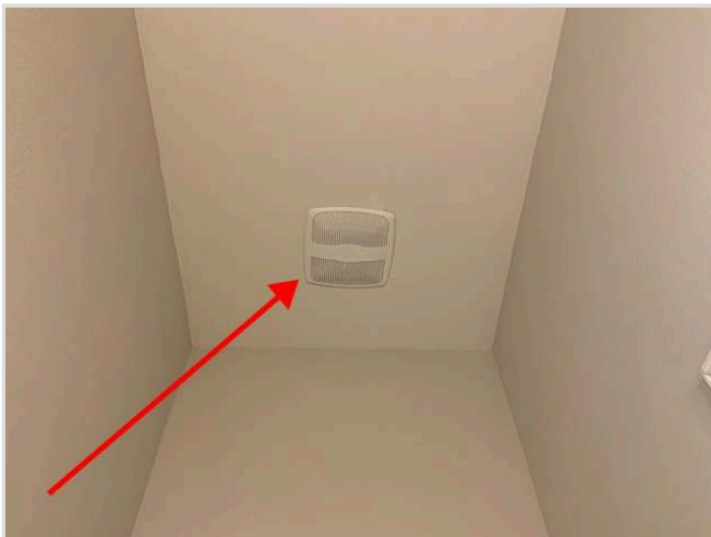
Half bathroom mechanical exhaust vent
