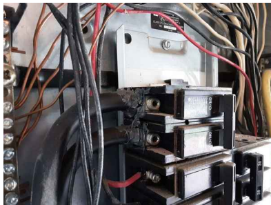
Aluminum service entrance wires with anti-oxidant compound
