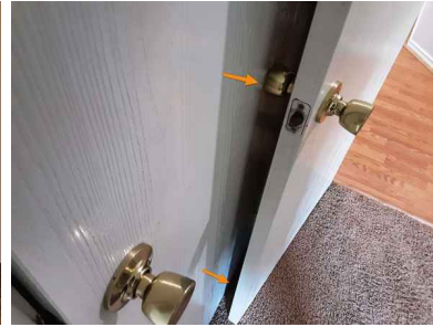
Missing door stoppers
