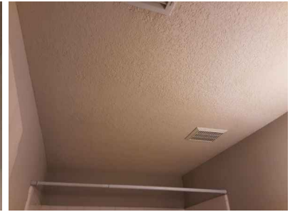
Ceilings and floors appear to be performing as intended at the time of the inspection
