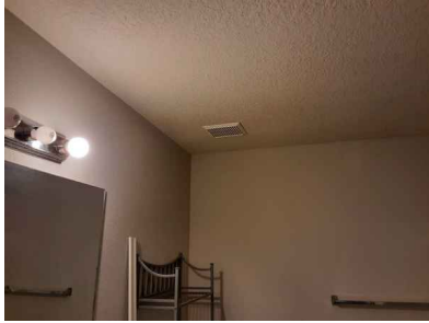
Bathroom exhaust vent
