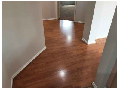
Ceilings and floors appear to be performing as intended at the time of the inspection
