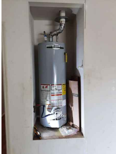
The water heater
