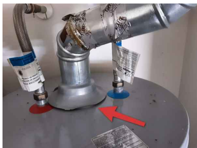
Improper draft hood Installation
