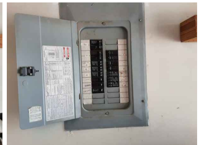
The electrical panel is labeled
