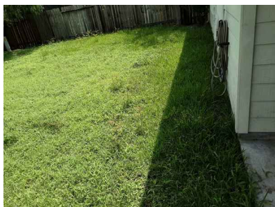
Negative Grading in the back of the house
