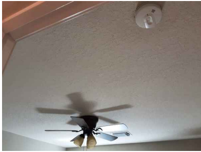
Ceilings and floors appear to be performing as intended at the time of the inspection
