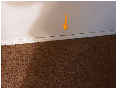
Minor baseboard crack
