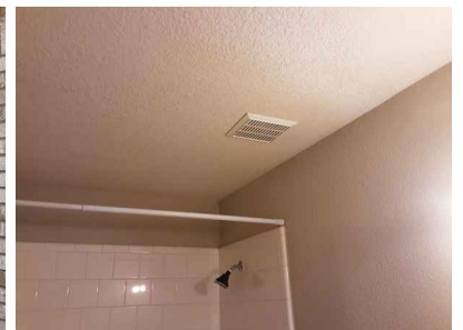
Bathroom exhaust vent
