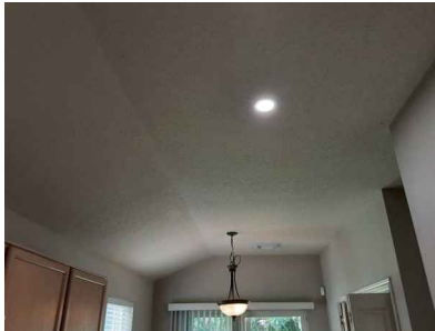
Ceilings and floors appear to be performing as intended at the time of the inspection
