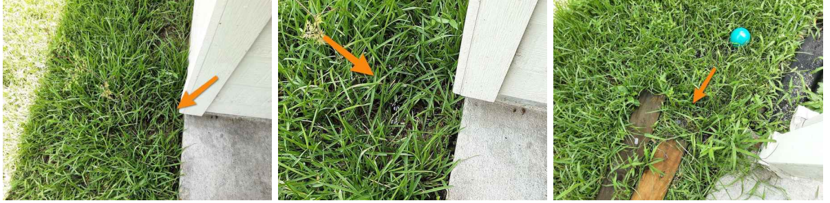
Standing Water in the back of the house Standing Water in the back of the house Standing Water in the back of the house
