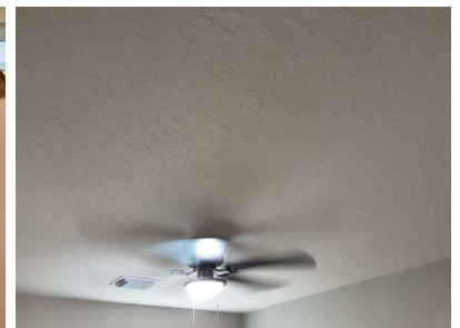
Ceilings and floors appear to be performing as intended at the time of
