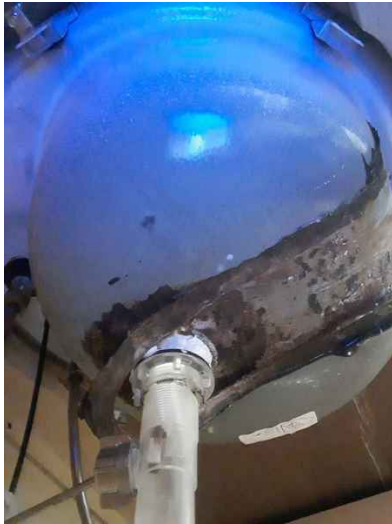
Sink overflow missing
