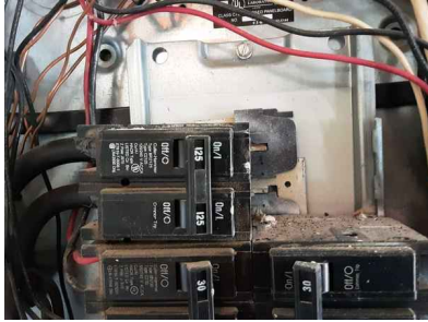
Main breaker amps
