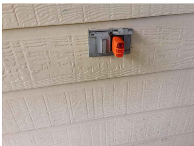
Outdoor outlets are not connected.
