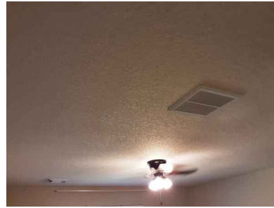
Ceilings and floors appear to be performing as intended at the time of the inspection
