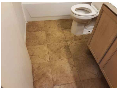
Ceilings and floors appear to be performing as intended at the time of
