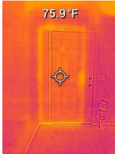
Some conditioned air escaping from the front door
