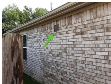
Kitchen exhaust termination
