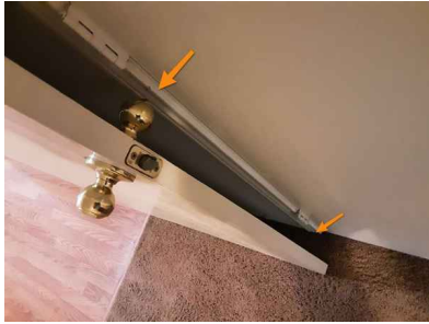
Missing door stoppers
