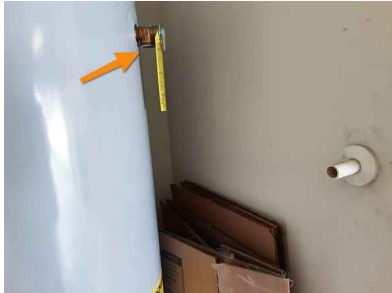
must terminate not more than 6 inches above the floor, or pan
