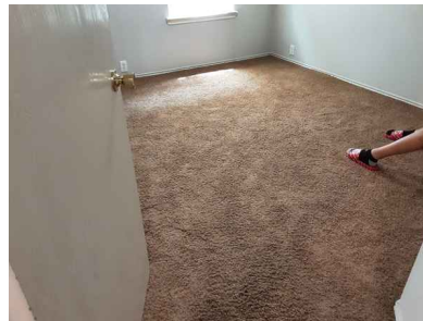
Ceilings and floors appear to be performing as intended at the time of the inspection
