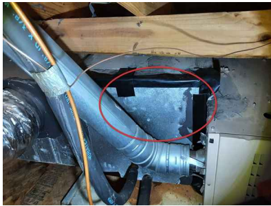
Missing correct sealing compound
