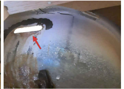
Sink overflow missing
