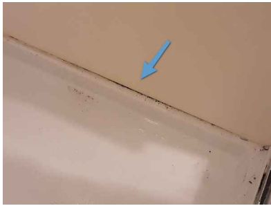
Shower wall debris
