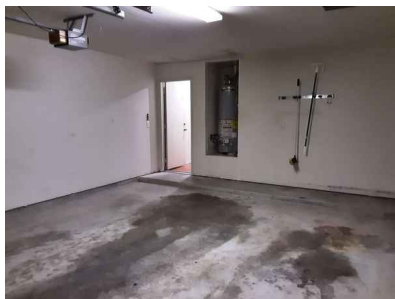
Garage door self closing mechanism missing
