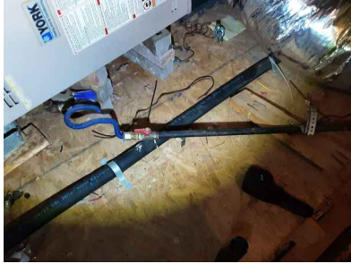
Sediment trap missing
