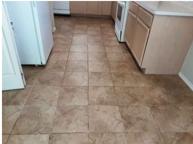
Ceilings and floors appear to be performing as intended at the time of the inspection
