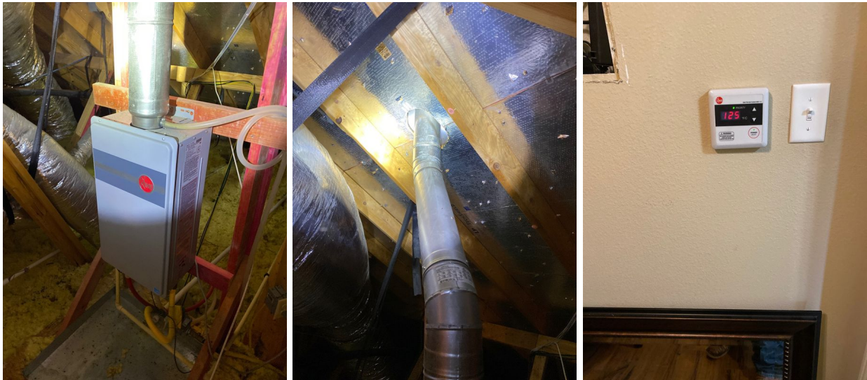
Observations:: Minor Wear and Tear
