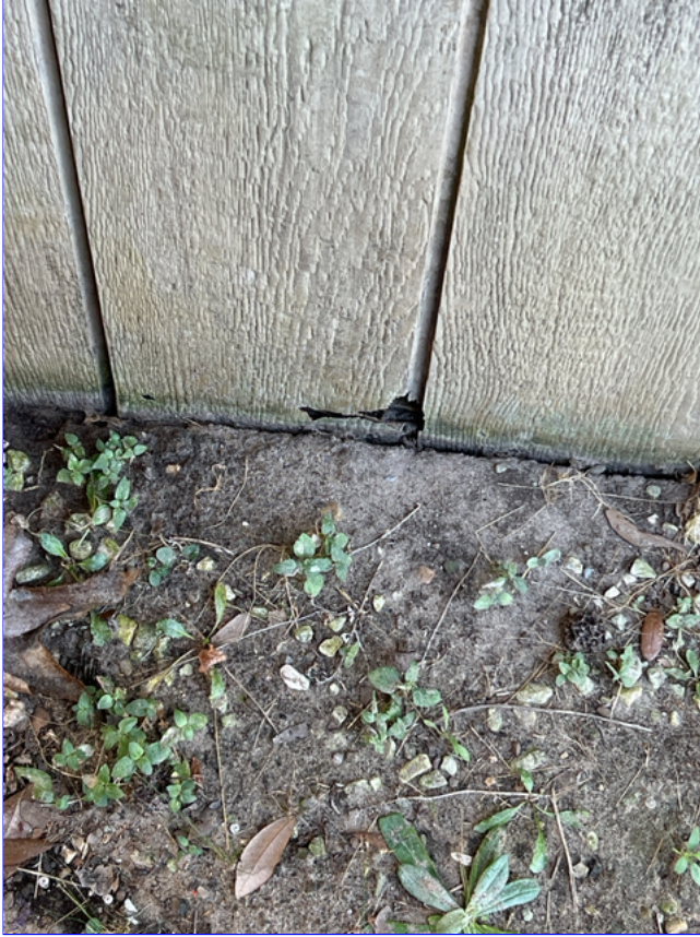
B. Photo 2(Picture) The grading and drainage around the garage is deficient.
