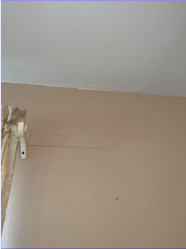
E. Photo 11(Picture) The drywall on the inside of the home has many structural cracks throughout.
