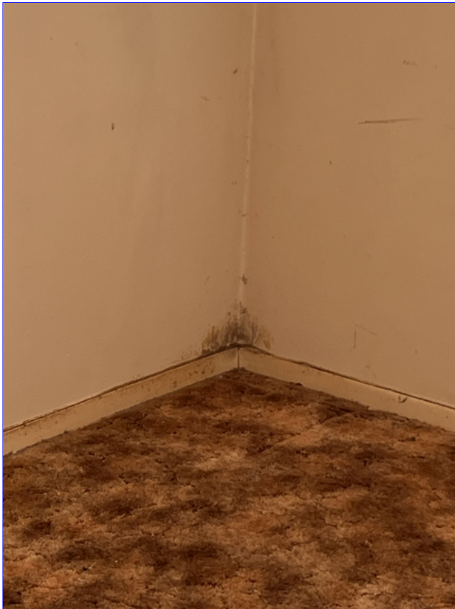
E. Photo 14(Picture) Stain was observed at the bottom of the wall in the corner of the left rear bedroom.
