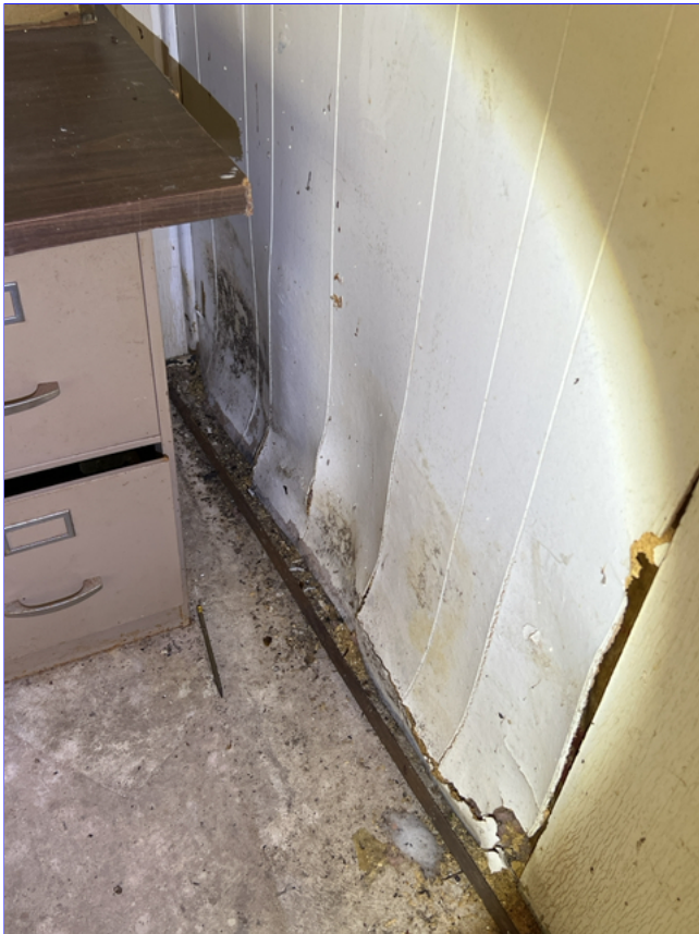
E. Photo 7(Picture) The poor drainage around the outside of the garage has caused moisture damage to the interior walls.
