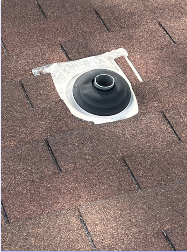
C. Photo 5(Picture) One of the roof jacks needs to have the piping extended
