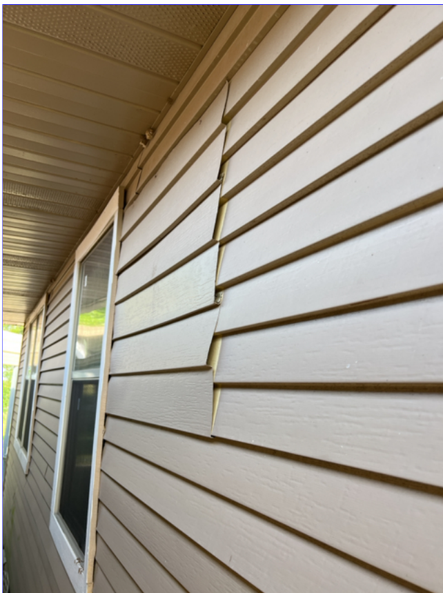
E. Photo 3(Picture) The wrong size siding was installed which is now causing large gaps.
