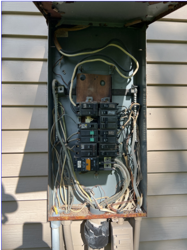
A. Photo 3(Picture) The main electrical service panel
