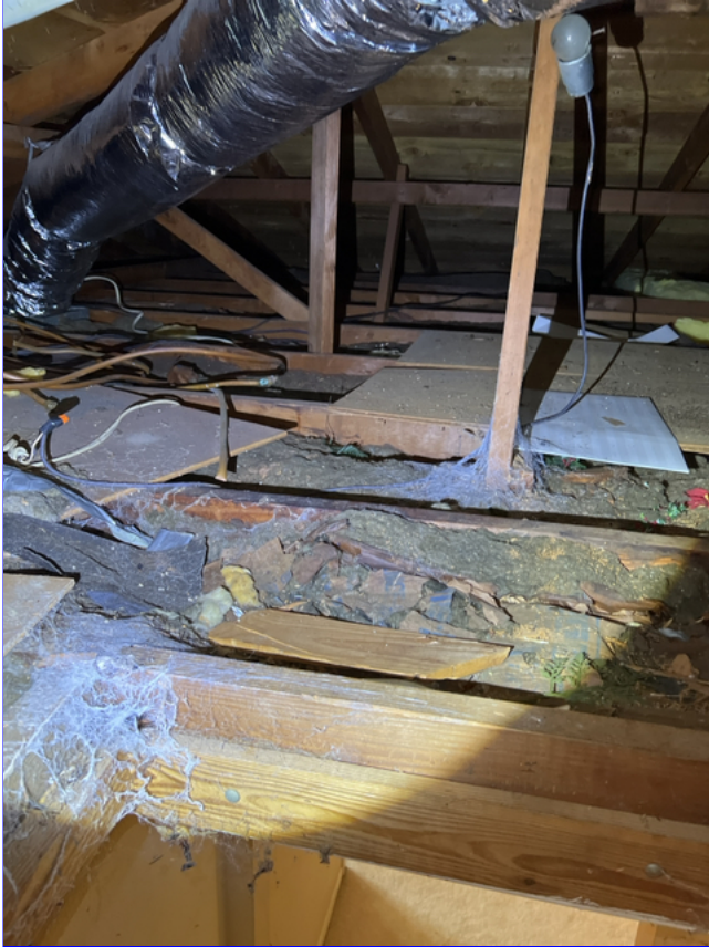
D. Photo 1(Picture) The insulation in the attic is matted down and no longer insulating as intended.
