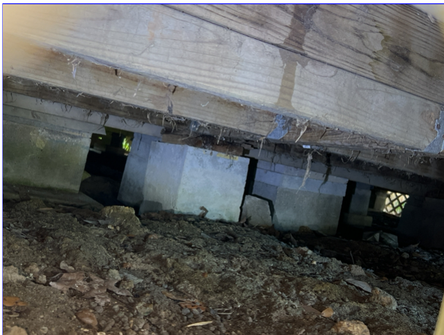
L. Photo 1(Picture) Termite shields are missing on top of some of the blocks under the house.
