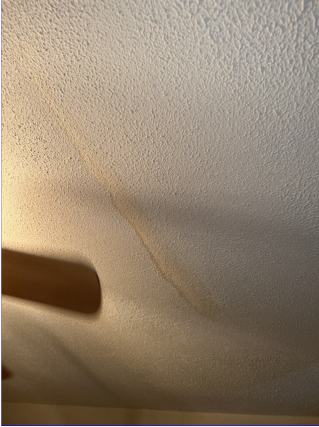
F. Photo 2(Picture) Water stains were observed to the ceiling in the front middle bedroom of the house.
