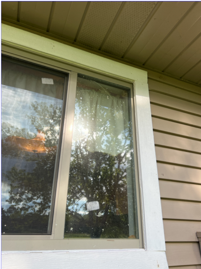
H. Photo 2(Picture) A window at the rear of the home has a broken pane of glass.
