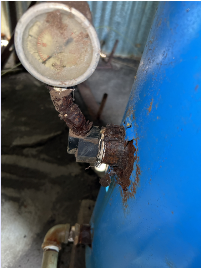
A. Photo 2(Picture) I also observed rust on the outside of the tank and at the pressure gauge.
