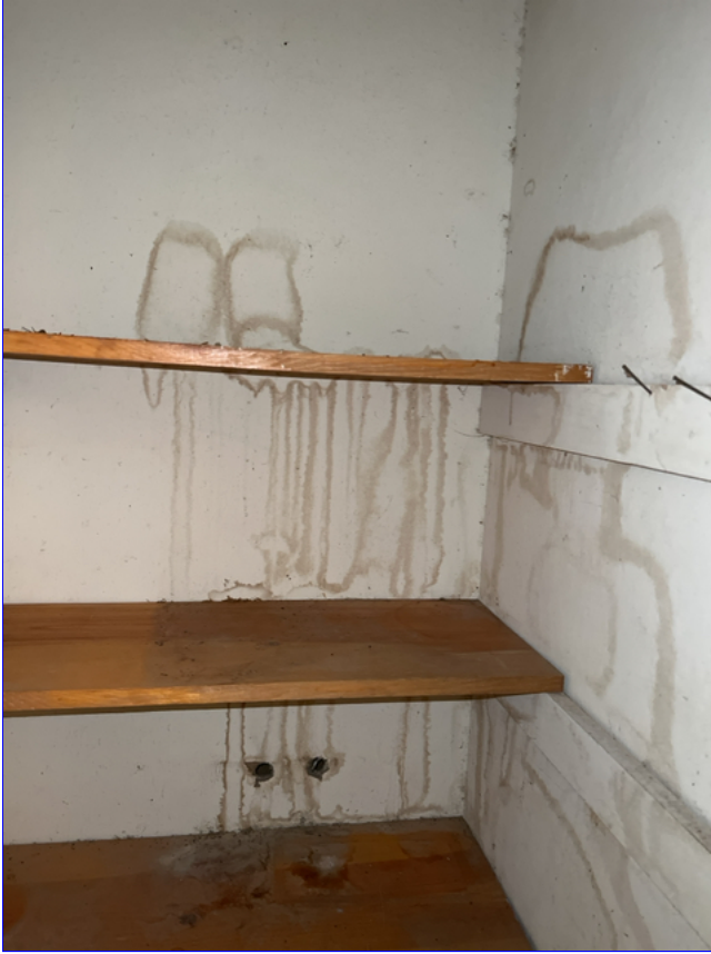
B. Photo 3(Picture) The interior space of this closet is showing moisture staining.
