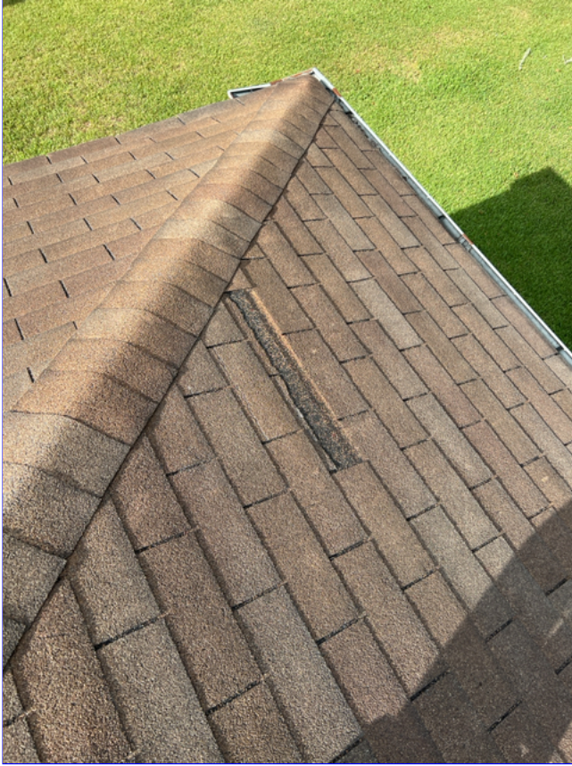
C. Photo 8(Picture) Several missing and damage shingles were observed on the roof.
