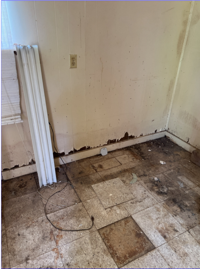
E. Photo 5(Picture) The poor drainage around the outside of the garage has caused moisture damage to the interior walls.
