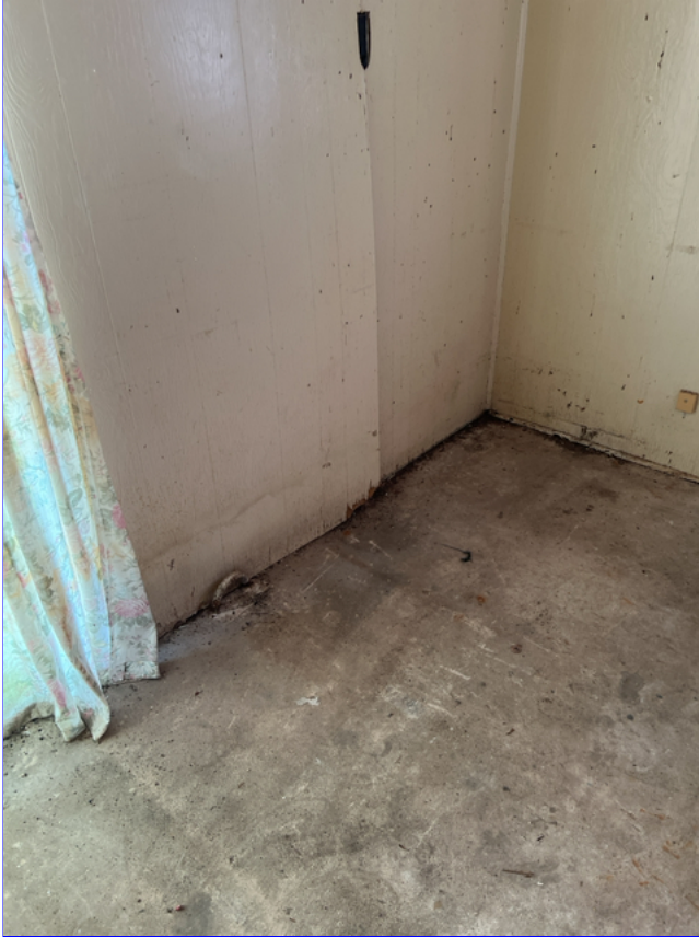
E. Photo 6(Picture) The poor drainage around the outside of the garage has caused moisture damage to the interior walls.
