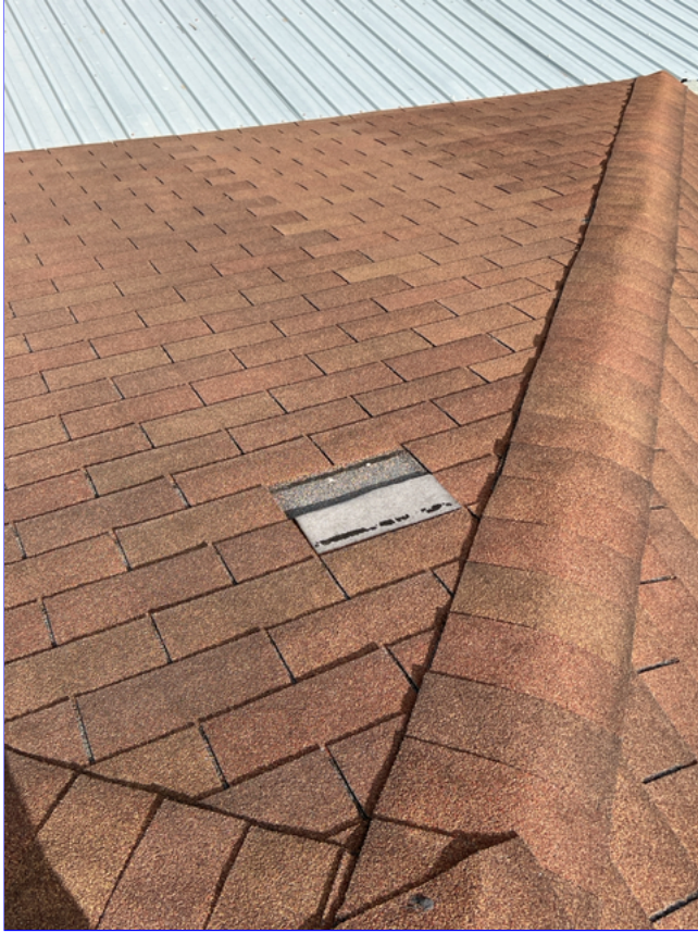
C. Photo 6(Picture) Several missing and damage shingles were observed on the roof.
