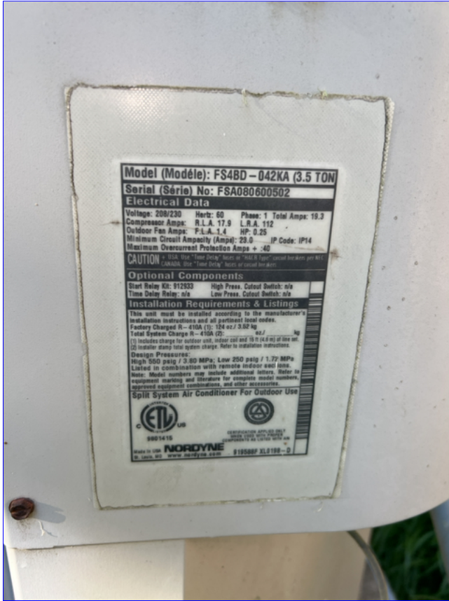
B. Photo 1(Picture) Air Conditioning service tag(s).
