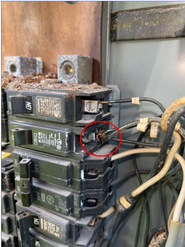
A. Photo 1(Picture) Some breakers, are triple tapped.
