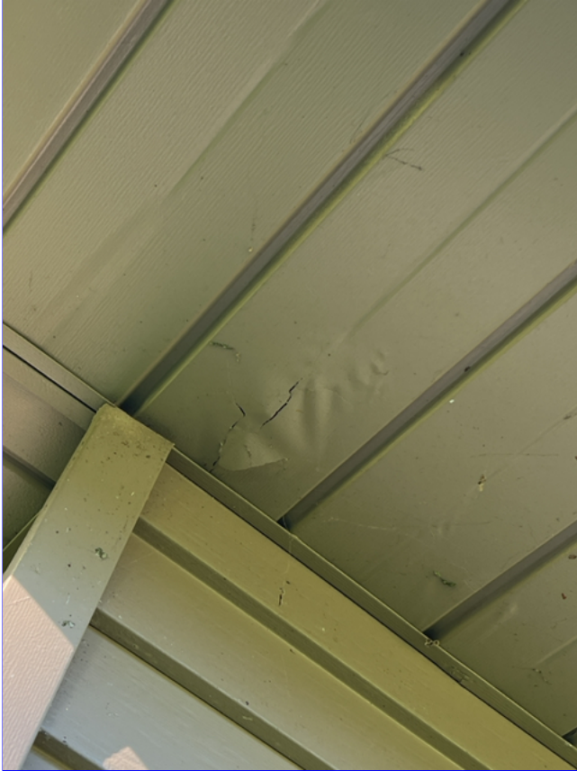
E. Photo 2(Picture) paint is peeling
