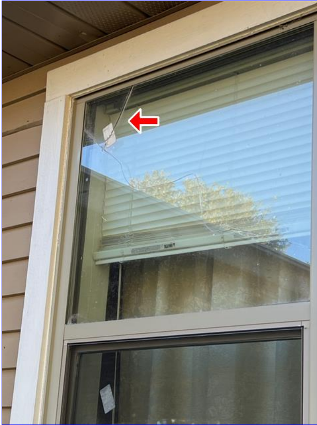
H. Photo 1(Picture) A window at the front of the home has a broken pane of glass.
