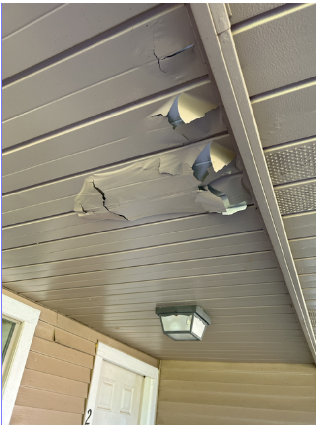
K. Photo 1(Picture) Paint is missing and peeling away under the front porch.
