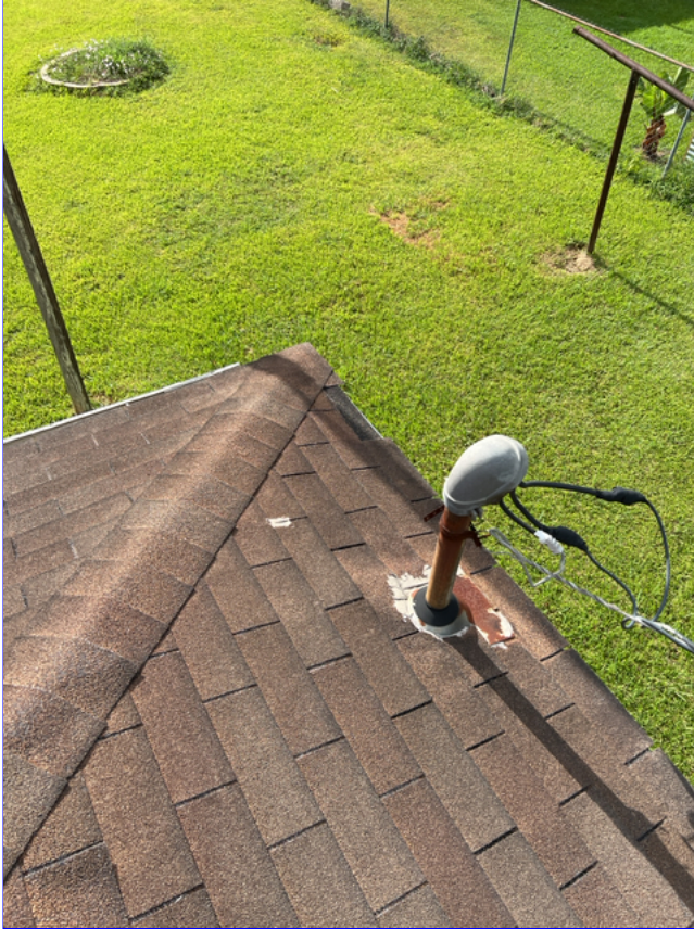
C. Photo 11(Picture) Several missing and damage shingles were observed on the roof.
