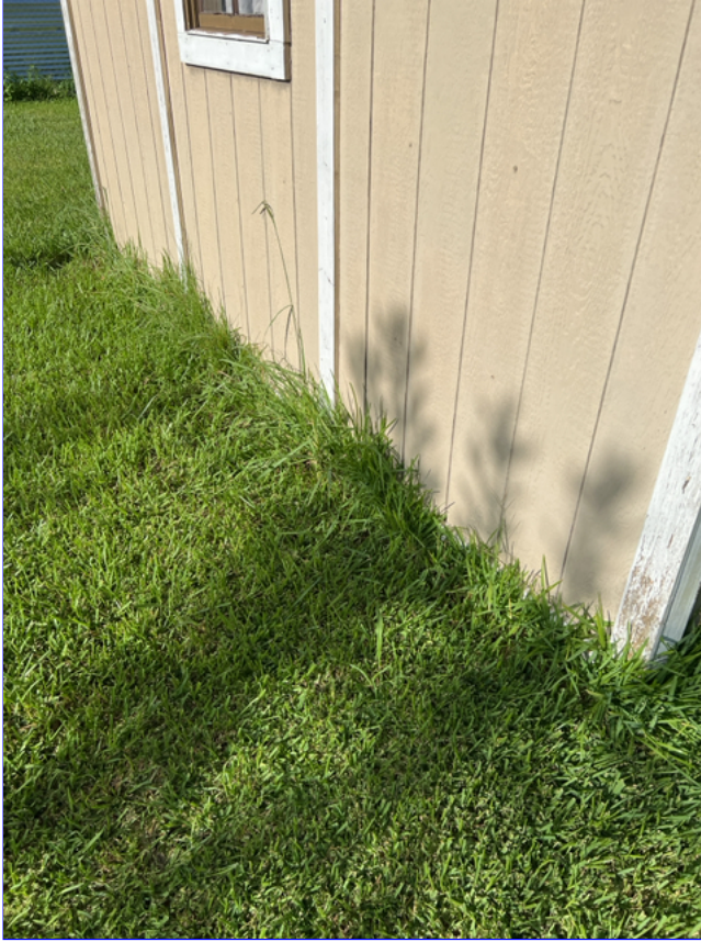
B. Photo 3(Picture) The grading and drainage around the garage is deficient.
