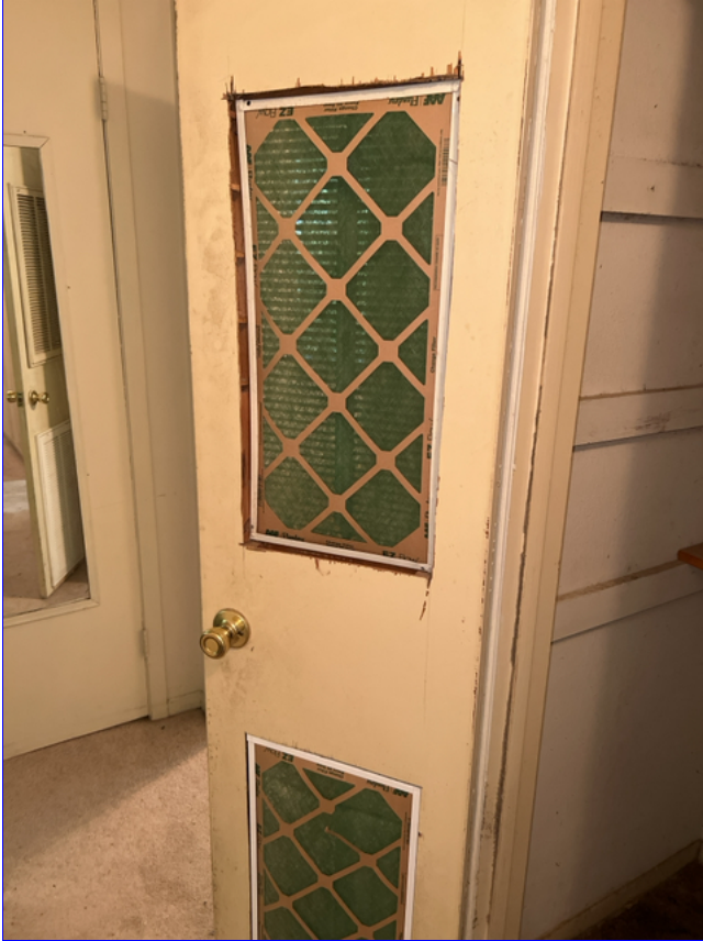
B. Photo 2(Picture) The hallway door has been cut out and filters have been installed.
