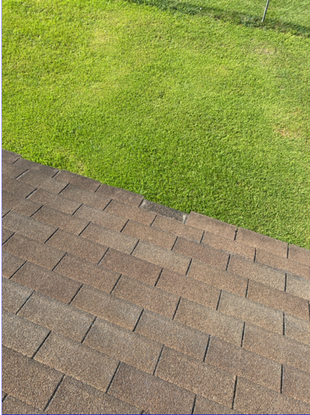
C. Photo 9(Picture) Several missing and damage shingles were observed on the roof.
