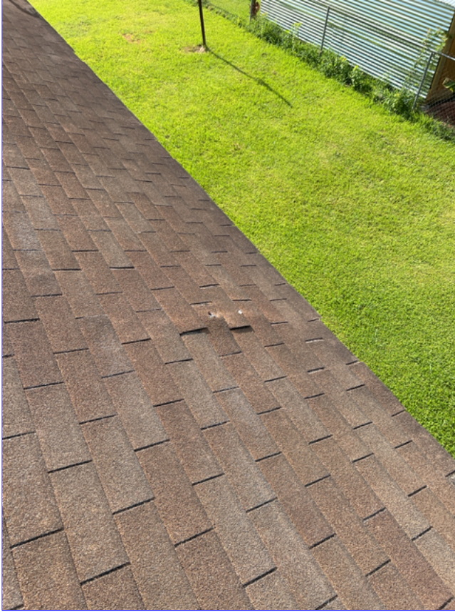
C. Photo 10(Picture) Several missing and damage shingles were observed on the roof.
