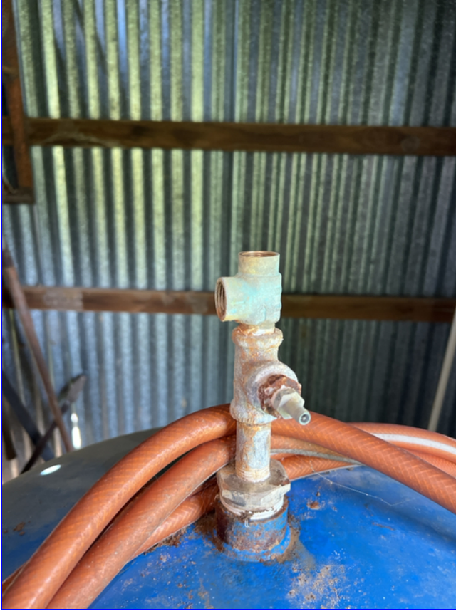
A. Photo 1(Picture) The water well is missing fittings at the top of the tank.
