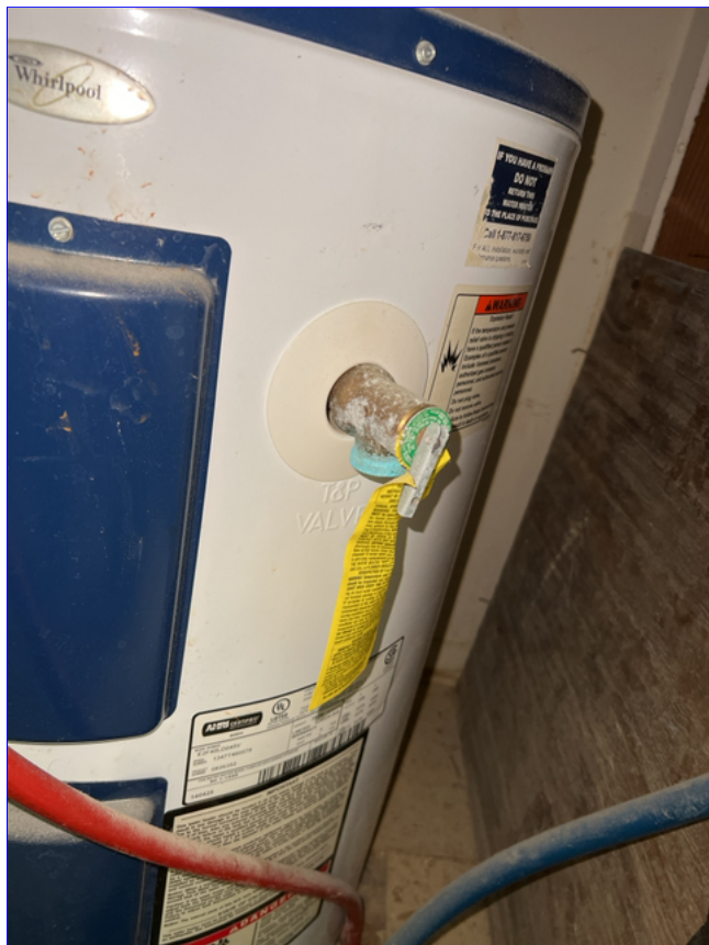
C. Photo 2(Picture) The T&P (Temperature and Pressure) relief valve on water heater
