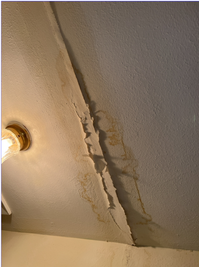
F. Photo 3(Picture) Water stains were observed to the ceiling in the front middle bedroom of the house.
