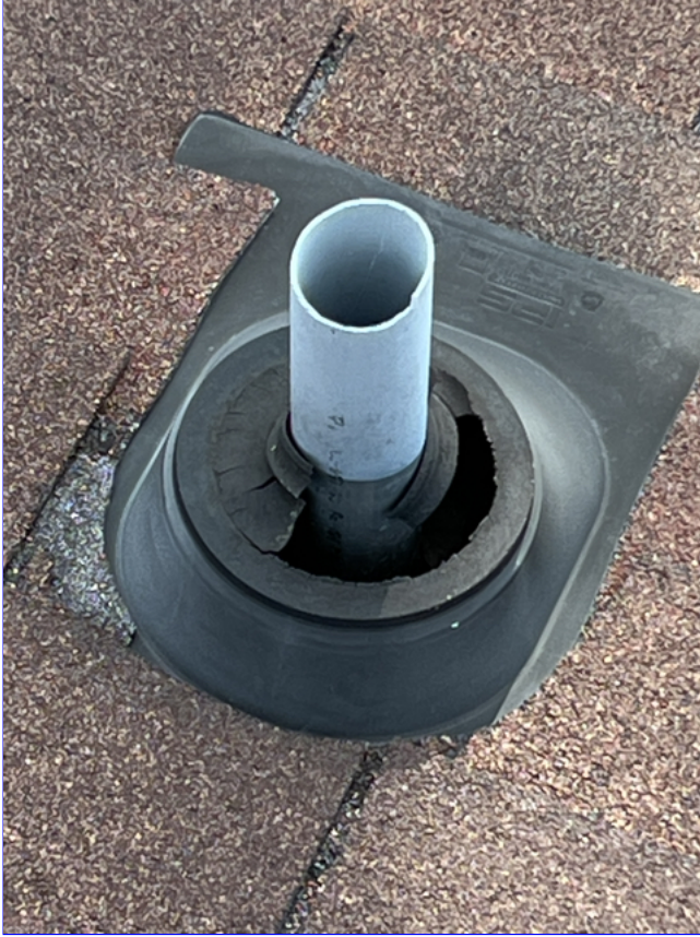
C. Photo 4(Picture) Both of the roof jacks above the kitchen area need to be replaced.
