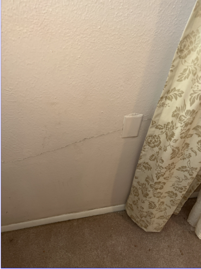
E. Photo 9(Picture) The drywall on the inside of the home has many structural cracks throughout.
