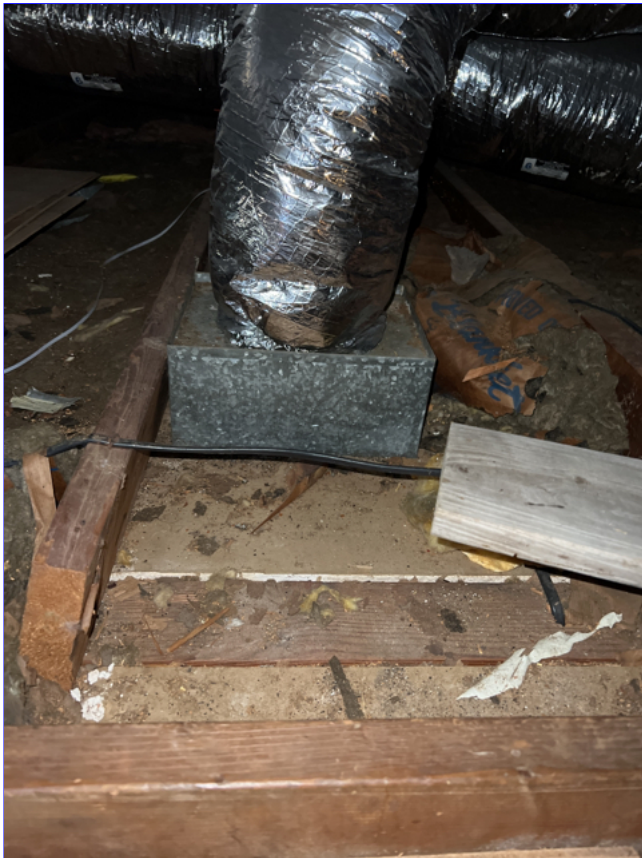
D. Photo 2(Picture) The insulation in the attic is matted down and no longer insulating as intended.
