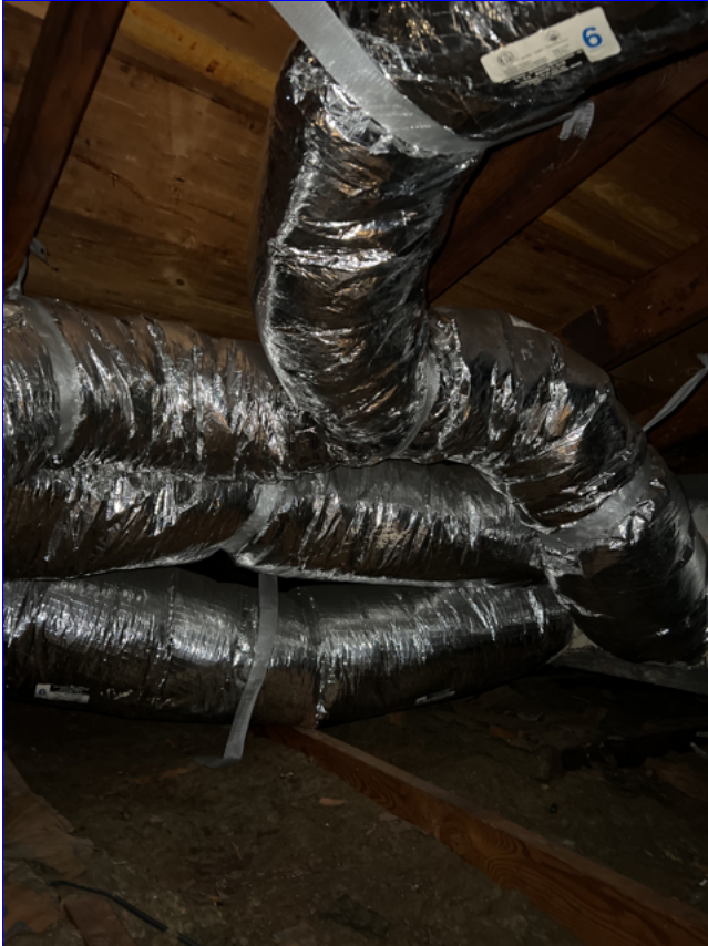
C. Photo 1(Picture) The ductwork in the home appears to have been replaced when the furnace was replaced.
