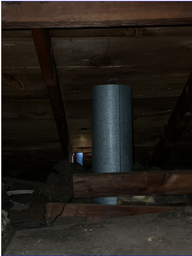
C. Photo 1(Picture) The vent piping for the range hood is terminating in the attic space.
