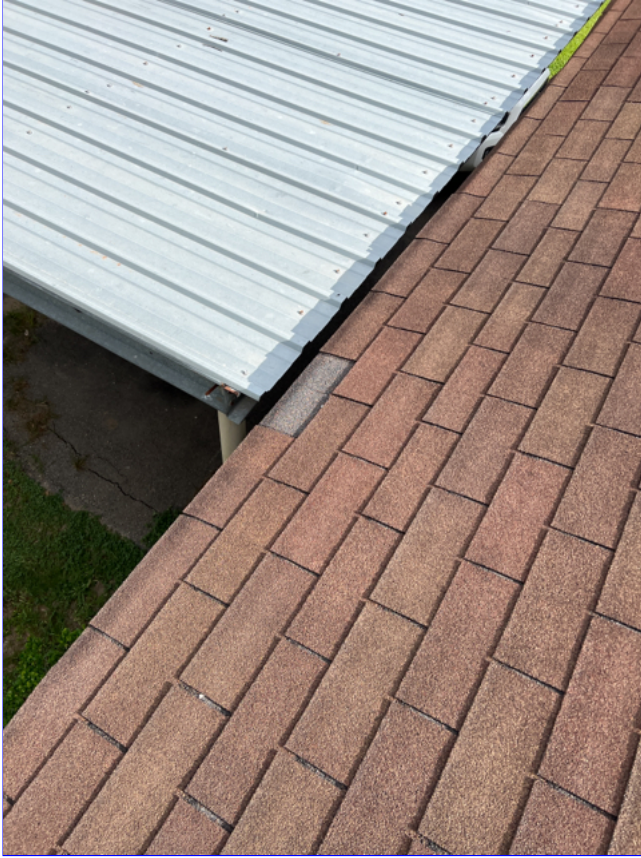
C. Photo 7(Picture) Several missing and damage shingles were observed on the roof.
