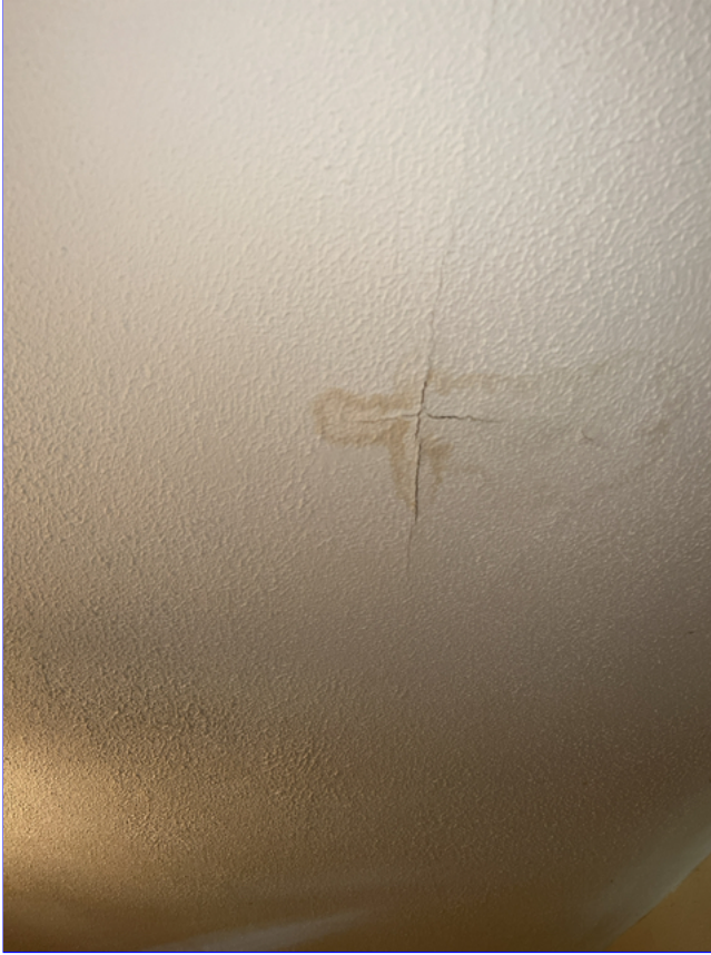
F. Photo 1(Picture) Water stains were observed to the ceiling in the front middle bedroom of the house.
