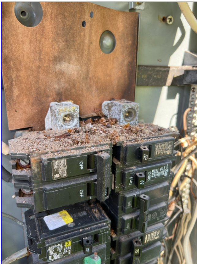
A. Photo 2(Picture) The main lugs and bus bar inside the electric panel are showing corrosion.
