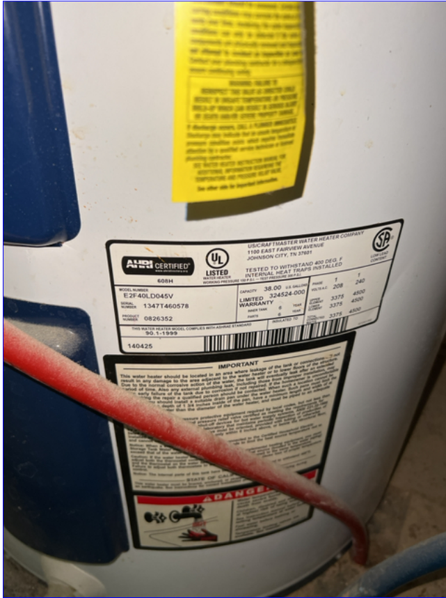
C. Photo 1(Picture) Water heater service tag.
