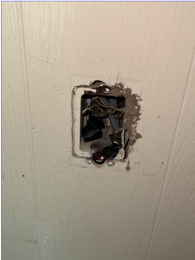
B. Photo 2(Picture) A missing electrical outlet was observed in the garage.
