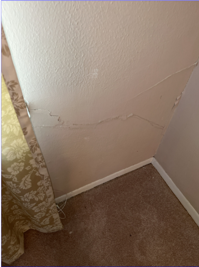
E. Photo 13(Picture) The drywall on the inside of the home has many structural cracks throughout.
