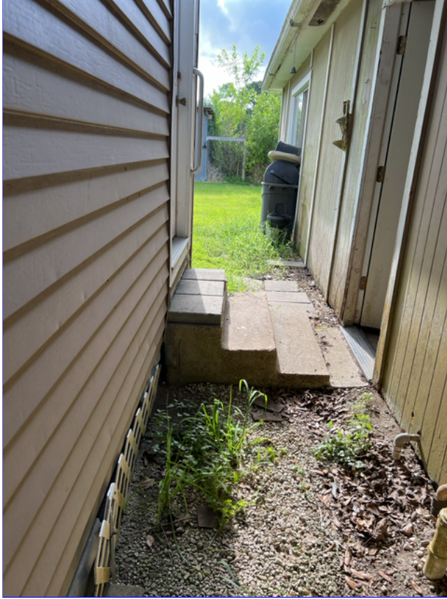
I. Photo 1(Picture) If more than three stairs are going into the home a hand rail is required.
