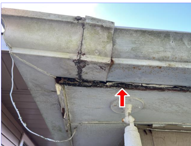
E. Photo 4(Picture) The fascia board behind the gutters on the garage is showing wood rot around most of the garage.
