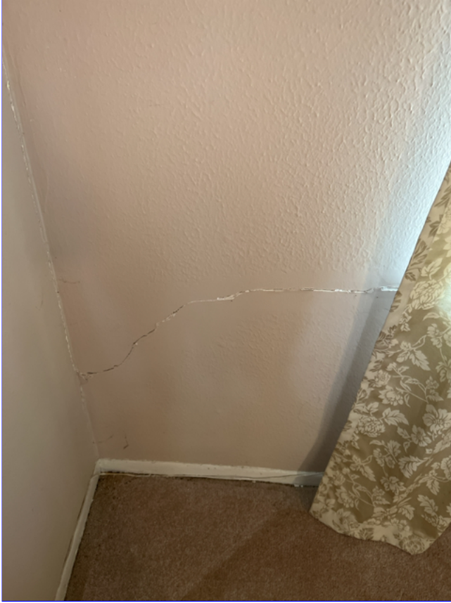
E. Photo 12(Picture) The drywall on the inside of the home has many structural cracks throughout.
