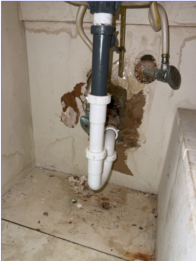
B. Photo 1(Picture) I did observe where the wall behind the bathroom sink was damaged during repair.
