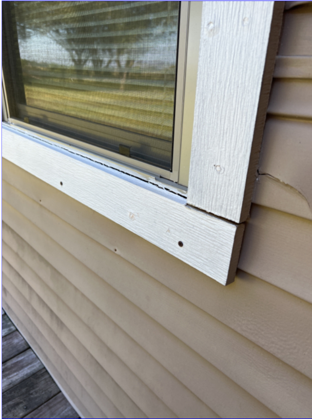
E. Photo 1(Picture) Separation in the trim around the windows was observed.
