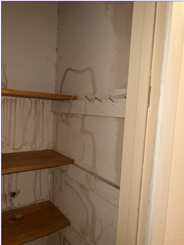
B. Photo 4(Picture) The interior space of this closet is showing moisture staining.
