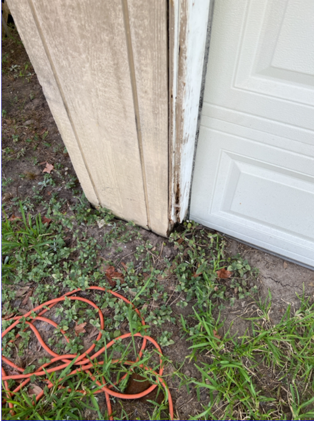
B. Photo 1(Picture) The grading and drainage around the garage is deficient.
