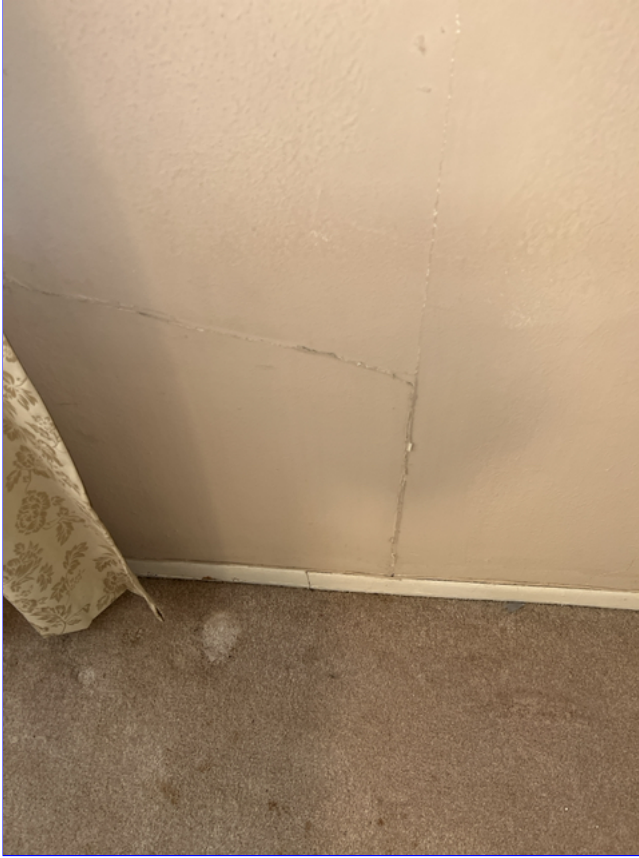
E. Photo 10(Picture) The drywall on the inside of the home has many structural cracks throughout.
