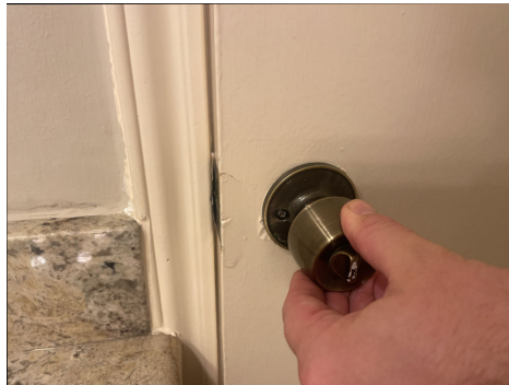
Door rubs the jamb; Bathroom
