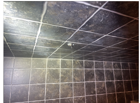
Secondary drain line draining into shower. Recommend servicing system.
