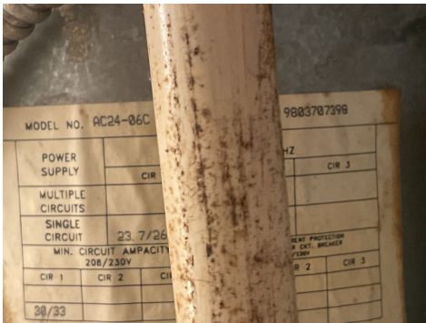
Evaporator coil data plate
