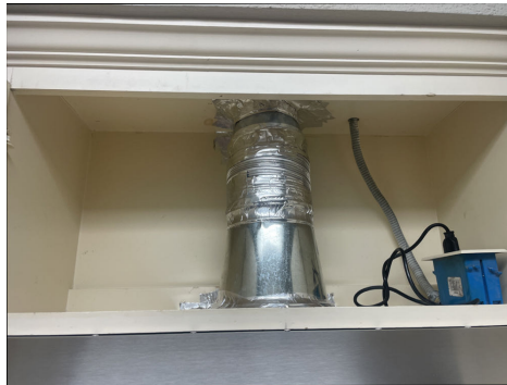
Improper vent material
