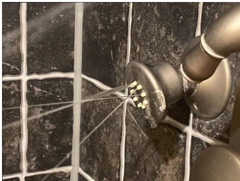
Spray jet clogged
