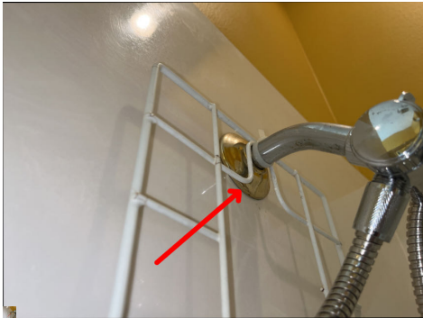
Bathroom 2: Caulk needed at escutcheon plate
