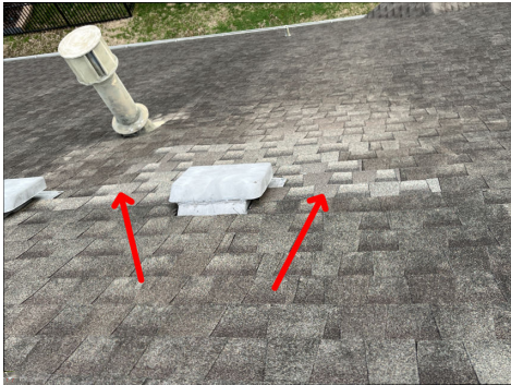
Evidence of prior repair
