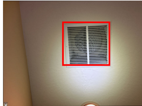
Missing filter at supplemental air returns
