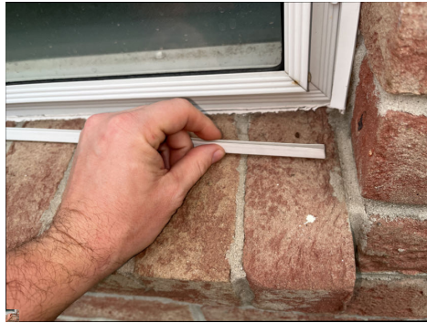
Left: Damaged weatherstripping
