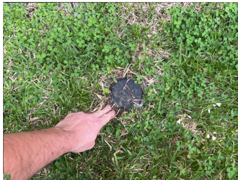
Bait stations: Evidence of previous termite treatment
