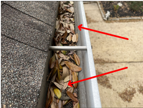
Debris in gutters
