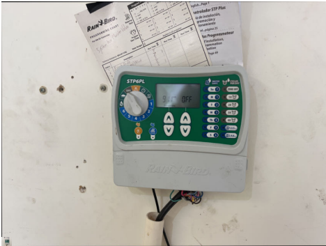
Garage: Controls to sprinkler system
