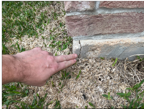
Left: Corner crack
