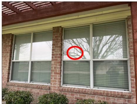
Bedroom 2: Damaged pane
