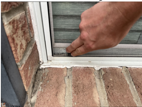
Front: Damaged screen
