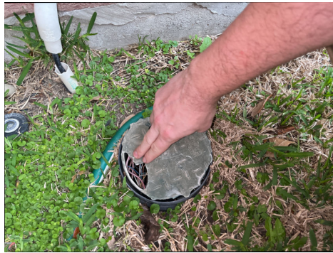
Left: Damaged valve cover
