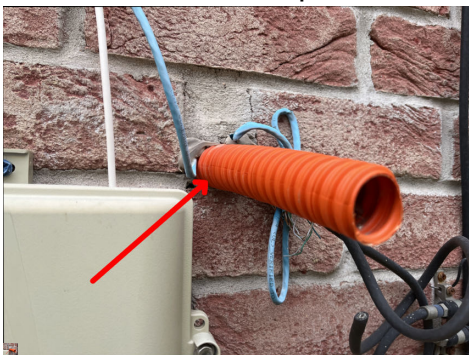
Around house: Deteriorated/insufficient caulk at wall protrusions
