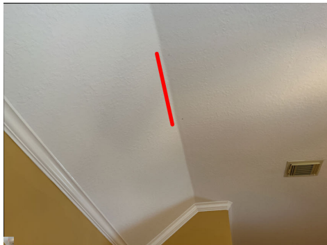
Bedroom 2: Hairline crack
