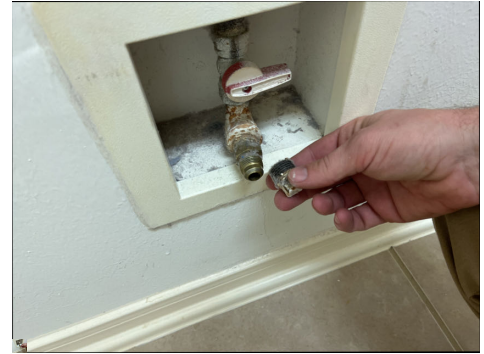
Laundry room: Uncapped gas line, wrong size cap
