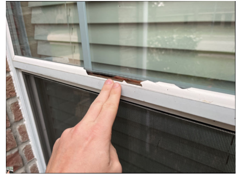
Front: Damaged weatherstripping
