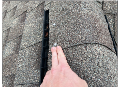
Exposed nail heads
