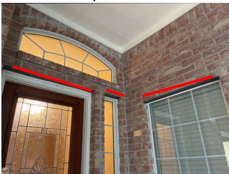
Front: Missing weep holes
