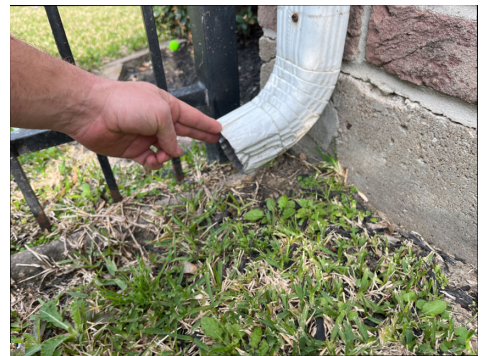
Downspout extension missing, discharge near structure
