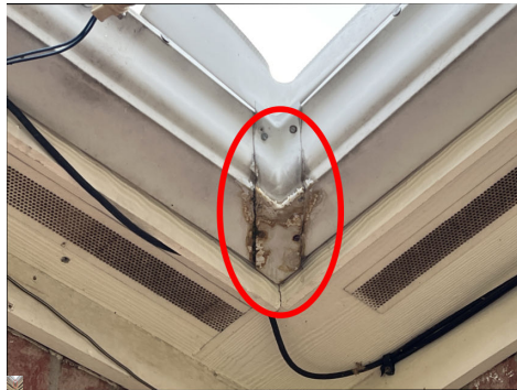
Left: Damaged/rusted gutter joint
