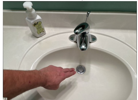
Bathroom 1: Drain stop did not retain water
