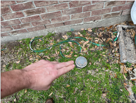
FYI: Main Cleanout located on the front left
