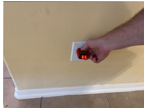
Living room: Outlet not GFCI protected
