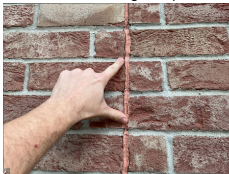
Left: Deteriorated caulk at expansion joint
