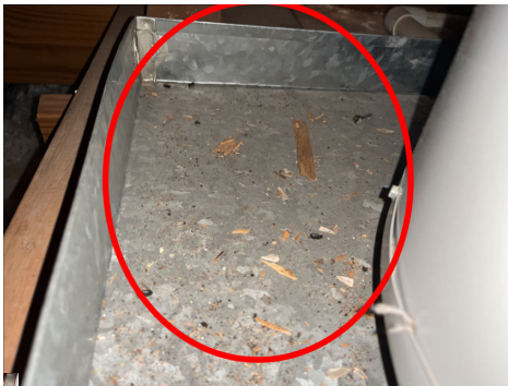
Debris in safety pan
