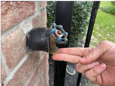
Rear right: Back flow preventer recommended
