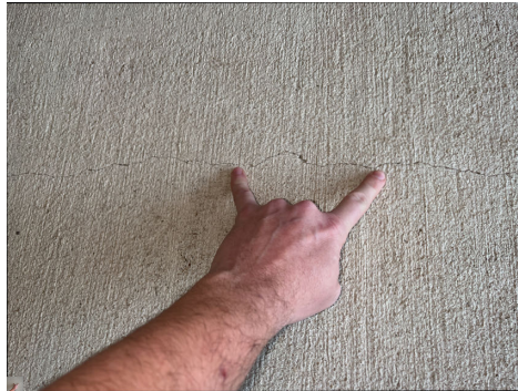
Porch slab: hairline crack
