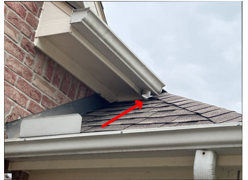
Downspout extension missing, discharge on roof
