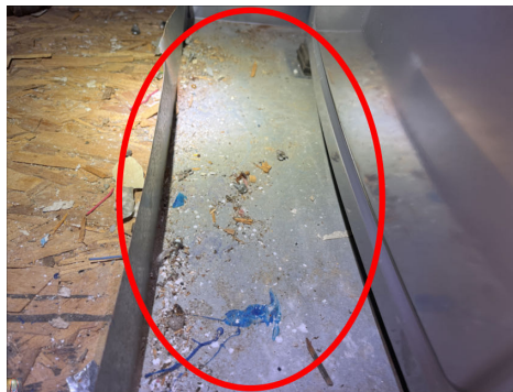
Debris in safety pan
