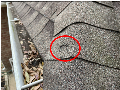
Front left: Damaged shingle
