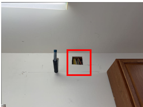
Garage: Hole in fire wall
