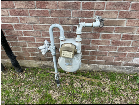
Right: Gas meter
