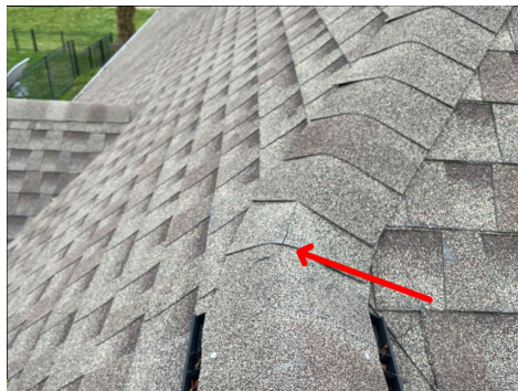
Left front: Damaged ridge shingles
