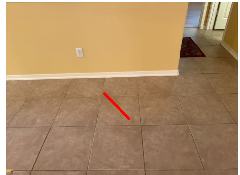
Entry hall: Cracked tile
