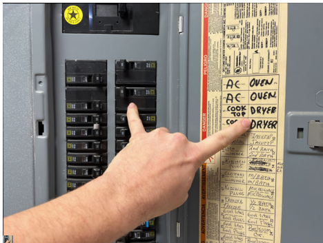
Dryer outlet: Not GFCI protected
