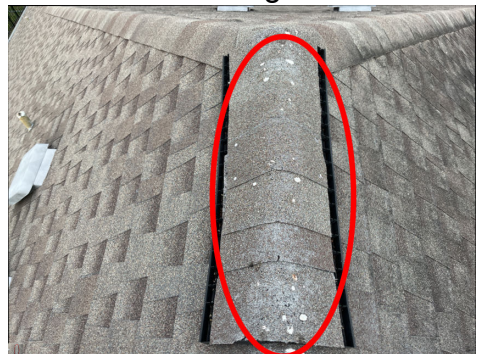
Top ridge: Granule loss/deterioration
