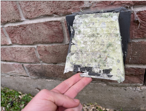
Right: Damaged damper
