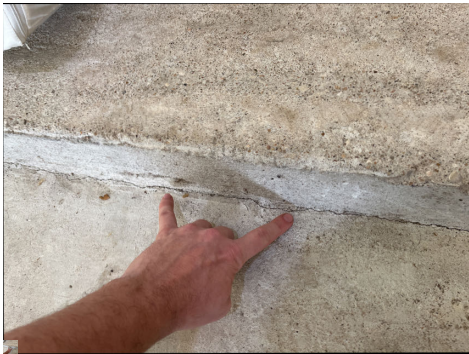
Garage: RTS hairline crack
