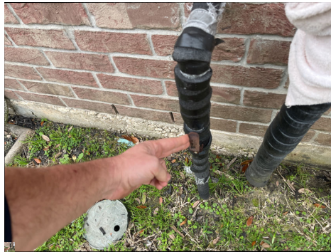
Right: Main Water Shutoff valve
