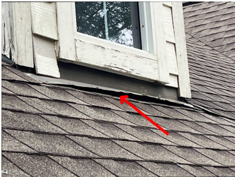
Front: Uplifted flashing
