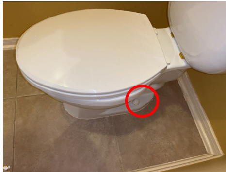
Bathroom 2: Loose toilet
