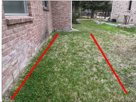
Around house: Insufficient grading/drainage
