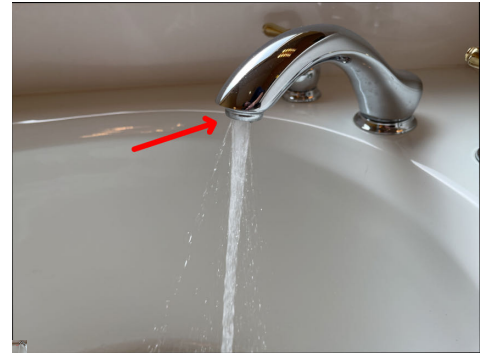
Bathroom 2: Blocked/dirty aerator
