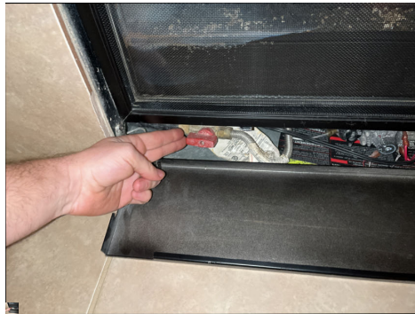
FYI: Fireplace gas valve
