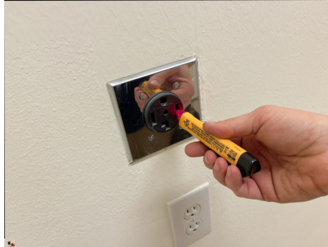
Laundry room: power confirmed at dryer outlet
