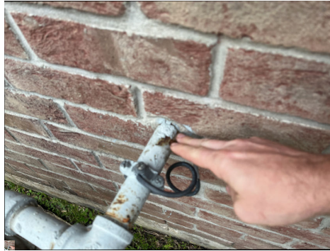
Gas meter: Rust on gas line
