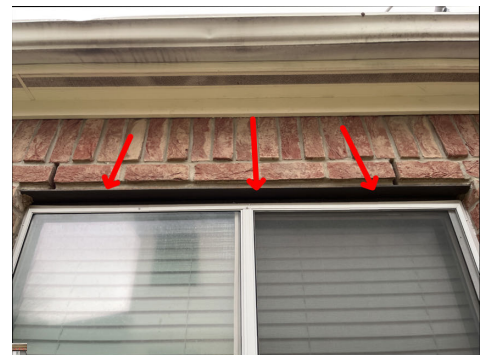
Around house: Rust on lintels
