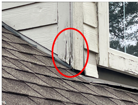
Front dormer: Wood decay at trim
