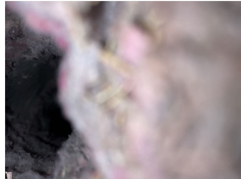
Dryer vent: Lint buildup
