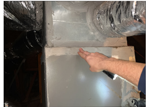
Attic: Evaporating coils sealed/unable to view coils
