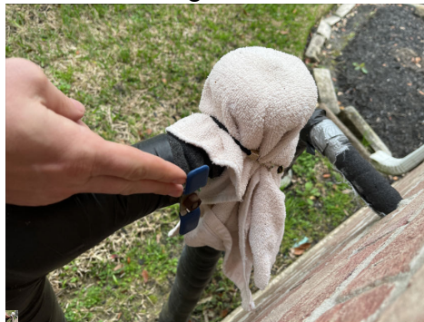
Backflow preventer off/winterized
