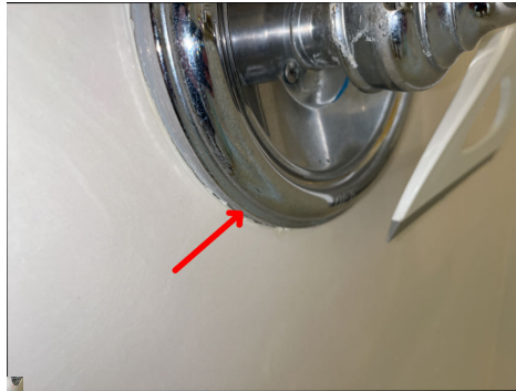
Bathroom 2: Deteriorated caulk
