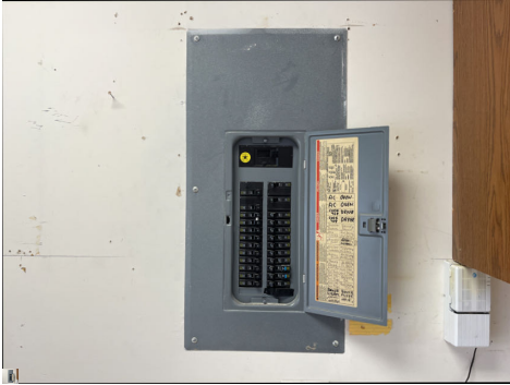
Garage: Square D service panel
