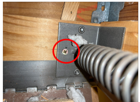
Improper fasteners used on attic stairs
