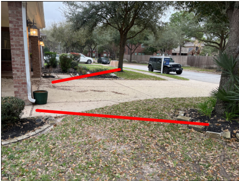
Front: Tree roots adjacent to foundation
