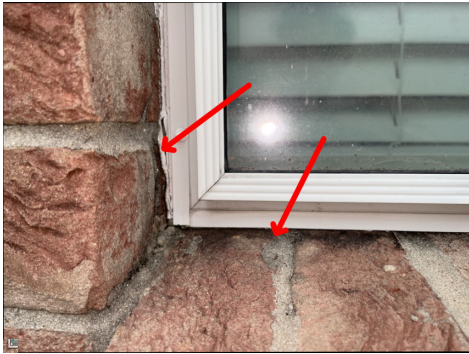
Around house: Deteriorated/missing caulk
