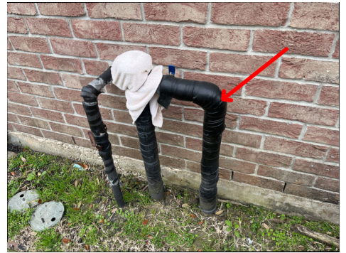
Right: Backflow preventer
