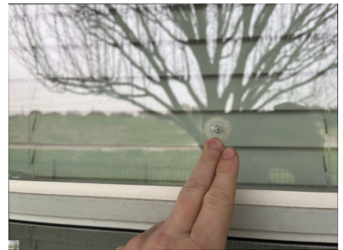
Bedroom 2: Damaged pane
