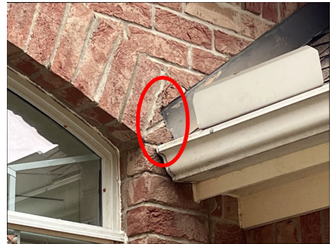
Missing kickout flashing
