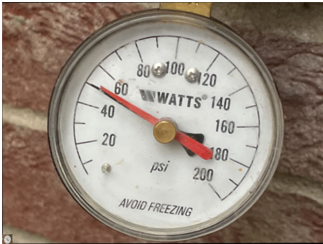
Static Water Pressure
