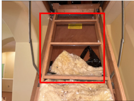
Pull-down stairs lacked sufficient insulation
