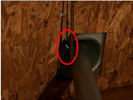
Daylight at roof protrusions
