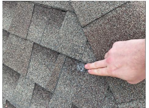
Various areas: Apparent weather damage
