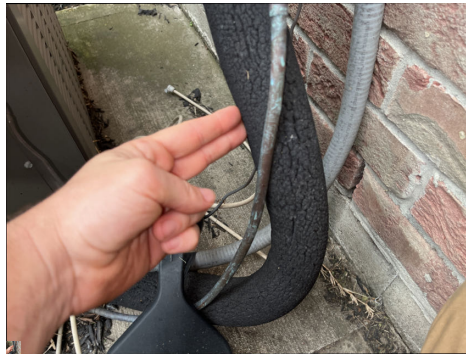
Old and deteriorated refrigerant line insulation
