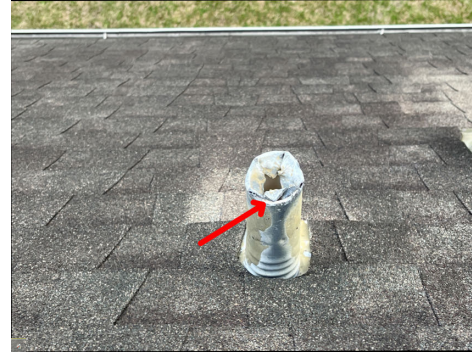
Damaged lead flashings
