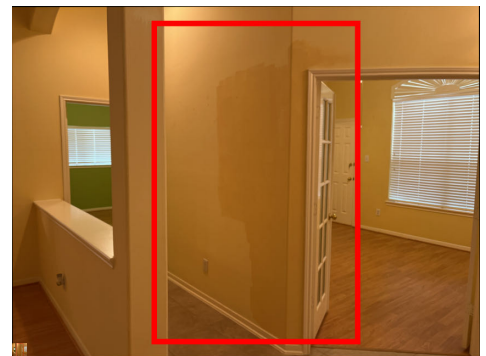
Foyer: Incomplete painting
