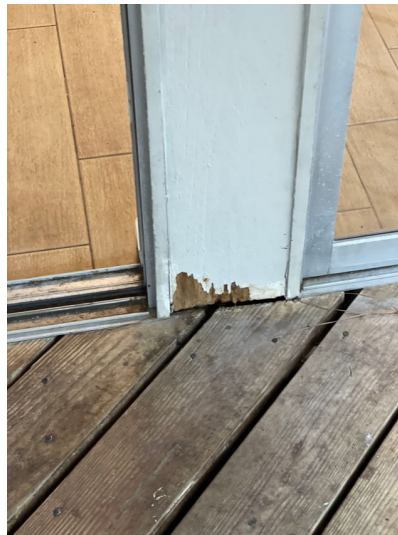
Damaged trim was noted at the back deck.
