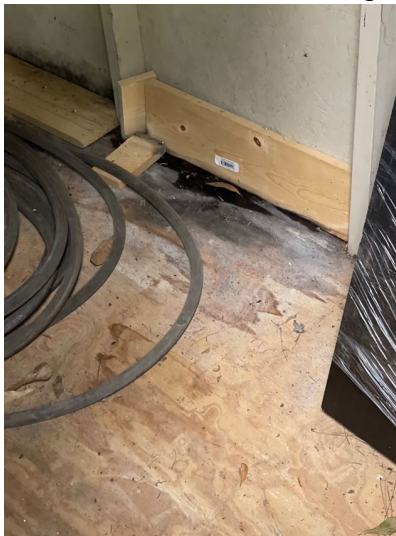
The rear storage shed had several areas of rotted flooring along with some siding damage.
