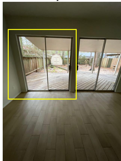
The left side living room sliding door would not open.
