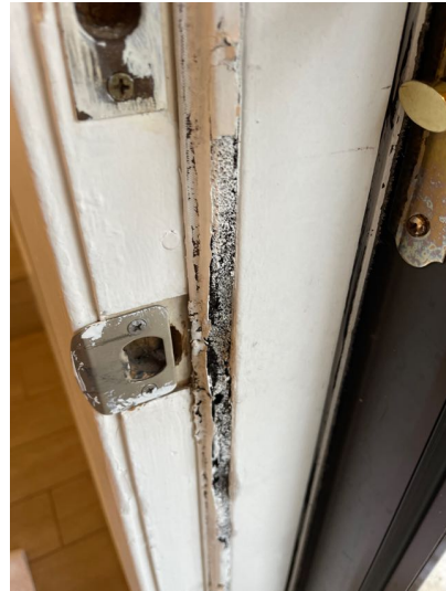
Weatherstrip was missing or worn at the front entry door.
