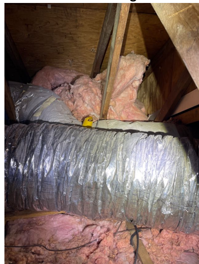
Structural Systems Roof Structure and Attic
