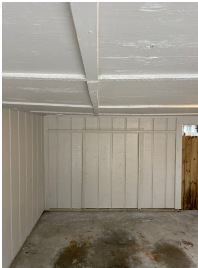
The ceiling in the carport area was sagging.
