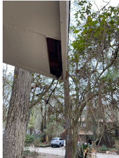
Soffit material was missing from the right front corner of the home.
