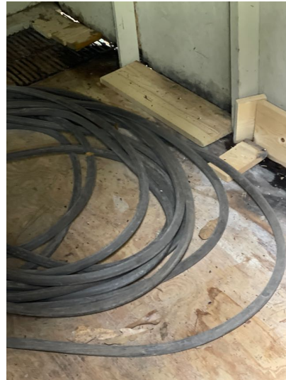
The rear storage shed had several areas of rotted flooring along with some siding damage.
