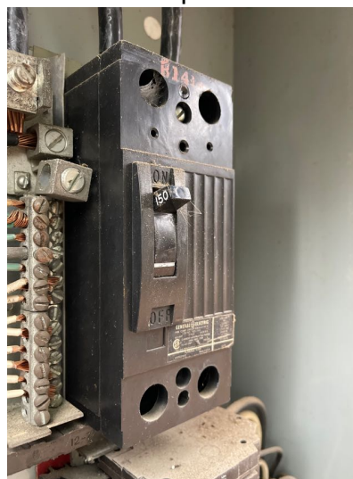
Electrical Systems Service Entrance and Panels
