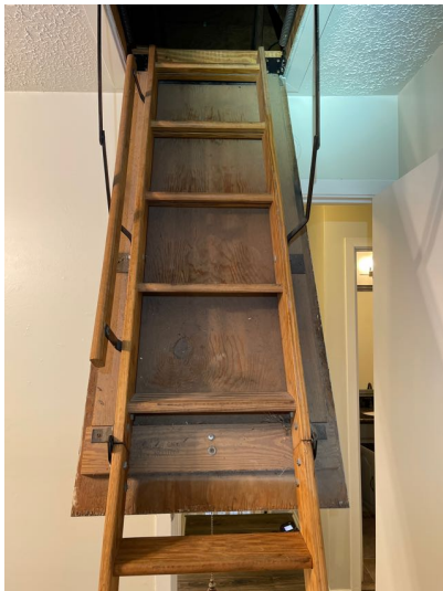
Attic access door was inadequately sealed and insulated.
