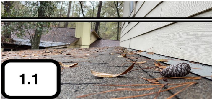
It appeared that improper roofing material was being used over the back patio cover. The slope of this roof area requires flat roofing material such as Modified Bitumen or single ply.
