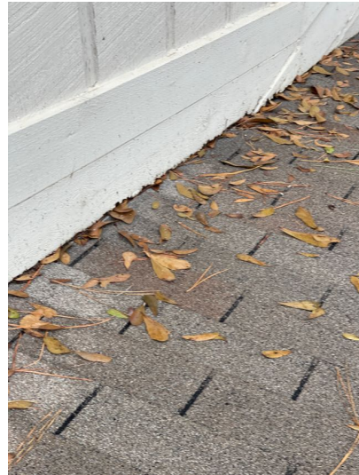
Siding was touching the roof surface at the left side of the home. In our opinion, siding should be at least 1" from the roof surface.
