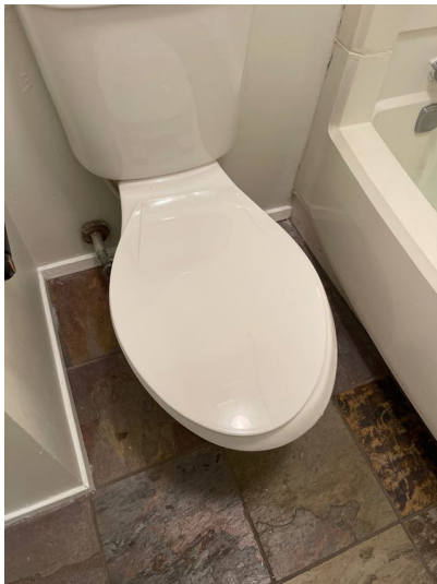
The toilet seat in the upper bathroom was loose.
