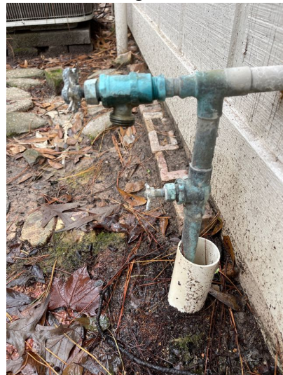
The left side hose bib was leaking.
