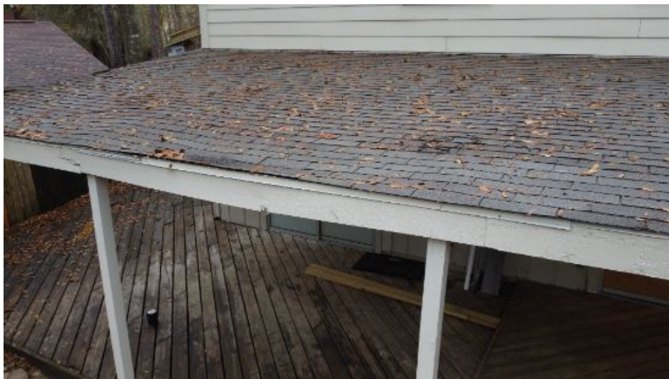
Rotted eave at the back deck cover.
