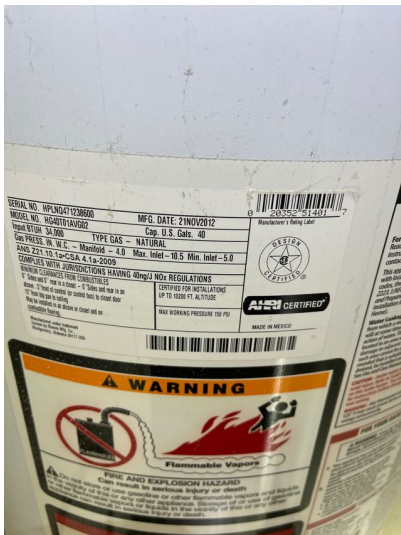
Water heater was gas powered and appeared to be manufactured by Rheem in 2012.
