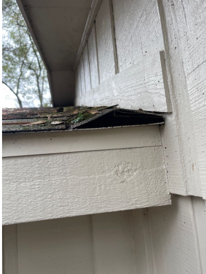
Flashing was lifted at the bottom of the vertical wall on the left side.
