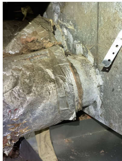
Duct work was aged and insulation exposed or missing in some spots.
