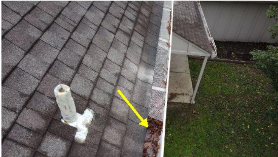
Gutters should be cleared to allow for proper drainage of rain water.
