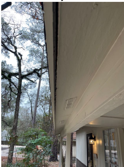
Soffit material was separated from the fascia in the front of the home.
