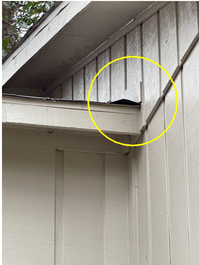
Kick out flashing were not observed a vertical wall and roof junctions.
