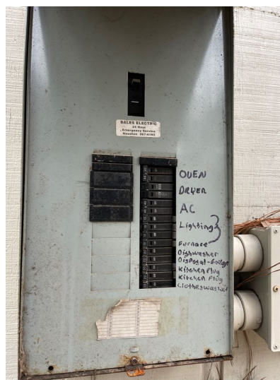
All breakers for the panel boxes and/or sub panels must be clearly and permanently labeled for identification of particular circuit.
