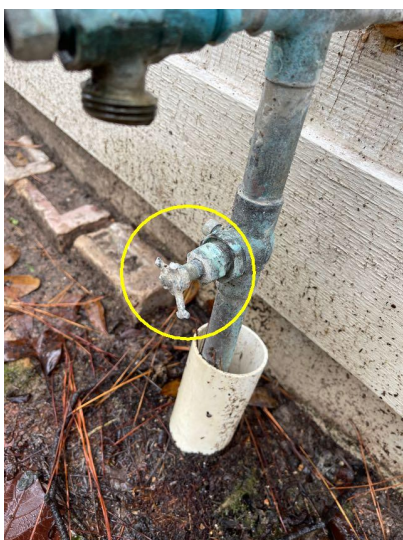
Main water valve handle was broken and unable to turn.
