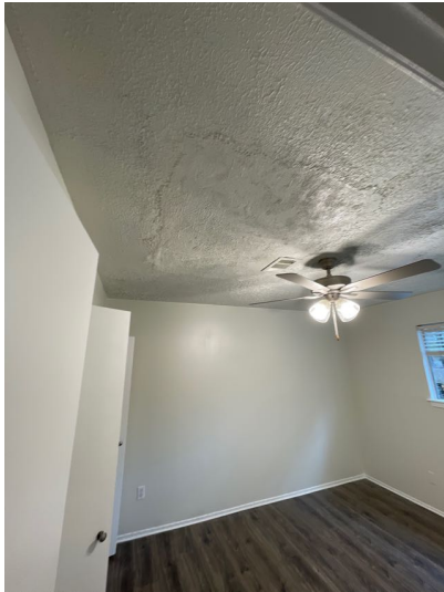
Evidence of drywall repairs were noted at the right front bedroom.
