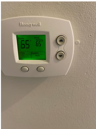
Thermostat was a Honeywell type digital non-programmable located in the stairway. This should be updated to meet current energy codes.
