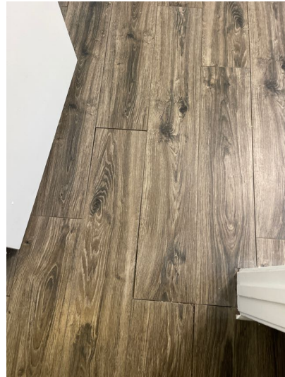
The flooring in the upper right bedroom was separated at the joints.
