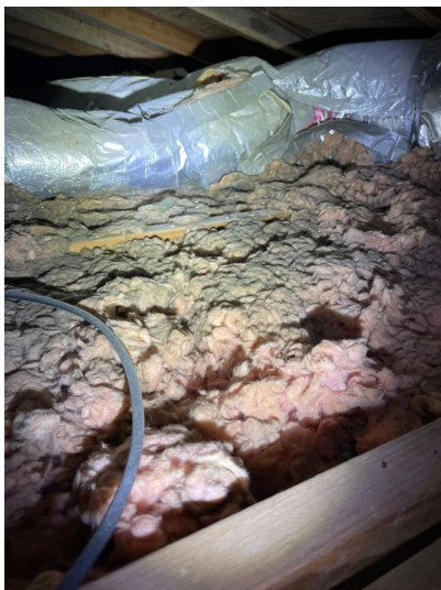
Low level of insulation and in need of improvement for better efficiency. Current efficiency standards are R38, and previously R30.
