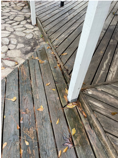
Rotten deck boards were noted in multiple areas.
