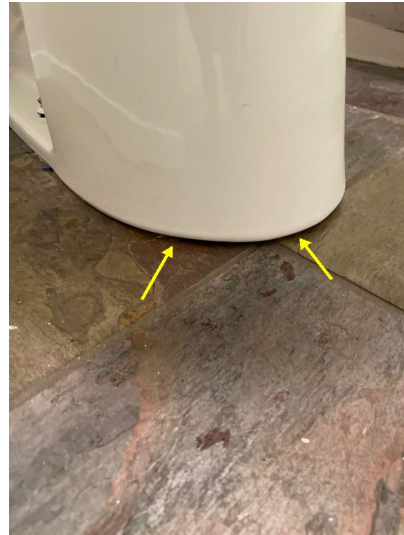
Where fixtures contact floors and walls (toilet bases, tubs, sinks) contact area should be water tight.
