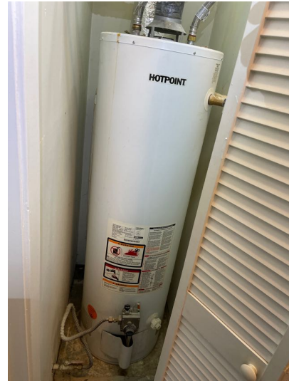
Gas fired water heater was located in the space adjacent to the upper bedroom and should be separated from the living space by a weather stripped self-closing exterior door and combustion air should be available from the exterior or attic.
