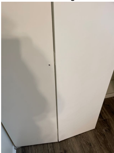
The pantry door and the upper bedroom closet bi-fold doors were missing a door handle.
