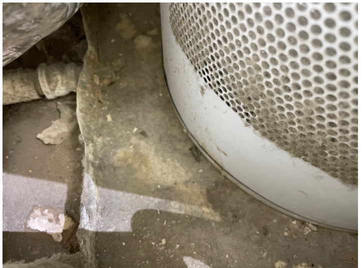
There was debris in water heater drain pan. This should be cleared to allow for proper drainage in the event of a leak.
