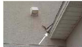
Fig 2: Improper installation (unsealed)
