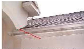
Figure 1: No kickout flashing
