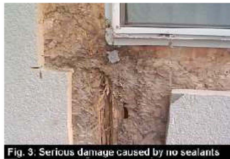
Fig. 3: Serious damage caused by no sealants
