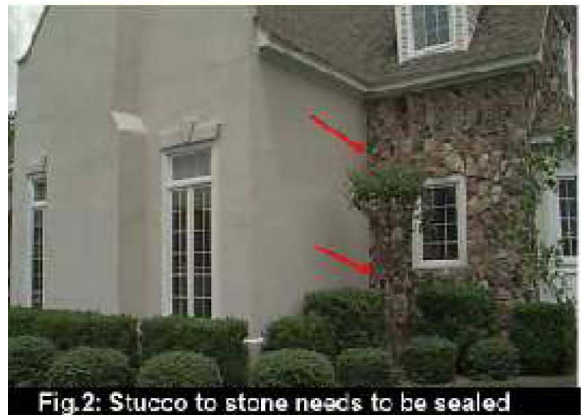
Fig.2: Stucco to stone needs to be sealed
