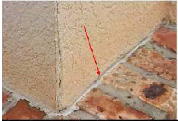
Fig.1: Stucco to brick transition needs sealing
