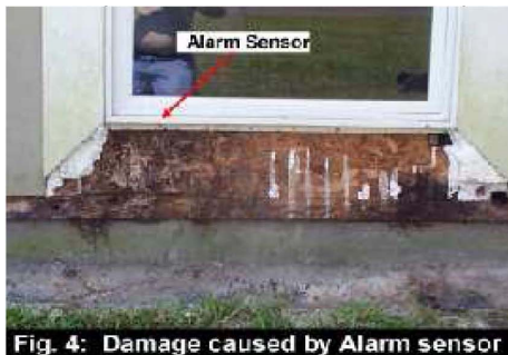
Fig. 4: Damage caused by Alarm sensor
