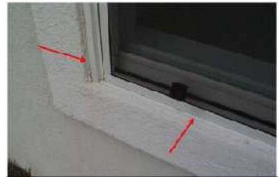
Fig. 2: Example of unsealed window perimeter
