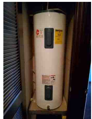
Hallway Hot Water Heater
