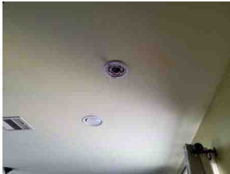
Primary BR Detector Missing
