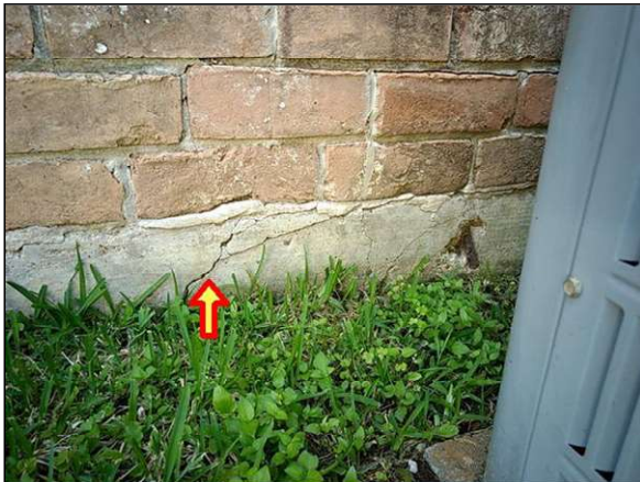
crack at foundation wall
