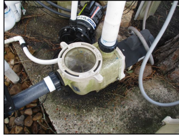
Pool filter pump
