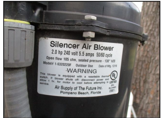
Air blower data plate
