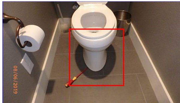
Caulking is missing around the base of the master bathroom toilet
