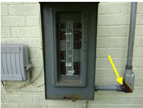
Conduit on the right and left side of home is not properly secured to wall and some areas have surface rust.
