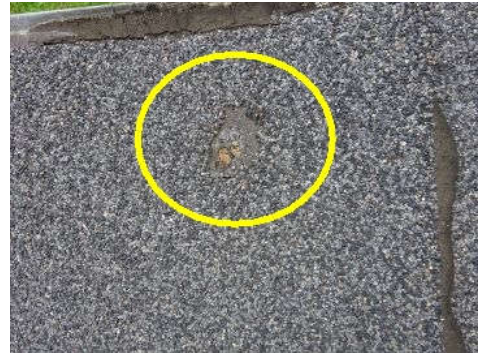
Observed mineral wear to surface of rolled roofing at rear enclosed porch in two locations.
