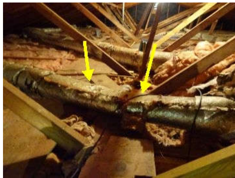
Partially collapsed duct in the attic at pathway.
