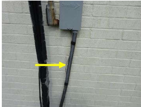
Flex conduit on the left wall of home below service disconnect for AC condensing unit is not properly secured to wall.
