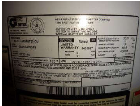
PLUMBING SYSTEM Water Heating Equipment
