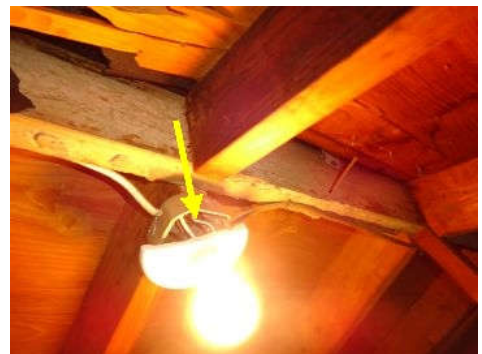
Damaged light fixture in the attic.
