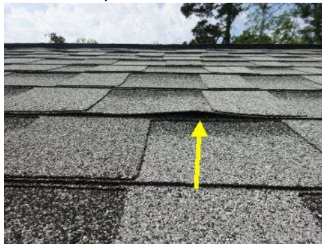
Observed a minor raised shingle on the front slope, generally a simple fix by a professional roofer.
