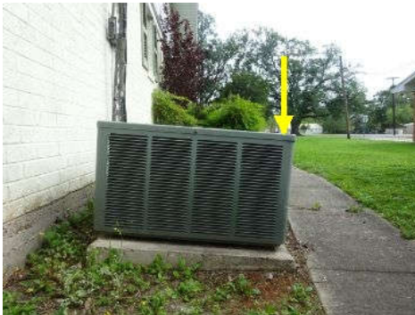
The exterior condensing unit is un level at time of inspection, unit should be level on its foundation / pad.
