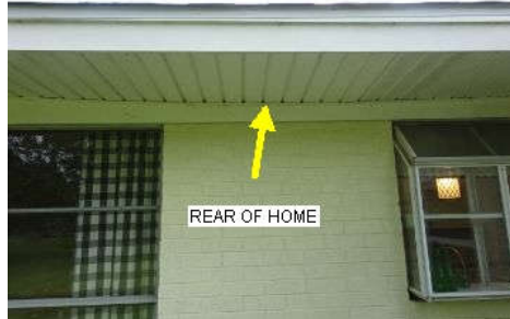
Sagging soffit vinyl in several locations.
