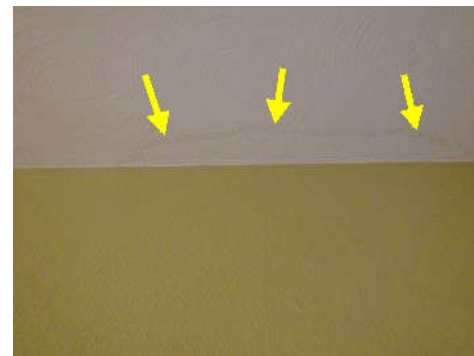
Observed a stain to ceiling in the hallway, however moisture levels are normal at time of inspection. Possible previous leak from drain pan under furnace.
