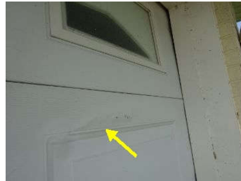
Doors have dents in several locations.
