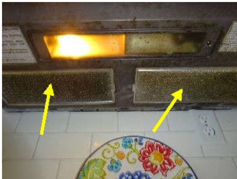
Filters are dirty and need cleaning.
