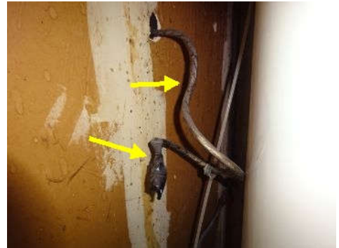
Non standard termination of romex in the water heater closet should be in protective junction box for safety reasons.
