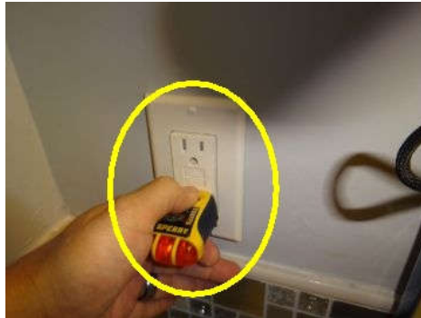
The GFCI receptacles in the master bathroom did not trip when tested with external tester.
