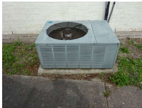
HEATING, VENTILATION AND AIR CONDITIONING SYSTEMS Cooling Equipment
