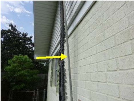
Conduit on the right and left side of home is not properly secured to wall and some areas have surface rust.
