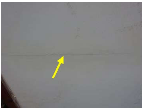
Observed loose tape seams / hairline separation at sheetrock tape seams in the garage, this is generally common due to the garage is not climate controlled.
