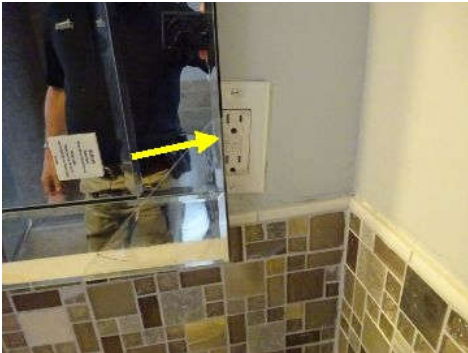
The right GFCI receptacle in the master bathroom is blocked by mirror.
