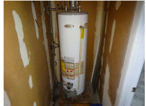
PLUMBING SYSTEM Water Heating Equipment
