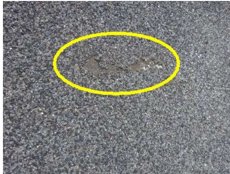
Observed mineral wear to surface of rolled roofing at rear enclosed porch in two locations.
