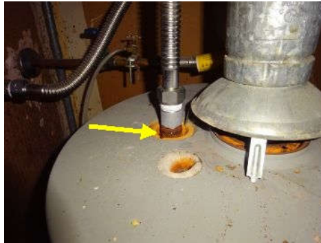
Observed surface rust to upper supply fitting atop water heater.
