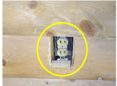
Replace all missing / damaged cover plates at receptacles and switches.
