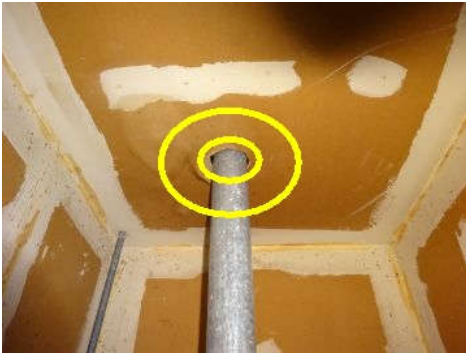
Missing heat shield at ceiling for gas vent stack.
