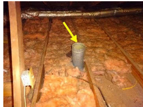
Vent hood terminates in the attic, this type should terminate to the exterior of home to meet "current industry standards".
