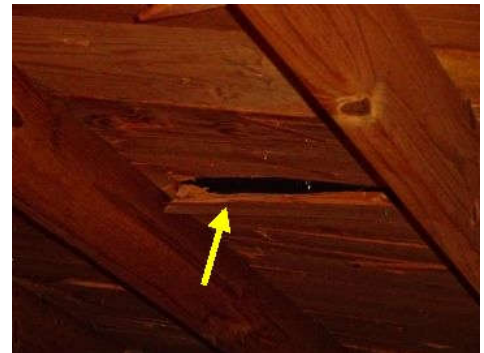
Observed several minor damaged decking boards, this is a common occurrence when installing a new roof on an older home and generally not a major concern
