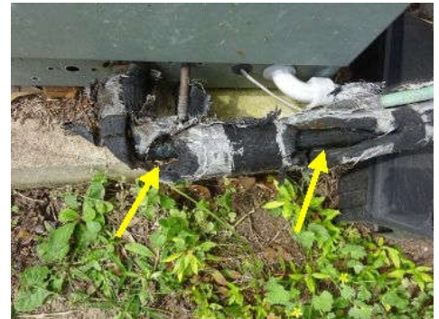
Missing / worn insulation at suction line at exterior AC unit.
