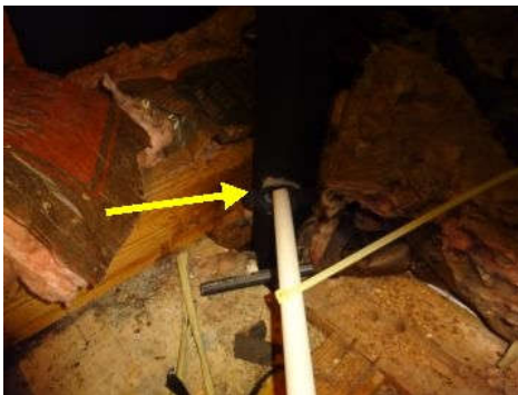
The primary drain line from coils terminates through side of cast iron plumbing vent stack in the attic, its required to terminate to approved location.
