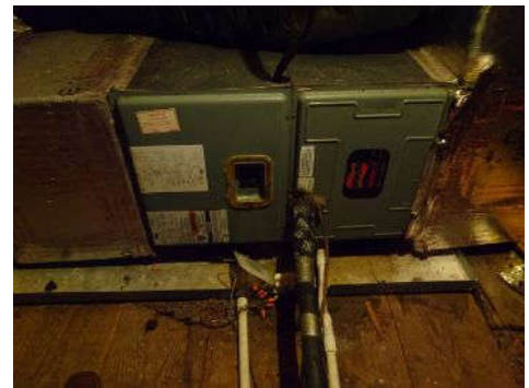
HEATING, VENTILATION AND AIR CONDITIONING SYSTEMS Heating Equipment
