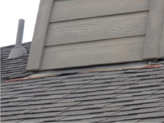
Damaged and rusted chimney flashing
