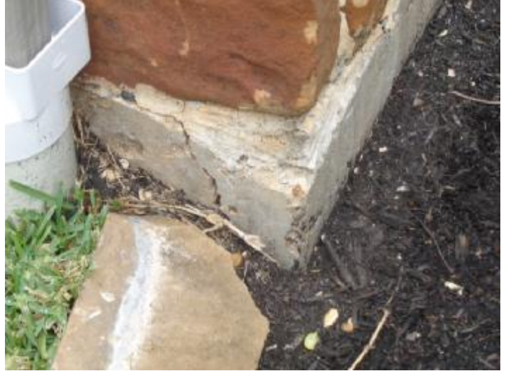
Left front corner of concrete slab foundation cracked
