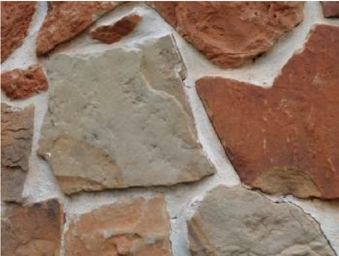
Cracks at stone mortar at left side
