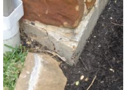
Popped corner left front
