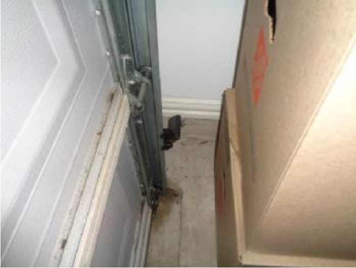
Electronic eye sensors installed to high from garage floor
