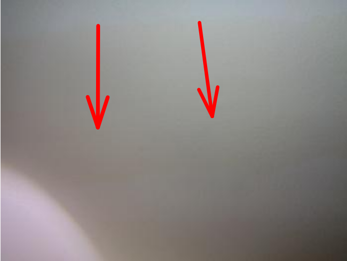
Water stains at upstairs hall ceiling
