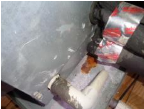
Rust in pan
