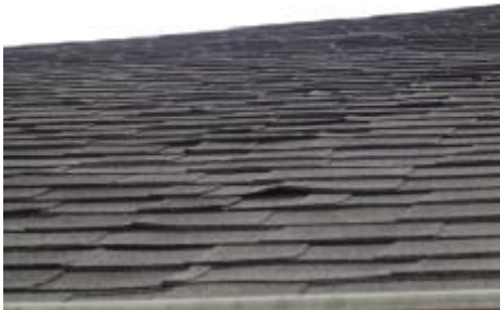
Roof raised shingle
