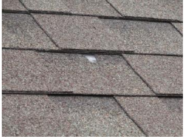
Granular/aggregate loss at roof surface - Damaged shingle
