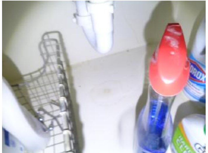
Evidence of leakage under sink in 2nd floor hall bath
