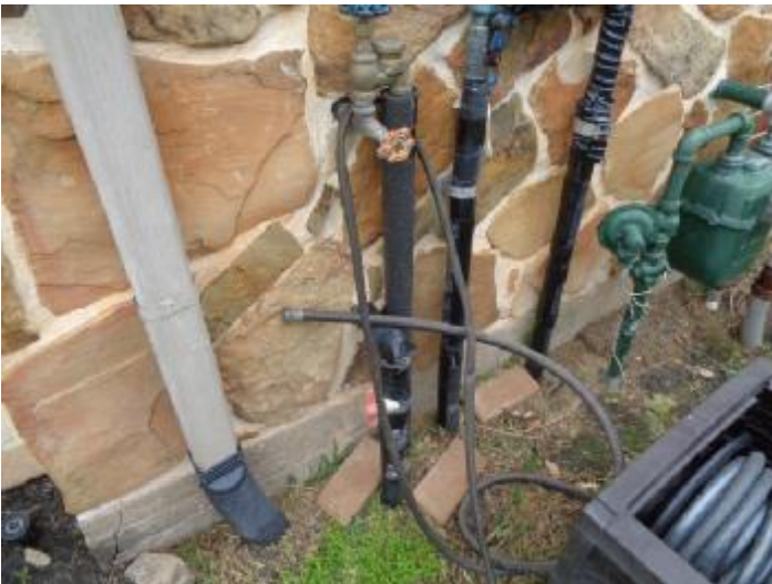
Main water shut off
