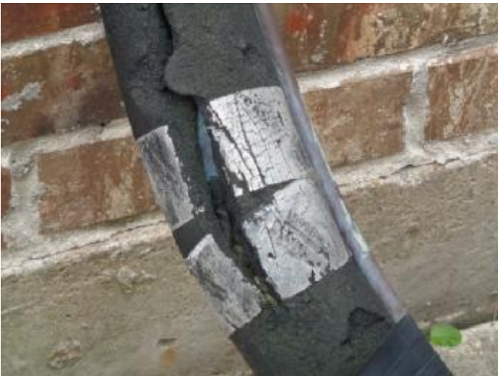
Damaged insulation on refrigerant line at air conditioner #2
