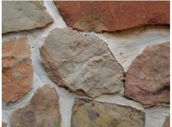
Cracks at stone mortar at left side
