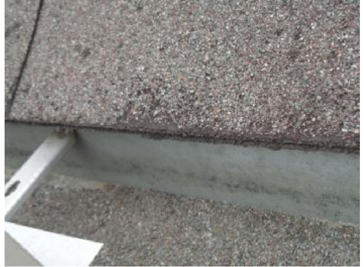
Granular/aggregate loss at roof surface
