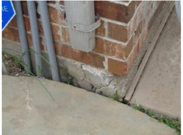
Rear right corner of concrete slab foundation cracked - Downspout lacks an elbow and extension
