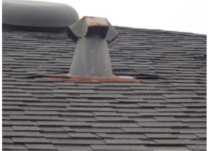
Rusted vent flashing
