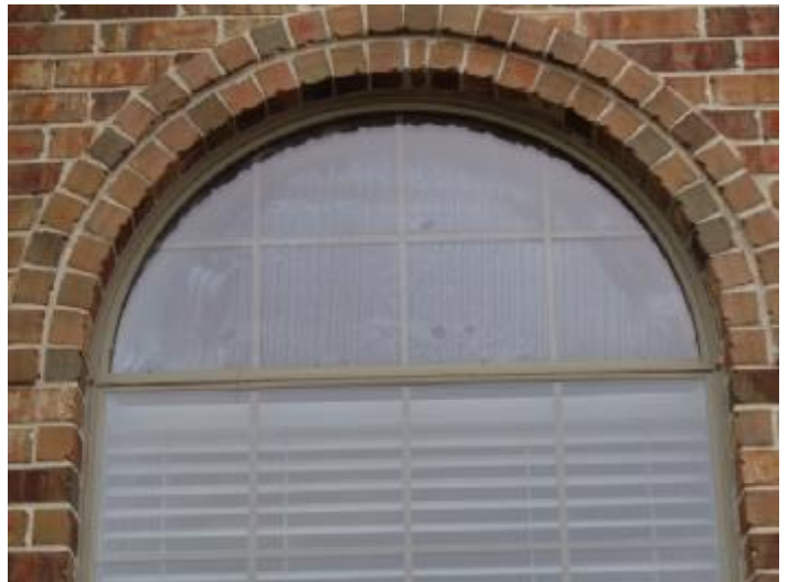
Breached thermopane window seal at front
