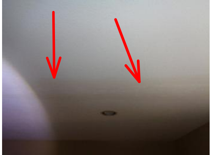
Water stains at upstairs hall ceiling
