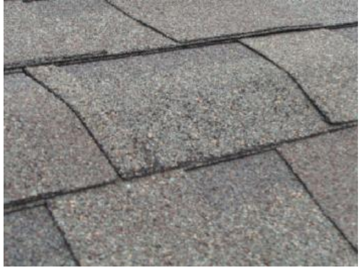
Granular/aggregate loss at roof surface
