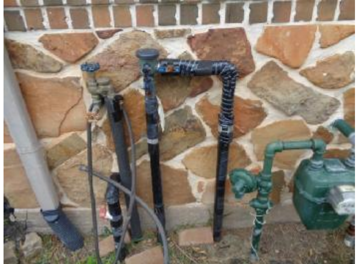
Sprinkler system backflow prevention device
