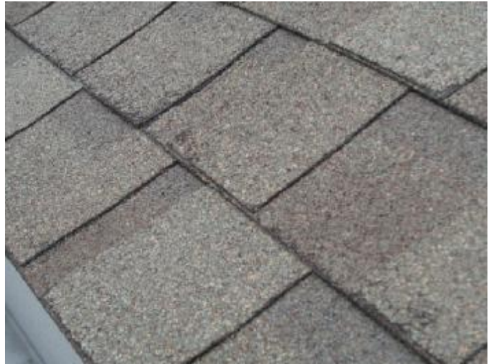
Granular/aggregate loss at roof surface
