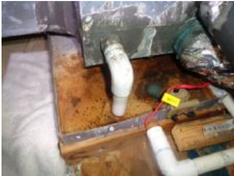
Rust in pan
