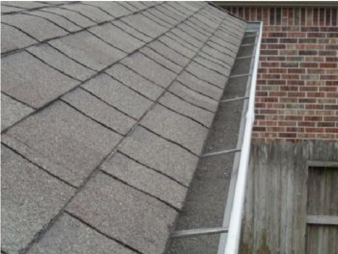
Gutter clogged with debris
