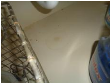
Leak under sink
