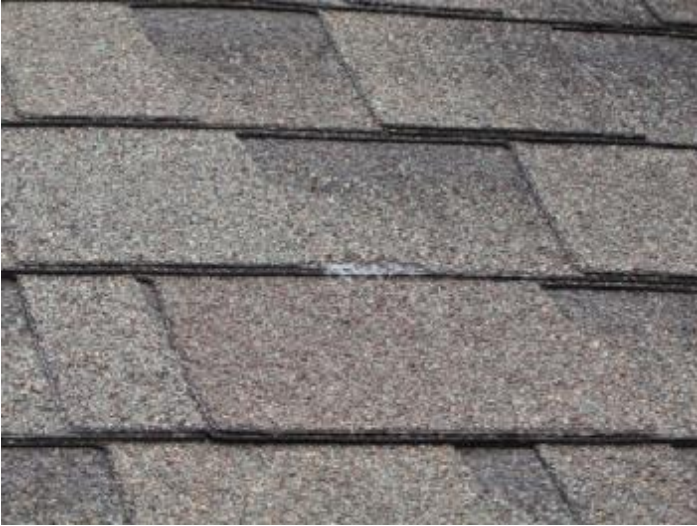
Granular/aggregate loss at roof surface
