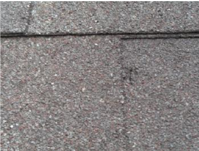
Pitting at rear of roof
