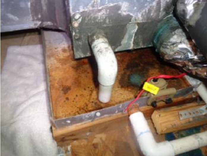
Rust in drain pan under furnace #2 in attic
