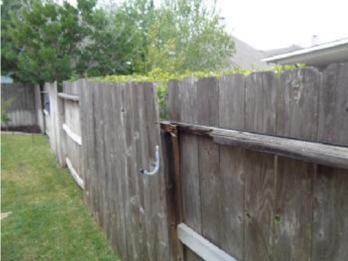
Yard fence is damaged/rotted
