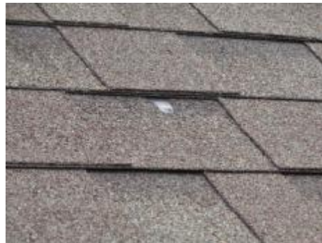
Roof aggregate loss
