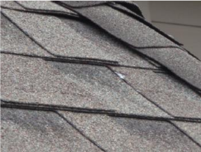
Granular/aggregate loss at roof surface - Damaged shingle
