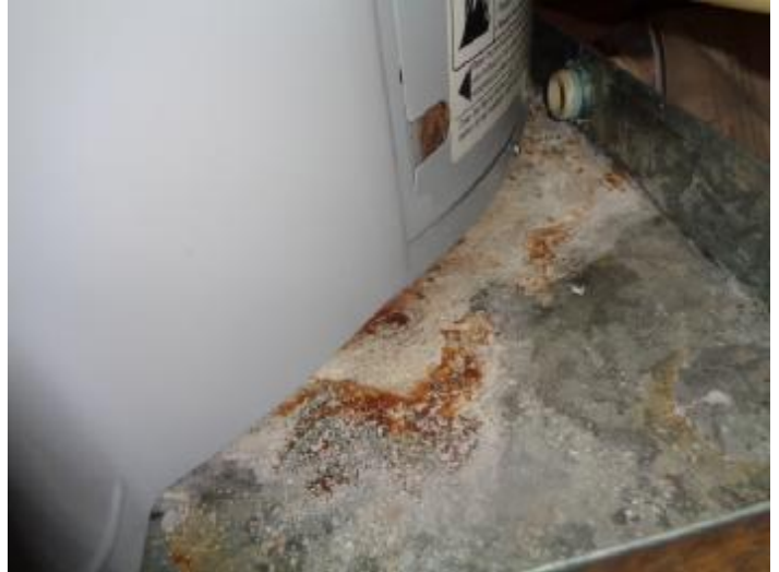
Rust in drain pan under water heater #2 in the attic
