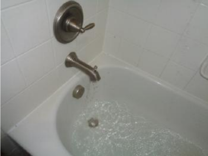
Shower diverter does not direct all water to shower head when in shower position in 2nd floor hall bath
