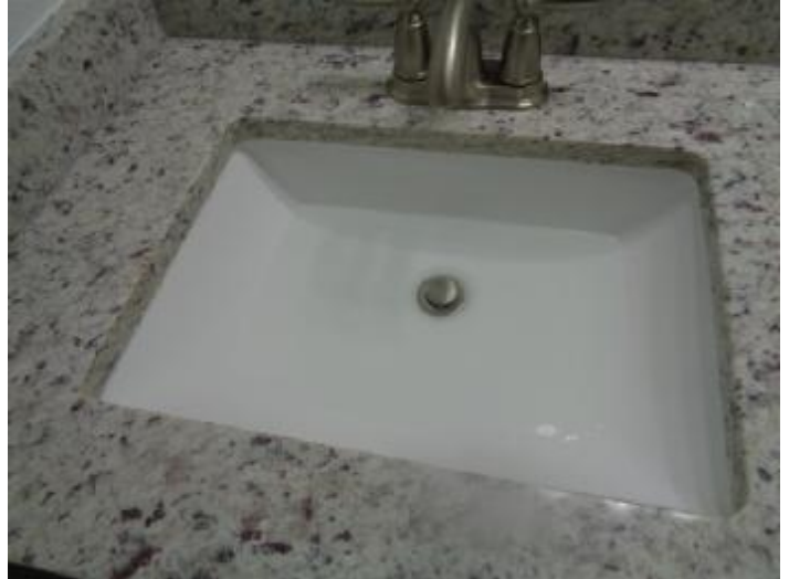
Drain stopper inoperative at sink in 2nd floor hall bath
