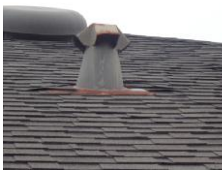
Rusted vent pipe
