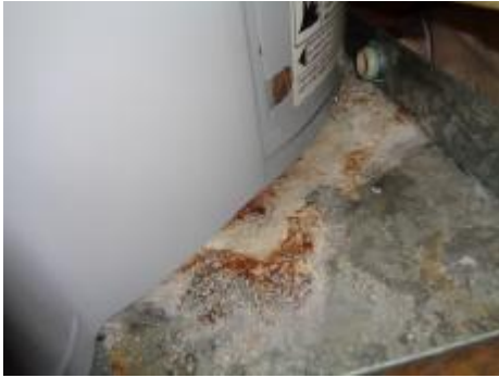
Rust in pan
