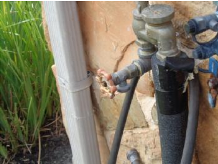
Right front hose faucet lacks an anti-siphon device
