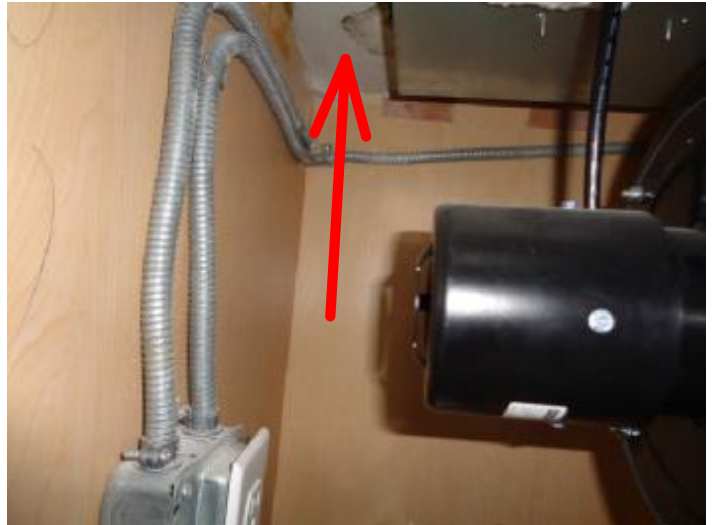
Suspected fungal growth in the cabinet below the stovetop at the top of the cabinet
