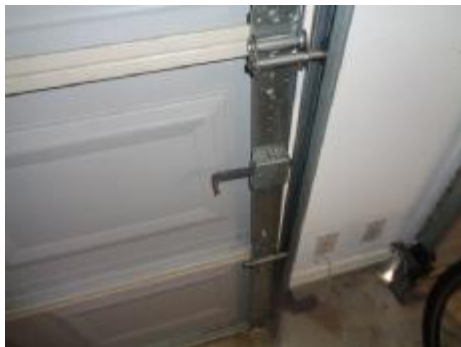
Garage bolt lock
