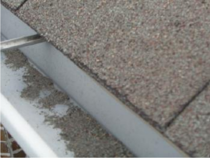
Granular/aggregate loss at roof surface
