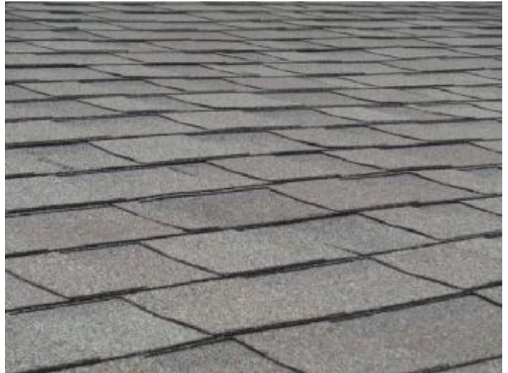
Granular/aggregate loss at roof surface
