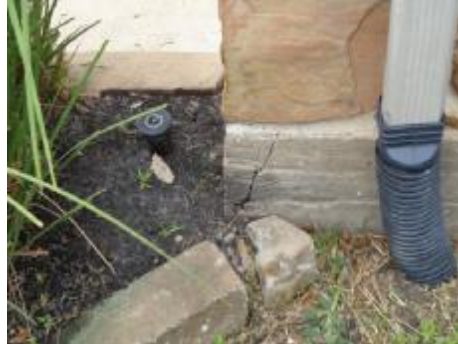
Popped corner front right
