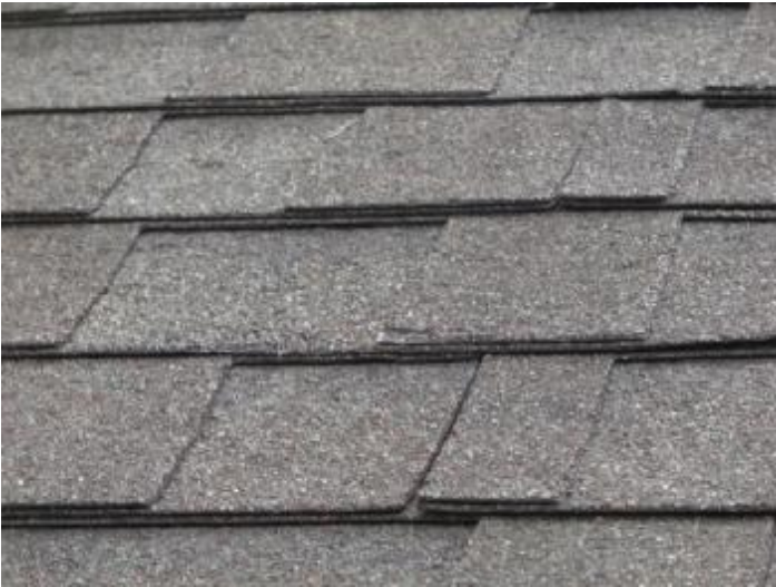
Granular/aggregate loss at roof surface
