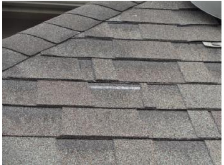
Granular/aggregate loss at roof surface - Damaged shingle
