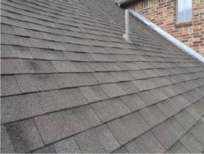
Granular/aggregate loss at roof surface
