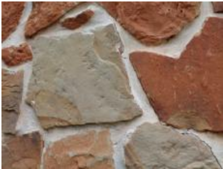
Crack in mortar
