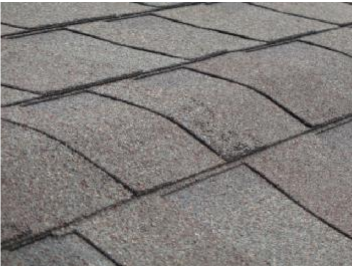
Granular/aggregate loss at roof surface
