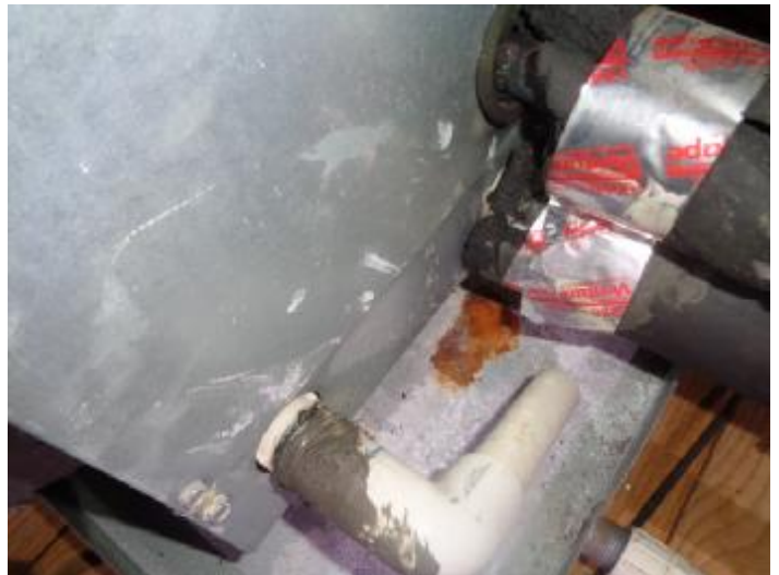
Rust in drain pan under furnace #1 in attic
