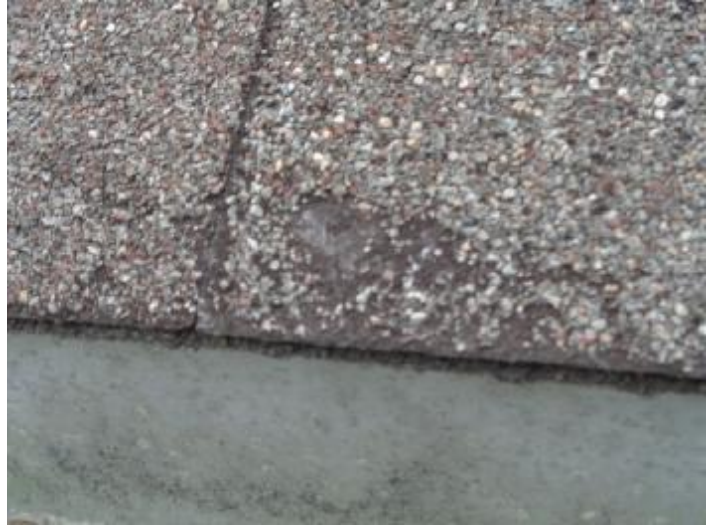
Granular/aggregate loss at roof surface
