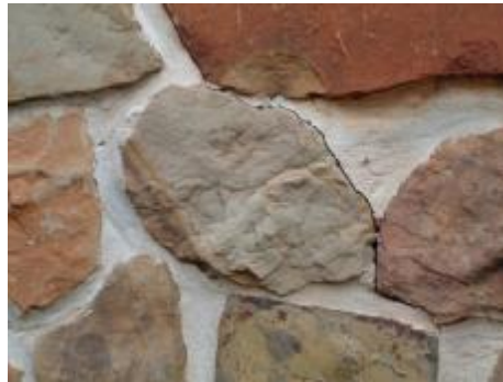
Crack in mortar
