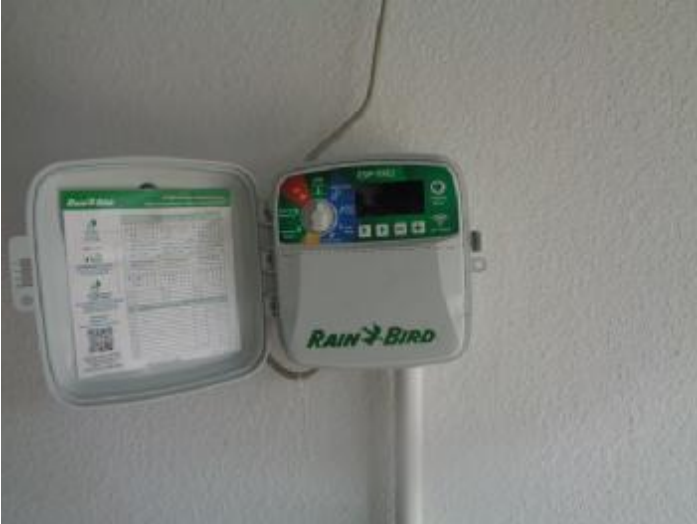
Sprinkler system control box
