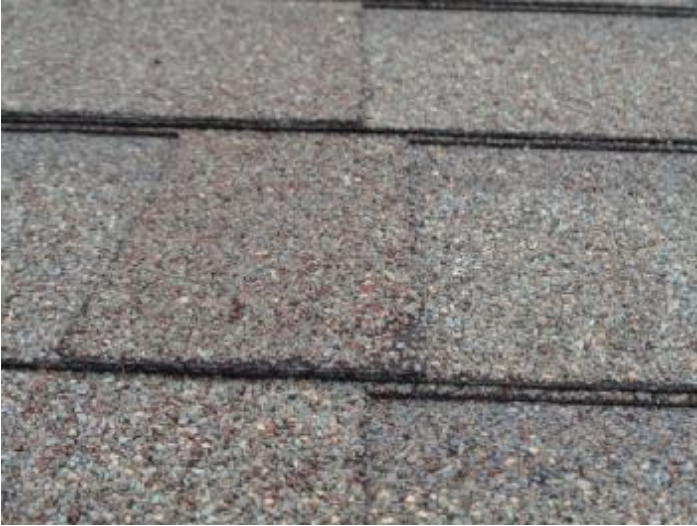
Granular/aggregate loss at roof surface
