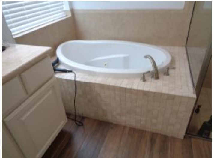
No visible access panel to whirlpool tub equipment
