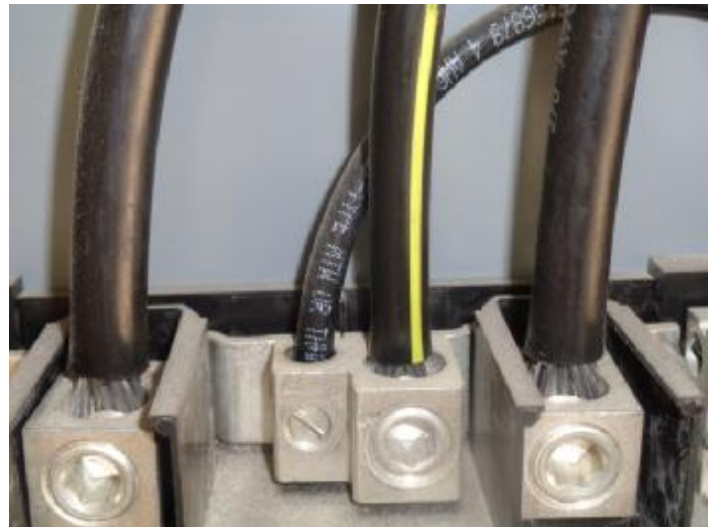
Aluminum service wire connections lack anti-oxidant paste in the electric panel
