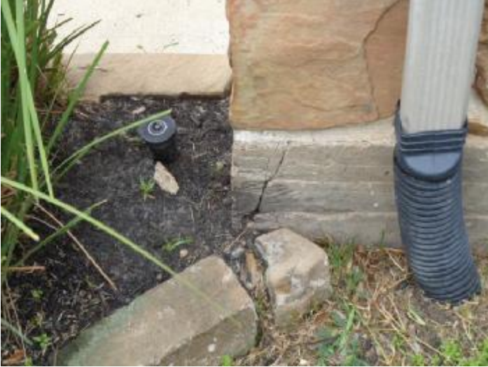
Front right corner of concrete slab foundation cracked
