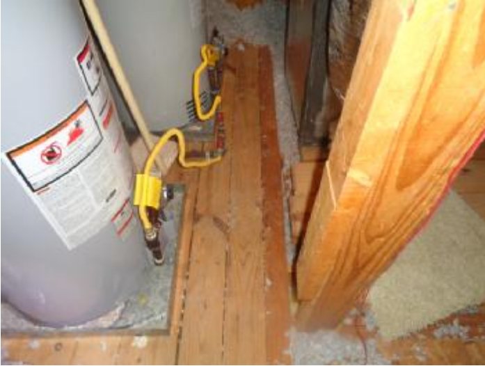
Service platform at water heaters is undersized
