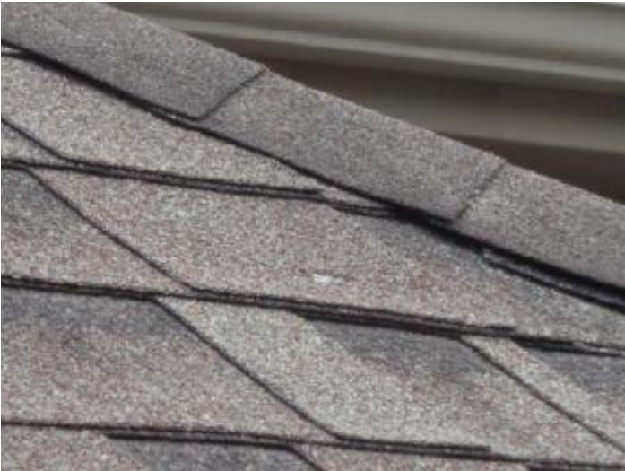
Granular/aggregate loss at roof surface - Damaged shingle
