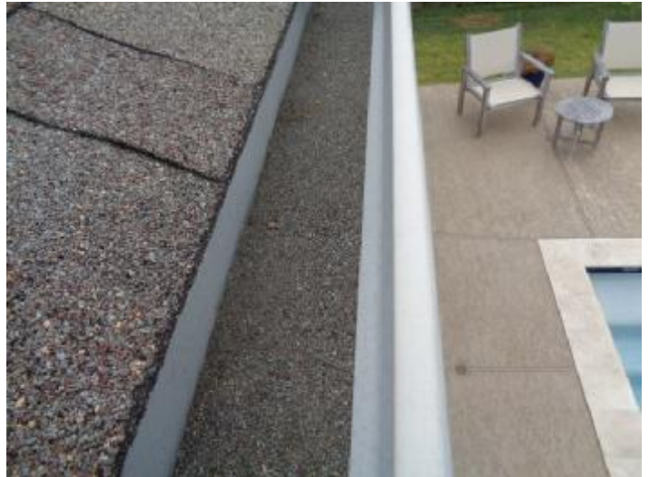
Gutter clogged with debris (Close up)
