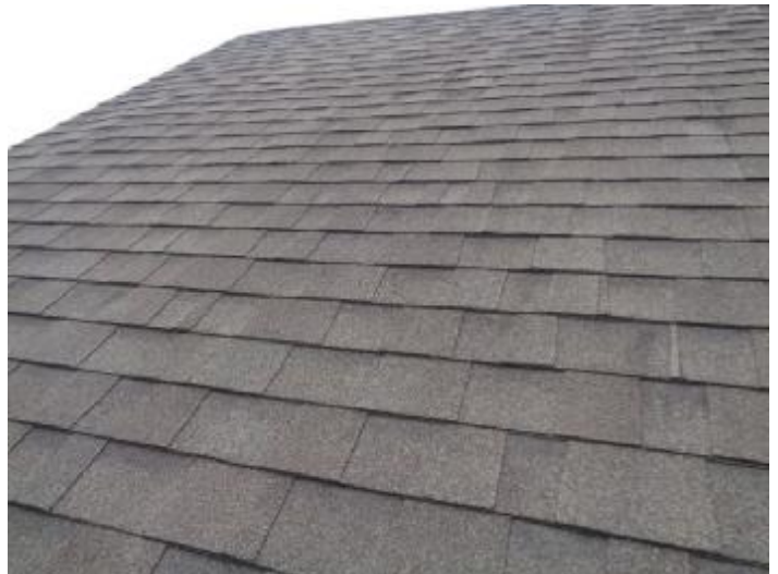
Granular/aggregate loss at roof surface
