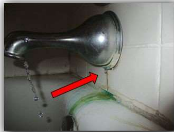
108. Observed tub spout leaking from back side when shower was tested. Recommend repair by a qualified plumber.
