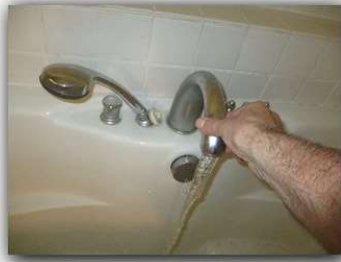
106. Faucets on tub are loose.
