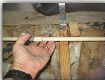
110. Water piping is not properly secured in attic areas. Recommend repair by a licensed plumber.
