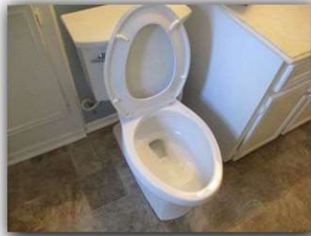
107. Toilets appeared loose. The toilet is fastened to the drain pipe and floor by bolts. The seal between the toilet and the drain pipe is usually a wax ring seal. If this seal is broken, the toilet will leak. The toilet(s) should be inspected for sealing and tightening.
