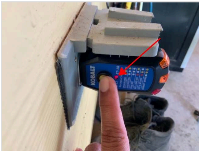
Tester showing receptacle not GFCI protected (exterior)
