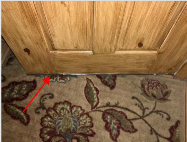
Torn/damaged weather stripping (front exterior door)
