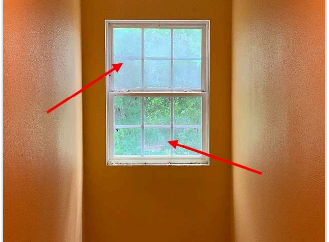
Lost seal (window above stairway)
