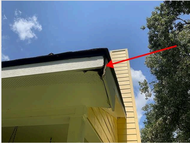
Wood/water damage (right corner-front porch)
