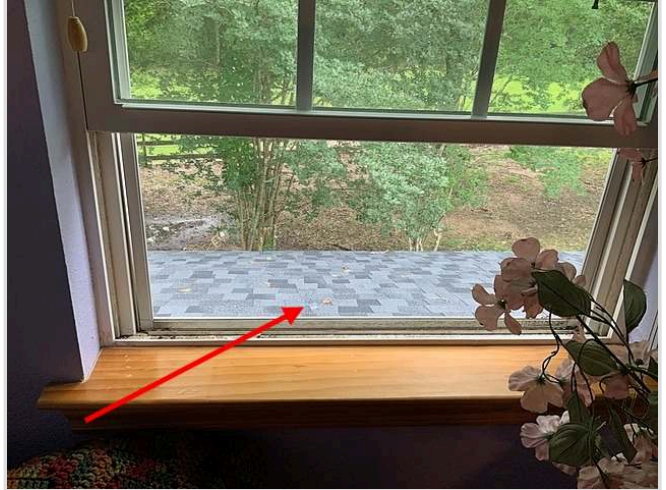
Damaged screen (left bedroom)
