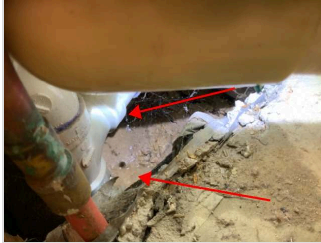
Leak point (master bathtub)
