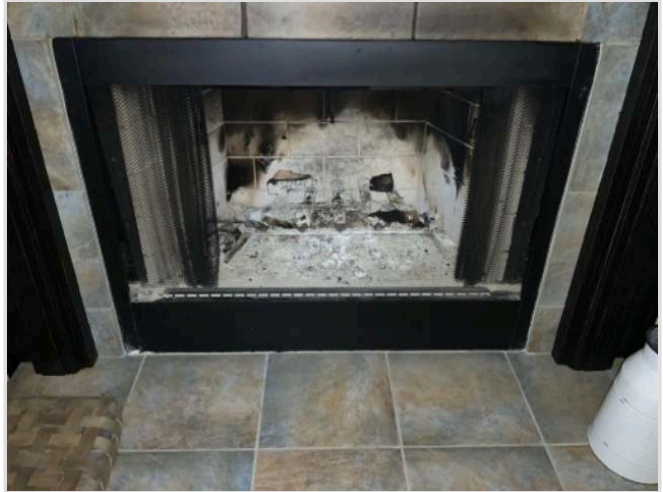
Needed to be cleaned
