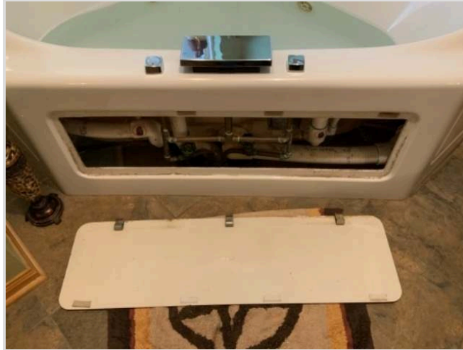
Cover removed for inspection
