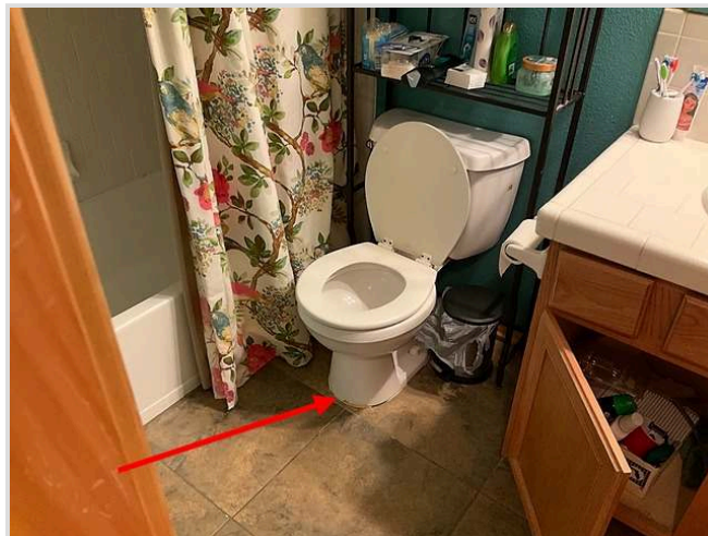
Loose at floor (upstairs bedroom)
