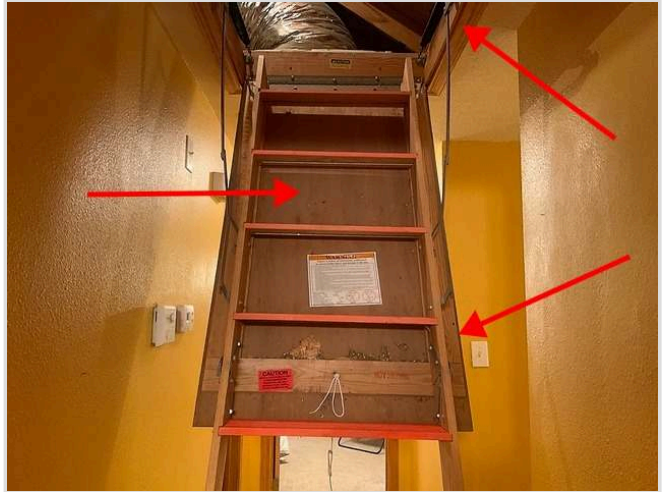
Not insulated/no weather stripping
