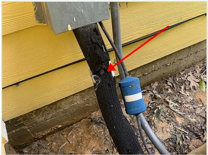
Needed additional insulation (outside unit)
