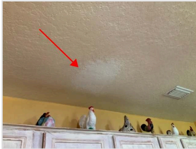
Signs of previous repairs (kitchen)
