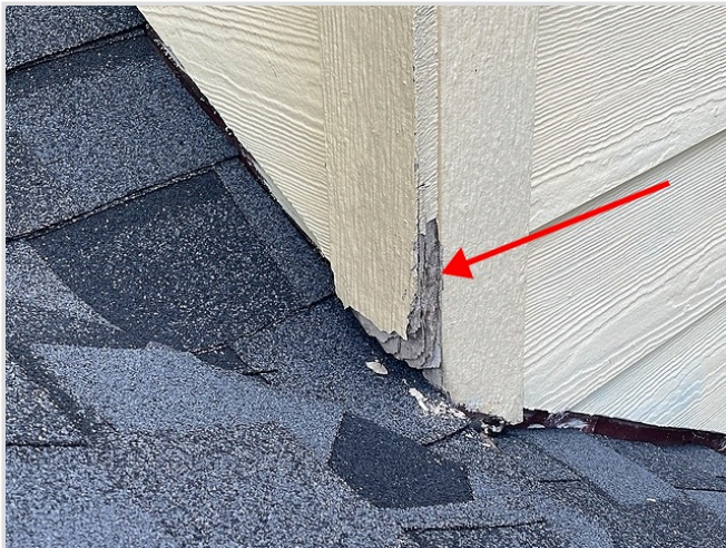
Trim damaged (chimney chase)
