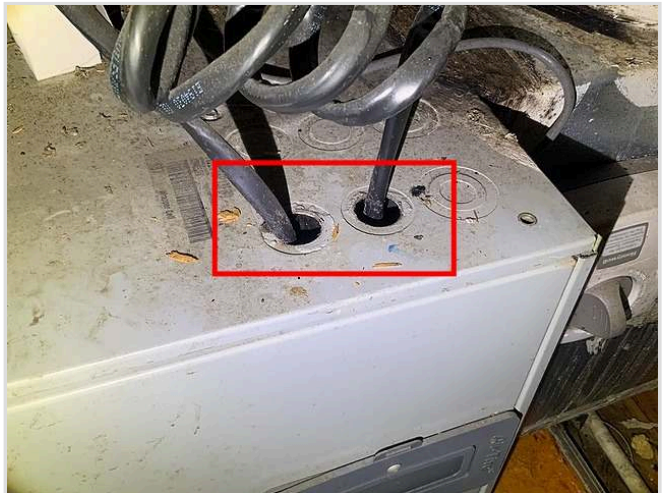
Wires not protected from abrasion
