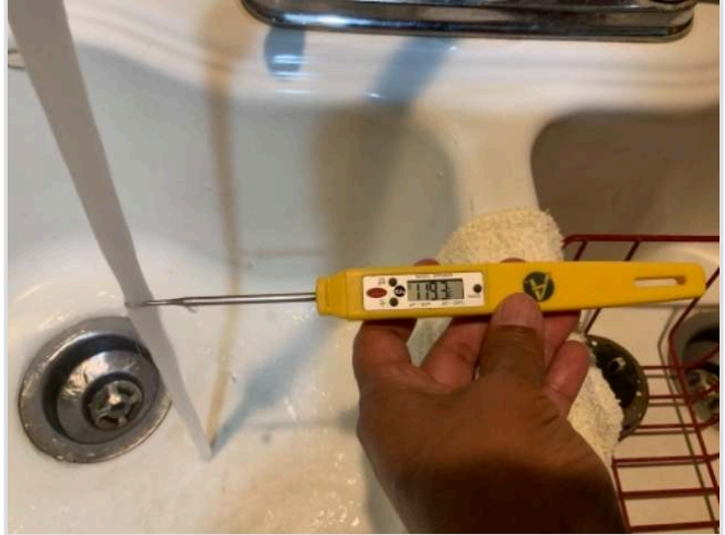
Measured water temperature at kitchen sink (119.3)
