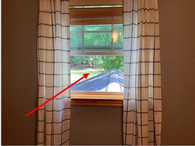
Missing screen (right bedroom)
