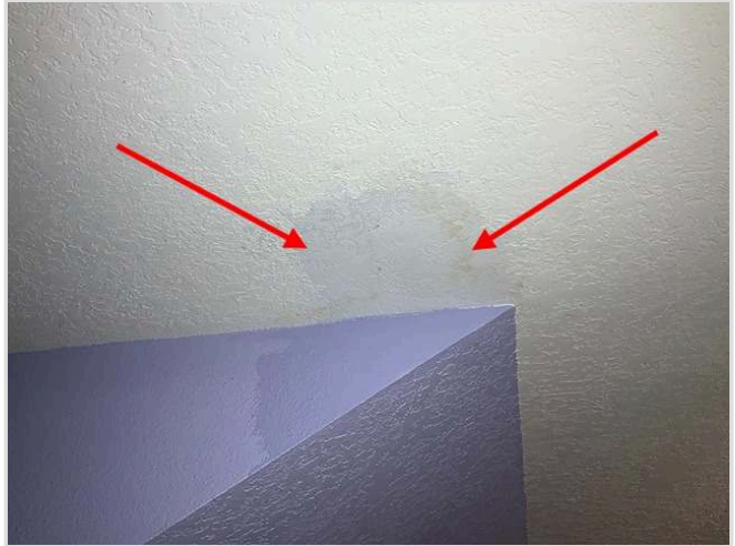
Signs of previous leaks (left bedroom)
