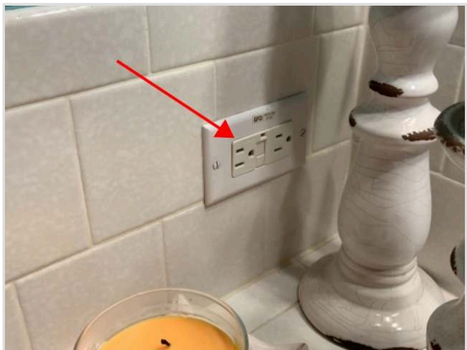
Loose (half bathroom)
