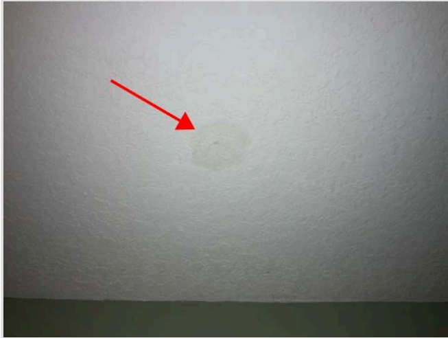
Signs of previous leaks (master bedroom)
