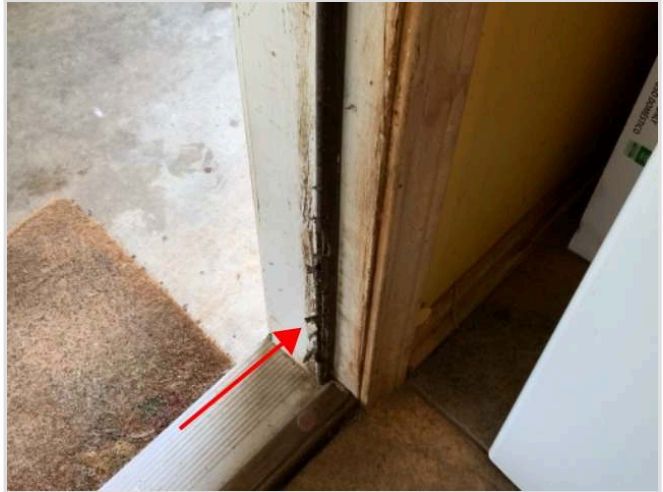
Torn/damaged weather stripping (exterior utility room door)
