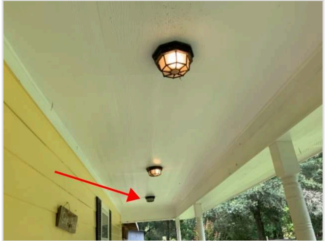
Would not illuminate (rear porch)
