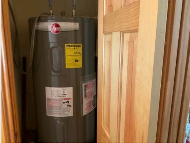
Water heater (utility room closet)
