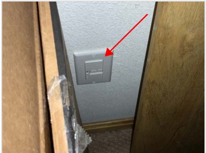
Hydro tub GFCI switch (front wall-master bathroom closet)
