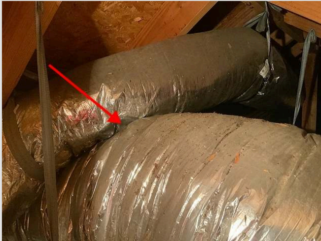
In contact with other duct
