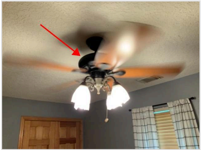
Not properly installed/loose (right bedroom)
