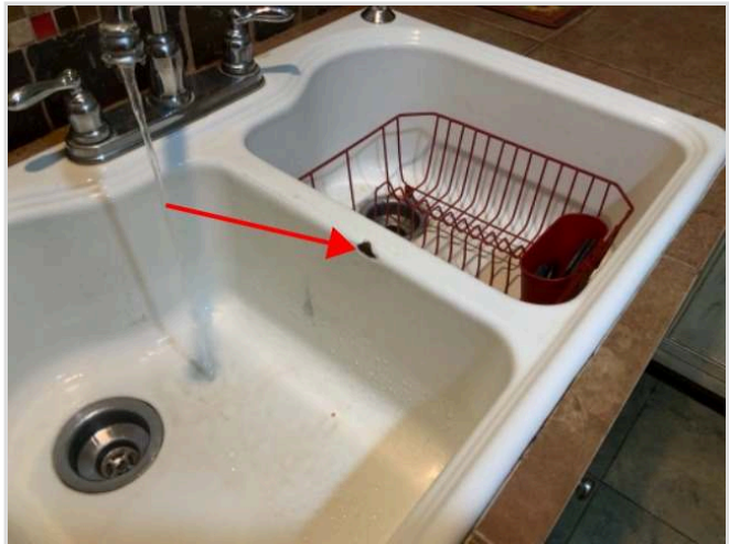
Chipped/damaged finish (kitchen sink)
