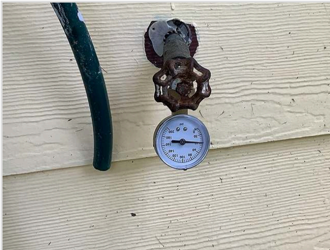
Static water pressure (30-40 psi)
