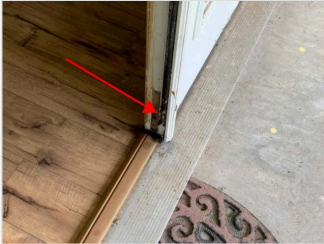
Torn/damaged weather stripping (rear exterior door)
