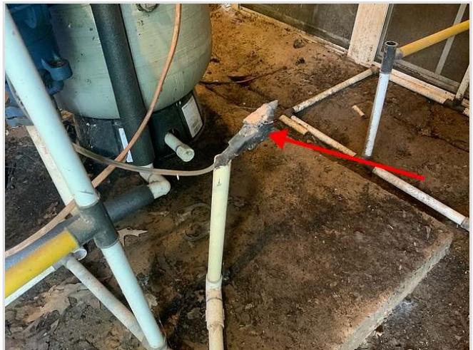
Wire connections not in a junction box
