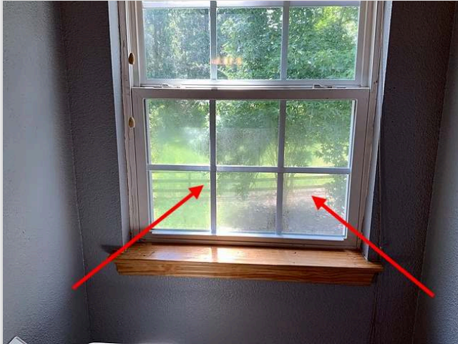
Lost seal (right wall-left bedroom)
