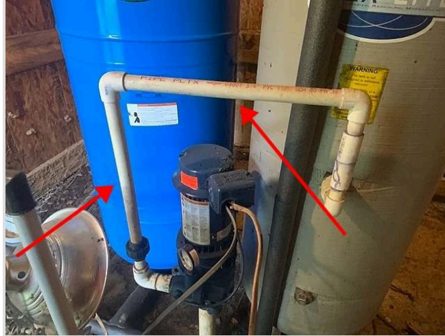
Supply pipe not insulated
