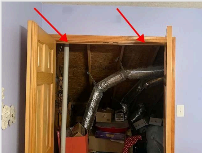
No weather stripping installed (left side access doors)
