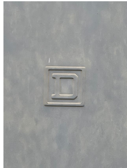
Electrical service panel brand name.
