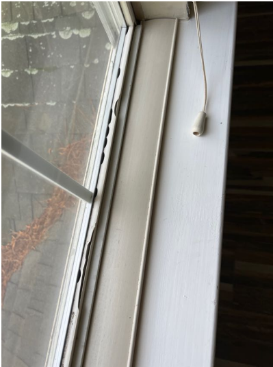
Several windows noted with damage
