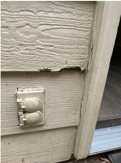
Damaged siding back side of house.
