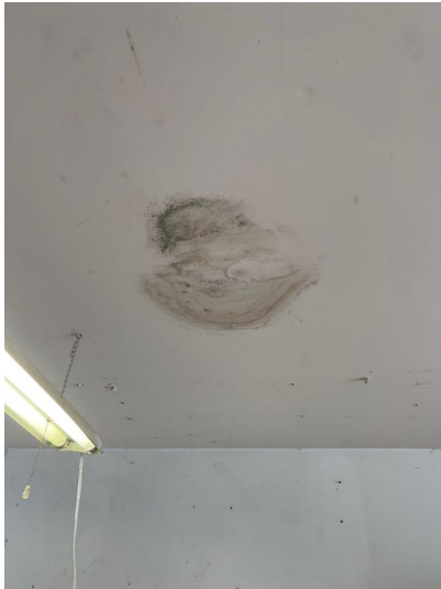
Moisture stain on ceiling.
