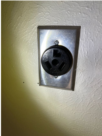
Female dryer outlet is the old three prong receptacle and should be exchanged for a four prong double grounded receptacle.
