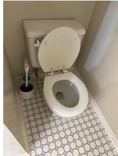
One or more commode(s) noted with constant water leaking into bowl from tank after flush cycle.
