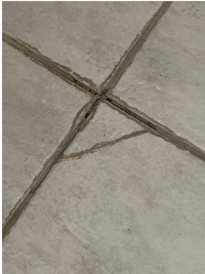
Damaged floor tile.
