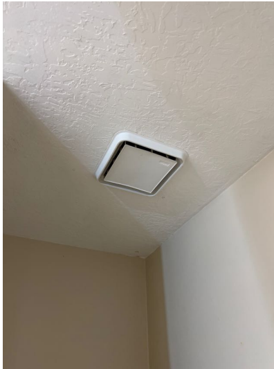
Bathroom exhaust fan noted with excessive noise.
