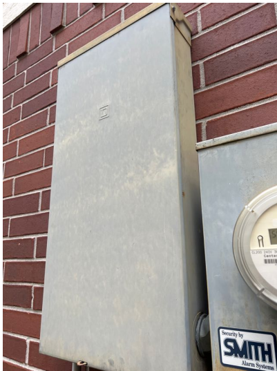
Picture of electrical service panel.
