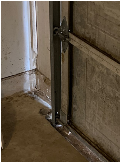
The garage door opener auto reverse sensors were missing at time of inspection.
