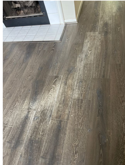
Damaged wood floor.
