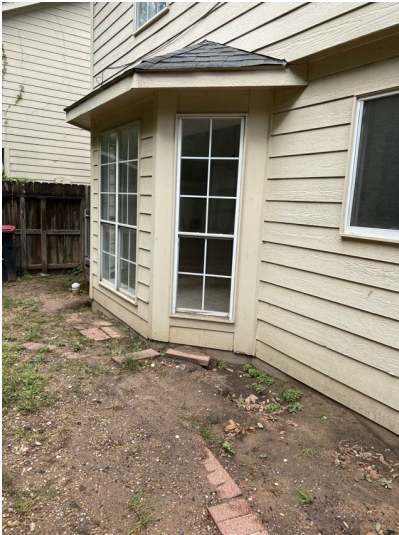
Windows missing screens.
