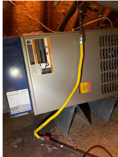
Gas Piping missing sediment trap.
