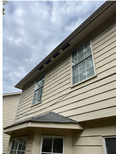
Windows missing screens.
