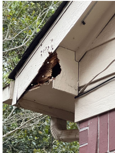
Damaged fascia board left side of house
