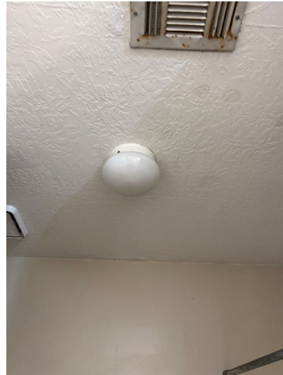
Light fixture not working
