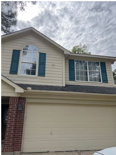
Windows missing screens.
