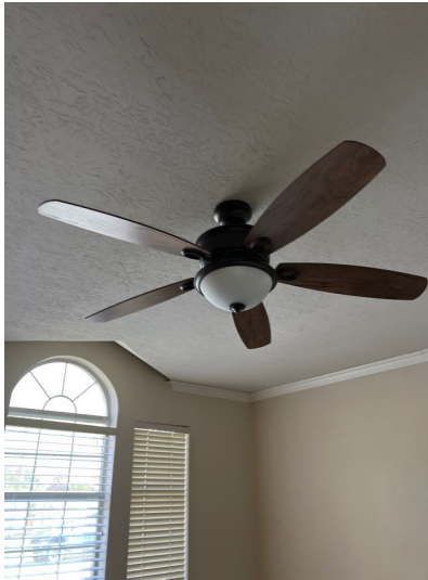
Ceiling fan not working
