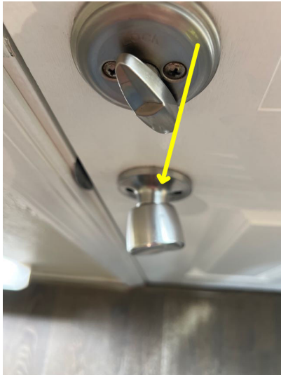
Back door noted with damaged door knob
