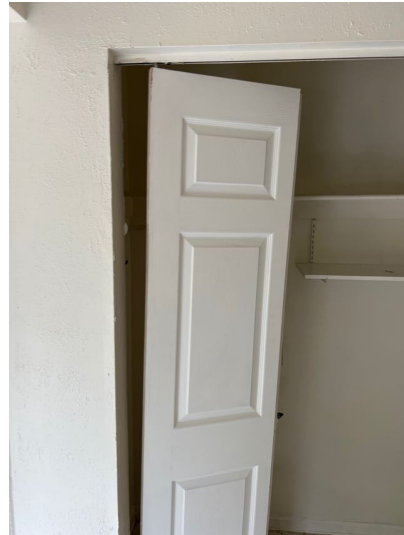
Utility room folding door not installed correctly
