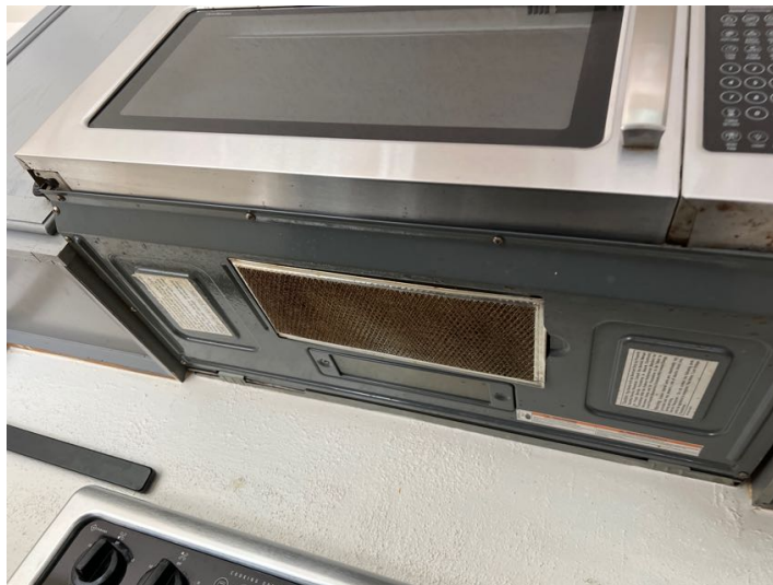
The vent hood light was not working at time of inspection.
