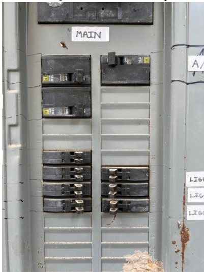
Picture of breakers
