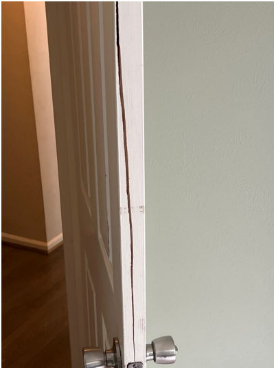
Bedroom door noted with damage
