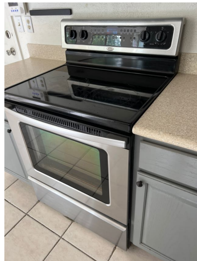
Anti-tip bracket is missing from range installation. All free-standing, slide-in ranges include an anti-tip device and is essential in the safe operation of the range. It provides protection when excess force or weight is applied to an open oven door
