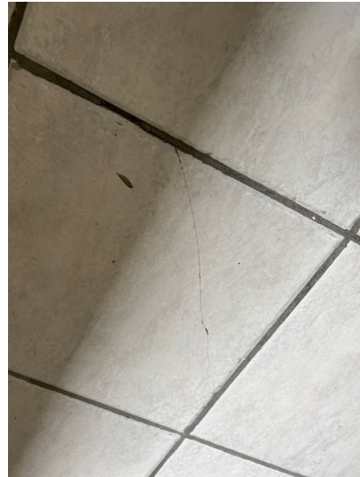
Damaged floor tile.
