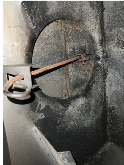
Fireplace damper missing damper clamp.
