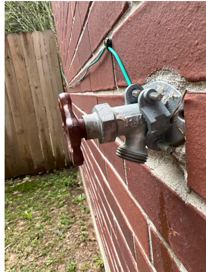
Hosebib missing anti-siphon device.
