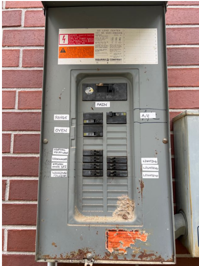
Picture of electrical service panel.
