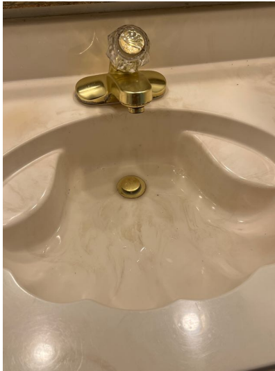
Downstairs half bathroom vanity noted with stopped drain
