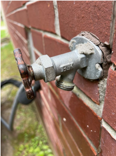
Hosebib missing anti-siphon device.
