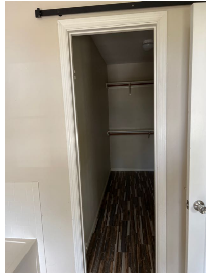
Master bedroom closet door missing
