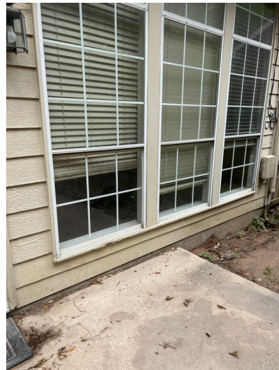
Windows missing screens.
