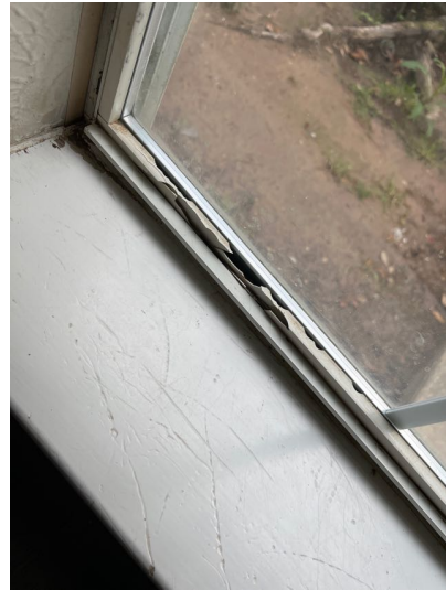
Several windows noted with damage
