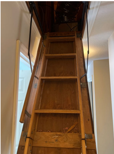
Attic access missing insulation.
