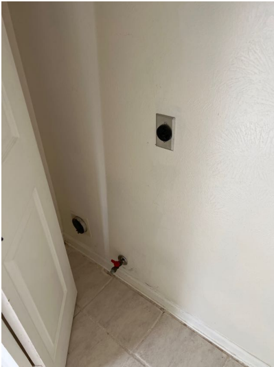
Electric and gas dryer connections present.
