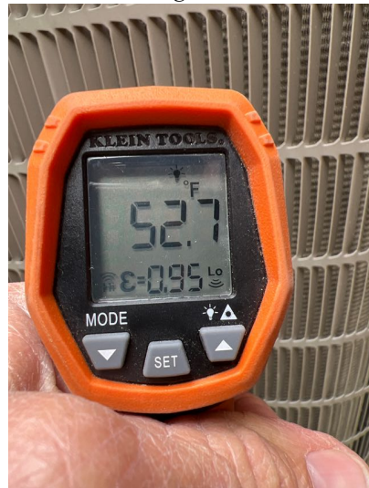
Temperature of AC condensing unit at time of inspection
