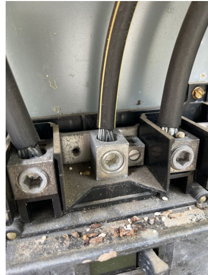
Aluminum service conductors missing anti-oxidant grease.
