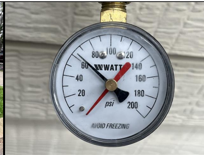
Static Water Pressure
