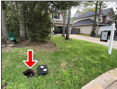
Water Meter Location
